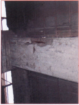
Spall with exposed rebar on column ES-5, SE
