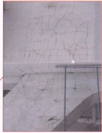
Map cracking in north exterior arch..
