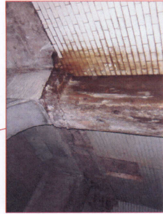
Heavy scaling, cracking and efflorescence, column ES-18, SE
