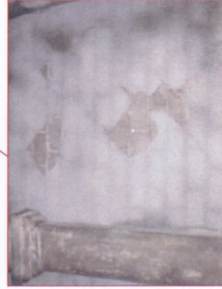
Block wall between arches has developed some cracks and mortar finish coat is spalling/peeling off.
