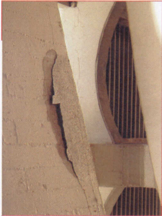
Delamination on north exterior arch..
