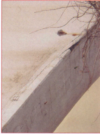
Cracking in north exterior arch..
