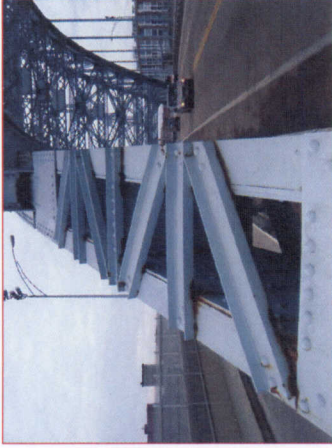
Pack rust beginning to reactivate in some locations between truss member components.
