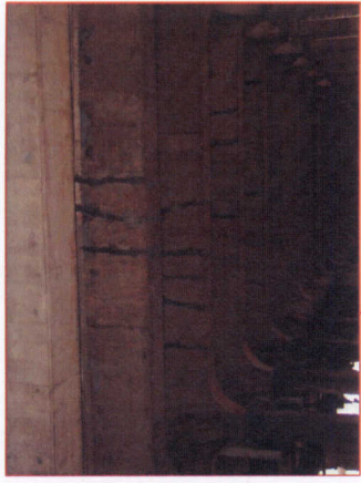
Most floorbeams in this span have been epoxy-injected at the flexure cracks. Repairs are performing well.
