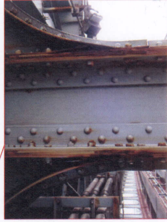
Typical reactivation of pack rust between plates of vertical (U1-L1 south truss shown here).
