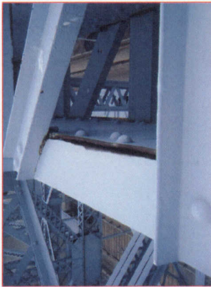
Pack rust beginning to reactivate in some locations between truss member components.
