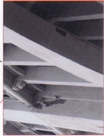
Spall due to crushing on north face, pier 5.
