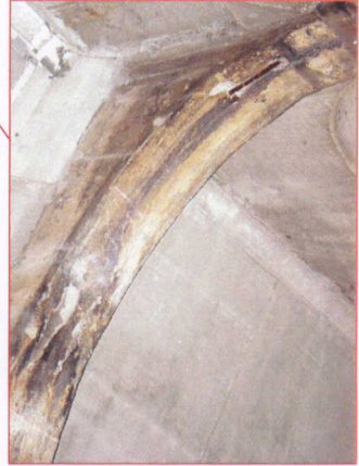
Spall with exposed rebar on underside of arch between 3-NI-10 and 3-NI-11..
