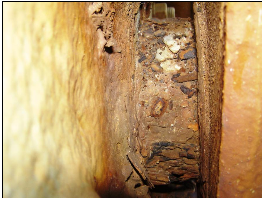
Photo 50: Corroded Pin Sleeve at L 4 North
