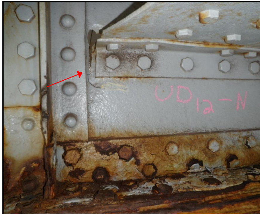
Photo 15: Hole in FB-U12-N Showing No Change from Previous Inspection
