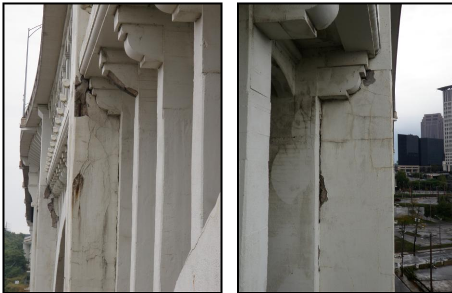
Photo 58 & 59: Typical Spalled and Map Cracked Concrete at the Tops of the Towers
