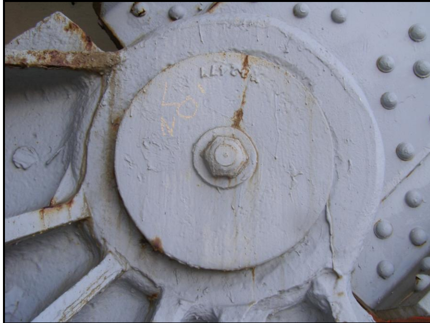
Photo 44: Cracked South Retaining Washer at L 0 - N
