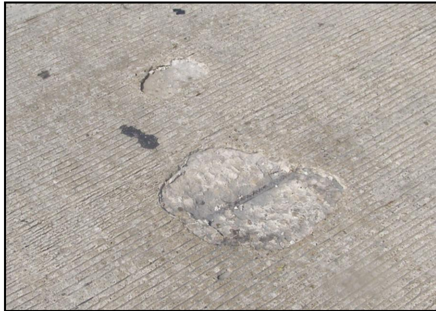
Photo 3: Wearing Surface Popout with Exposed Reinforcing Steel
