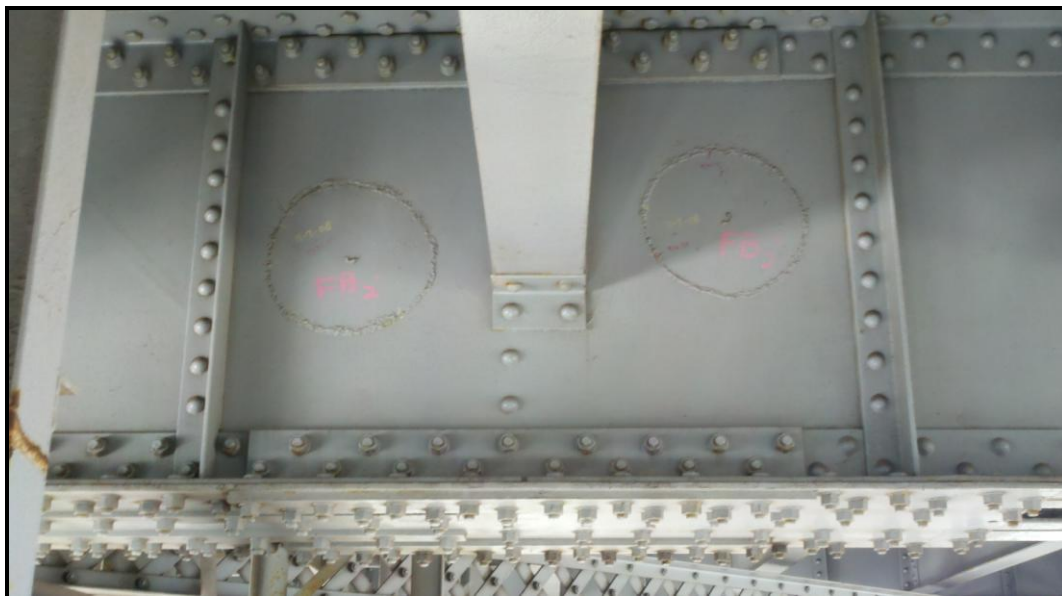
Photo 19: Showing Location of Circular Welds in the South End of FB-U2'
