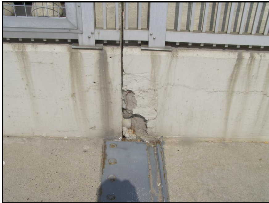
Photo 7: Fractured Concrete Parapet at Joint 9
