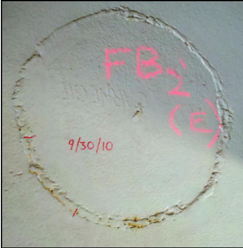
Photo 20: Showing the New Cracked Weld in the Southern Circular Weld in FB-U2'
