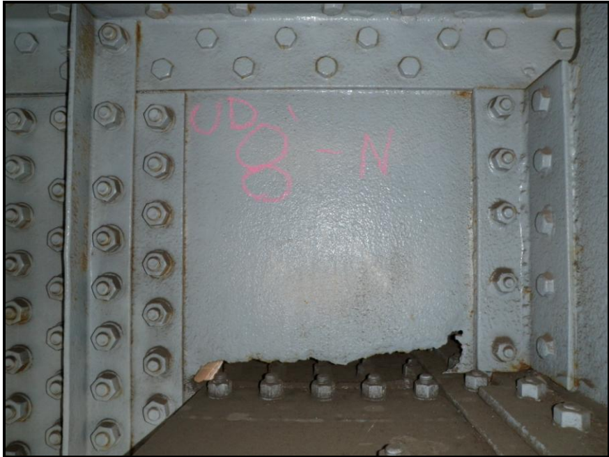
Photo 17: Hole in FB-U8'-N Showing No Change from Previous Inspection
