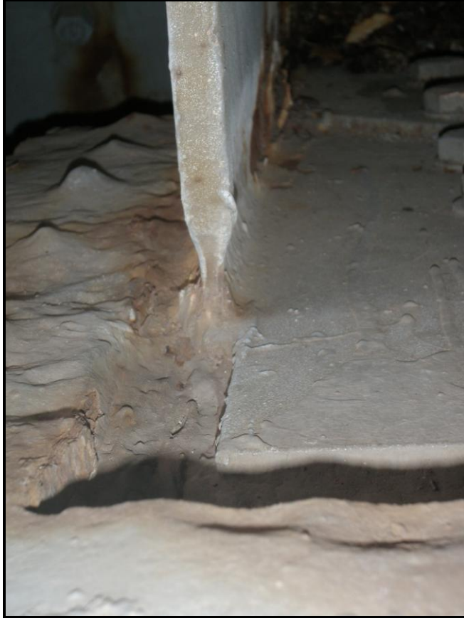
Photo 32: Typical Groove Pitting along the Gusset Plates at the Top of the Lower Chord
