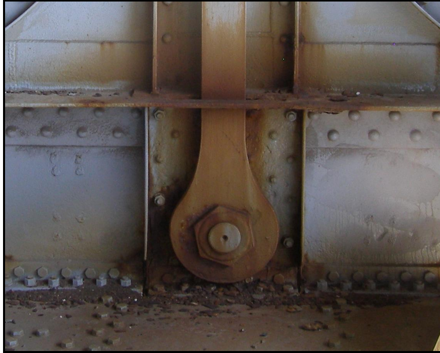
Photo 51: Corroded Eye-Bar at L_4 -S. No Cracks Visible.
