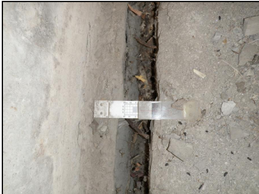
Photo 54: Crack Monitor Installed at the Interface between the Top of the Lower Deck and Tower B
