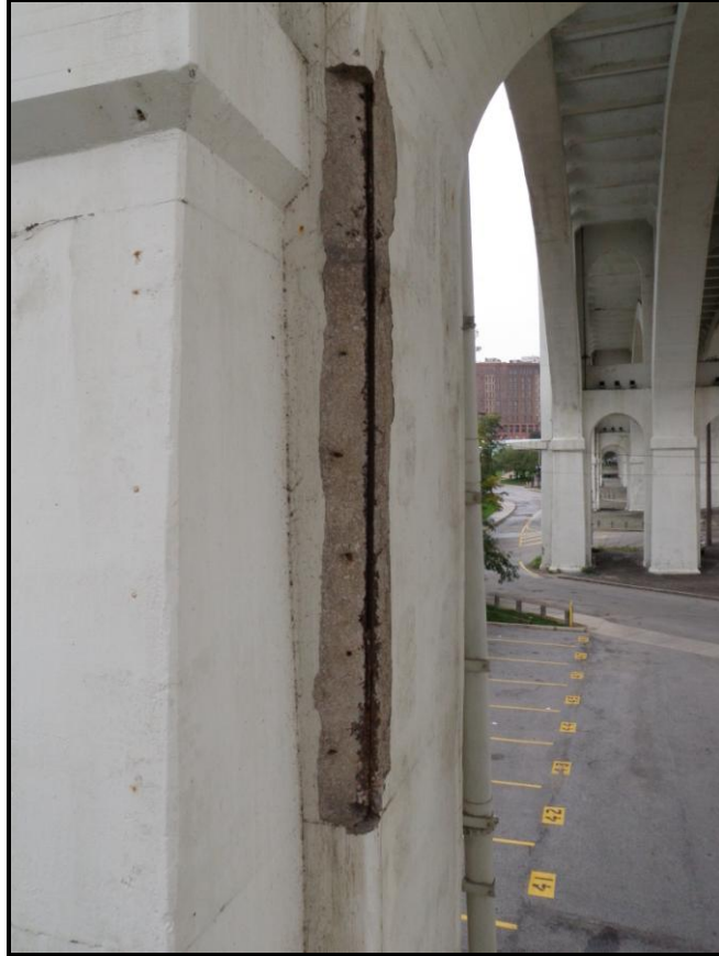
Photo 60: Typical Large Corner Spall on Tower 5
