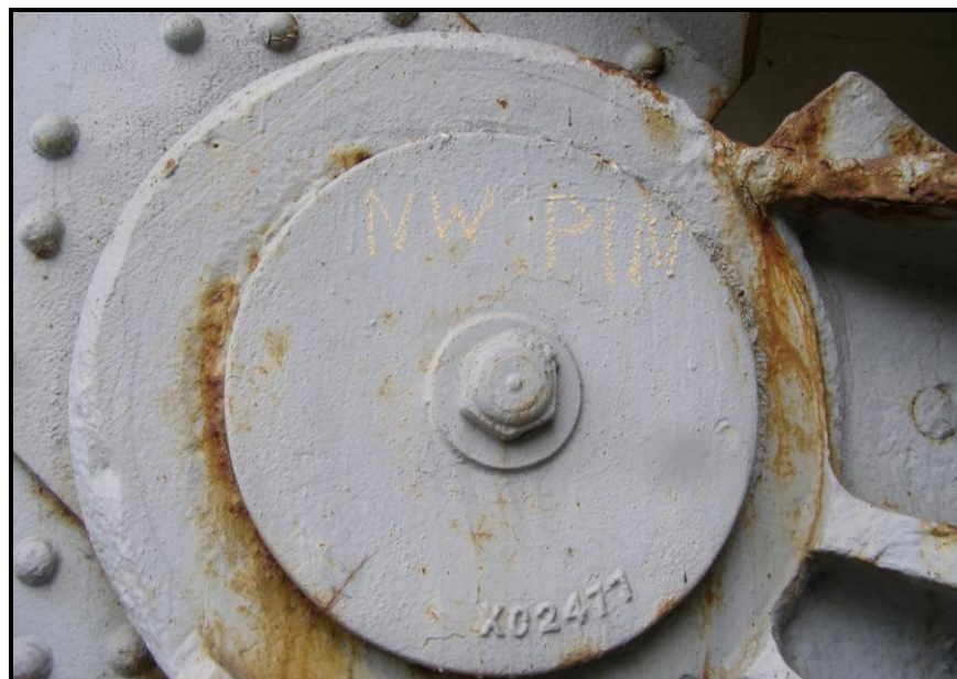
Photo 45: Cracked South Retaining Washer at L 0 - N
