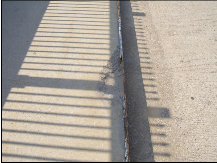
Photo 5: Typical Sidewalk Spall
