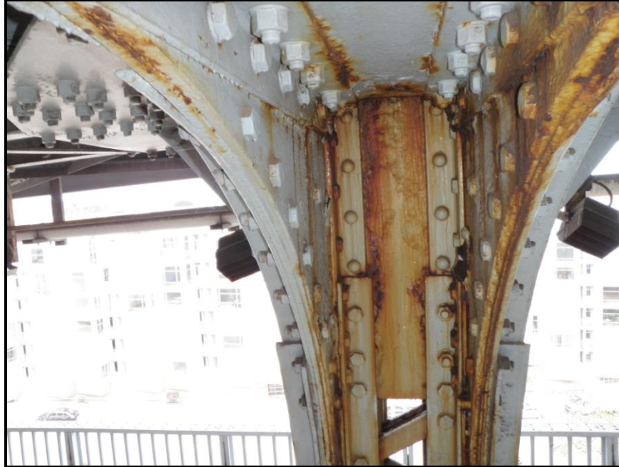
Photo 27: Typical Corrosion on Vertical Member Immediately Below the Upper Deck Pass-Through
