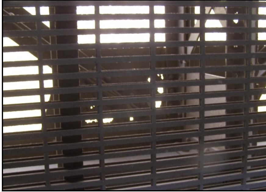
Photo 33: Through Holes in the Gusset Connecting the Lower Lateral Bracing with the Northern Most Exterior Stringer as seen through the Fiberglass Deck Panel
