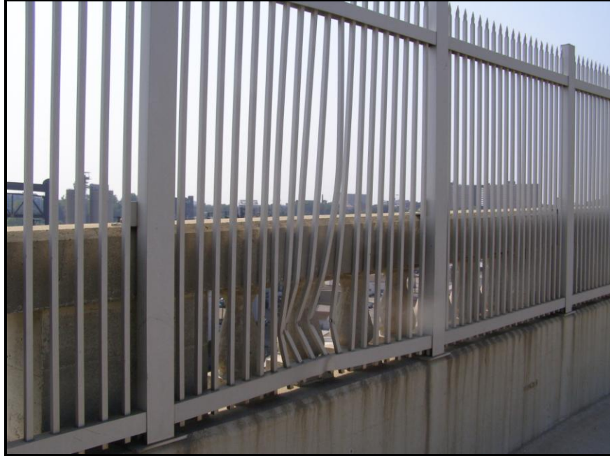
Photo 8: Damaged Vandal Protection Fence
