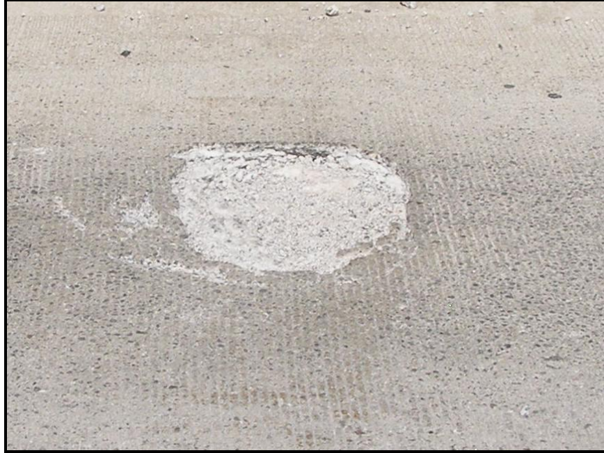
Photo 4: Large Spall at Panel Point 7
