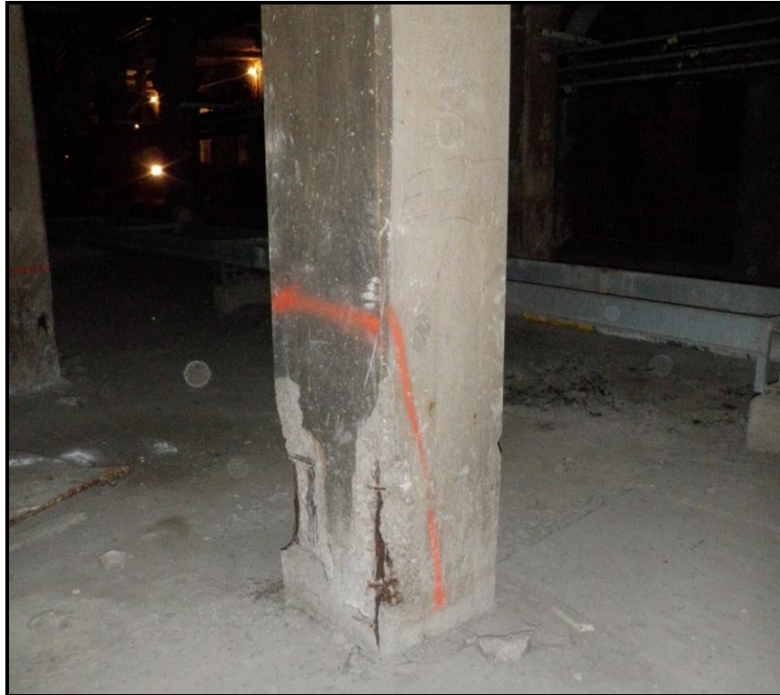
Photo 40: Typical Spalled Column Base
