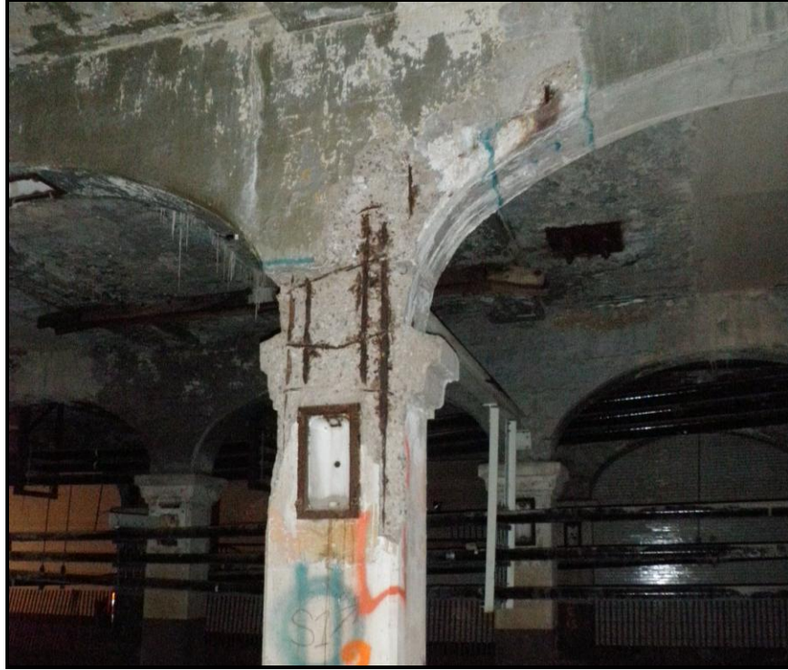
Photo 41: Typical Spalled Column Capital
