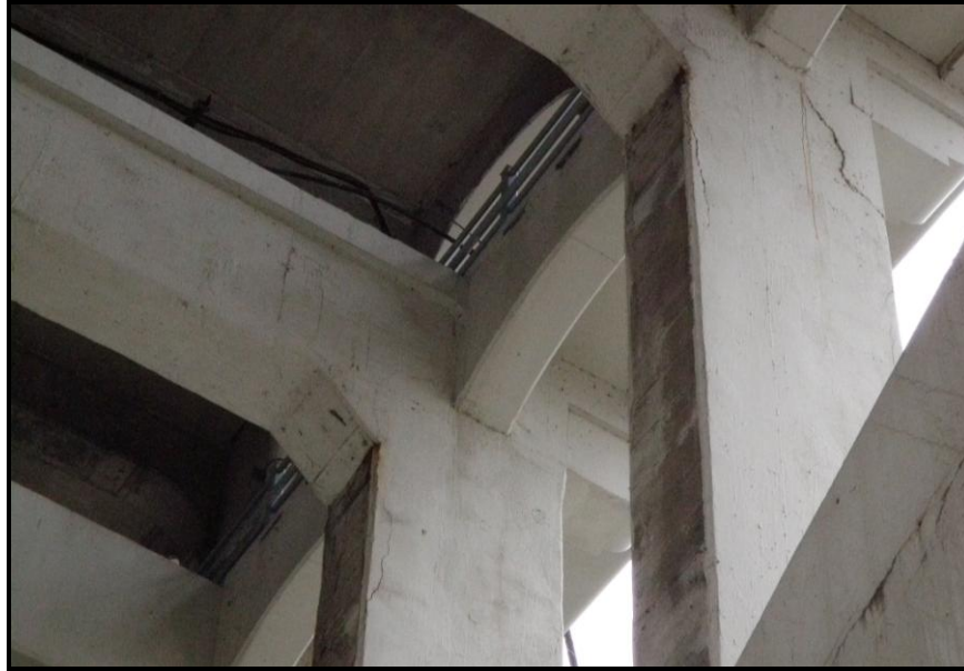
Photo 42: Typical Arch Column Cracks
