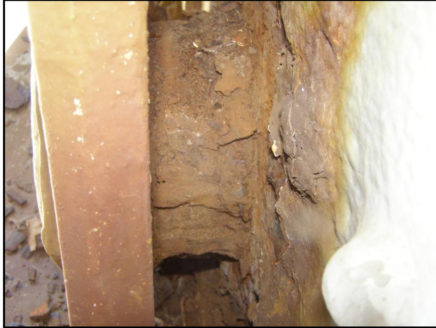
Photo 49: Corroded Pin Sleeve at L 4 North
