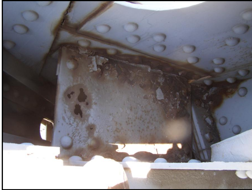
Photo 34: Typical Corrosion and Through-Hole in a Batten Plate inside of the Portals
