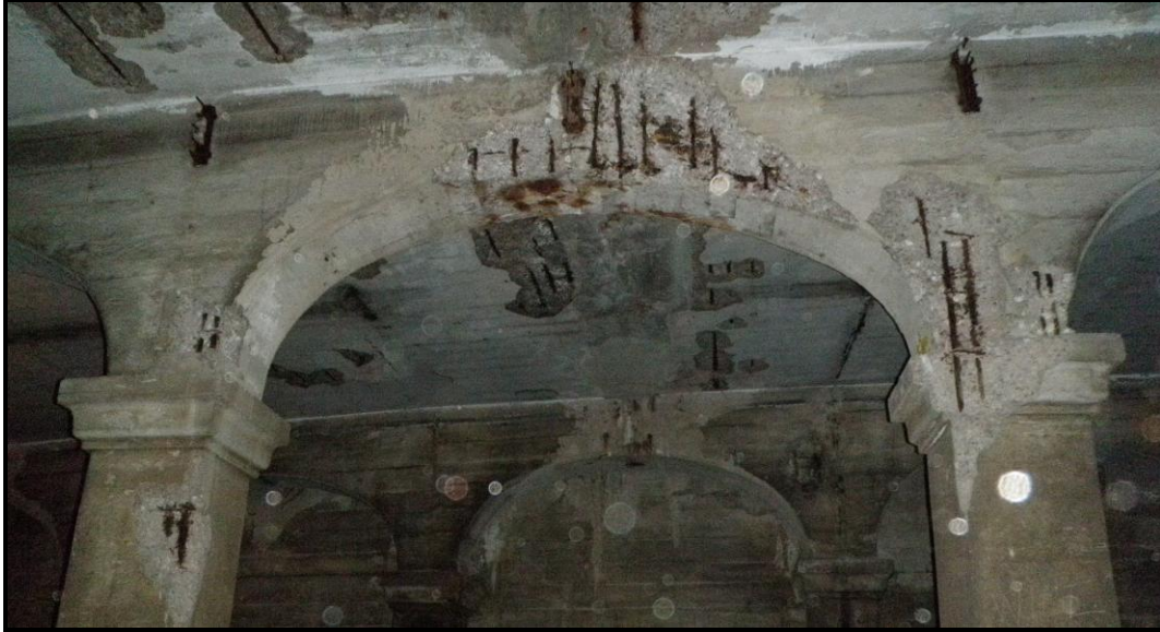
Photo 35: Typical Spalled Jack Arch in the West Tunnel
