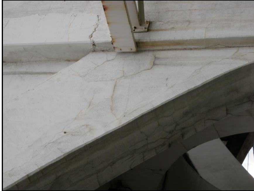
Photo 38: Typical Map Cracking in the Spandrel Arch Rib Concrete
