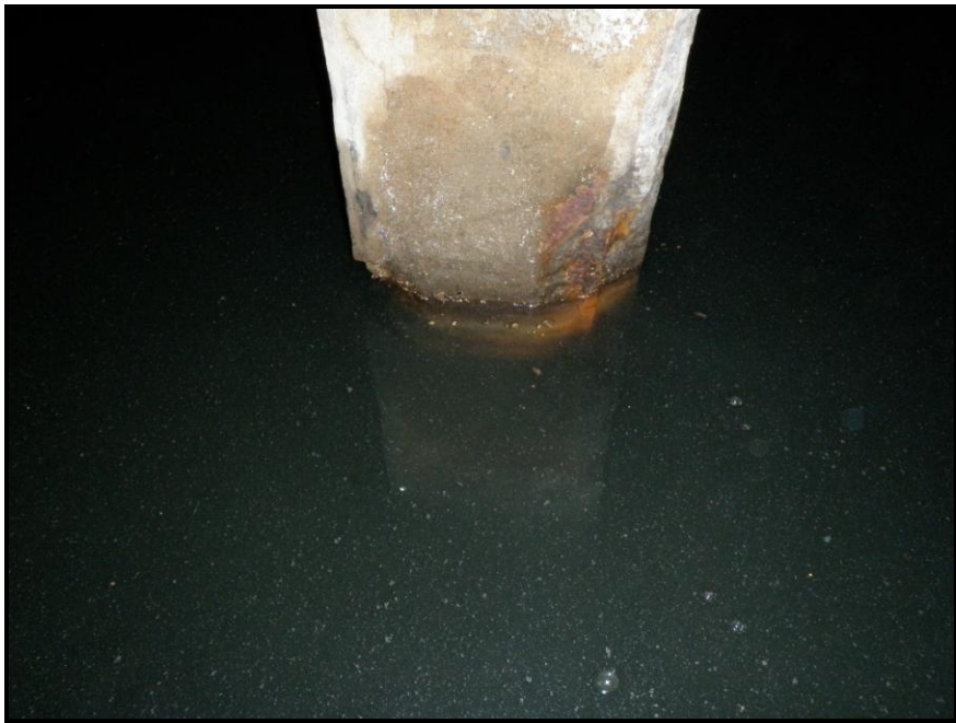
Photo 10: Standing Water in the East Tunnel
