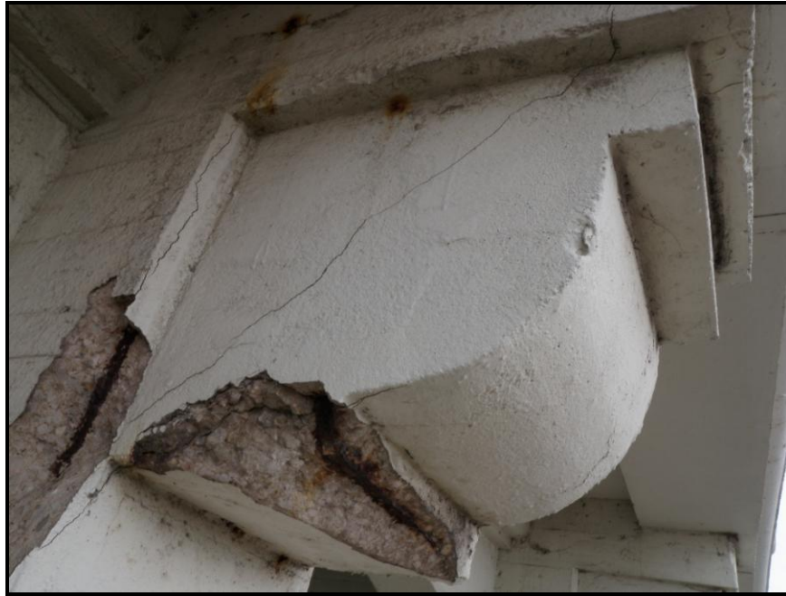
Photo 25: Corbel 12, Span 6 Completely Delaminated and Loose
