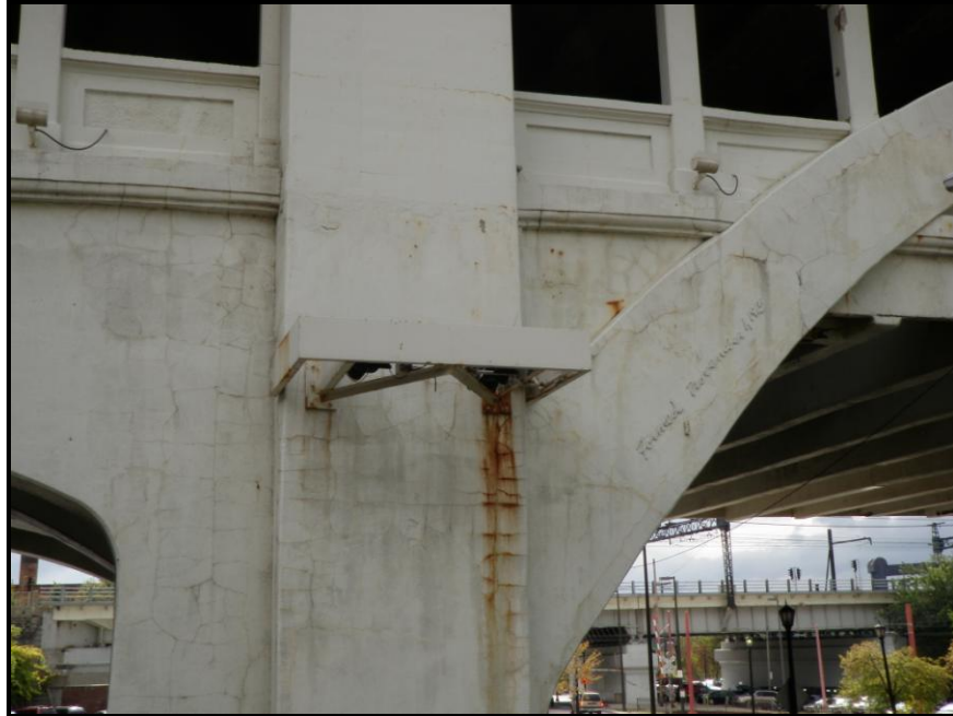
Photo 57: Typical Map Cracked Concrete at the Base of the Towers
