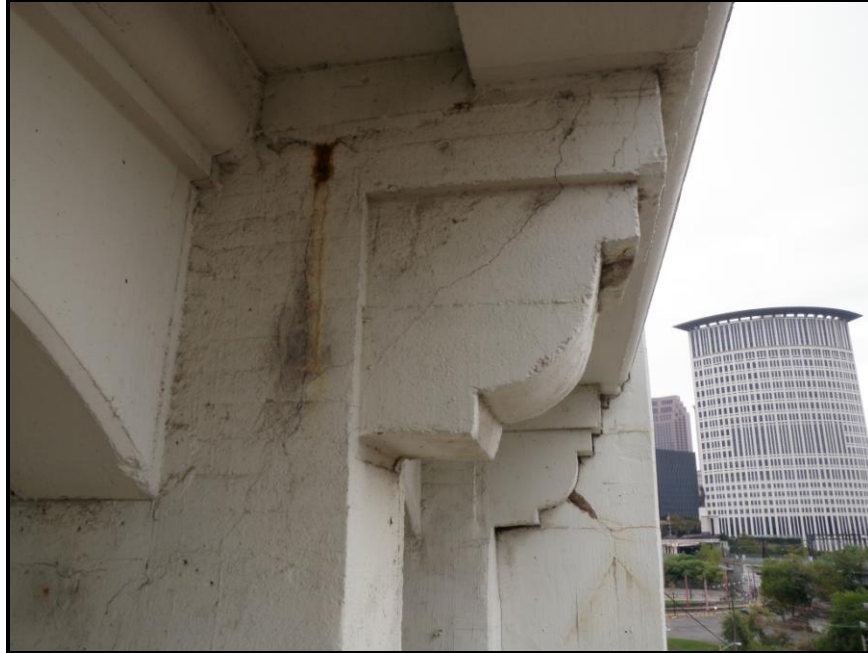
Photo 26: Corbel 14, Span 6 Completely Delaminated and Loose
