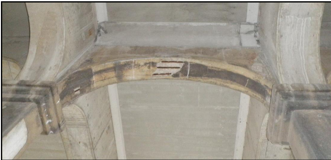
Photo 36: Typical jack arch spall in Spans 1A, 1B, 1-3 and 4-13
