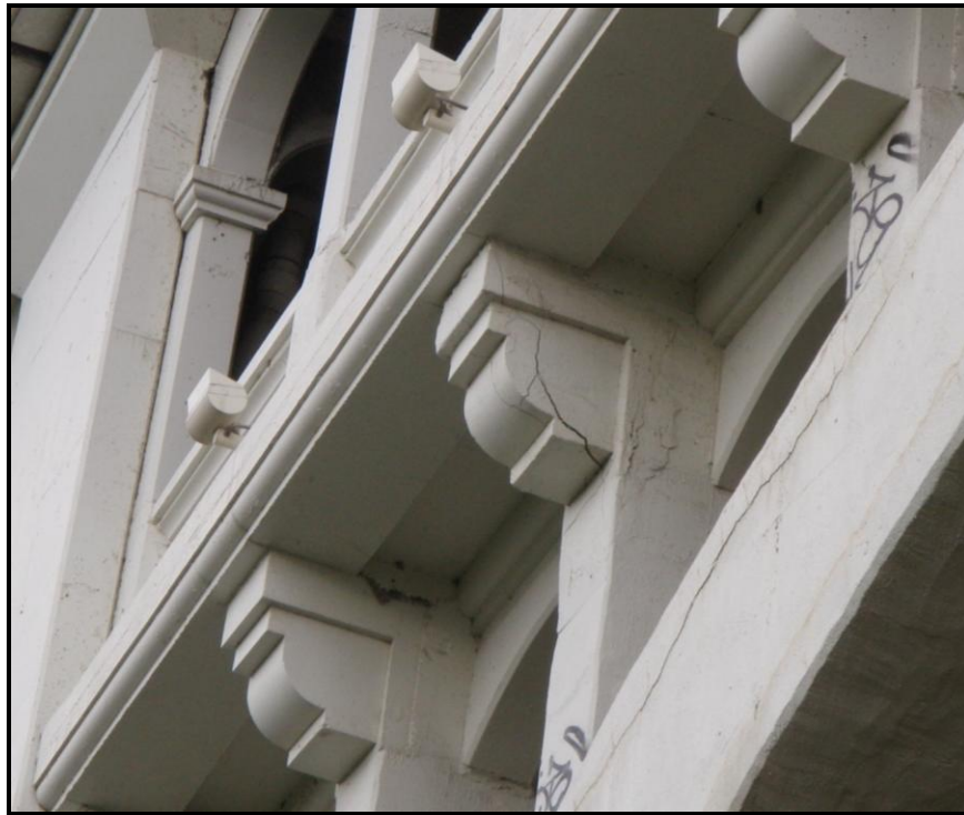
Photo 24: Corbel 4, Span 2 Cracked and Loose
