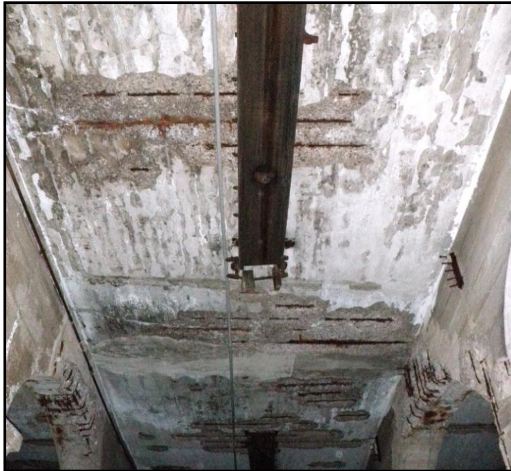
Photo 2: Typical Large Spalled Areas with Exposed Reinforcing Steel in the West Approach Tunnel
