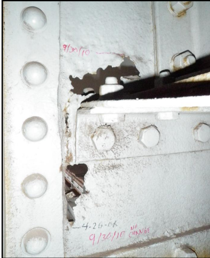
Photo 18: Hole in FB-U6'-N Showing No Change from Previous Inspection
