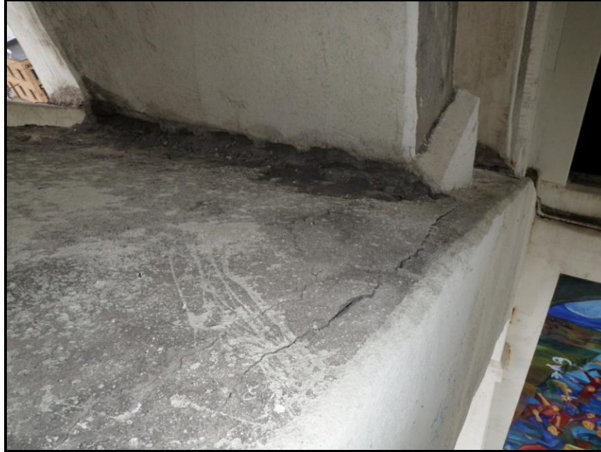
Photo 37: Typical Corner Crack in Spandrel Arch Rib
