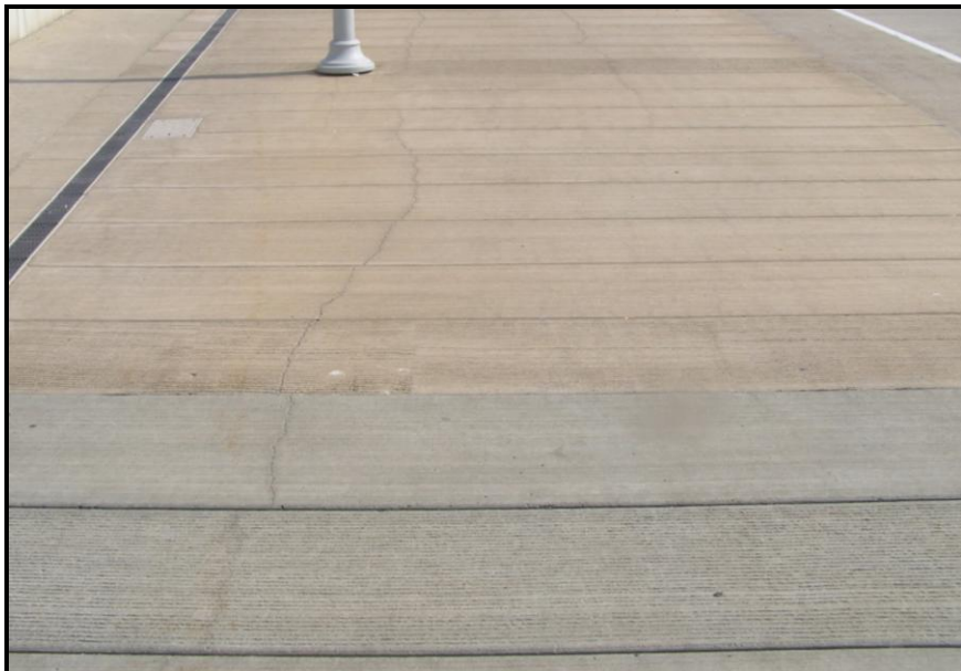
Photo 6: Typical Longitudinal Cracks in the Sidewalk
