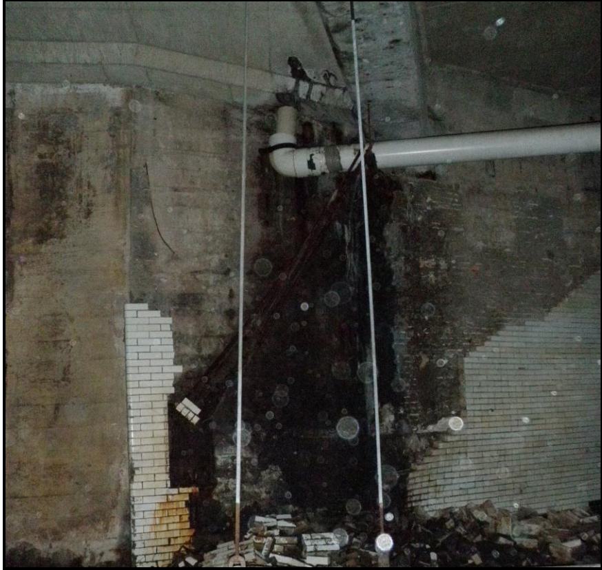
Photo 9: Broken and Leaking Drainpipe near the East Abutment
