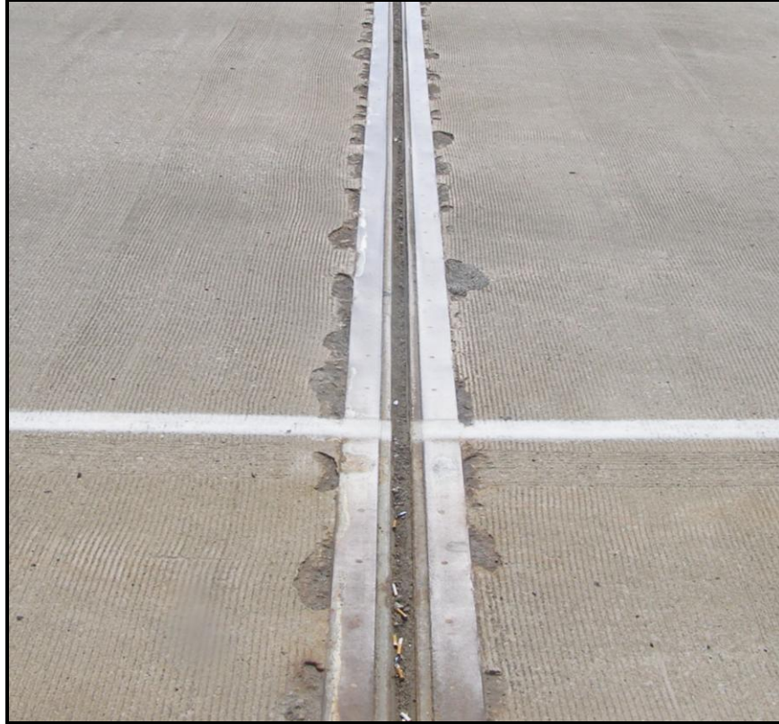
Photo 11: Typical Spalls on Both Sides of the Joint Armor
