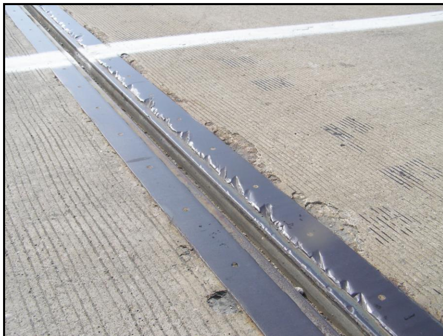
Photo 12: Typical Plow Damage to Joint Armor
