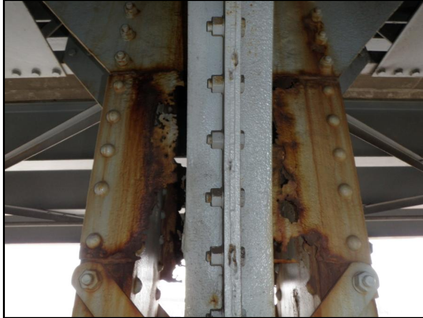
Photo 29: Through Holes in Cover Plate of L 0 -S Vertical
