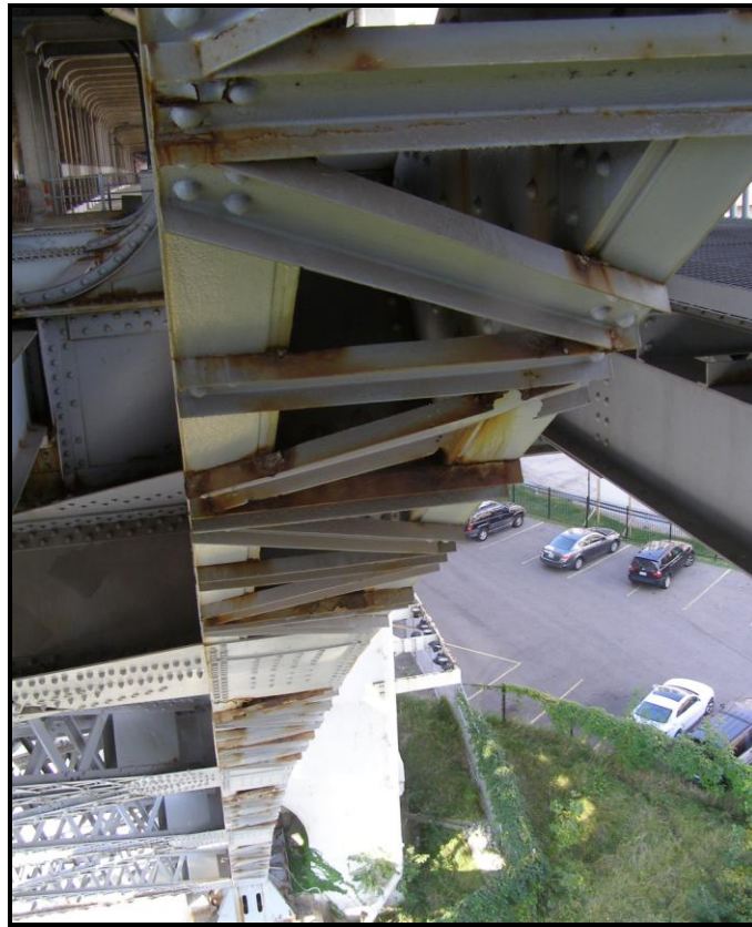
Photo 31: Corrosion and Holes to the Bottom of the Lower Chord from Panel Point L 0 -L 4
