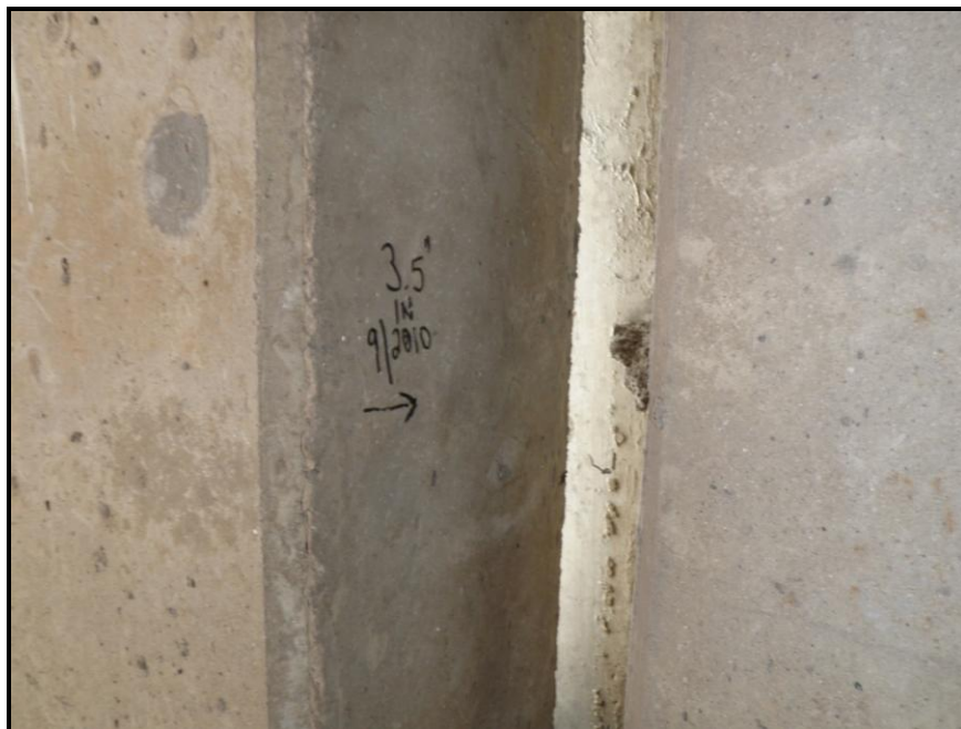
Photo 56: Gap Measurement between the East Edge of Tower B Showing the Amount of Rotation Away from the Surrounding Structure
