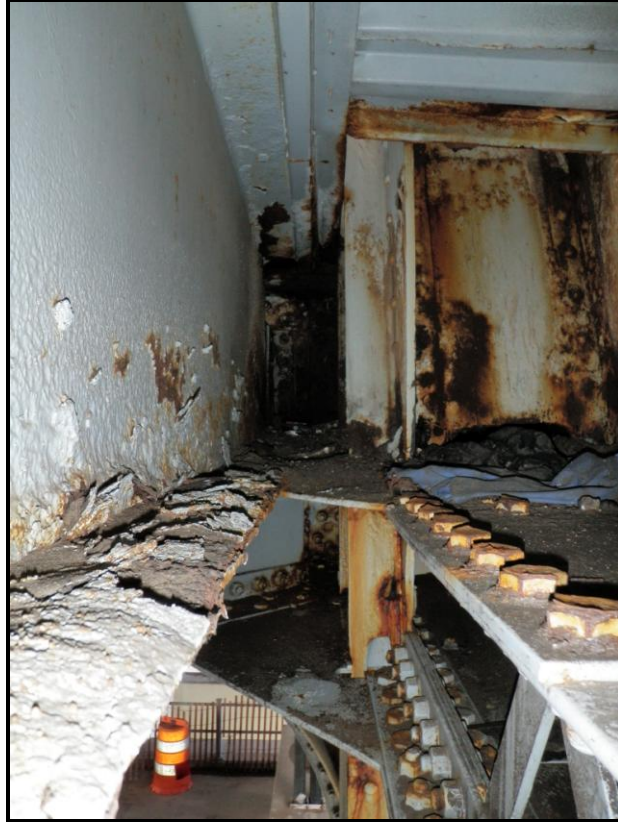
Photo 14: Typical Corroded Bottom Flange of Upper Deck Stringer
