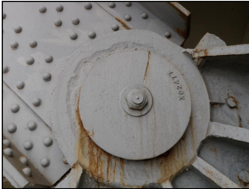
Photo 48: Cracked South Washer at L 0 - S
