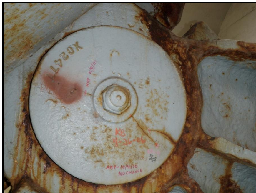
Photo 47: Cracked North Retaining Washer at L 0 - S. Note the New Crack on the Other Side of the Center Bolt.
