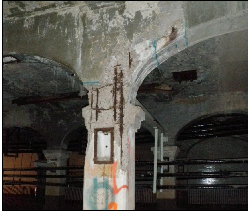
Photo 41: Typical Spalled Column Capital
