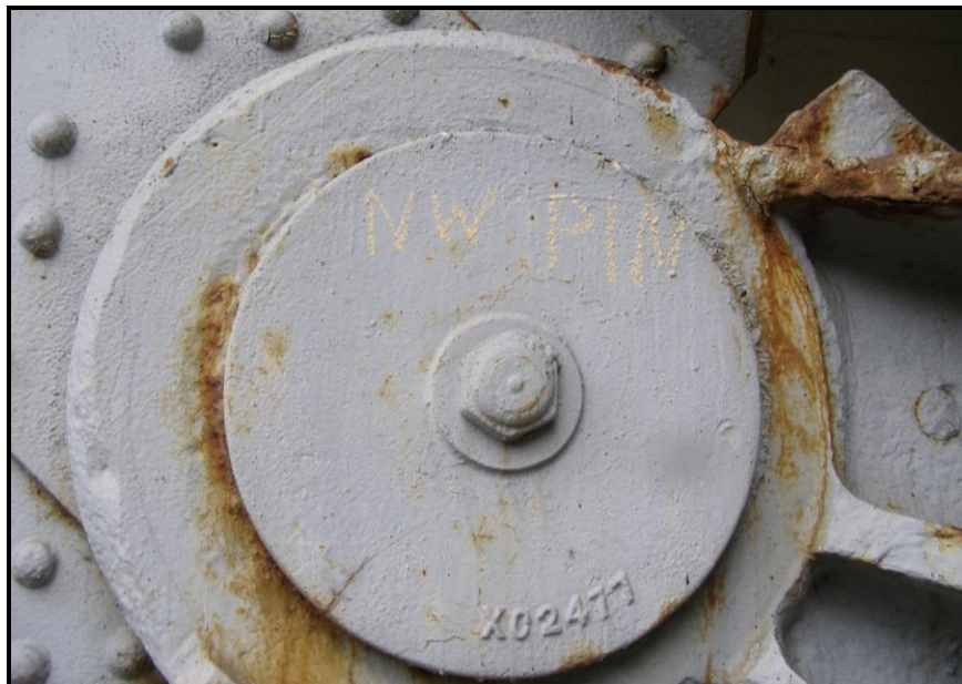
Photo 45: Cracked South Retaining Washer at L 0 - N
