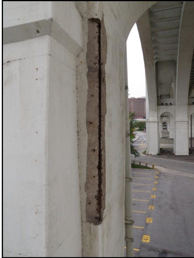
Photo 60: Typical Large Corner Spall on Tower 5
