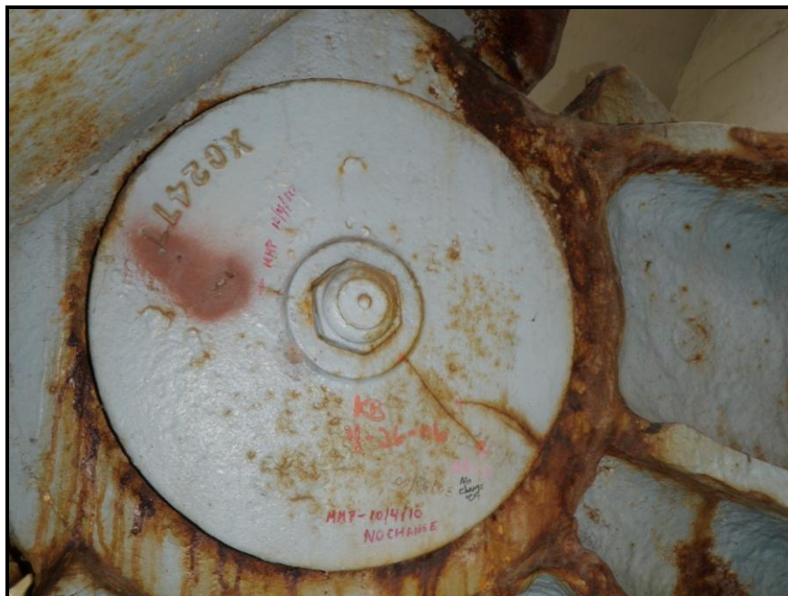
Photo 47: Cracked North Retaining Washer at L 0 - S. Note the New Crack on the Other Side of the Center Bolt.
