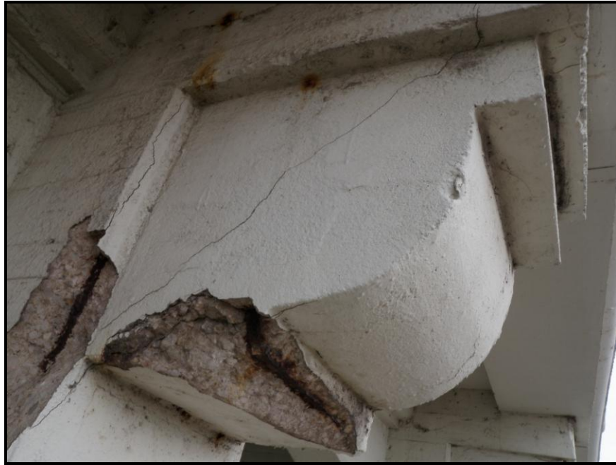
Photo 25: Corbel 12, Span 6 Completely Delaminated and Loose
