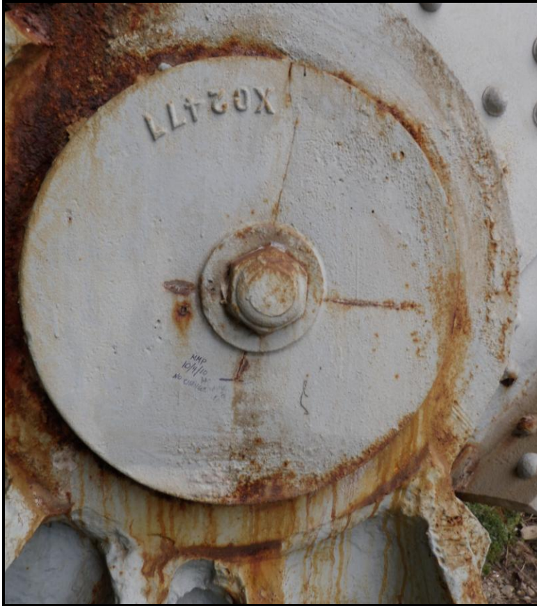
Photo 46: Cracked South Retaining Washer at L 0 - S. No Change to Previously Noted Cracks.
