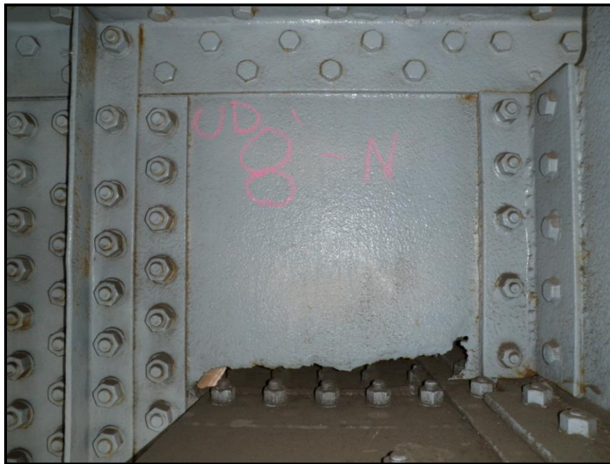
Photo 17: Hole in FB-U8'-N Showing No Change from Previous Inspection
