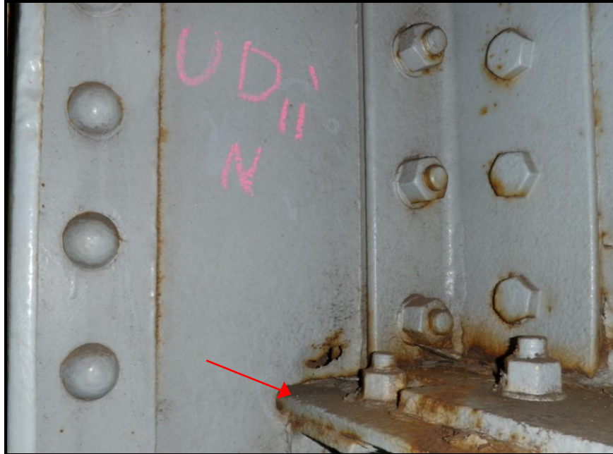
Photo 16: Hole in FB-U11'-N Showing No Change from Previous Inspection
