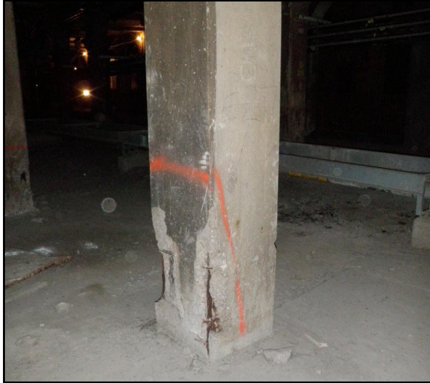
Photo 40: Typical Spalled Column Base
