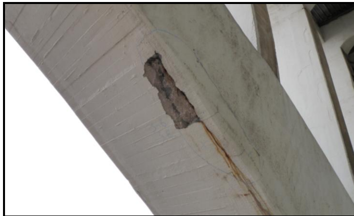
Photo 39: Spalled and Delaminated Area in the South Exterior Arch Rib of Span 6
