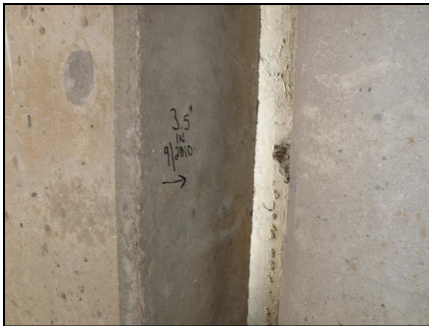
Photo 56: Gap Measurement between the East Edge of Tower B Showing the Amount of Rotation Away from the Surrounding Structure
