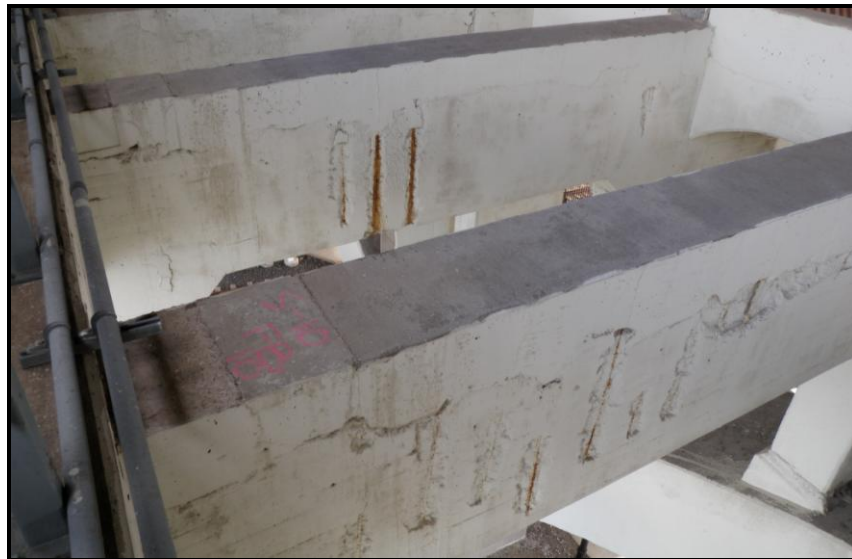
Photo 23: Typical Shallow Spalls over the Vertical Legs of the Stirrups in the Face of the Floor Beam
