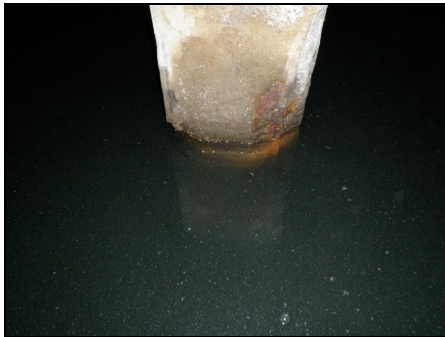
Photo 10: Standing Water in the East Tunnel
