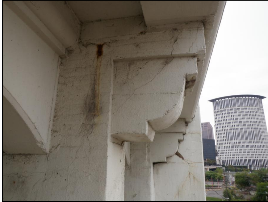
Photo 26: Corbel 14, Span 6 Completely Delaminated and Loose
