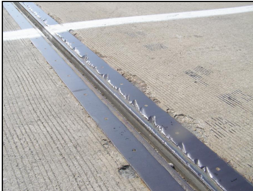
Photo 12: Typical Plow Damage to Joint Armor
