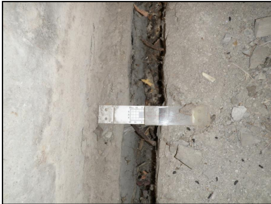
Photo 54: Crack Monitor Installed at the Interface between the Top of the Lower Deck and Tower B
