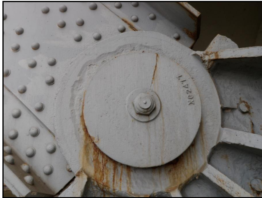
Photo 48: Cracked South Washer at L 0 - S
