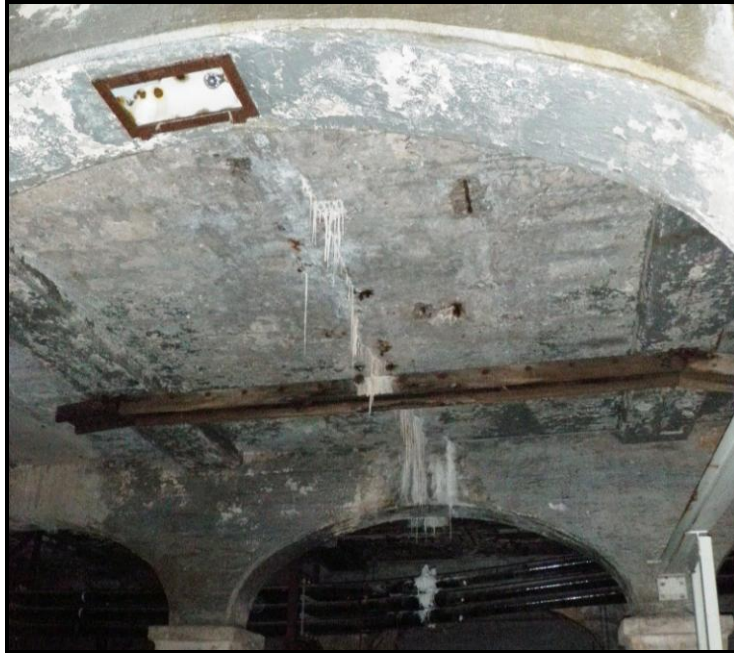
Photo 1: Large Crack with Efflorescence in the West Approach Tunnel
