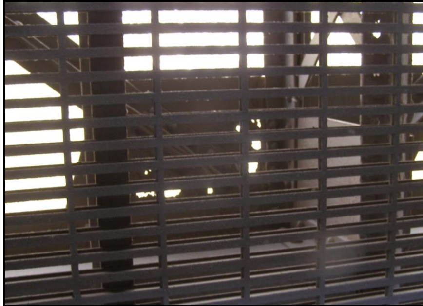
Photo 33: Through Holes in the Gusset Connecting the Lower Lateral Bracing with the Northern Most Exterior Stringer as seen through the Fiberglass Deck Panel
