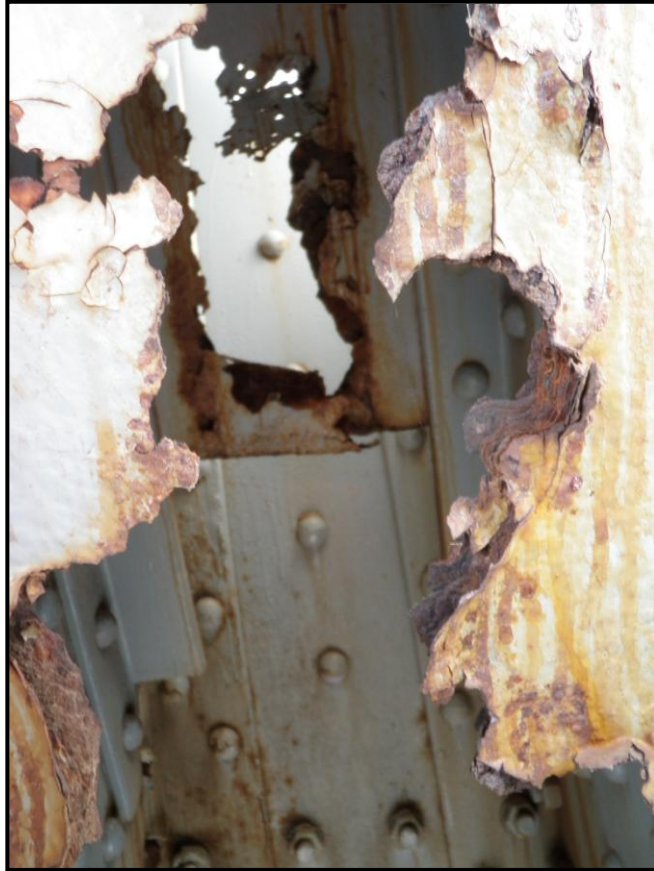
Photo 30: Holes through the Ends of the Vertical and Diagonal Members at the L 2 Panel Point in the South Arch
