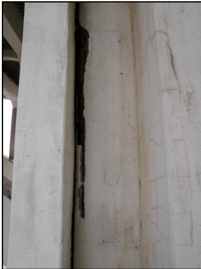
Photo 43: Large Corner Spall Removed along Column 1 on the North Exterior Arch Rib of Span 6. The Spall along Column 1 on the North Interior Rib is Similar.
