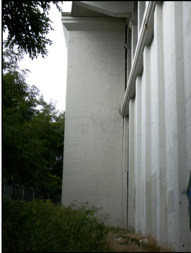
Photo 53: Tower B Rotating South Away from the Bridge. Note the Large Gap between the Top of the Tower and the Adjacent Jack Arch Column.
