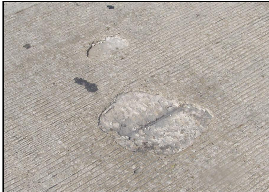
Photo 3: Wearing Surface Popout with Exposed Reinforcing Steel
