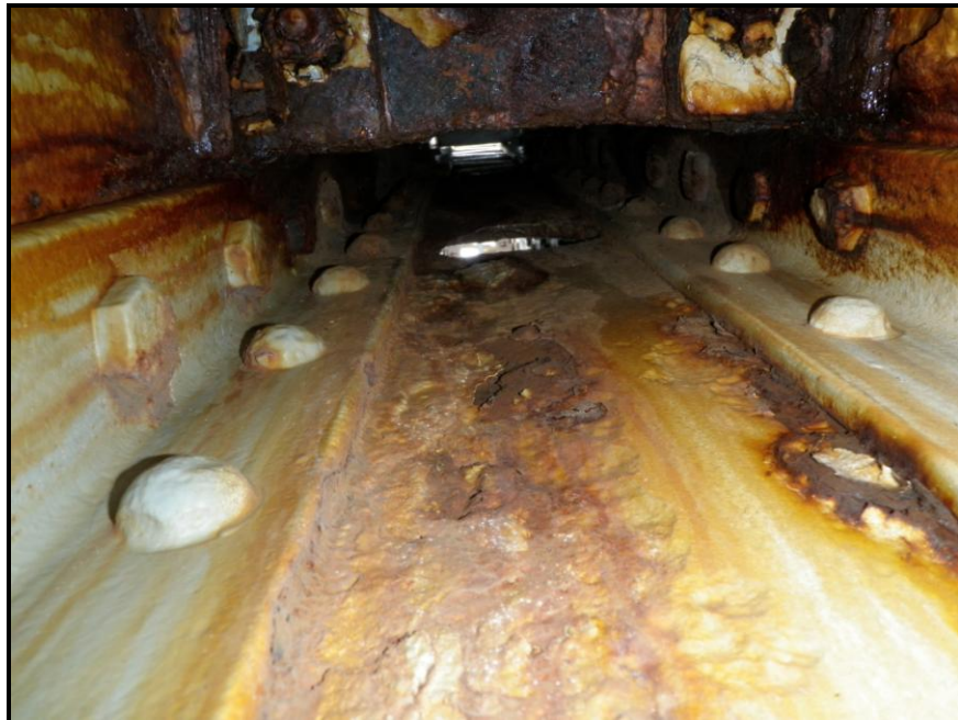
Photo 28: Through Holes in Cover Plate of L0-S Vertical
