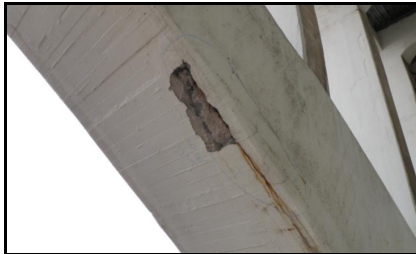
Photo 39: Spalled and Delaminated Area in the South Exterior Arch Rib of Span 6
