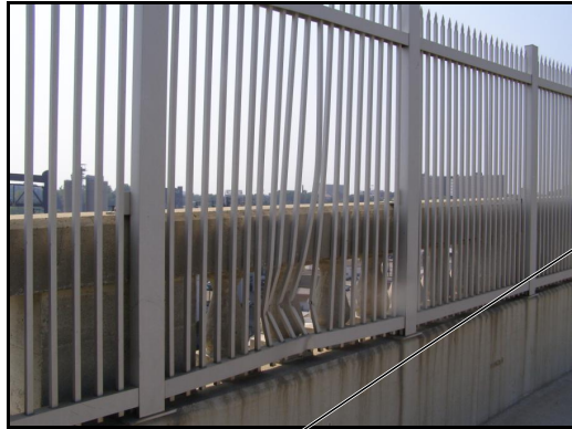
Photo 8: Damaged Vandal Protection Fence
