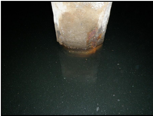
Photo 10: Standing Water in the East Tunnel
