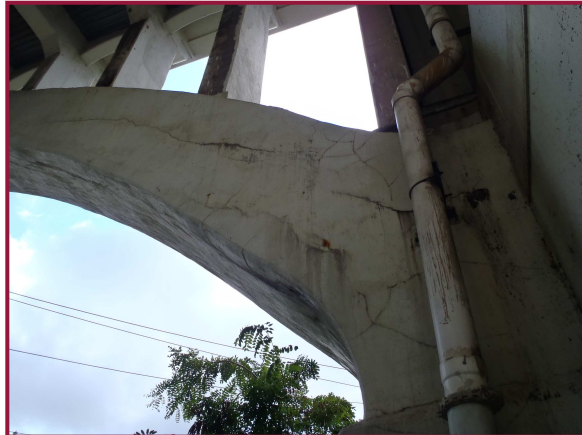
North face of Arch D in Span 2 with widespread cracking in the western 25' of the arch. Arch cracking is typical in Spans 1-3; however, the condition shown is worse than typical due to the adjacent drainage elements at this location.
