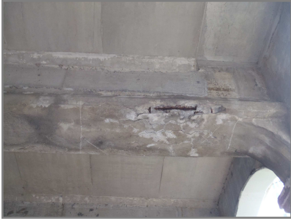
Photo 10 – Isolated spall with exposed reinforcement on the bottom face of upper Floorbeam 6 in Span 13. Note the retrofitted bottom flange.
