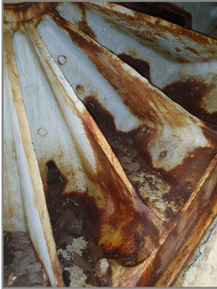
Photo 24 – Southwest truss bolster with significant section loss to the bearing stiffeners and rust reactivation.
