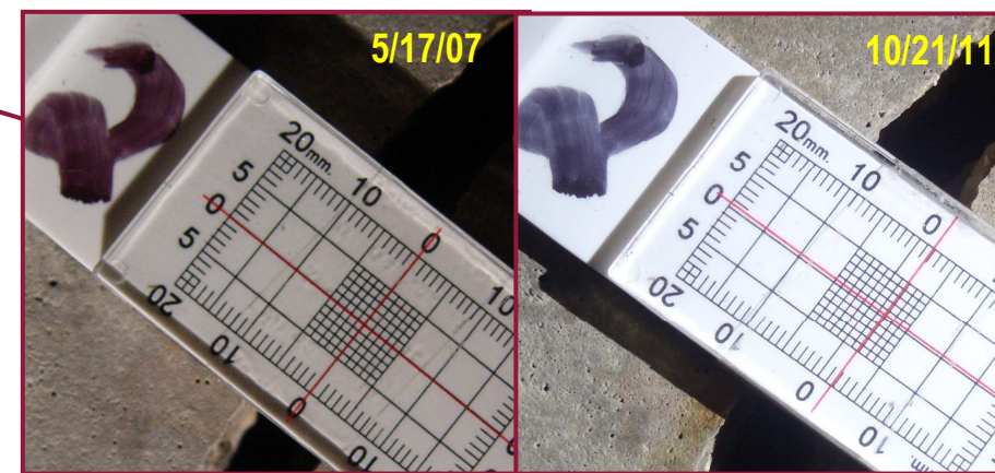
Crack Gauge 2 in Cell 2S of Span 1A exhibits approximately 2mm of movement since the gauge was installed in 2007.
