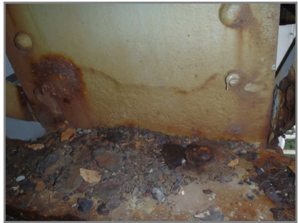
Photo 16 – Interior face of U4' L4' web with 1/16" deep pitting along the lower floorbeam top flange interface.
