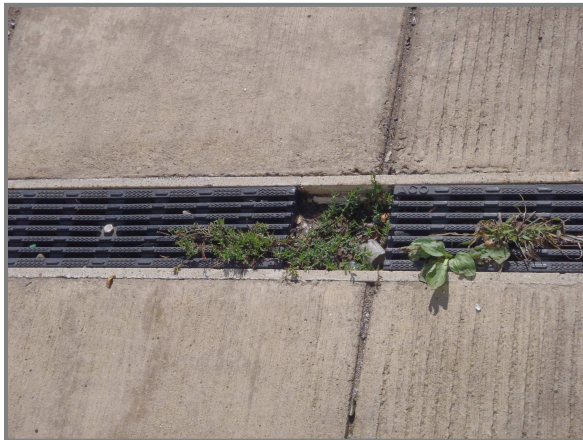
Photo 5 – Missing grate at longitudinal north sidewalk trench drain and vegetation becoming established.
