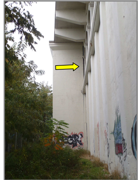
Photo 32 – Leaning South Tower B. Note the gap between the upper portion of the tower and the lower deck fascia members.
