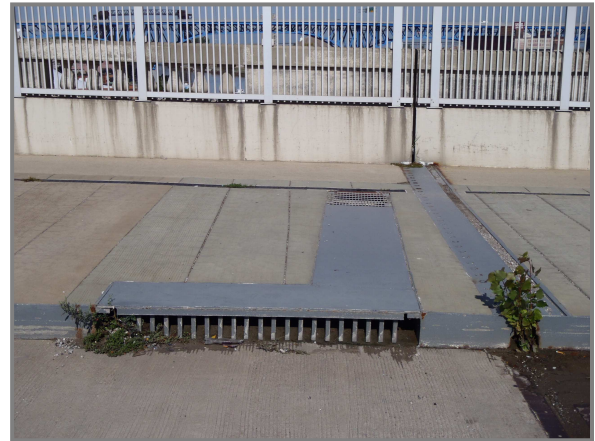
Photo 4 – Typical curb drain and heavy granular debris in the joint membrane at the curb.
