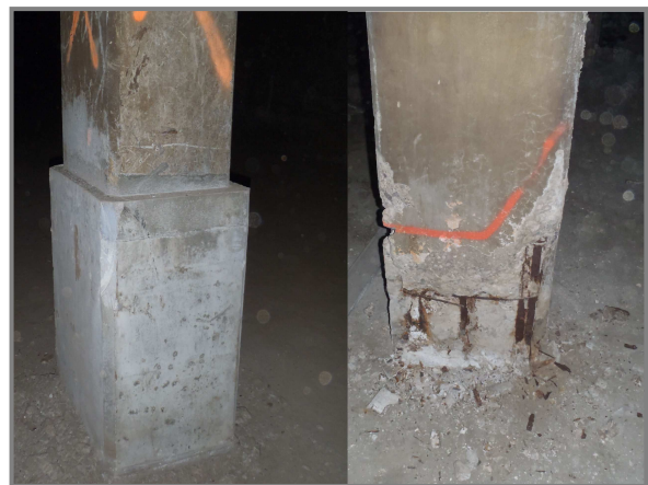
Photo 29 – Typical column base repaired (left) and unrepaired conditions (right).
