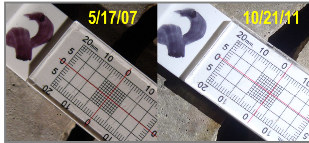
Photo 35 – Crack Gauge 2 showing approximately 2mm of movement since the installation in 2007.
