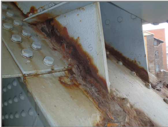
Photo 21: – West free edges of the south truss L2 gusset plates with pitting from 1/16" to 3/16" deep along the lower chord interface.
