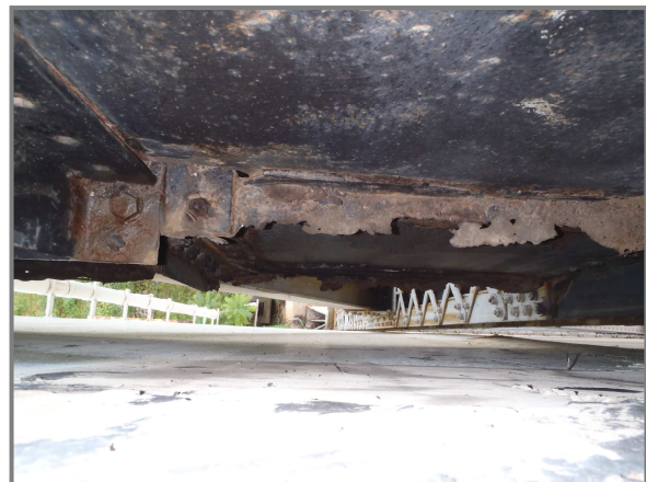
Photo 12 – West face, Floorbeam 0 north cantilever with heavy losses to both west flanges.
