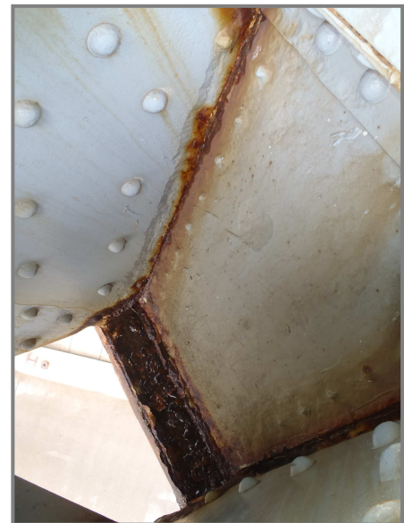
Photo 19 – Heavy losses on the interior face of the lower chord web plate at L1'LO'.
