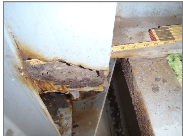
Photo 25 – Saddle bearing with 100% section loss.
