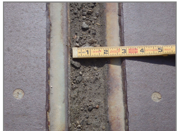
Photo 6 – Typical joint membrane with heavy granular debris.
