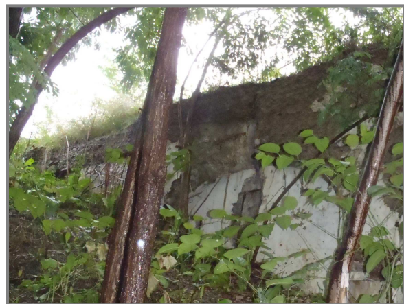
Photo 37 – Heavy deterioration of concrete at the southwest wing.
