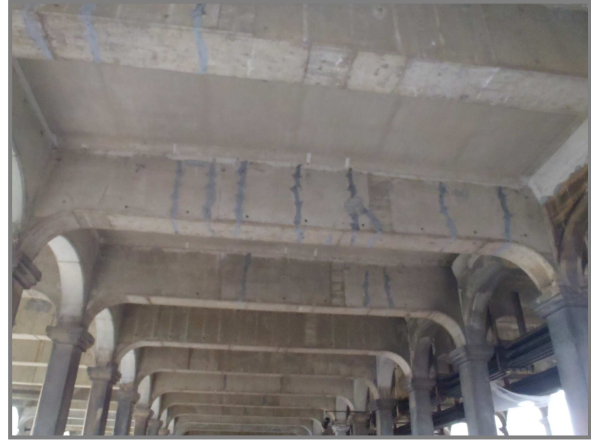
Photo 11 – Floorbeam 9 in Span 6, Bay B-C with epoxy injection repairs at transverse floorbeam cracking.
