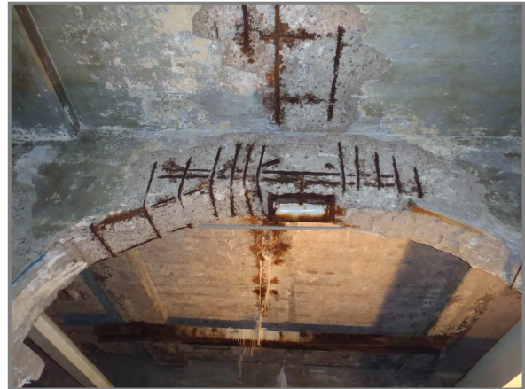
Photo 2 – Deck spall with exposed reinforcement and crack with heavy efflorescence in the West Approach.
