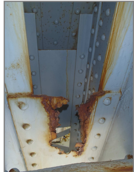
Photo 18 – Holed through portion of the underside stay plate at the lower panel connection of U1L2.
