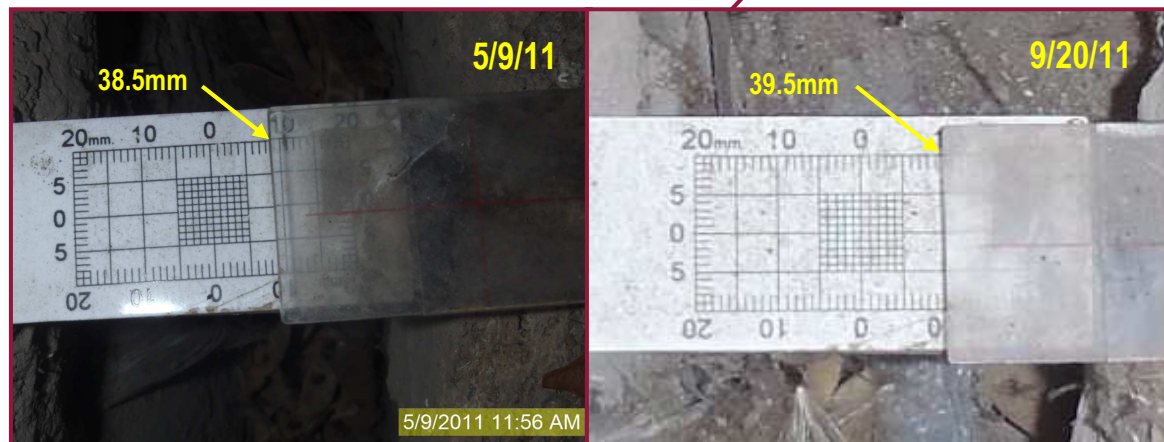
South Tower B crack gauge at the upper deck level showing 1mm of movement over a 4-month period. This gauge was originally installed in 2006 and indicates approximately 48.5mm (1.91") of movement since.
