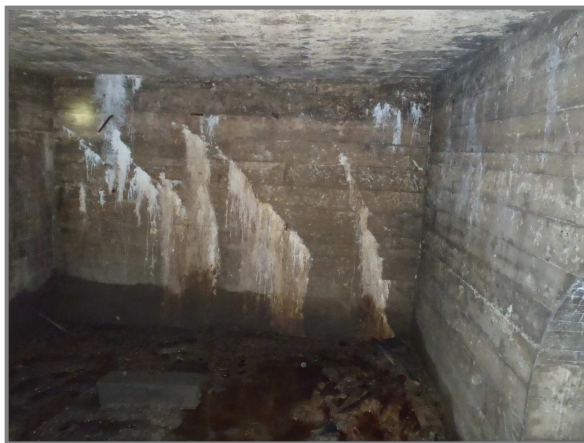
Photo 36 – Diagonal cracking and heavy efflorescence, north wall of North Cell 1.
