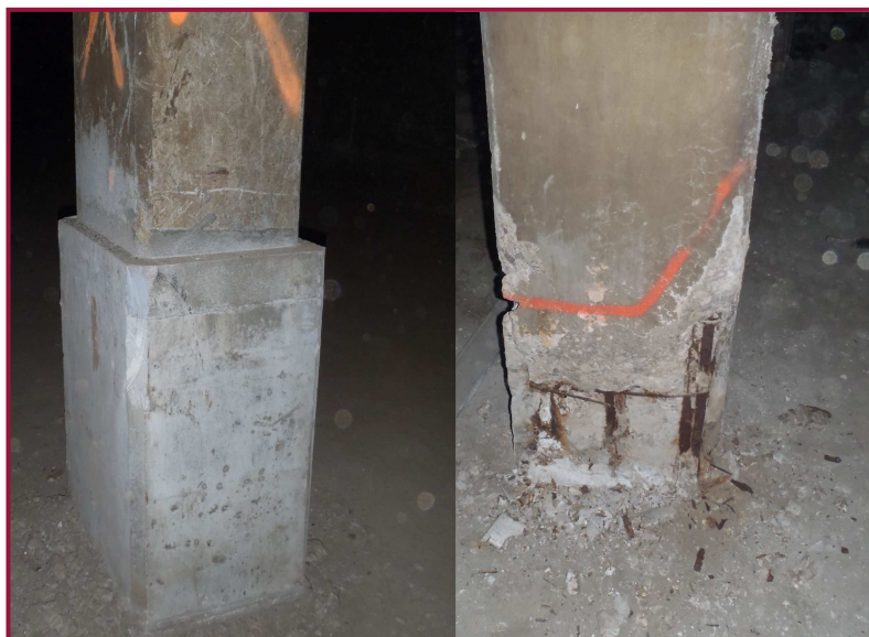
Columns in the West 25 th Street tunnel with typical base repair (left; column 6) and base deterioration (right; column 12).
