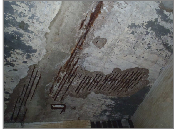
Photo 1 – Deck spall near the junction of the West 25th Street tunnel and the West Approach Spans.
