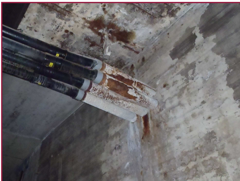
The utility conduit in Bay 31 (transverse to the tunnel) exhibits moderate corrosion of the projecting pipes at both walls (west wall shown). Note that the deck slab is leaking above this location, contributing to the corrosion.
