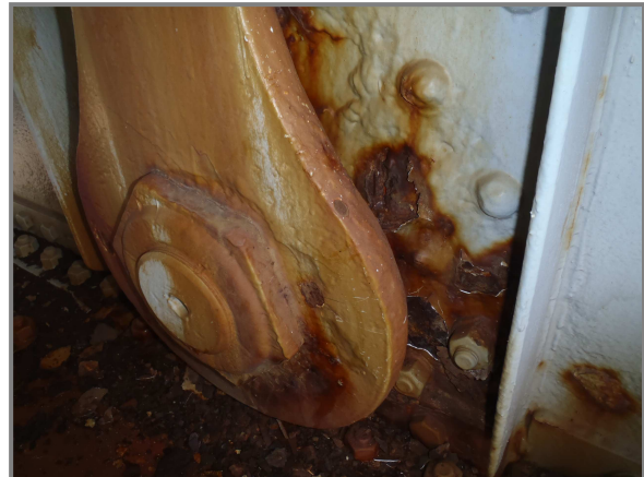
Photo 30 – East hanger, lower deck Floorbeam 4 of the North Truss with 3/16" - 1/4" deep pitting to the exterior face of the eyebar at the net section. Note the reactivation of rust and the advanced losses to the adjacent web-reinforcing pin plate.
