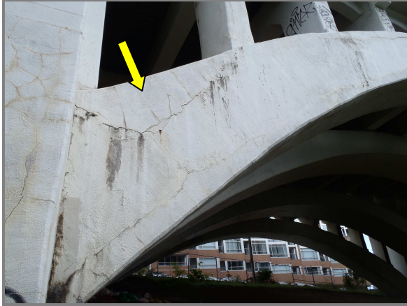
Photo 26 – Arch D in Span 1, South Elevation showing 1/16" wide cracking in the arch near the tower base. Note the large (~30sqft) delamination between the tower and column 1 (arrow).
