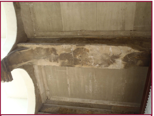
Floorbeam 16 between jack arch Lines C & D with transverse hairline cracking and light efflorescence throughout the bottom face. This condition is isolated throughout Spans 1-3, especially at floorbeams that have not been rehabilitated, as shown.
