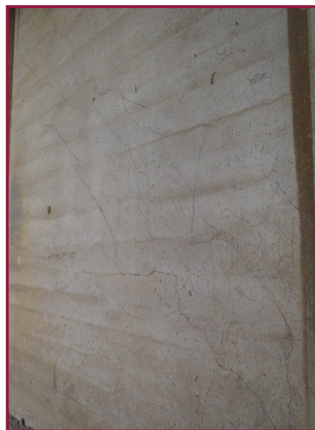
The south face of the South Center curtain wall in Span 1A exhibits diagonal cracking up to 1/16" wide.
