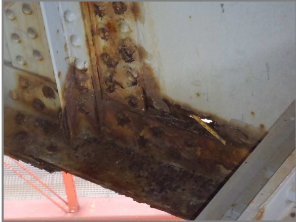
Photo 13 – Holed through Floorbeam 7' web (6" long x 1" tall) between south hanger and Stringer 10.
