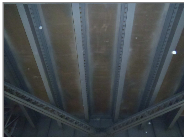
Photo 9 – Upper deck typical stringer condition, Bay 1-2 shown.
