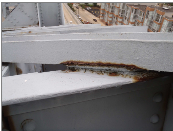
Photo 20 – Member L8L9 on the North Truss with 3/4" impacted rust between the middle intermediate diaphragm flange and the upper lacing channel.
