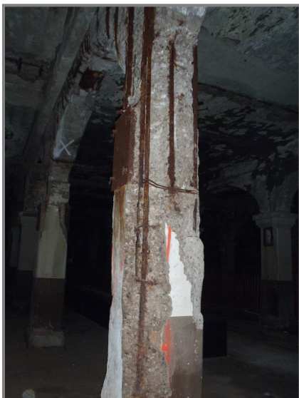
Photo 28 – Jack arch line B, Column 16 in the West Approach span with nearly 100% loss of cover.
