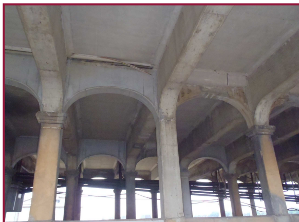
Jack arch Line B in Span 3, typical for Spans 1-3. Note that portions of the arches, columns and floorbeams have been repaired (light in color), while other portions were not (discolored).
