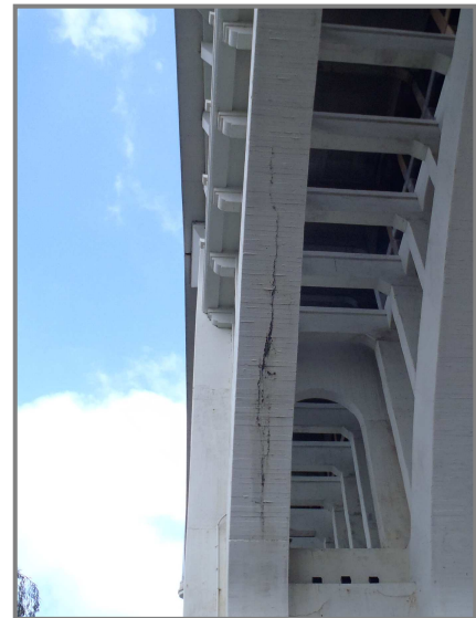
Photo 27 – Arch A in Span 5 with an approximately 1/4" wide x 40' long longitudinal crack.
