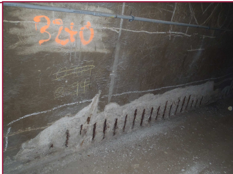
Approximately 8' long section of localized spalling of the bottom 2'-3' of the east wall in Bay 11. Exposed reinforcement exhibits negligible loss.
