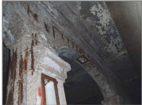
Photo 7 – Jack arch spalling in the West Approach. Jack arch 12-13 in Line C shown.
