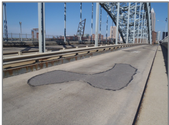
Photo 3 – Large spall with asphaltic patch in Span 4 right eastbound traffic lane.
