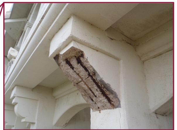
Span 7 Column 10 corbel outside northernmost concrete arch with front face spall and exposed reinforcing.
