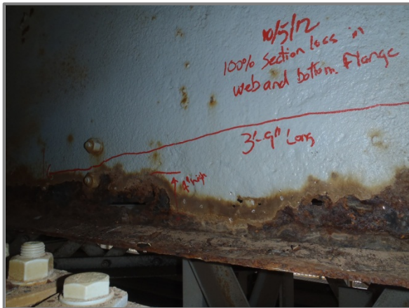
Photo 9 – Stringer P between Floorbeams 20 and 21 with 100% section loss in web and bottom flange.
