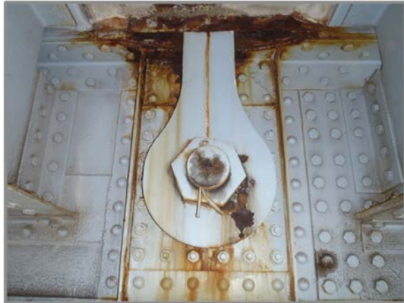
Photo 42 – West face of eyebar at connection to south lower pin at Panel Point 11. Note moderate corrosion throughout area but section loss on eyebar.
