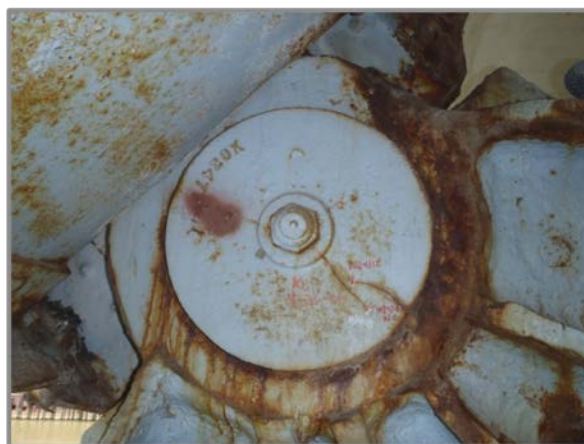
Photo 33 – North pin retaining washer at L0 South Truss with 2 radial cracks.
