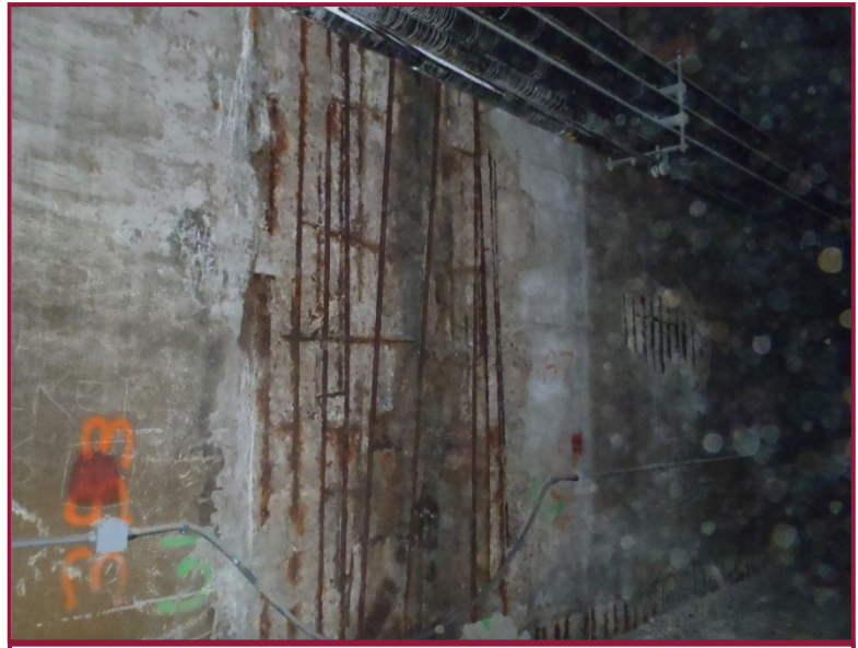
Full height by 8' wide spall with exposed reinforcement in south wall between Columns 19 and 20 (joint location). Several reinforcing bars have 100% section loss. This condition is common at joint locations throughout the Detroit Avenue Tunnel.
