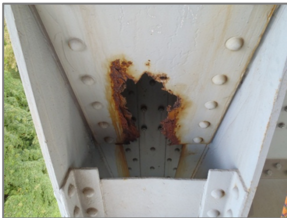
Photo 22 – Holed through portion of underside batten plate of North Truss U1-L2 at lower chord gusset plate.
