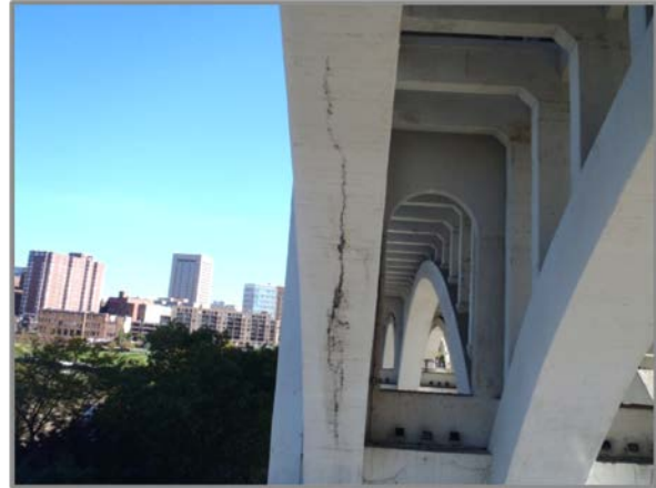
Photo 36 – Span 5 Arch A exhibiting longitudinal crack approximately 1/4" wide by 40' long on underside of arch rib.
