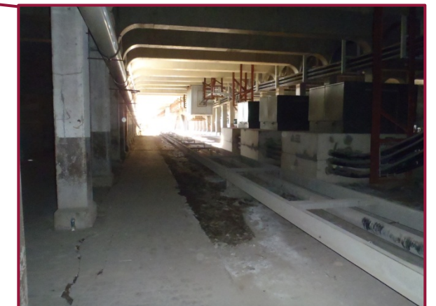
General view looking west through center bay of West Side Station. Note utility conduits mounted to structural elements within the area.
