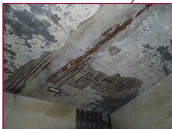
Large spall (~30 ft 2 ) in the deck underside between jack arch Lines G and H. Spalls are common throughout the upper deck floor in the West Approach, typically ranging from 2 ft 2 -10 ft 2 .
