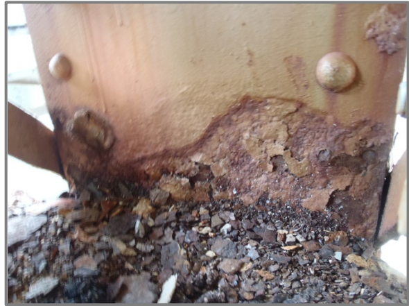
Photo 20 – South Truss vertical member U3-L3 with heavy active corrosion and section loss to interior faces of box section (west web plate shown).
