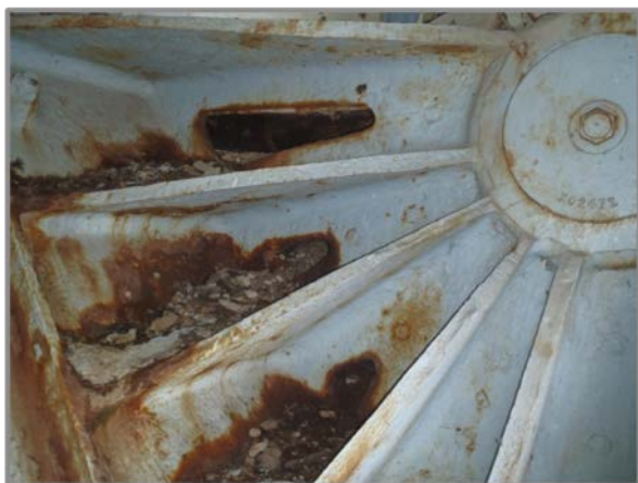
Photo 32 – Northwest truss bolster with substantial section loss to bearing stiffeners and rust reactivation.
