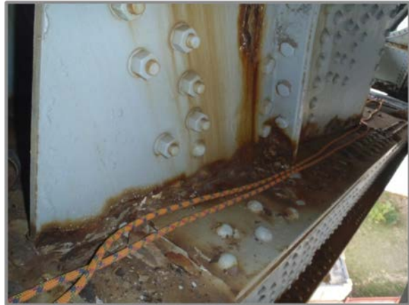
Photo 26 – North truss interior L20 gusset plate with heavy pitting and active corrosion on south face along west lower chord connection.
