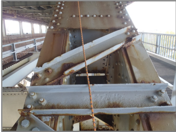
Photo 25 – North Truss member L20-L21 with heavy section loss on top lacing channels east of L20.
