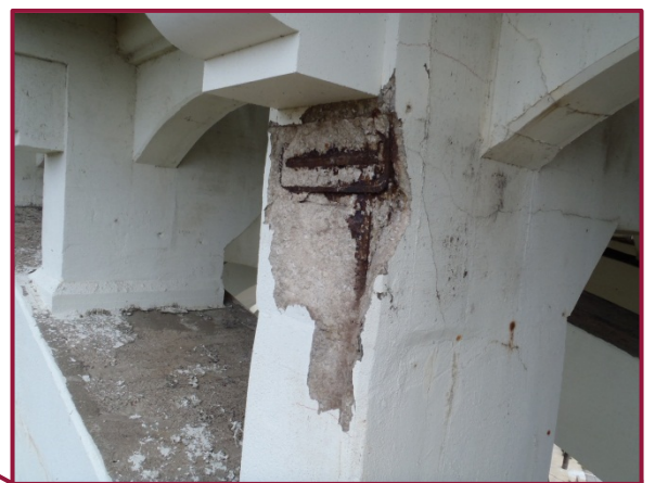
Arch A Column 5 in Span 7 exhibits a spall with exposed reinforcing 39" high x 25" wide x 3" deep below the lower concrete corbel.
