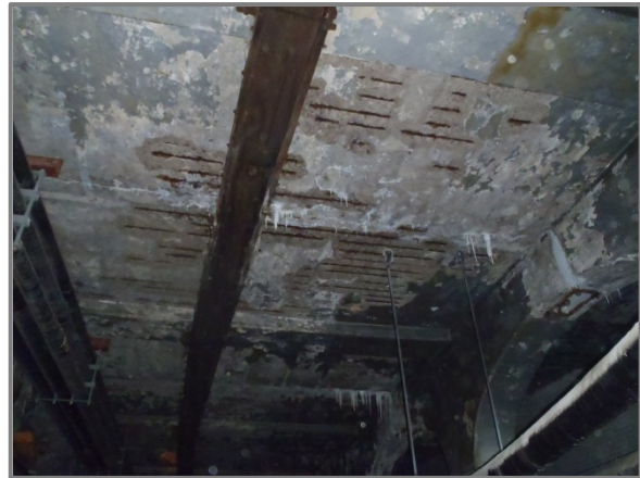
Photo 1 – Deck underside spall and heavy efflorescence in West Side Station between column lines D and E.
