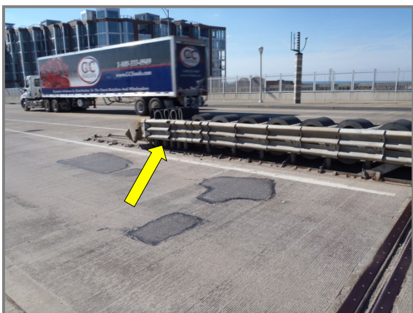
Photo 53 – Eastbound impact attenuator exhibiting damage from vehicular impact at the west end of the South Truss.
