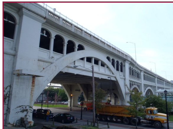
General view of Span 12 overall (north elevation shown). This span is unique in that the lower deck is supported by concrete hangers, making this span a through-arch system.
