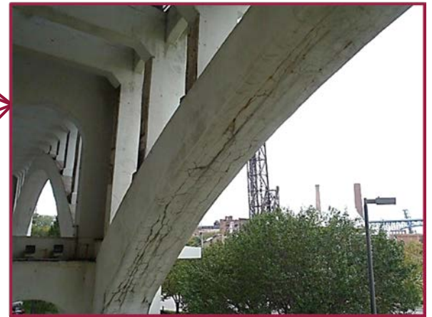
Arch A in Span 10 exhibits widespread map cracking throughout the bottom face of the arch rib, especially in the end 30' to 40' adjacent to the piers (west end at Pier 9 shown, east end similar).
