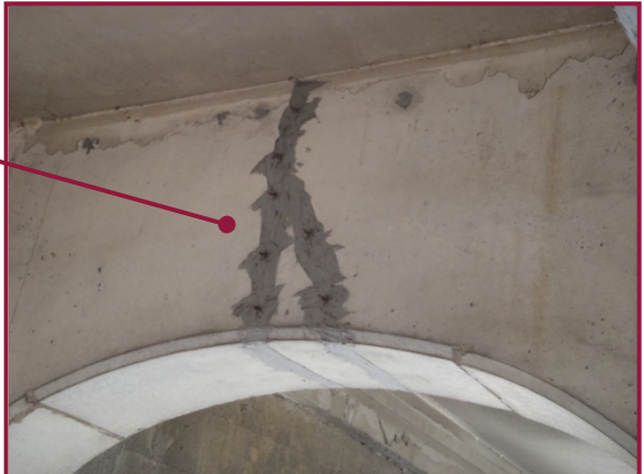
Typical replaced concrete jack arch in Span 9 (Line B between Floorbeams 4 and 5 shown). The jack arch at this location exhibits transverse vertical cracks that have been repaired by epoxy injection.
