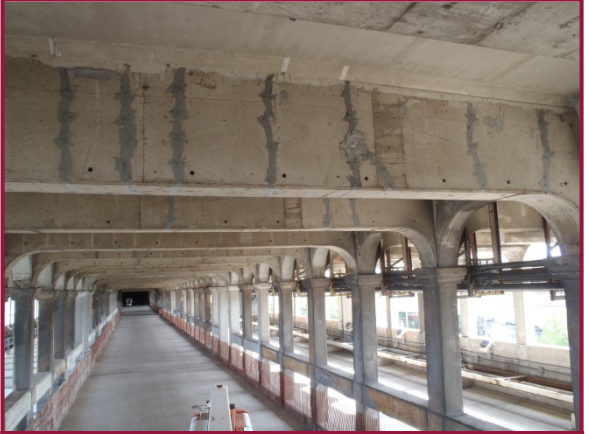
Span 9 Floorbeam 6 with vertical cracks repaired by epoxy injection between Column Lines B and C (west face shown). This repair detail is common throughout the East Approach Spans.
