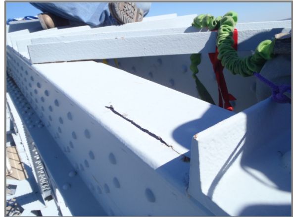
Photo 23 – South Truss U7-U8 with 8" long by 1/2" wide by 1/16" thick laminar tear in north top flange angle.
