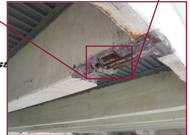
Isolated hangers and floorbeam members in Span 12 consist of concrete-encased steel beams. The underside of Floorbeam 4 is spalled at the connection to the south fascia, exposing a portion of the embedded steel beam and surrounding reinforcing.
