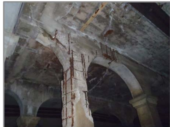
Photo 38 – Easternmost column in West Side Station jack arch Line C with heavy spalling and exposed rebar on all faces.
