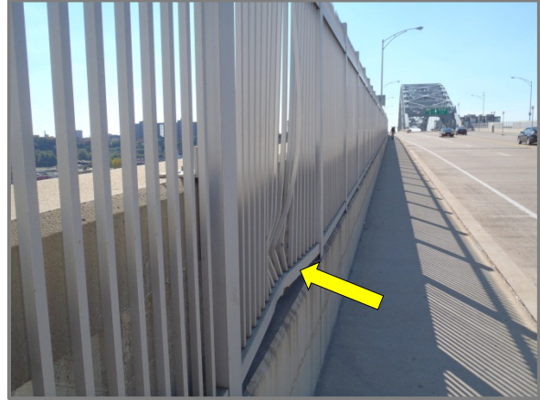
Photo 4 – Pedestrian protection fence with impact damage in Span 7.
