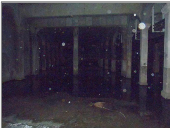
Photo 5 – East approach cellular construction with standing water.
