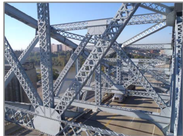
Photo 30 – General view of main truss sway bracing, looking west from Panel Point 8.
