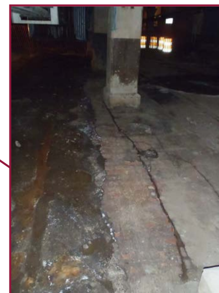
Crack in lower deck up to 1" wide extends from approximately Column 3 to Column 14 along Line D.
