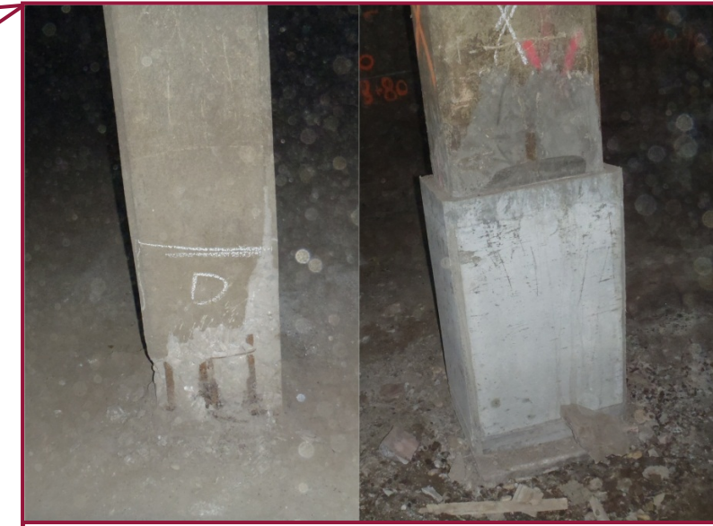
Isolated columns throughout the West 25 th Street Tunnel exhibit delaminations or spalls with exposed reinforcement at the base (left; Column 14). Numerous column bases have received repairs at this location (right; Column 6).
