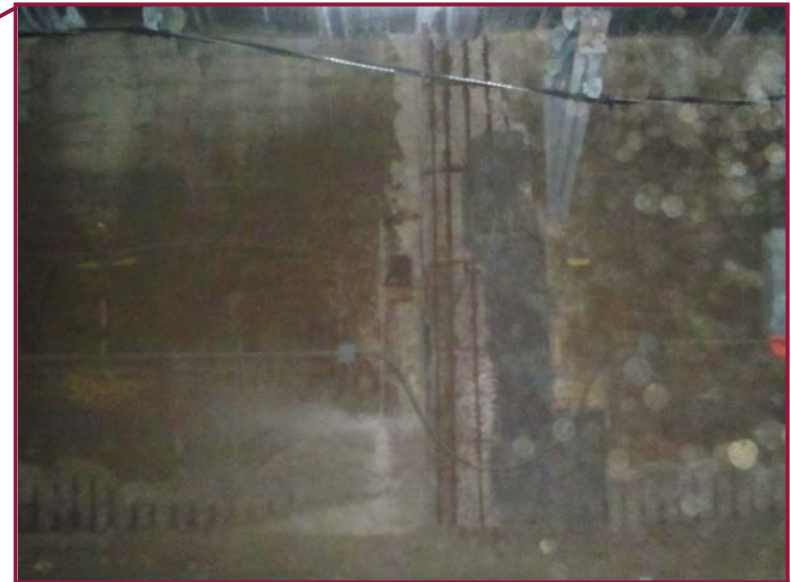
The east wall in Bay 30 (joint location) exhibits a full height spall and partial concrete repair. This condition is common at joint locations throughout the West 25 th Street Tunnel.
