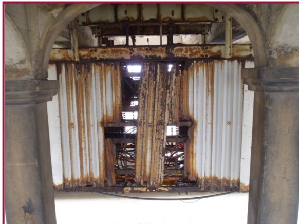
Utility junction box in Span 6 with advanced corrosion throughout and failed corrugated metal outer containment. Deterioration is due to water infiltration through access manhole above.
