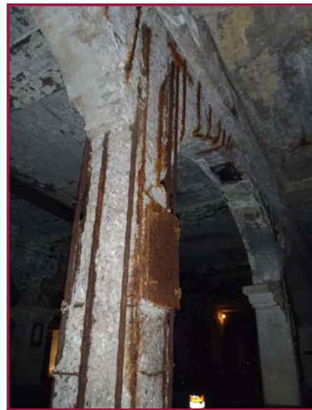
Column 16 in jack arch Line A with advanced spalling and fully exposed reinforcement with section loss.
