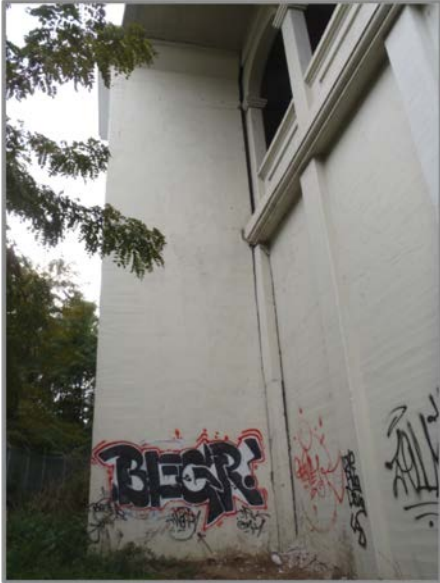
Photo 44 – East elevation of South Tower B. Note the gap between the upper portion of the tower and the lower deck fascia members.
