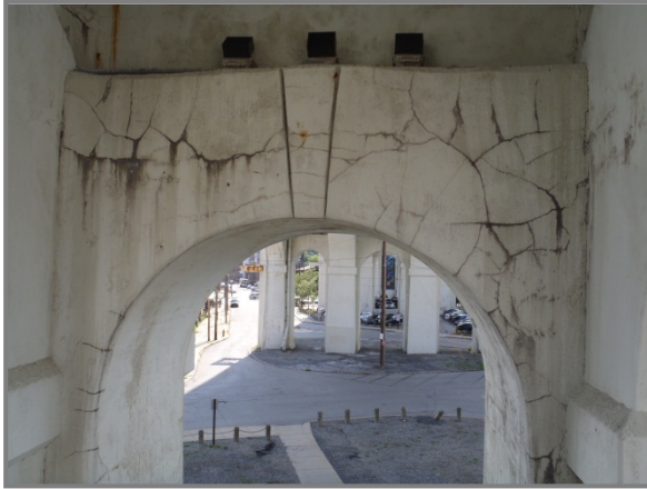
Photo 47 – Pier 7 lateral strut between Arch lines B and C with map cracking throughout.
