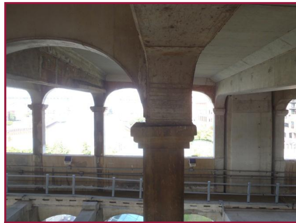
Jack arch to floorbeam connection misaligned horizontally with approximately 4" offset to the east with respect to column B8 below in Span 11.
