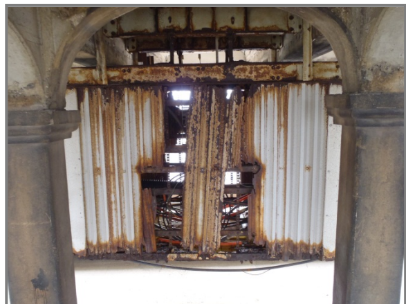
Photo 54 – Utility junction box in Span 6 with advanced corrosion throughout and failed outer containment. Deterioration is due to water infiltration through access manhole above.
