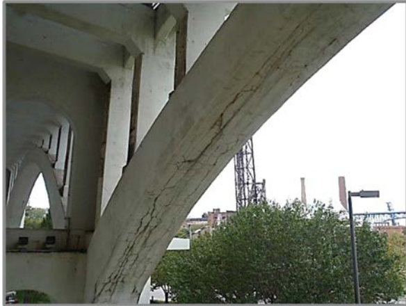
Photo 35 – Map cracking throughout underside of Arch A in Span 10, looking west toward Pier 9.
