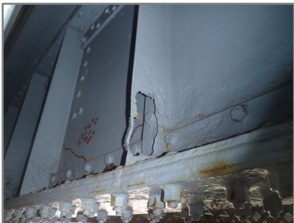
Photo 17 – West face of Floorbeam 0 with heavy losses to the web plate, web stiffeners and bottom cover plates.
