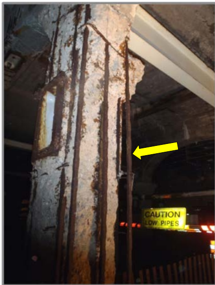
Photo 37 – Column C13 in West Side Station with advanced spalling and fully exposed reinforcement exhibiting moderate loss of section. Condition has worsened since previously noted during the 2011 inspection.
