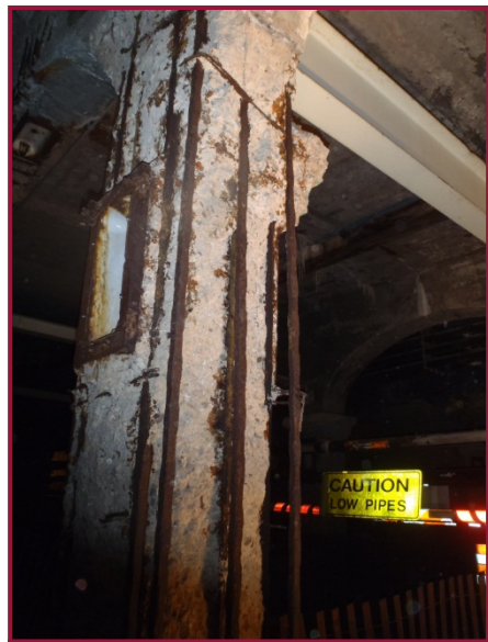
Column 14 in Line C exhibits up to 5" deep spalling, significant loss of concrete cover and exposed rebar with minor section loss. While large spalls are common throughout the concrete columns, the magnitude of deterioration shown here is isolated to only a few locations.
