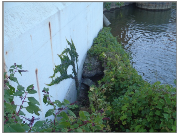
Photo 51 – Sinkhole along north face of Pier 4 which has increased in size since last inspected.
