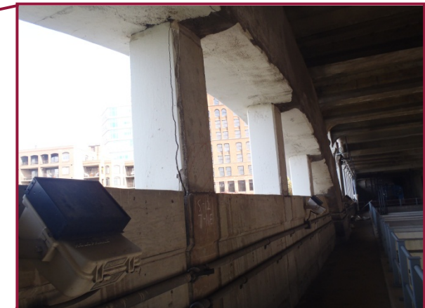
Isolated cracking is common on the concrete arch ribs and hangers in Span 12. The arch ribs typically exhibit moderate map cracking on the undersides as they pass through the lower deck, while large vertical cracks and delaminations are common on the concrete hangers.
