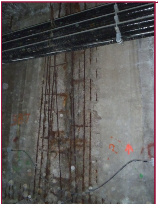
South wall exhibits a 6' wide by full height spall with exposed reinforcement adjacent to Column 23. Several vertical bars exhibit 100% section loss
