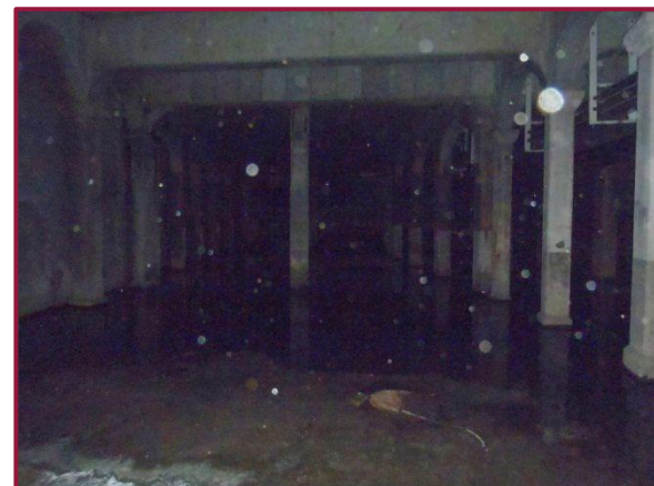
East approach cellular construction with standing water on the lower deck level, looking east. This standing water covers the entire width of the deck, beginning midway through the East Side Station and increasing to a maximum depth of roughly 3' at the east end.
