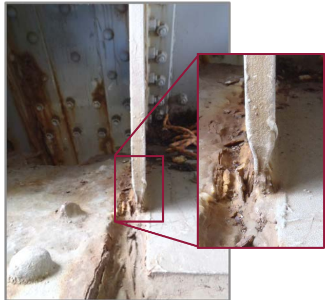
Photo 27 – South Truss L2 interior gusset plate with 1/4" effective thickness remaining for 24" along connection to member L2-L3.
