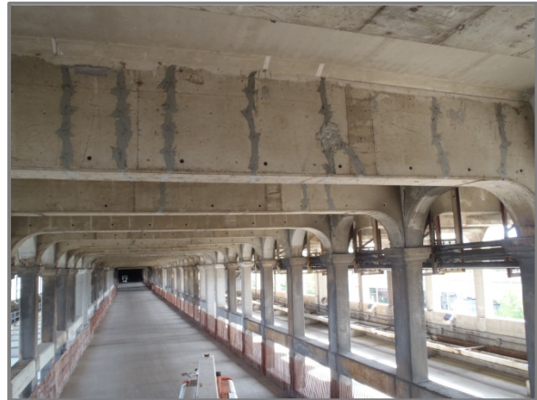
Photo 13 – Span 9 Floorbeam 6 west face with epoxy injection crack repairs between interior column lines.
