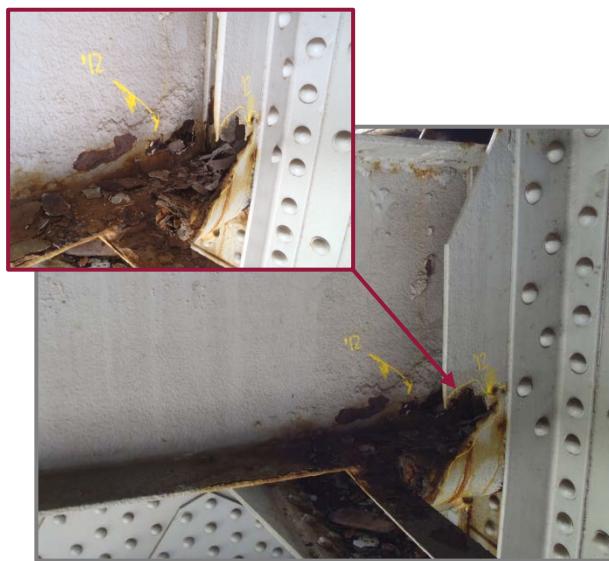
Photo 34 – Lower deck Stringer 10 south face saddle bearing at Floorbeam 21. Note 100% section loss on the stringer web, bottom flange, and saddle bearing.
