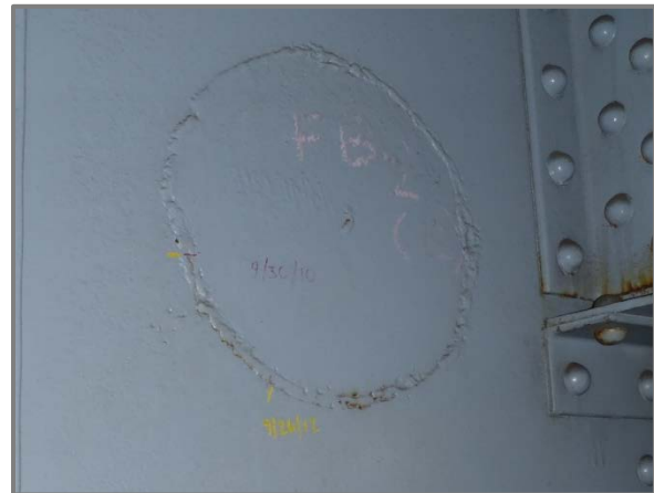
Photo 19 – Floorbeam 23 east face near North Truss with circular retrofit exhibiting a broken weld which has propagated a total of 3/8" since the 2010 inspection.
