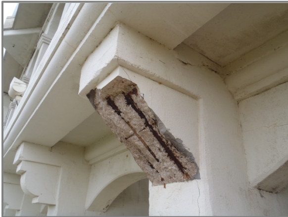
Photo 12 – Span 7 Column 10 corbel outside northernmost concrete arch with front face spall and exposed reinforcing.
