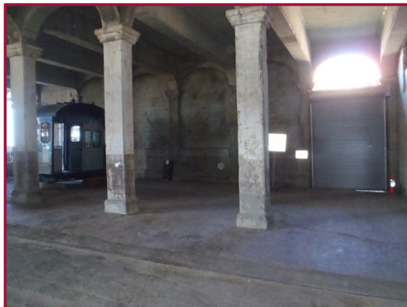
The concrete columns in the East Side Station typically do not exhibit significant deficiencies.
