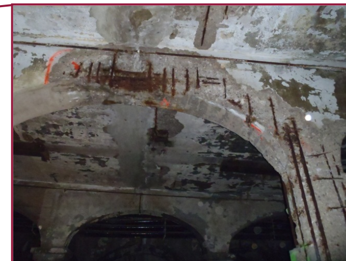
The Line C jack arch between Columns 24 and 25 exhibits advanced spalling with exposed reinforcement throughout the north face. This spalled area extends into Column 25.
