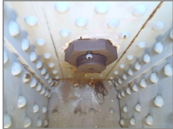
Photo 43 – Unpainted west pin nut on upper eyebar connection at L13 North. Active rust present with no measureable section loss.
