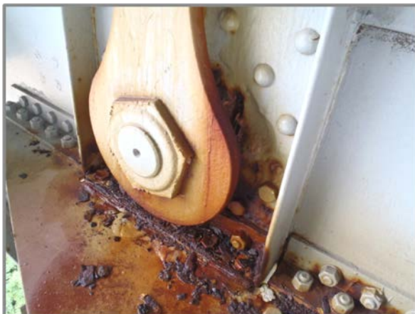
Photo 41 – East lower eyebar connection at L4 North. Note active corrosion in area and up to 3/8" pitting on pin plate.
