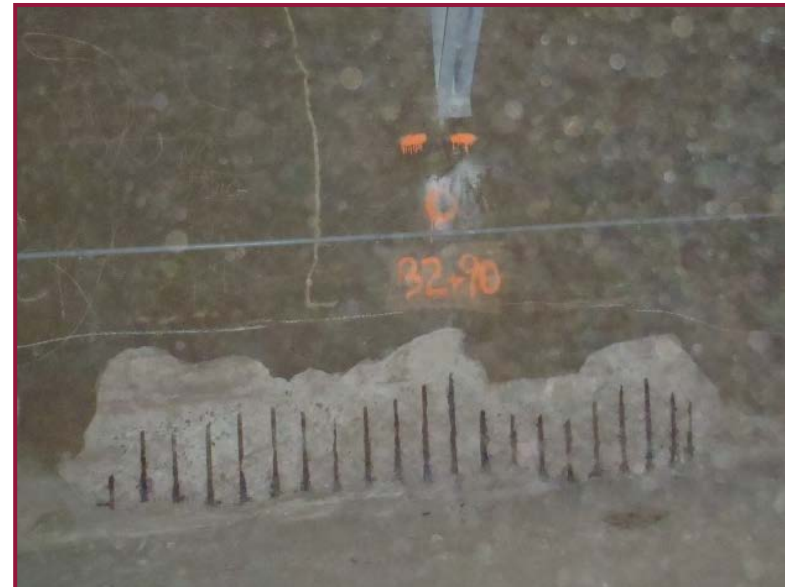
Approximately 8' long section of localized spalling along the bottom of the west wall in Bay 12. Exposed reinforcement typically exhibits negligible loss.
