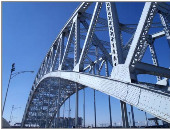
Photo 40 – General view of South Arch, looking west, showing overall paint condition of members above deck.
