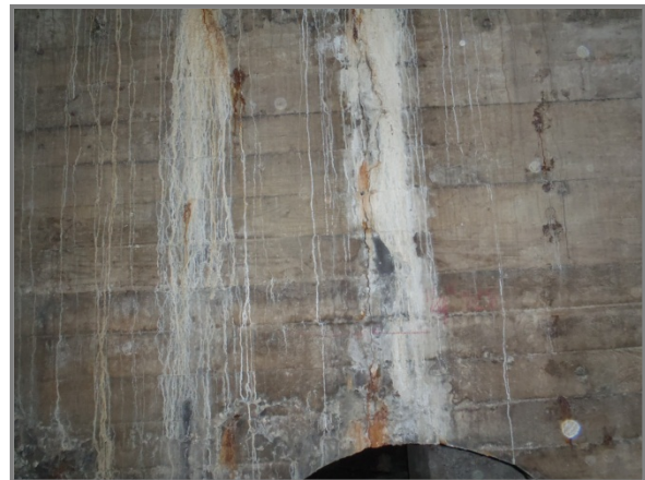
Photo 49 – Cell 0N in Span 1B with 1/2" crack with spalls and heavy efflorescence on east face.
