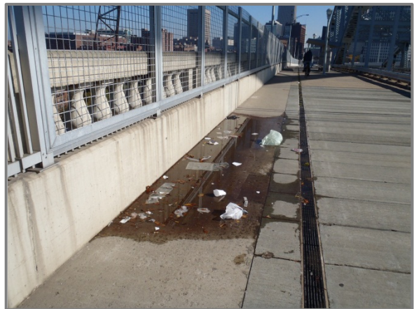
Photo 6 – Standing water on north sidewalk in Span 4, looking east.
