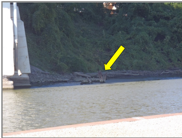
Photo 50 – Failed sheet pile protection downstream of Pier 3.
