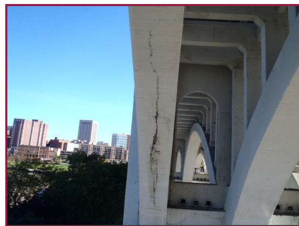
Arch A at the east end of Span 5 exhibits a longitudinal crack approximately 1/4" wide by 40' long on the arch rib underside. This represents the most advanced cracking in the concrete approach spans.
