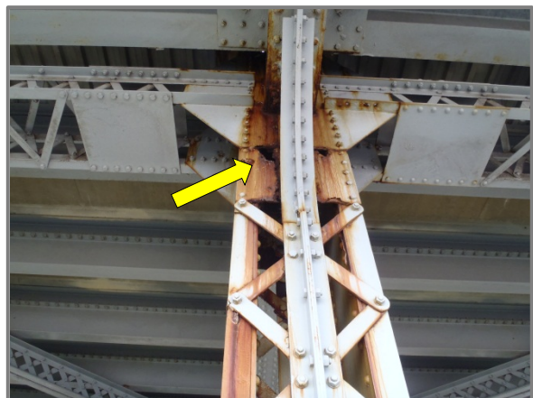
Photo 21 – North Truss U3-L3 north face with 100% section loss in batten plate at longitudinal strut connection.
