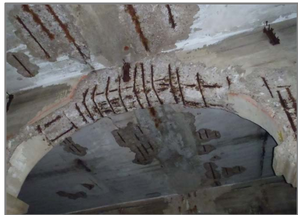
Photo 8 – Spall with exposed reinforcing in West Side Station jack arch between Columns B26 and B27.
