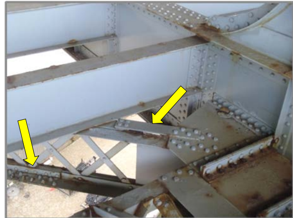
Photo 29 – Lower framing lateral bracing member with multiple bolted retrofits near connection to east face of Floorbeam 16.
