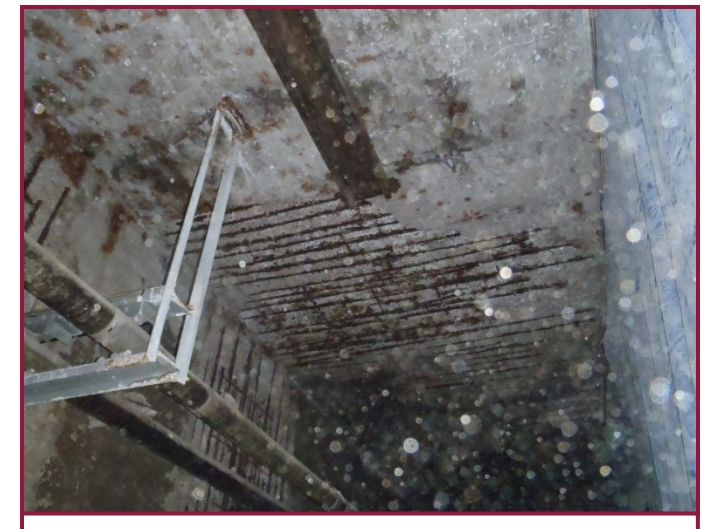
Large spall (~200 ft 2 ) in deck underside adjacent to the north wall between Columns 46 and 47. All transverse reinforcing bars are exposed within spalled area.
