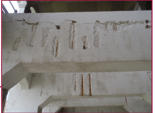
Lower floorbeam 10 in Span 10 exhibits intermittent spalling across the west face between Arches A and B, corresponding to locations of reinforcement. This condition is typical for the north bay in Span 10.
