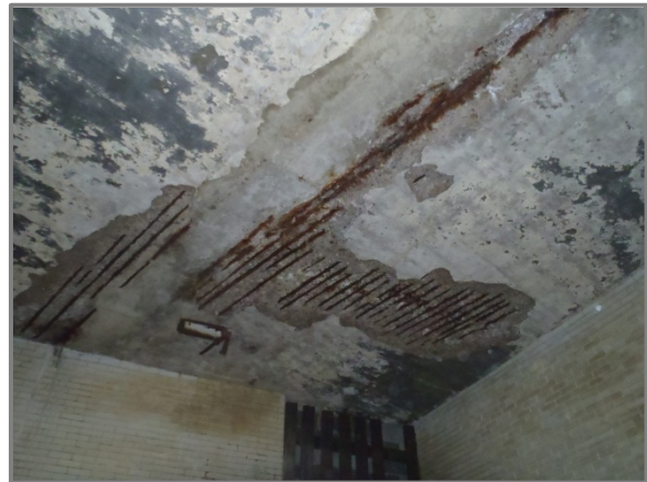
Photo 2 – Spall with exposed reinforcing in West Side Station deck underside adjacent to West 25th Street Tunnel.
