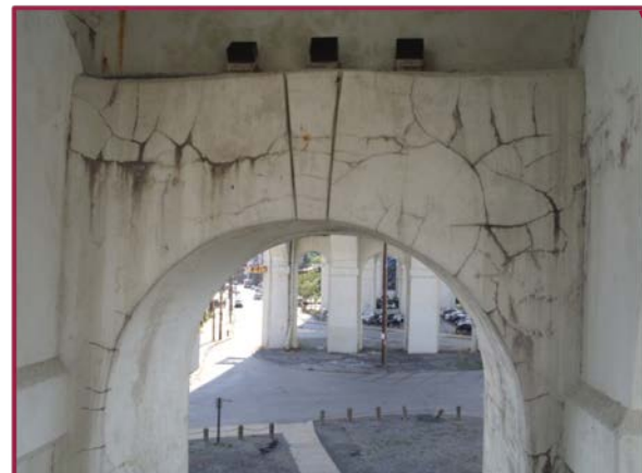
Pier 7 lateral strut between Arches B and C with map cracking throughout. Minor to moderate map cracking is typical at the thrust blocks at each tower base and throughout these adjacent lower struts.
