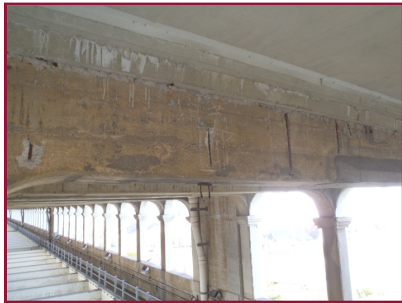
Floorbeam 3 in the north bay of Span 12 exhibits isolated web spalling at vertical reinforcement locations along the east face.
