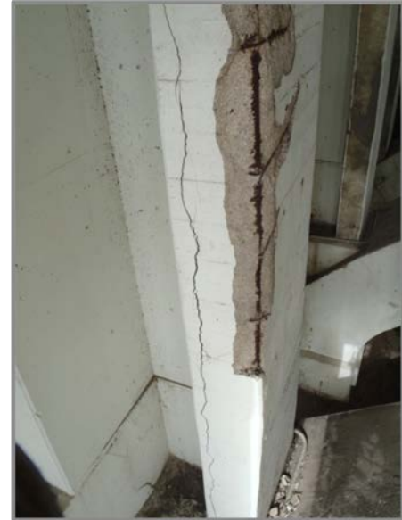
Photo 39 – Span 2 Column 1C with southeast corner spall and exposed reinforcement with section loss.
