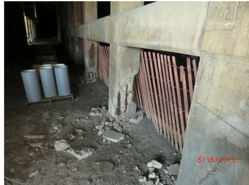
Arch columns 8,9 and 10 in South Interior row at west approach span 1B.
