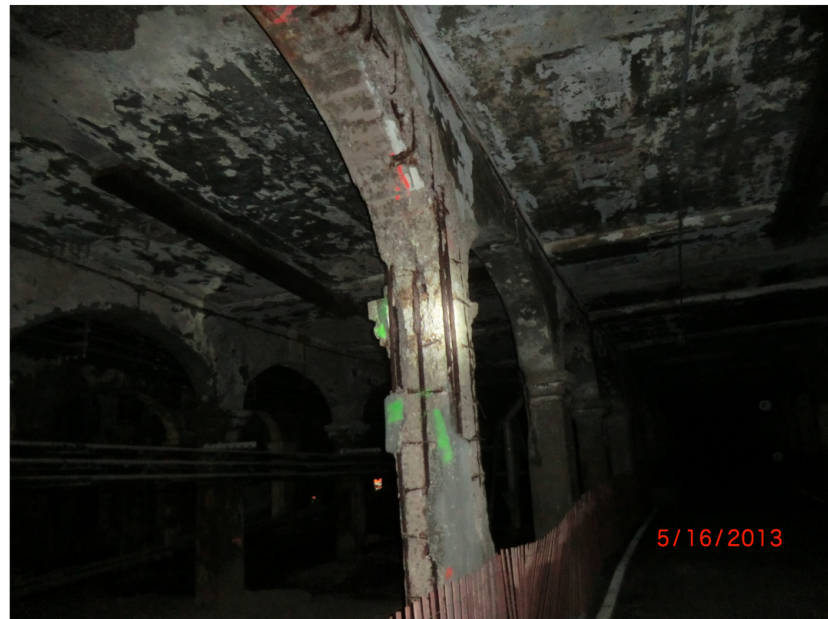
Spalling with 360 degree reinforcement exposure at Column 12 in Row C, West Side Station
