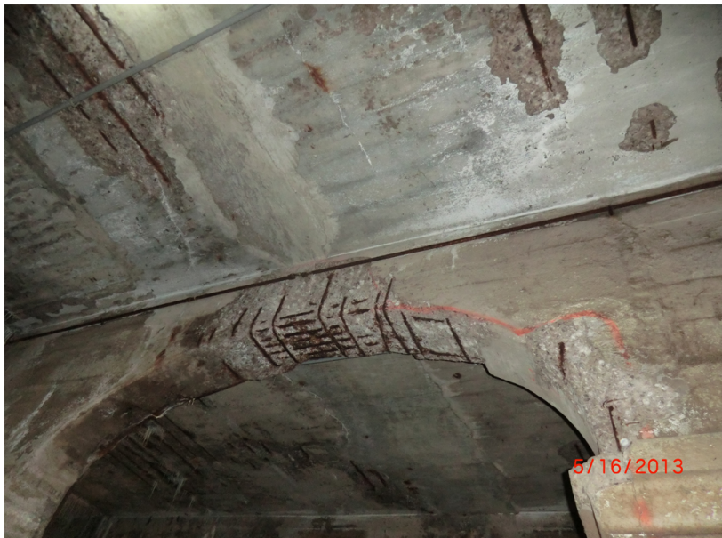
Spalling between columns in row C at the West Side Station.
