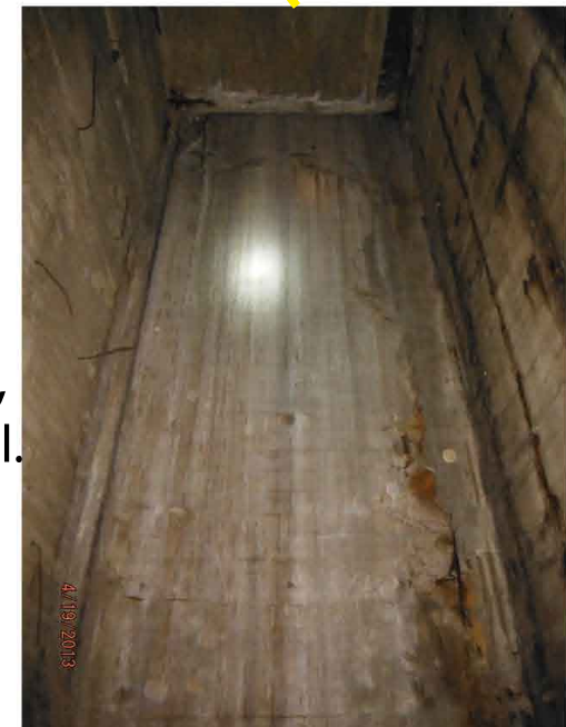
Large crack in wall behind Tower B
