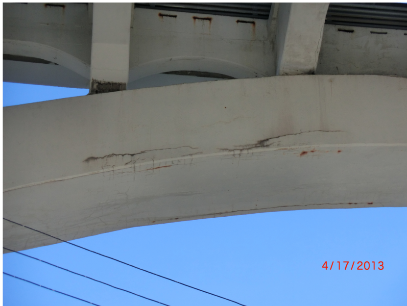
Delaminations to north arch in Span 7.
