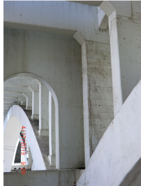
Typical delaminated arch column.
