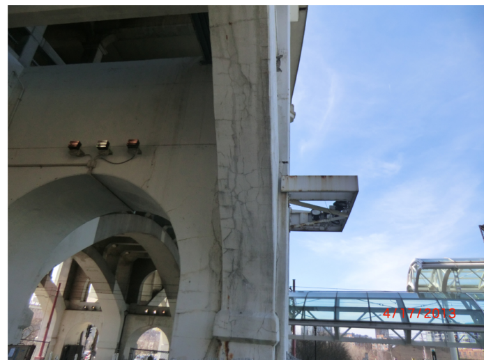
Map cracking in north arch Span 11.
