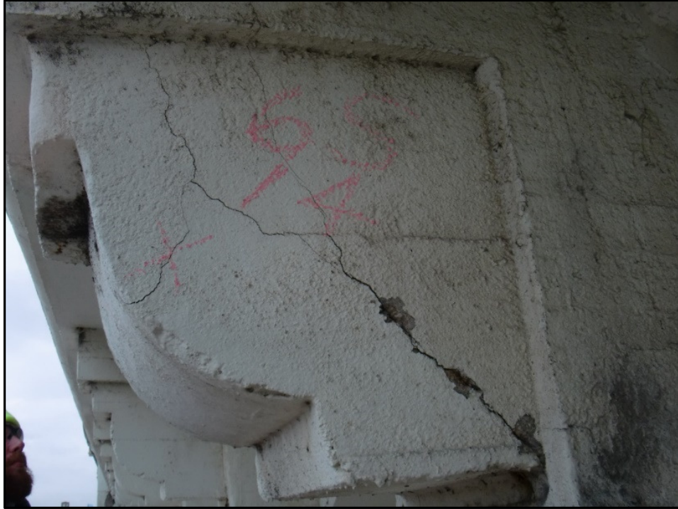
Photo 29 – Common Crack in Line of Primary Reinforcement, Lower Deck Corbel.
