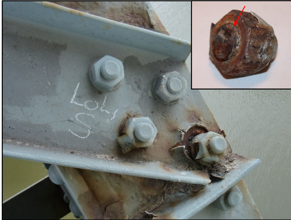
Photo 37 – Fractured Bolt, South L 0 L 1 . (Inset: Fracture Origin at Arrow.)
