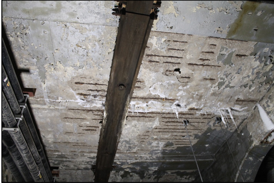
Photo 5 – Active Efflorescence, Water Infiltration & Rebar Corrosion, Panel D12, West Station.
