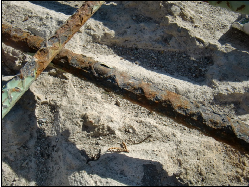
Photo 7 – 1/8-Inch Deep Section Loss of Epoxy Coated Rebar Following 18 years of Service.
