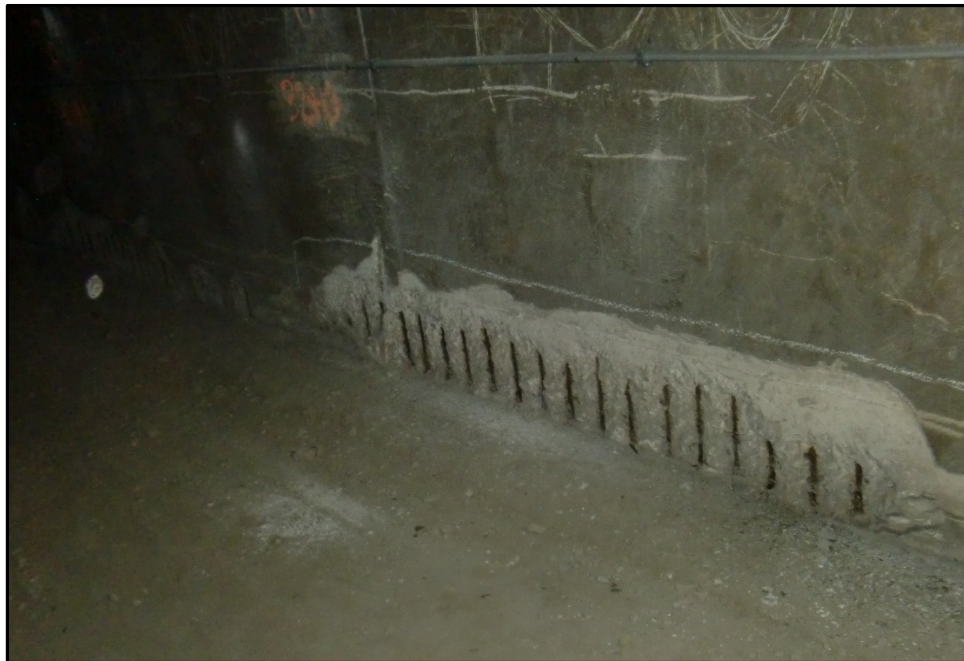
Photo 46 – Typical Wall Base Spalls, Detroit Ave. & West 25 th St. Tunnel.
