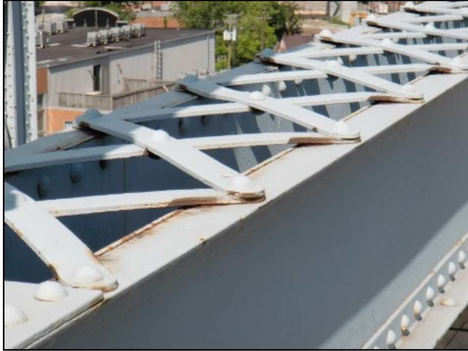
Photo 45 – Oxidized Top Coat & Light Rust Staining Above Upper Deck.
