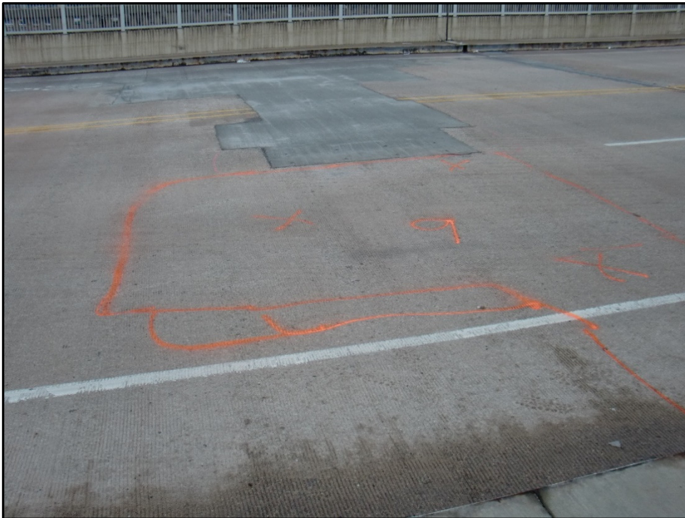
Photo 12 – Delaminated Wearing Surface Adjacent to November 2015 Repair, Span 9.
