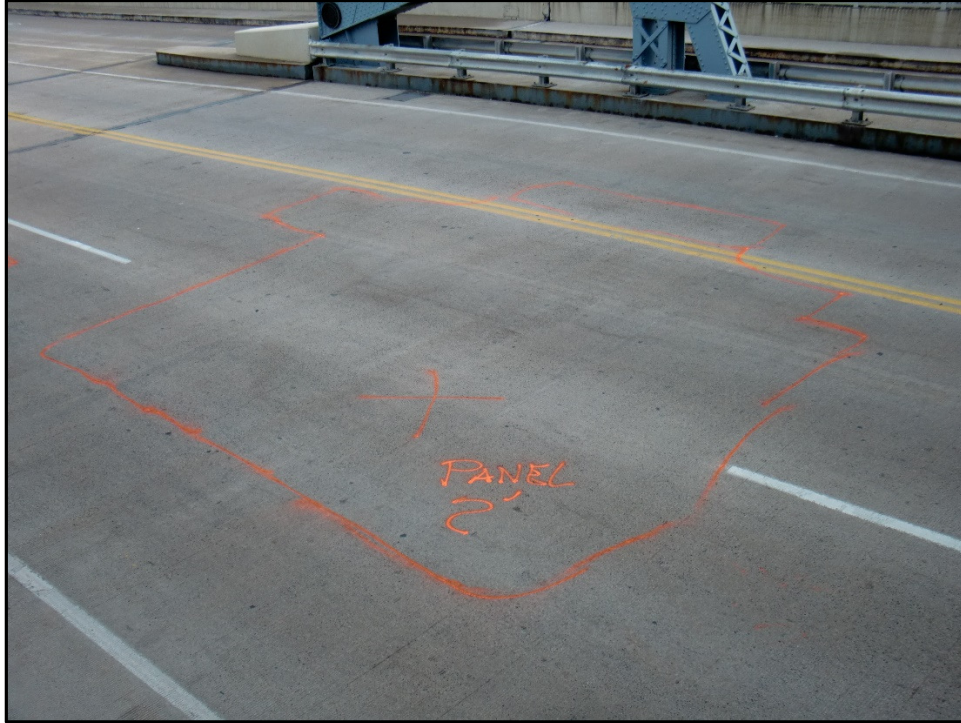
Photo 11 – Large Area of Delaminated Wearing Surface, Panel 2', Span 4.
