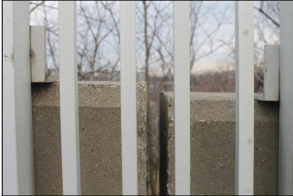
Photo 15 – Uneven Top of South Rail, Tower A.
