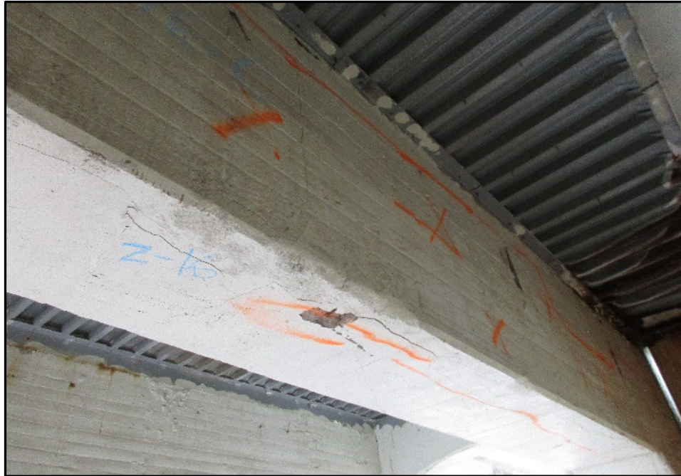
Photo 27 – Delaminated Surfaces of Lower Deck Floorbeam 16, Center Bay, Span 2.
