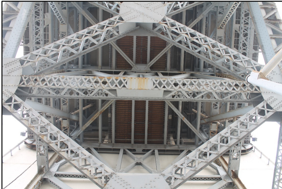
Photo 40 – Light Corrosion Stains, Lower Lateral Bracing.
