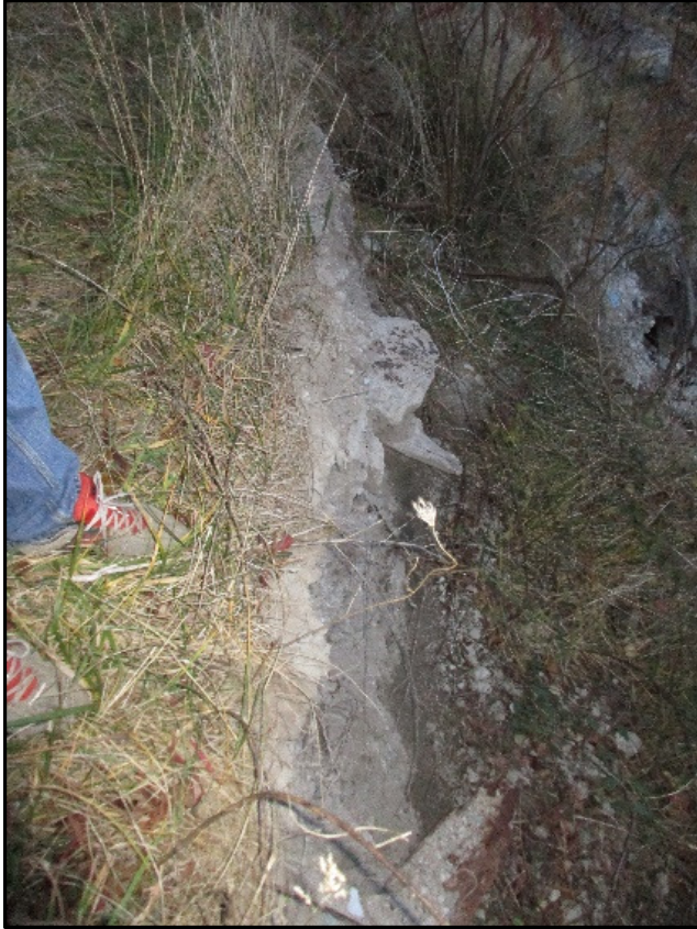
Photo 54 – Slope Settlement, Beneath Span 3.
