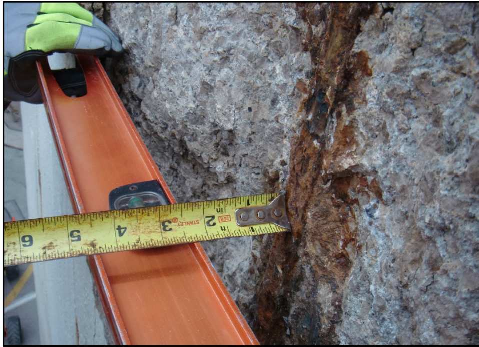
Photo 48 – Scaled Concrete & Rebar Corrosion, SE Lower Deck Shaft.
