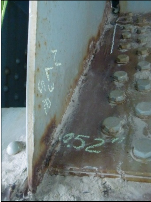
Photo 38 – 0.23" Deep Section Loss x 6" Long at Edge of Gusset Plate, North L 3 .
