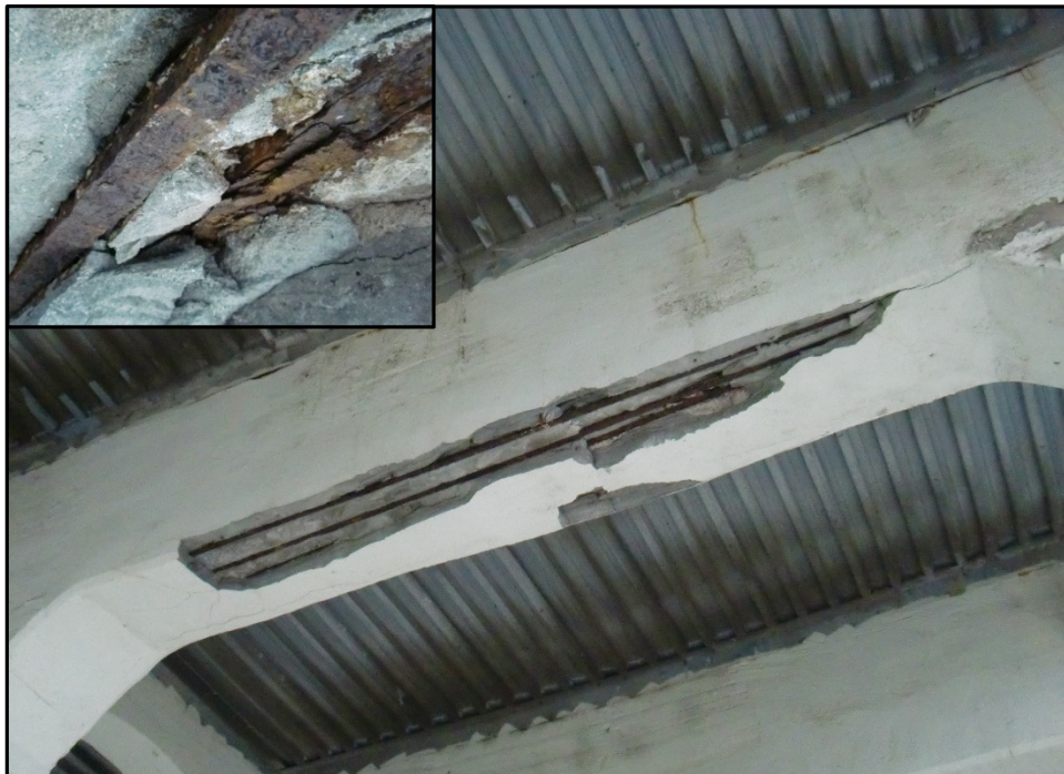
Photo 28 – Spalled 1996 Shotcrete Patch, Lower Deck Floor Beam 14, South Bay, Span 6. (Inset: Continued reinforcement corrosion at shotcrete patch/original concrete interface.)
