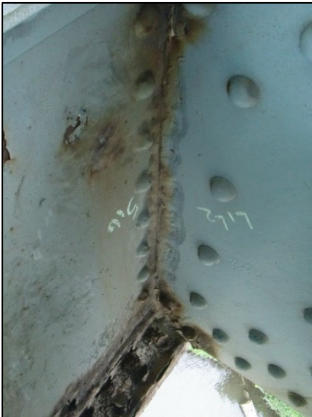
Photo 36 – Moderate Isolated Section Loss on Lower Chord Web Plate, Below Upper Deck.
