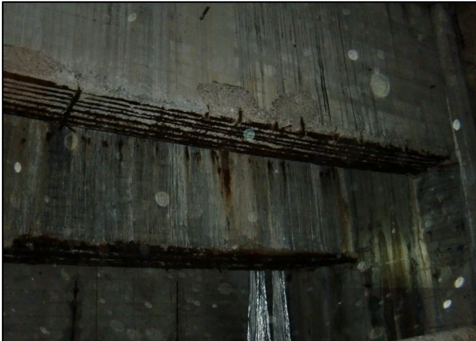
Photo 30 – Exposed Bottom Reinforcement Mat, Lower Deck Floorbeams 1 & 2, North Bay, East Station.
