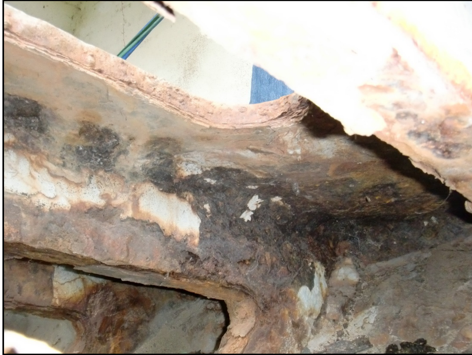
Photo 43 – Typical Corrosion Interior Surface of Bearing Casting.
