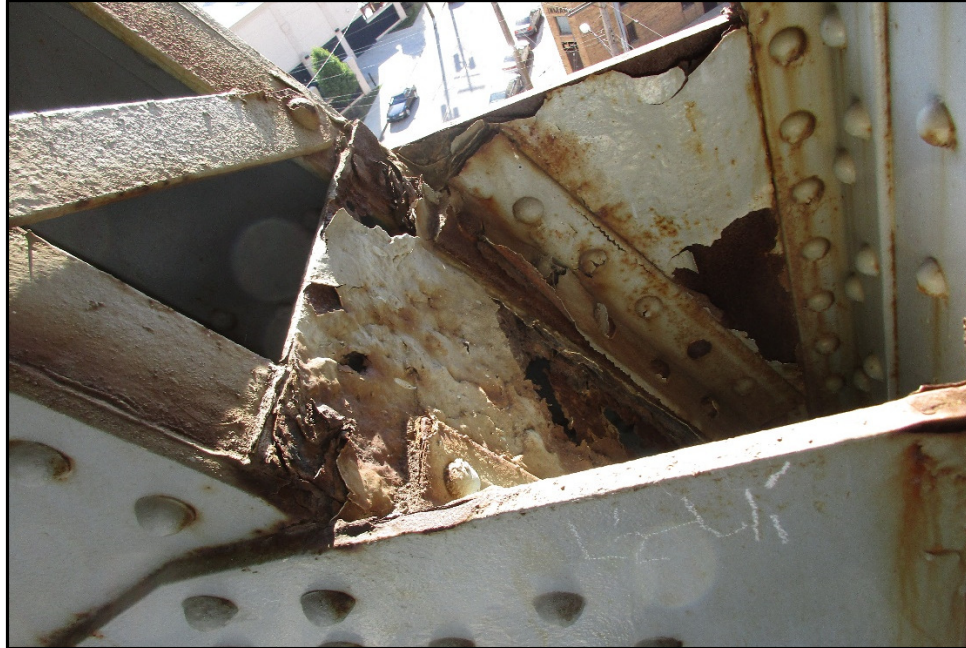
Photo 33 – Minor Pitting Top Stay Plate, U1'-L2' South.
