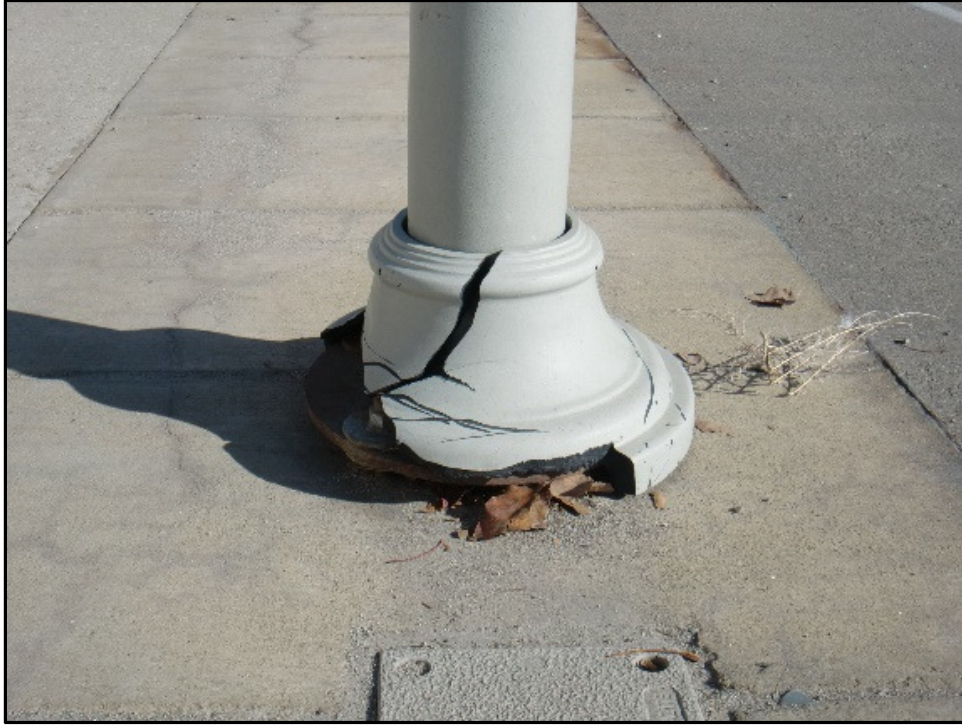
Photo 19 – Fractured Light Base, North Sidewalk.
