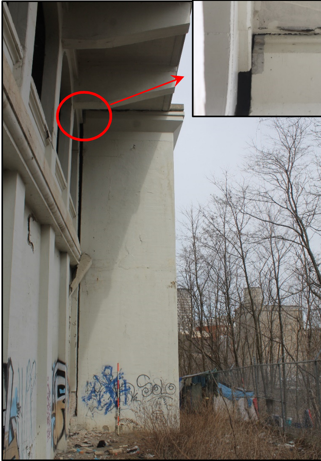
Photo 52 – Rotation of Tower B South (Inset: 6" rotation at top NW corner.)
