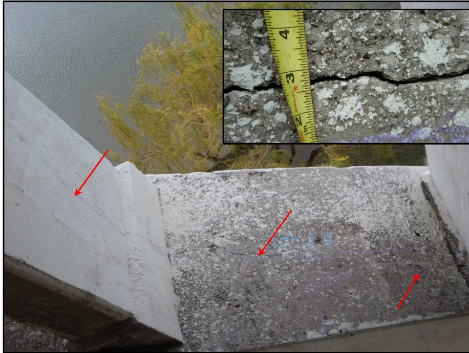
Photo 20 – Open Crack (at Arrows) on NE Arch Rib Extrados, Panel 14, Span 5.
