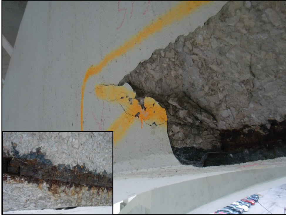
Photo 23 – Outline of Delaminated Arch Rib Corner, SI Arch Rib, Span 7. (Inset: Active rebar corrosion present.)
