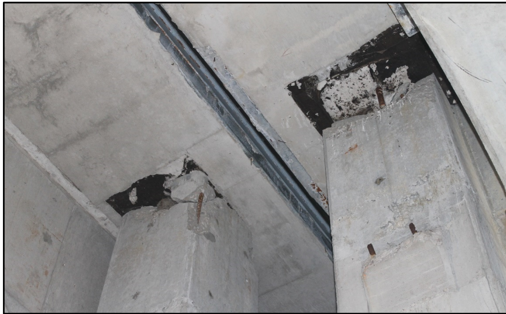
Photo 53 – Fracture of Top Interior Section Against Upper Deck Slab, Tower B South.
