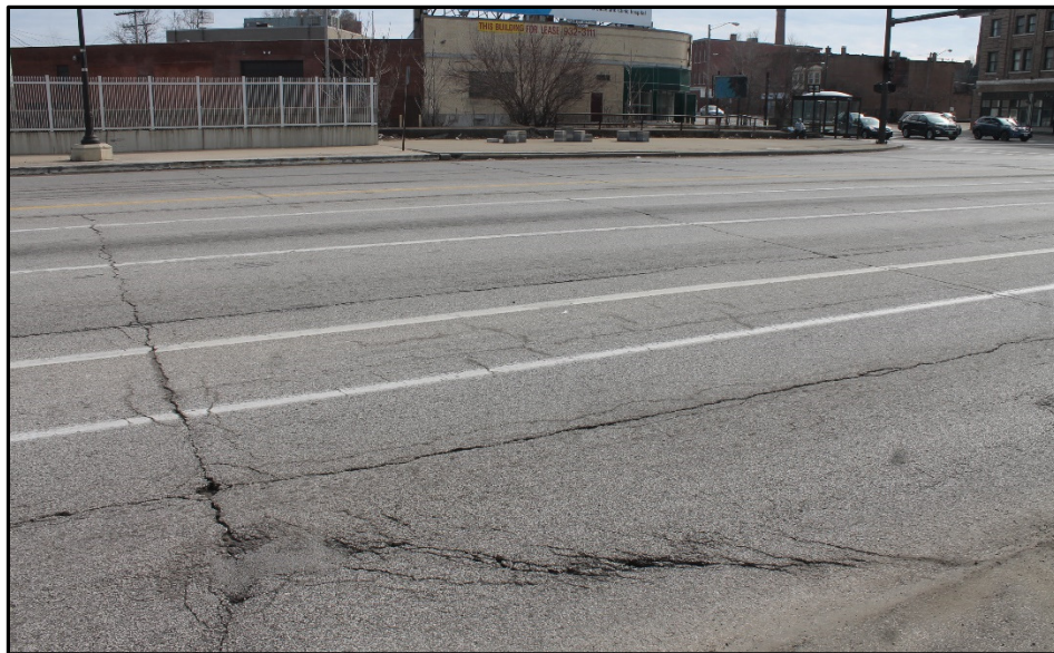
Photo 10 - Cracked Asphalt Wearing Surface, West Station.
