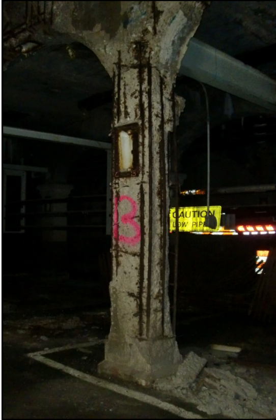
Photo 51 – Advanced Concrete Corrosion, Column C13, West Station.
