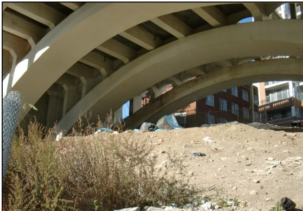
Photo 58 – Homeless Tents Within Intended Span 1 Secure Zone.
