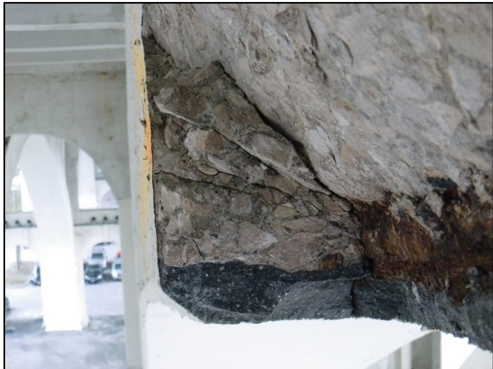
Photo 24 – Sound 1996 Shotcrete Patch & Fractured Original Concrete, SI Arch Rib, Span 7.
