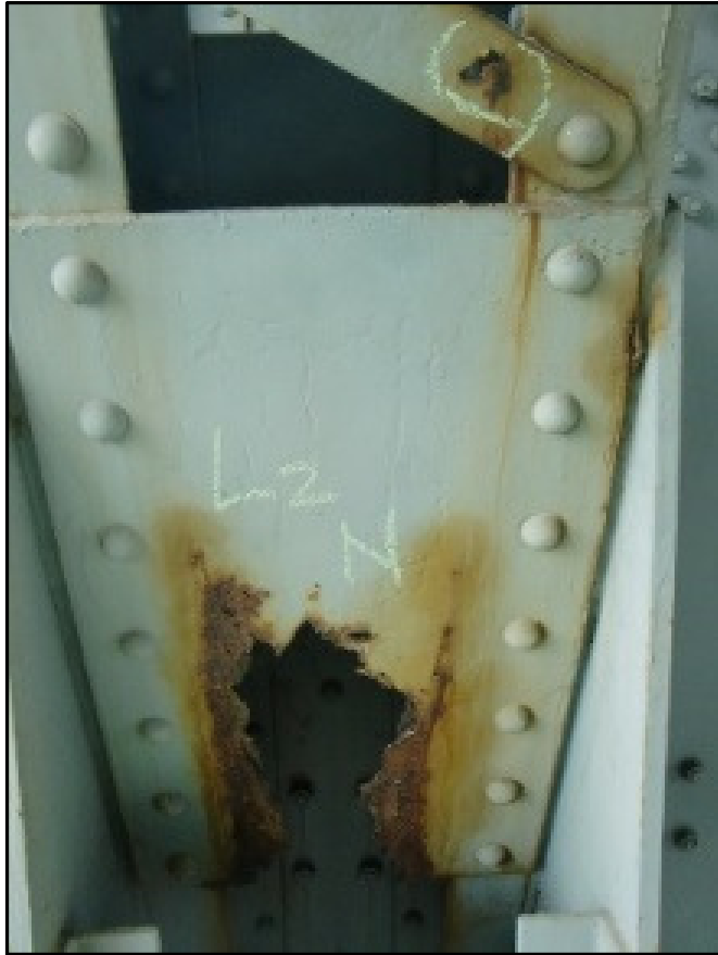
Photo 41 – Perforation of Sway Brace Stay Plate & Lacing Bar, North L 2 .
