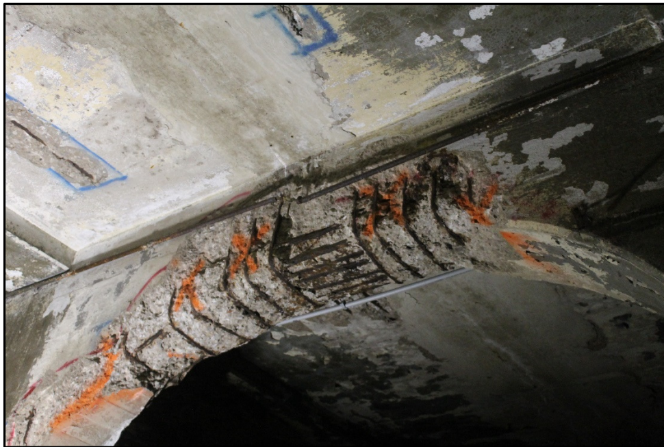
Photo 31 – Spalled Beam D22, West Station.
