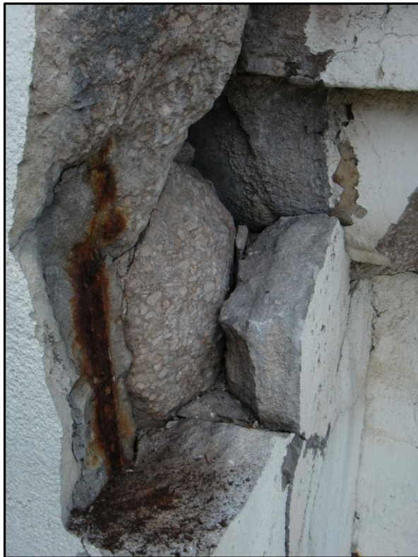
Photo 49 – Deeply Cracked East Face of South Exterior Lower Deck Shaft, Pier 5 at Lower Deck Corbel.
