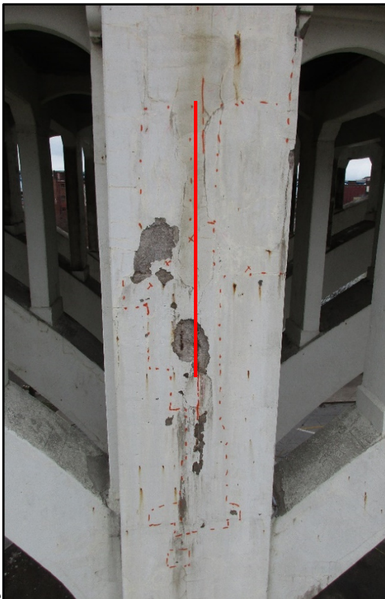
Photo 47 – Scaled Concrete Core, SE Lower Deck Shaft, Outlined in Dotted Paint. (Note: Original encased drain pipe is located behind red line.)
