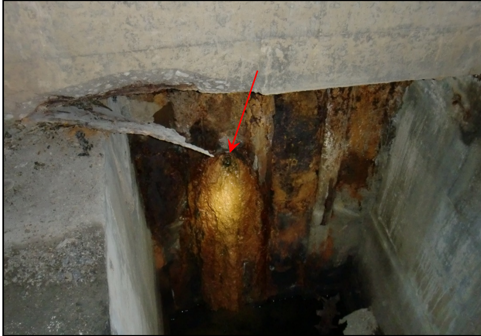
Photo 45 – Possible Deposit Clogged Pedestrian Tunnel Drain Outlet (at Arrow), East Abutment Cellular Construction.
