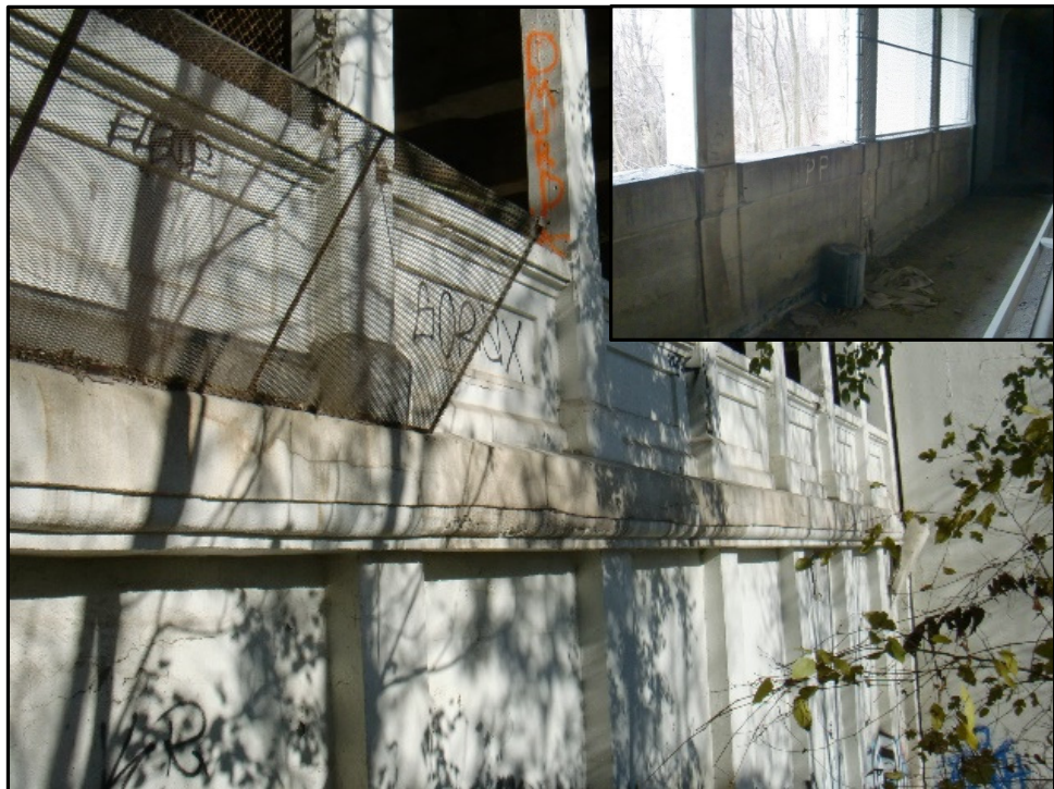
Photo 56 – Continuation of Unauthorized Access to Span 1A Lower Deck. (Inset: Trash can used to exit lower deck.)
