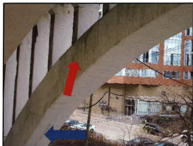
Photo B1 – Panels 1-4.
