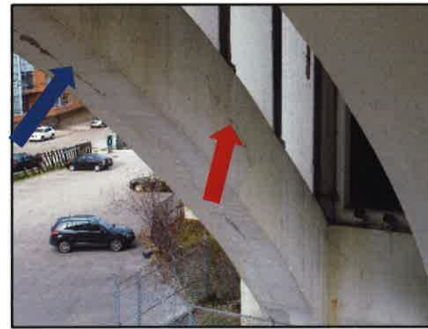
Photo B8 – Panels 16-18.
