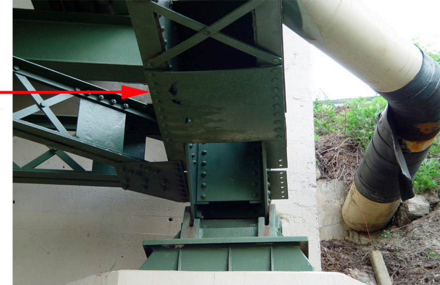
PHOTOS SHOW RUSTED THRU HOLES TO LOWER GUSSET PLATE OF TRUSS #4 (SOUTH).
