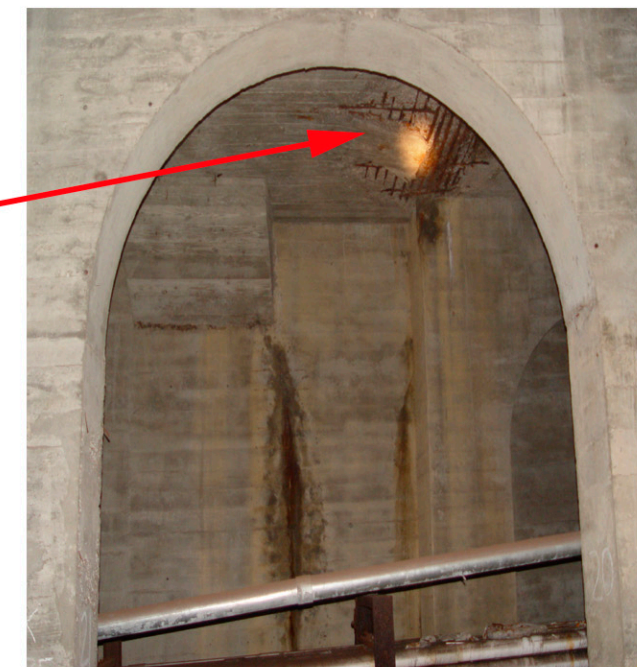
PHOTO SHOWS A SPALL FORMING OVER UTILITY CONDUIT INSIDE FINISH (EAST) ABUTMENT CELLULAR CONSTRUCTION. THIS IS APPROXIMATELY 75' WEST OF EAST CELLULAR ABUTMENT WALL.
