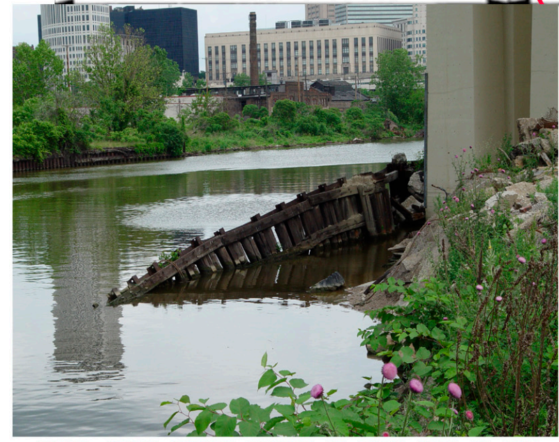
PHOTO SHOWS DAMAGED FENDER TO EAST SIDE OF THE RIVER.
