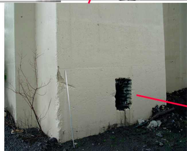
PHOTO SHOWS A DRILLED OUT HOLE AT BASE OF START (WEST) SIDE OF LEFT (NORTH) COLUMN. HOLE IS 19" W BY 22" H.
