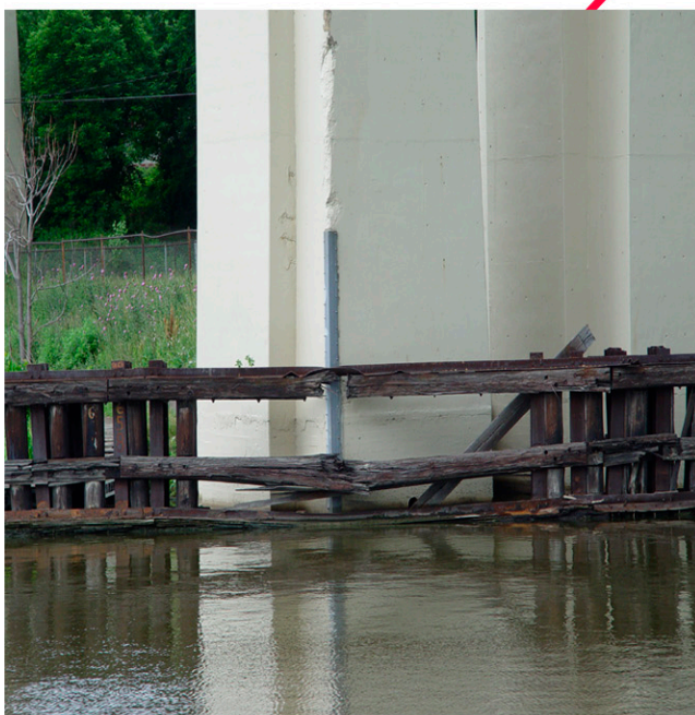
PHOTO SHOWS DAMAGED FENDER TO THE WEST SIDE OF THE RIVER.
