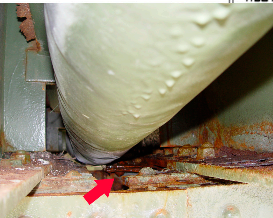
RED ARROW SHOWS WATER LEAKING ONTO STEEL FROM LEFT (SOUTH) TRUSS EXPANSION JOINT TROUGH.
