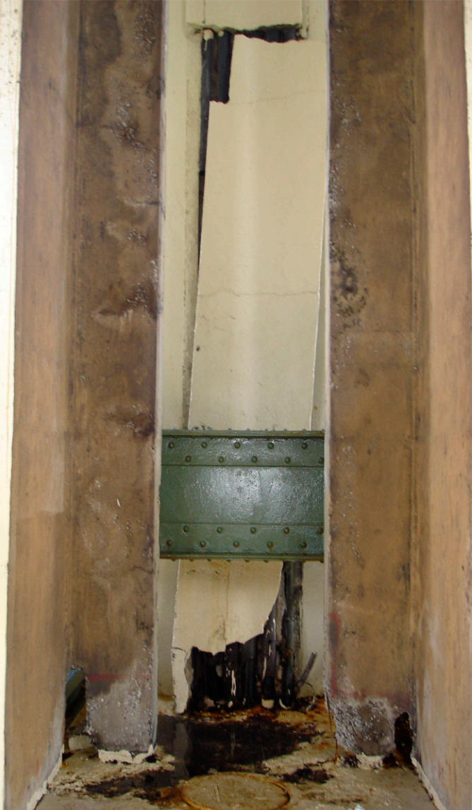
PHOTO SHOWS SOUTH FACE OF THE RIGHT (NORTH) ARCHITECTURAL PILASTER, ELECTRICAL CONDUIT RUNS THRU HERE. NOTE THE CONCRETE ENCASUREMENT HAS SHEARED OFF AND IS WEDGED BETWEEN PILASTER AND LOWER CORD STRUT.
