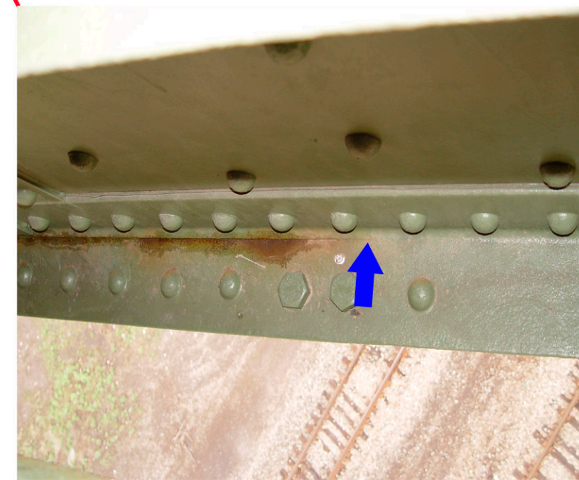
BLUE ARROW SHOWS END OF CRACK. THIS IS LOCATED TO TRUSS #3 (SOUTH MIDDLE). CRACK WAS MARKED IN THE FIELD.
