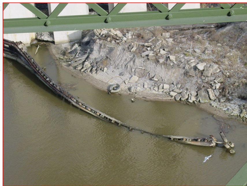
Collapsed (failed) timber fenders in river.
