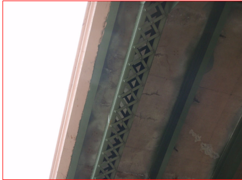
Leakage through deck under south sidewalk (visible in wet spots).
