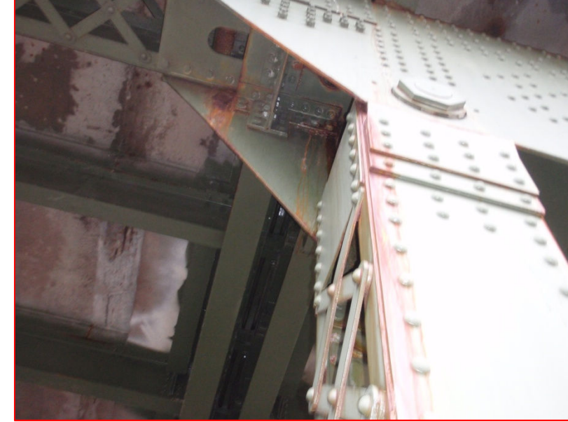
Efflorescence, rust staining on the outside of the new paint in areas below the joints that are leaking (typical at all joints).
