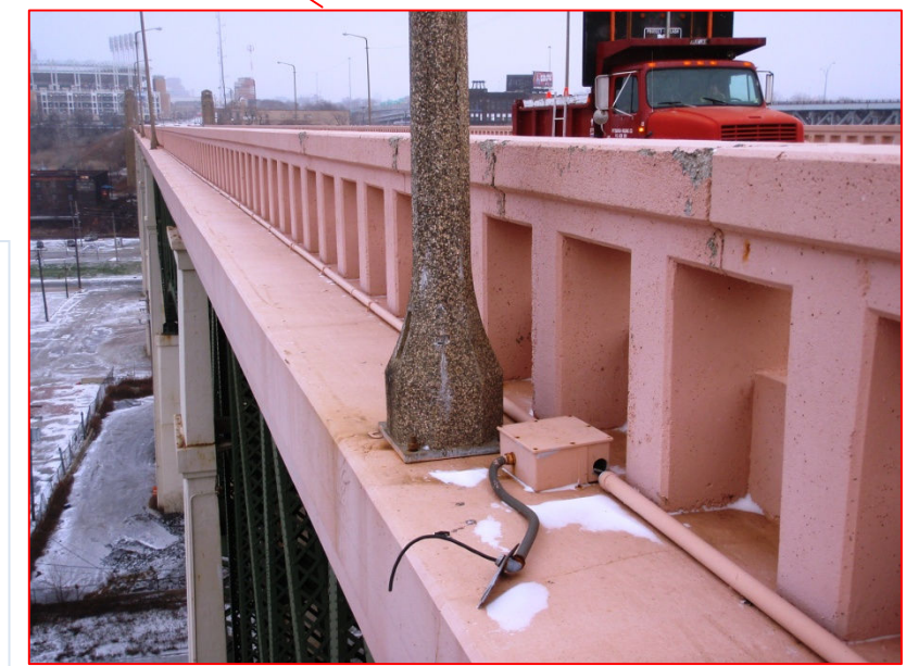
Precast concrete light pole is cracked, cover for hand access hole is missing, (typical of multiple locations).
