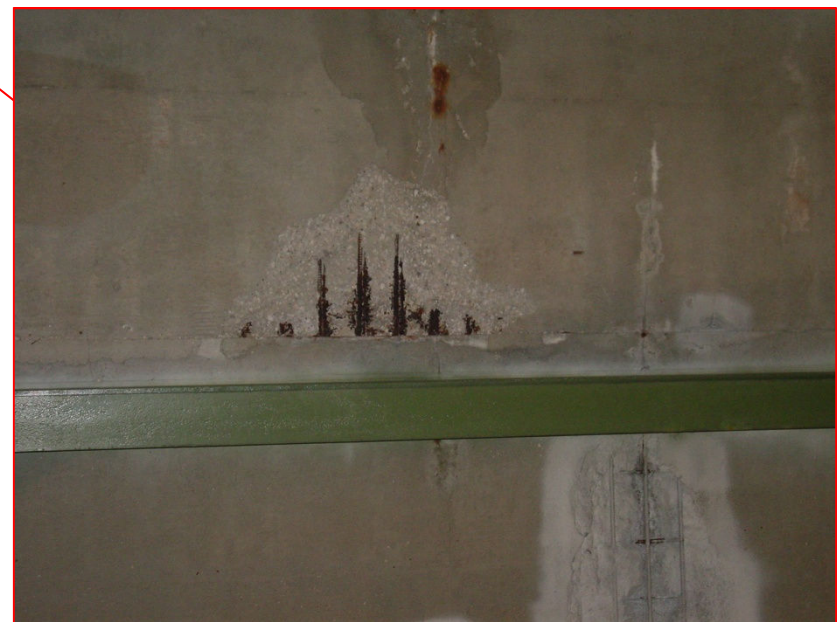
Spall, 6'x3', in underside of deck, span 11 between U7 and U8.
