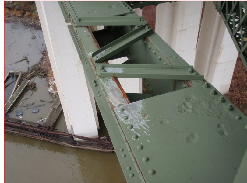
Efflorescence on lower chord and new corrosion (rust staining) directly below leaking areas in the south sidewalk.
