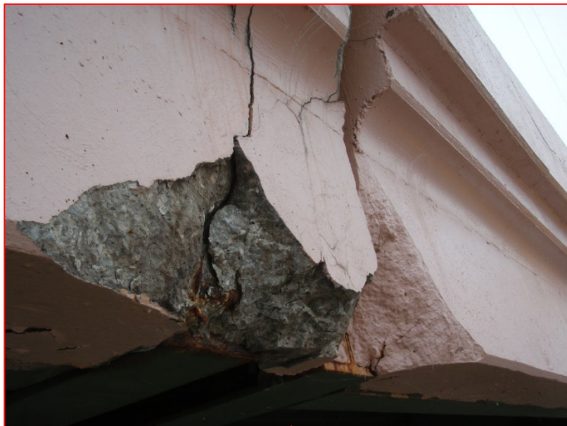
Spalling at top of decorative details over piers, exterior faces.
