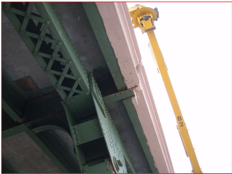
Leakage through joints at the ends, visible here in the form of icicles – typical all expansion joints.
