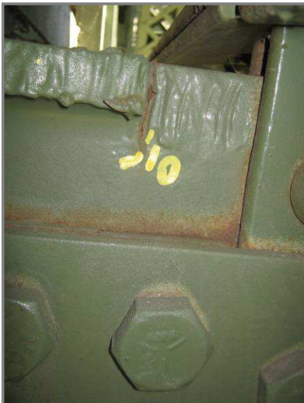
Photo 16– Crack in web of FB37 at CL37.
