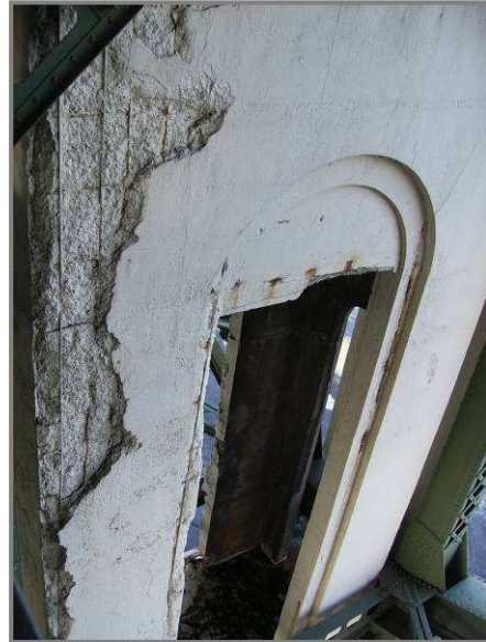
Photo 56– Typical spall with exposed rebar pier tower.
