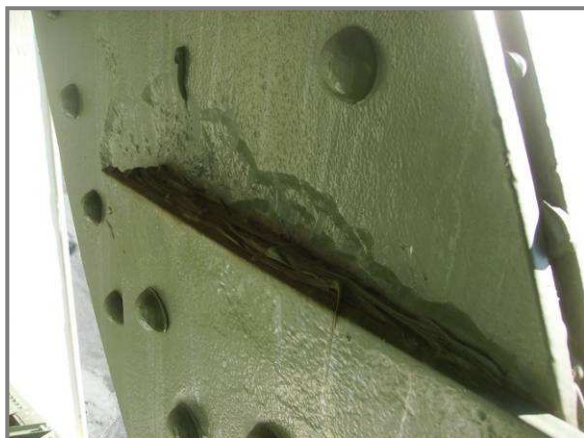
Photo 22 – Pitting up to 1/4" on the north web of member DL43-DU44 at interface with DL43 gusset plate. Note impacted rust present.
