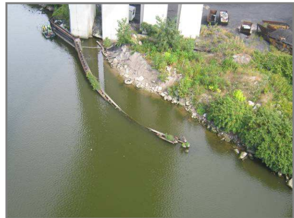
Photo 61– South half of the east bank fender system collapsed towards river centerline.
