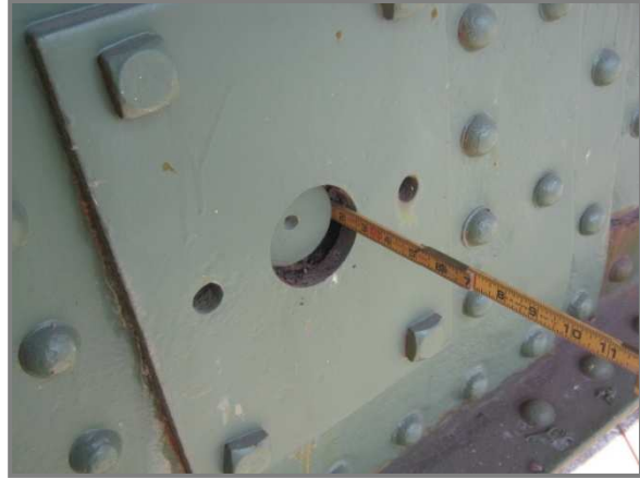
Photo 52 – Sliding pin at CL12S not fully bearing on the outermost pin plate due to impacted rust between the web plate and gusset plate.
