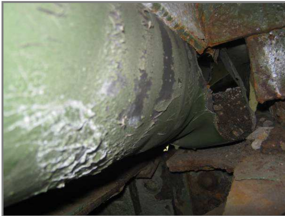
Photo 9 – Isolated torn neoprene trough with debris spilling onto roadway framing members adjacent to Panel Point DU35.
