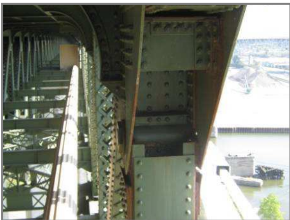
Photo 50– Active minor surface corrosion at DU12.
