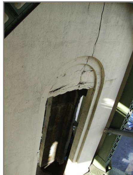
Photo 59– Vertical crack in Pier 13 north tower section.
