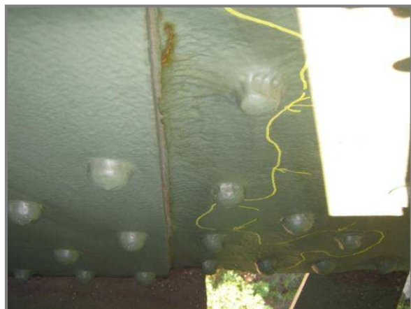
Photo 31 – DL7-DL8 1/4" pitting over full height of south web at DL8.
