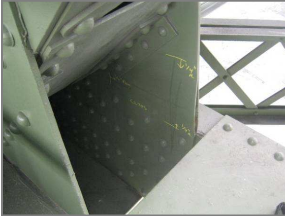
Photo 40 – Bounds (marked by yellow paint stick) of lamellar tear at CL70S (west end of plate).
