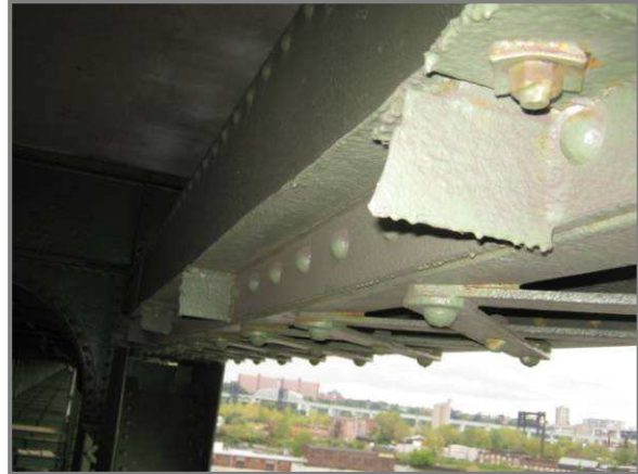
Photo 28 – Abandoned platform connection to the top chord member AU120-AU121 with typical field welds.
