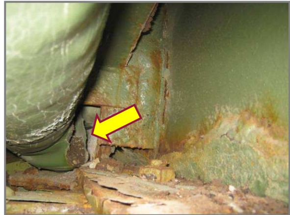
Photo 8 – Isolated torn gland with debris spilling onto roadway framing members adjacent to Panel Point DU35.
