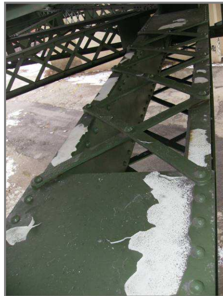
Photo 51– Isolated peeling paint in Span 21.
