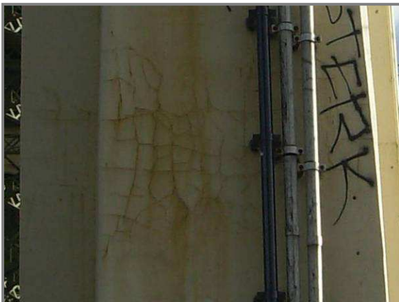
Photo 58– Isolated patch of map cracking on pier wall with rust staining.
