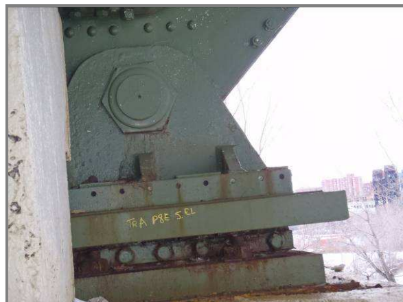
Photo 47– Roller nest assembly at AL21 with active surface corrosion present.
