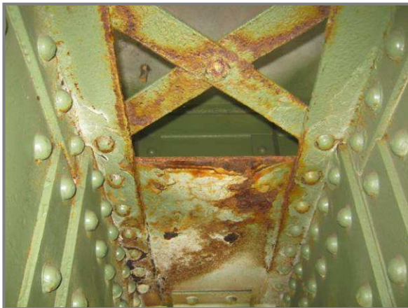
Photo 26 – Active surface corrosion to lacing bars and batten plate beneath area of leaking deck at AU120.
