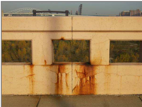
Photo 6 – Typical parapet hairline cracks with rust staining.
