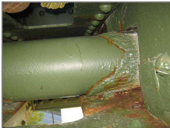
Photo 54– Sliding pin at AL17 seized due to impacted rust which has been painted over.
