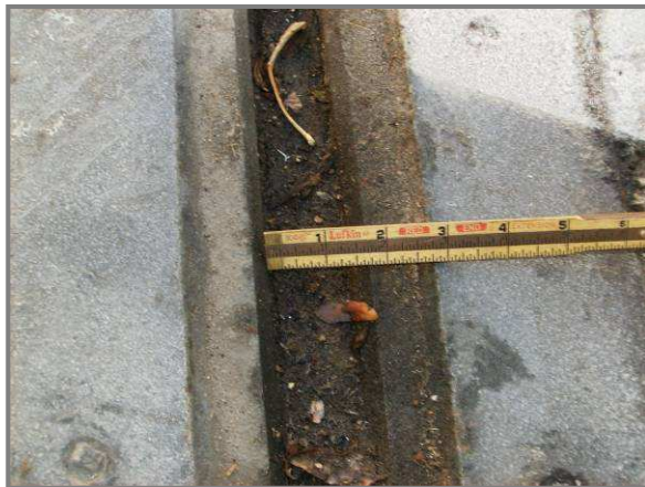
Photo 10 – Typical granular debris buildup in Joint 0 at West Abutment.
