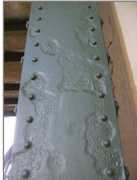
Photo 18 – BL0-BU0 1/8" pitting with isolated 1/4" pitting over the lower half of the north web plate.
