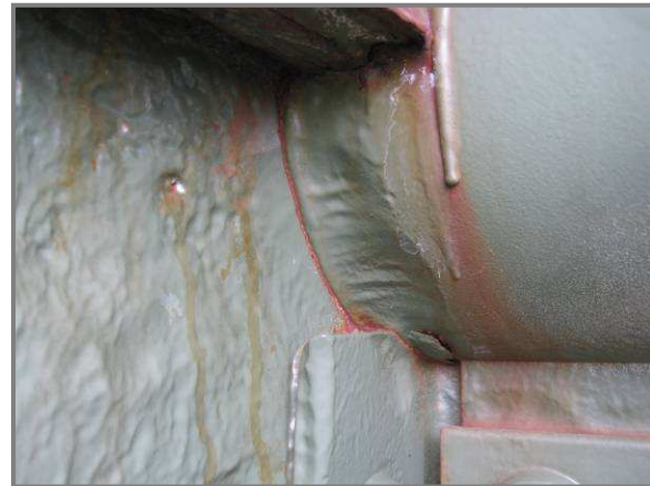
Photo 53– Wear along vertical pin at AL12 up to 5/16" loss over the lower half of the pin circumference.
