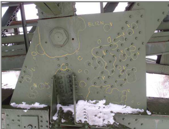
Photo 38 – Up to 1/4" pitting (highlighted in yellow) at gusset plate (BL12N). Note pitting around pin and chord members.
