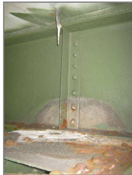
Photo 2 – Isolated location exhibiting a stalactite formation dripping onto Truss D at Panel Point DU47.
