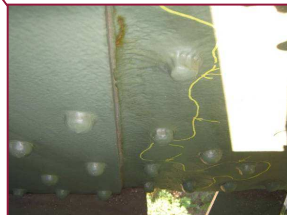
Pitting up to 5/16" deep was noted over the full height of the north web plate of DL7-DL8 adjacent to DL7.
