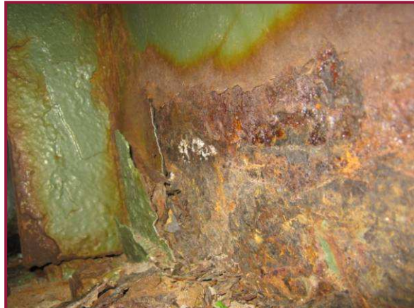
Active heavy corrosion with 1/16" pitting on the bottom flange and lower 1/3 of the web of Floorbeam 0, adjacent to a failed deck joint.
