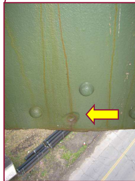
The north web plate of AL26-AL27 exhibits isolated advanced loss of section with a 2" diameter perforation within the bounds of the vertical leg of the bottom flange.
