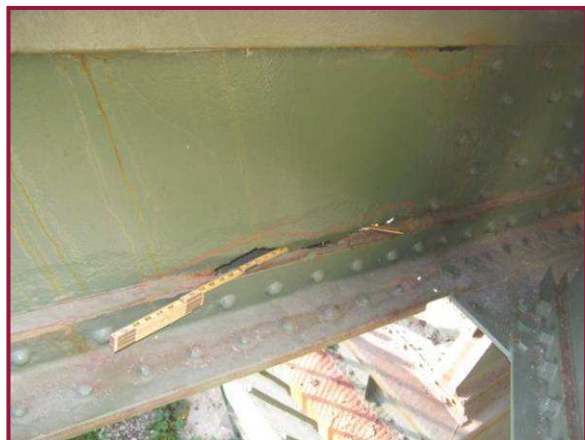
DL0-DL1 exhibits a 2'L x 3"H hole in the north web plate near the bottom flange angle and a 6"L x 2"H hole adjacent to the top flange angle, 5' from DL0.
