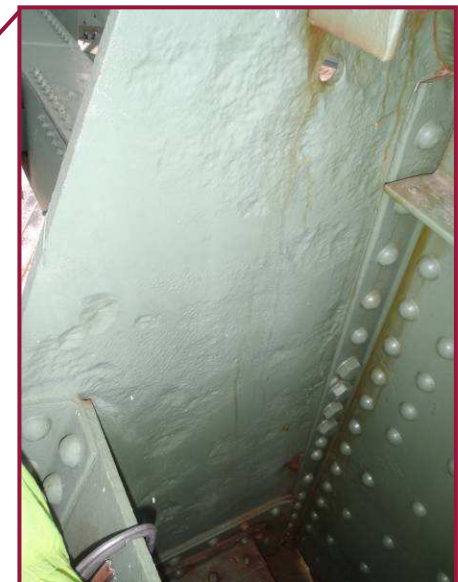
The north face of the south gusset plate exhibits isolated areas of pitting up to 1/4" deep.
