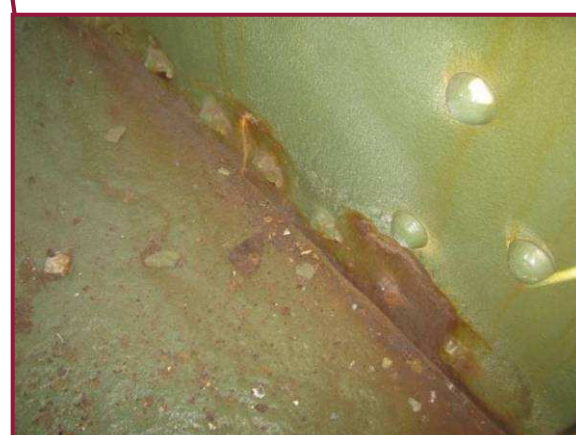
DL12-DL13 exhibits moderate corrosion and pitting up to 1/4" deep over the lower 1/3 of north web plate, with a 2" Ø hole near the bottom cover plate interface.
