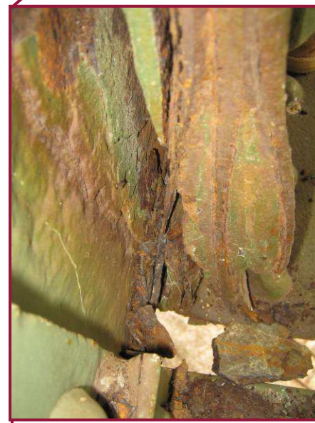
CL12-CL13 exhibits advanced section loss and heavy pack rust at the sliding pin location at CL12. A thin internal fill plate has rusted away at this location, and built up member connections are becoming distressed due to the pack rust and subsequent distortion of the web members, as shown.
