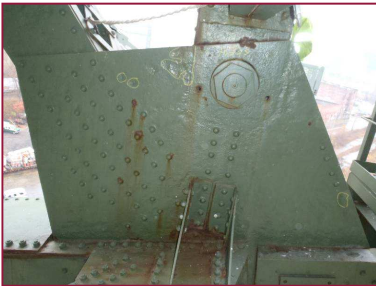
AL35S exhibits heavy pitting throughout the south face of the plate, with 1/4" losses in isolated areas.
