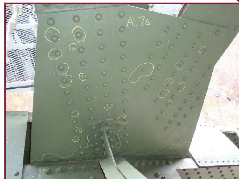
Small areas of pitting 1/4" deep pitting are scattered throughout the south face of AL7S, as indicated with field markings.
