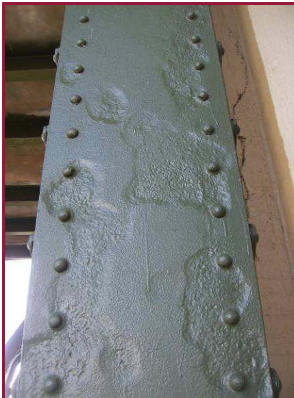
The north web plate of BL0-BU0 exhibits 1/8" to 1/4" deep pitting (see Section A-A).
