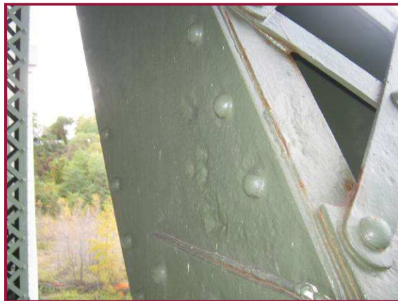
The south web plate of AL23-AU22 exhibits pitting up to 3/16" deep along the gusset plate interface.
