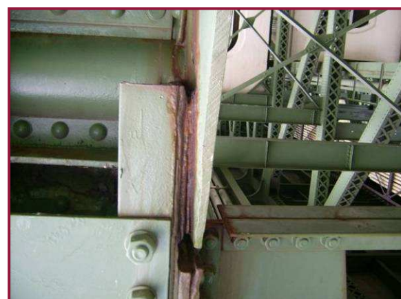
Active pack rust between the north gusset plate and vertical member angle at DL12
