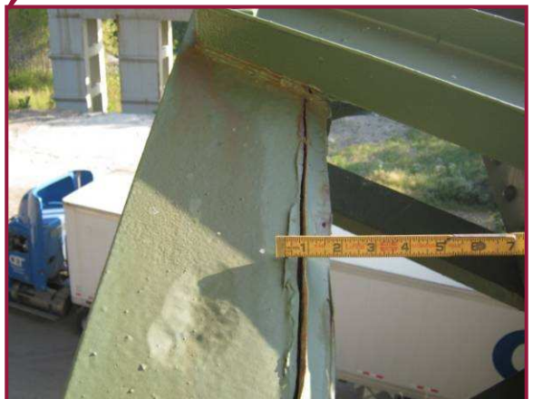
Typical evidence of pack rust reactivating between top flange angle and web plate (DL1-DL2 shown).
