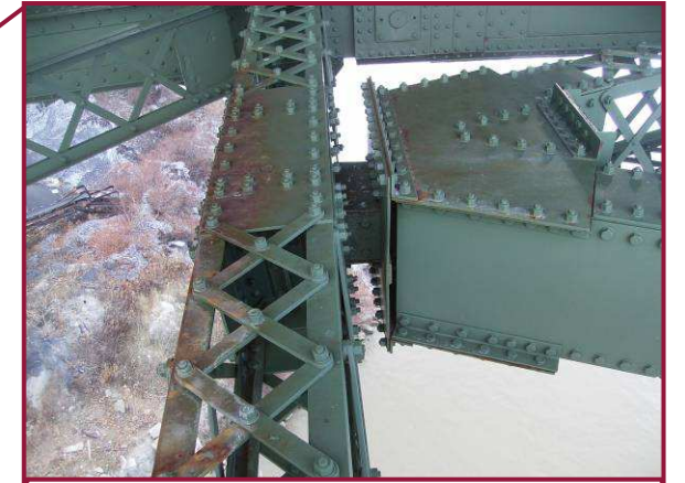
The built up strut at AL41 exhibit active surface corrosion throughout.
