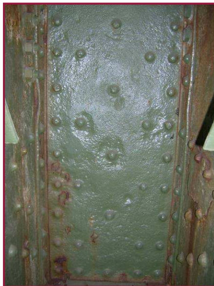
The internal diaphragm plate at CL12 exhibits heavy pitting around the rivet heads and along the edge of the plate at the gusset plate interfaces. Note the active rust throughout.
