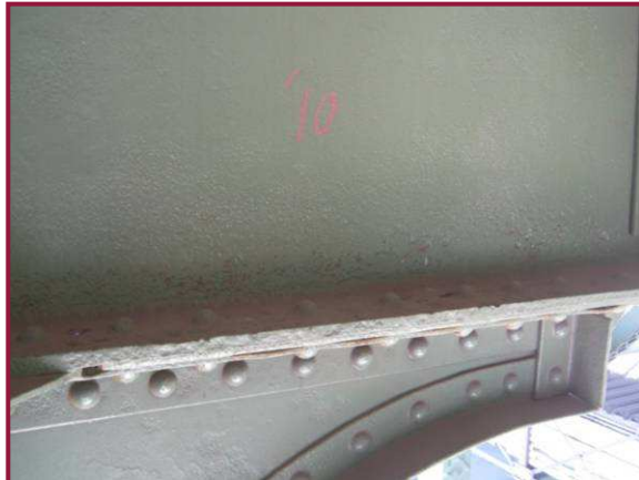
Floorbeams in Span 7 typically exhibit 1/16" pitting with isolated 1/4" pitting on the web and flanges between Truss D and Stringer 2 (first interior stringer) (Floorbeam at DU18 shown).
