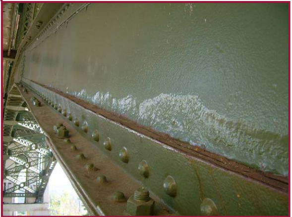
The north web plate of CL0-CL1 exhibits 6" tall, 1/4" pitting throughout the bottom half of the web.
