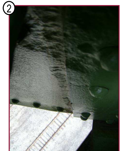
Up to 1/4" pitting (cleaned and painted) extends the full height of the north web of DL14-DL15 adjacent to DL15. This condition is typical for Span 7 lower chord members.
