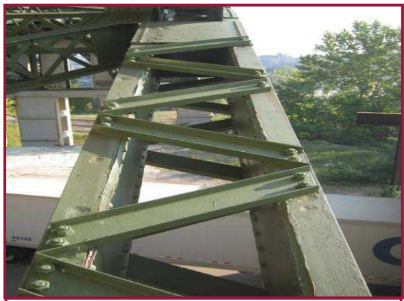
Bottom chord members in Span 6 typically exhibit localized 1/4" pitting (cleaned and painted) on the top flange angles and cover plates (DL1-DL2 shown).
