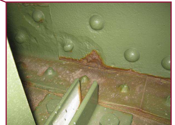
The south web splice plate at AL27 exhibits 1/4" pitting with reactivating rust along the lower flange. Additionally, the adjacent bottom flange exhibits pitting up to 1/4" deep and the rivet heads connecting the lateral bracing connection plate exhibit significant loss of section.
