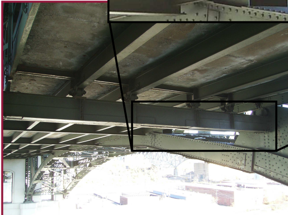
The utility deck Floorbeam 78 has received extensive web retrofits throughout the length of the member.
