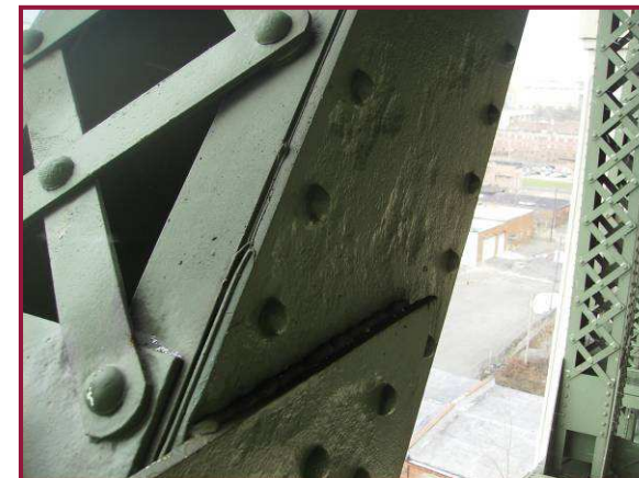
Heavy pitting is present along the web of AL73-AU74 at the lower gusset plate interface (Section A-A).
