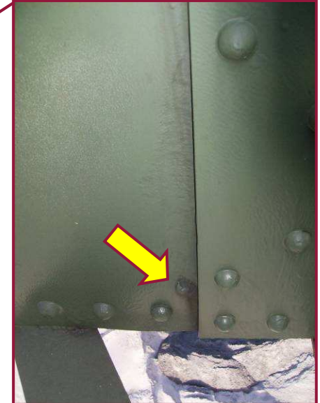
Adjacent to the north gusset and above the bounds of the lower flange angle, the lower chord web plate at DL72 is perforated by a 1" diameter hole.
