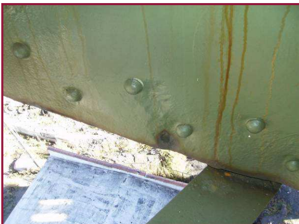
The south web plate of BL77-BL78 near BL78 is perforated, exhibiting a 2" diameter hole opposite the bottom flange angle. Adjacent 1/4" deep pitting is present at this location.
