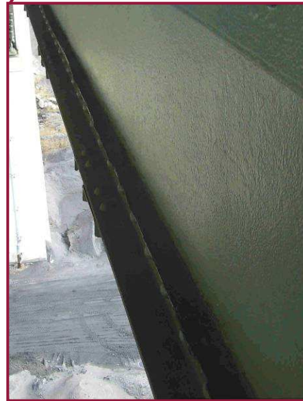
The lower chord member DL69-DL70 exhibits pack rust up to 2" thick between the north web plate and the lower flange angle. Pitting up to 3/16" was noted on the north web plate along the flange angle.
