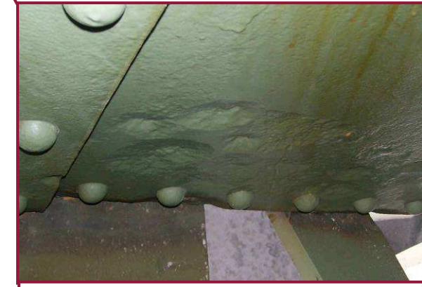
The lower half of the interior face of the DL64-DL65 north web plate exhibits pitting up to 5/16" deep adjacent to the DL64 gusset plate. This condition is typical for Truss D lower chord web plates at the panel interfaces throughout Span 11; however, pitting varies from 1/8" to the 5/16" depth at DL64.
