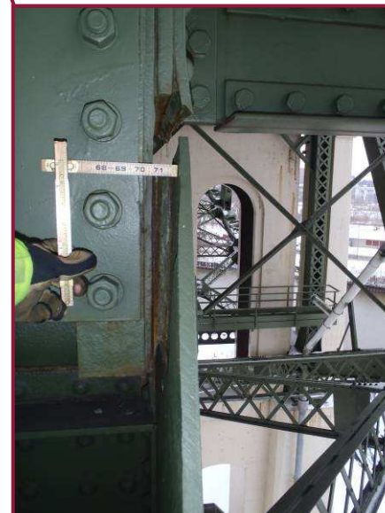
Pack rust up to 1.25" has formed between the north gusset plate and the vertical member near the lower vertical pin at BL58.
