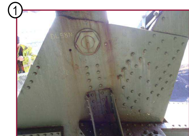
The north gusset plate at DL58 exhibits up to 3/16" pitting, a condition typically found at the expansion locations throughout the structure.
