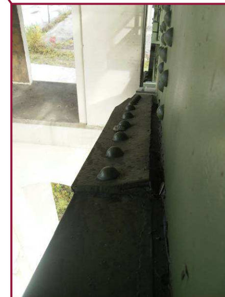
The top flange splice plate at CL74S is distorted due to pack rust.
