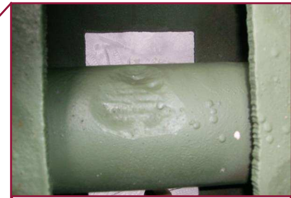
The lower sliding pin at DL63 has a 4" diameter area exhibiting up to 5/16" deep pitting. This location has been cleaned and painted with no active rusting.
