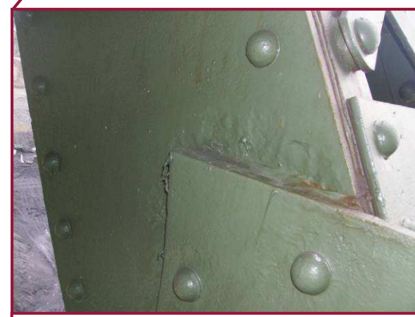
Pitting of the north web plate at the gusset plate interface on diagonal member DL64-UL65 is up to 3/16" deep with light surface corrosion along the seam between the two plates. This condition is typical for Span 11, Truss D for other web members. Only member DL59-UL58 in Span 11 exhibited heavier pitting at this interface, with up to 5/16" loss.
