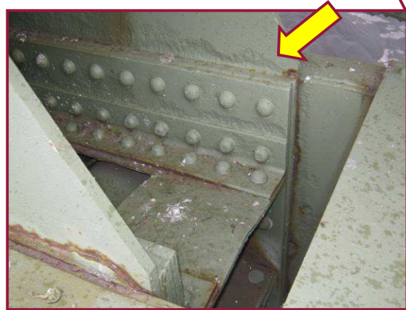
Active rusting is typical along the seams of the built up members at DL58. The south face of the north gusset plate exhibits 1/8" pitting that has been cleaned and painted, while the same location on the south gusset plate exhibits up to 1/4" loss (arrow). Additionally, note that the horizontal stiffener plate between the two gussets is bowed up, measuring approximately 1" from its original plane.
