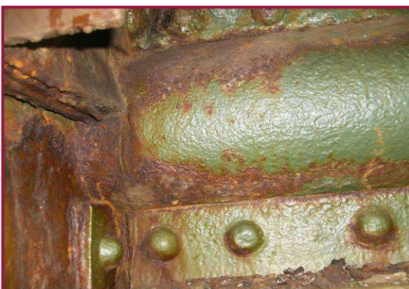
At the main bearing pin at vertical member DL58-UL58, surface rust is typical throughout with light to moderate pitting of adjacent components. Note: this condition is common among the truss pins, especially those below failed deck joints.
