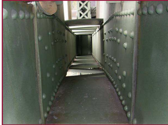
Pack rust between the gusset plates and web plates at DL67 has caused 1/2" bowing of the gusset plates.
