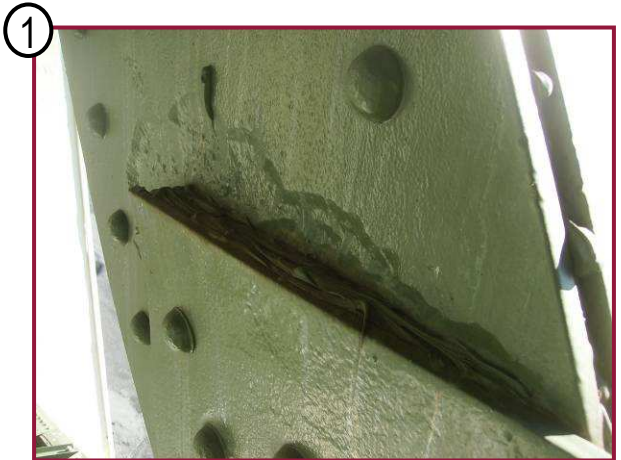
Member DL50-DU51 exhibits pitting of the north web plate at the interface with the lower gusset plate. Pitting at this location averages between 1/8" to 1/4" deep for the width of the plate.
