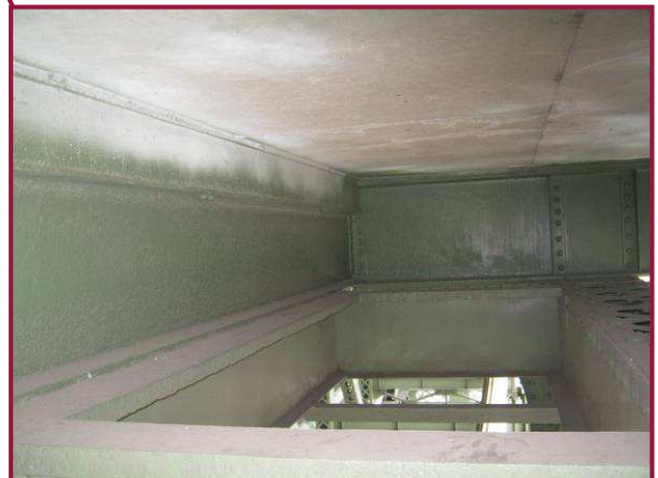
Between Floorbeams 53 and 54 an appurtenance (platform) is stitch welded to Stringer 1 and the interior face of the upper chord of Truss D.
