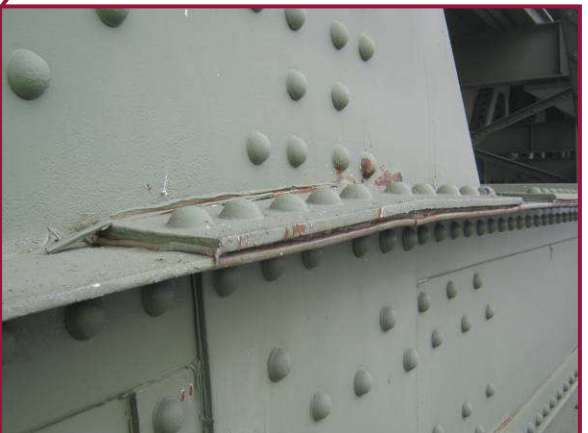
At the flange splice plate at panel DL49, 1/2" thick pack rust has developed and is deforming the flange angles. Reactivating pack rust at this detail is typical of lower chord splices throughout Span 10.
