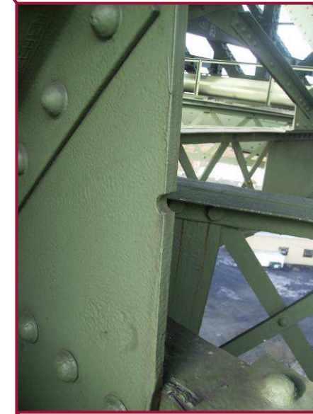
Both gusset plates at DL71 have misplaced drill/punch holes along the east free edge.
