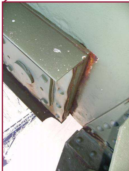
The north gusset plate at BL58 shows signs of abrasion with the lower chord at the sliding pin location, indicating movement of the suspended span. Note also the swelling of the pin plates between rivets on the lower chord member.
