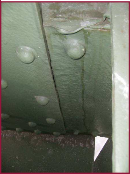
DL50-DL51 exhibits up to 1/4" deep pitting over the full height of the north web at DL50. 1/8" pitting is typically found at similar locations throughout the lower panels in Span 10.
