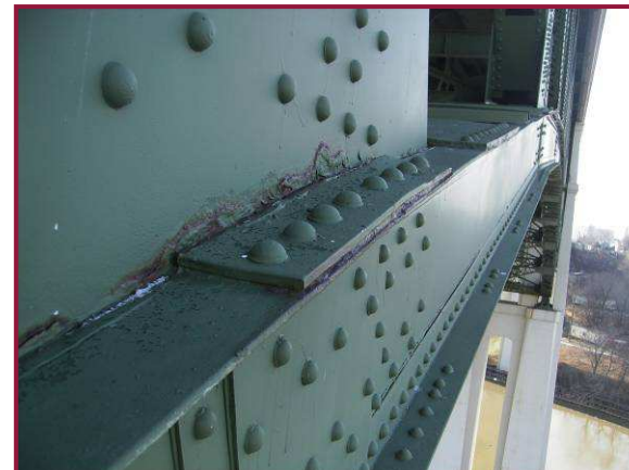
The top flange splice at AL53 exhibits minor distortion due to pack rust forming. Note the adjacent active rust on the gusset plate.
