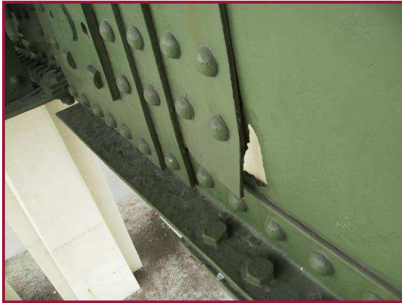
Corrosion has produced a 5"x 4" hole in the south web plate of CL113-CL114 at the bottom corner of the innermost pin plate.
