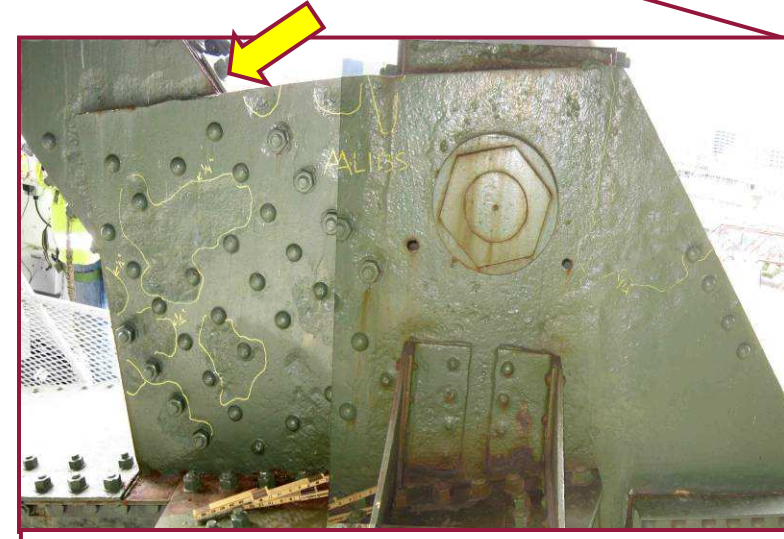
The south face of the south gusset plate at AL113 exhibits widespread heavy losses. The areas highlighted on the plate in yellow exhibit pitting of 1/4" deep or greater. The interior face of the south plate exhibits isolated areas with up to 1/4" loss. Additionally, note the 1/4" deep pitting along the full height of the web of the diagonal member AU112-AL113 near the gusset plate interface.
