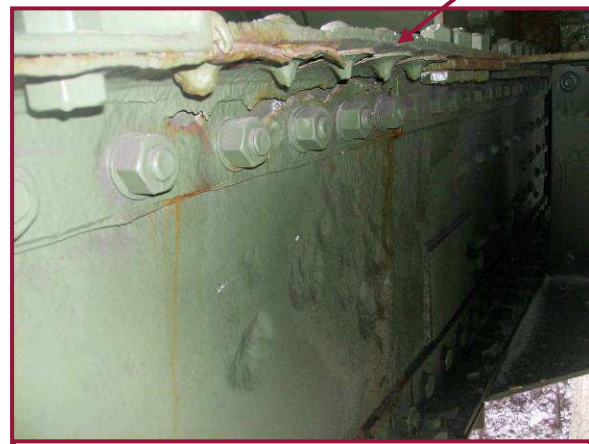
Lower chord member AL112-AL113 exhibits advanced section loss at several components of the built up member at AL113. These losses are depicted in Section A-A. Note multiple retrofits at this location.
