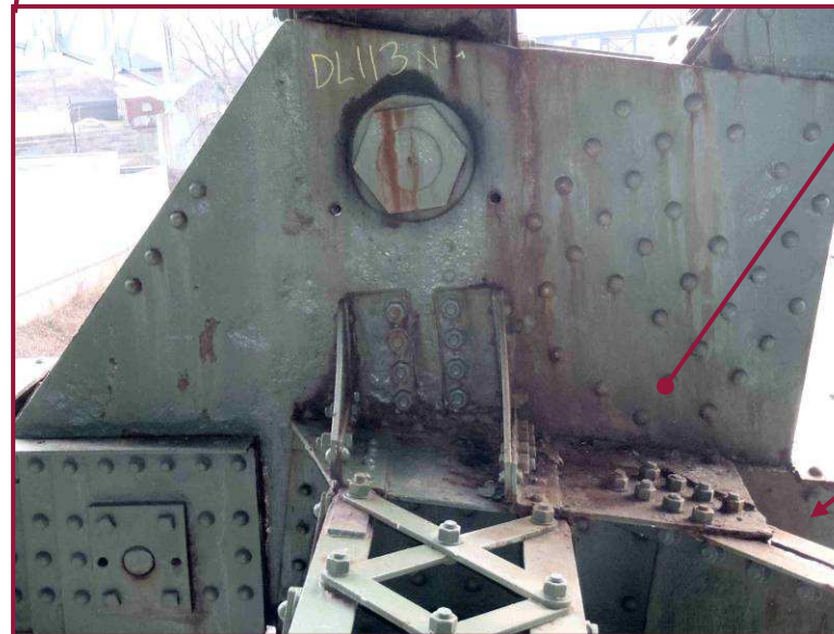
DL113N exhibits heavy pitting throughout both faces of the plate (north face shown). Active corrosion is present due to the leaking deck joint above this location.
