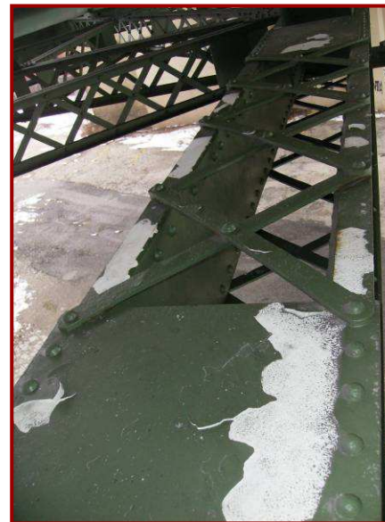
BL130-BL131 exhibits extensive areas of peeling paint.
