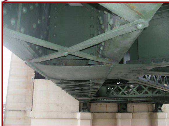
The lateral bracing connection plate/bottom cover plate CL130 is bowed due to active pack rust up to 1" thick.
