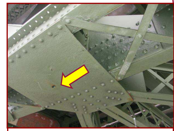
The north face of AL131S exhibits pitting up to 1/4" between the lower chord rivets. The lateral bracing connection plate/bottom cover plate is perforated with a 2" diameter hole.
