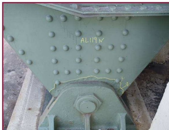
The north gusset plate at AL119 exhibits 1/4" deep around the bearing plate above the pin, with one 3" diameter area with up to 3/8" pitting.
