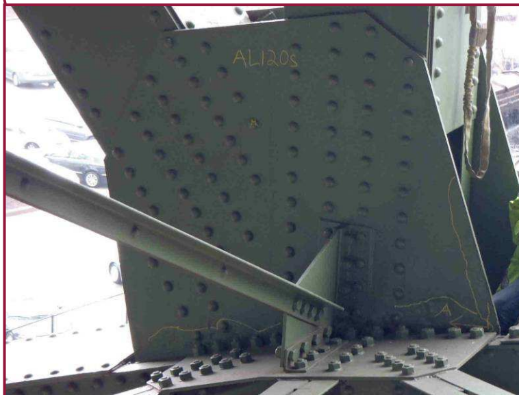
The south gusset plate at AL120 exhibits heavy pitting along the lower chord interface for the entire length of the plate.
