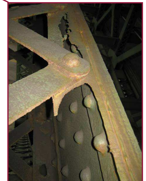
The horizontal leg of the flange angle of AU120-AU121 exhibits advanced section loss with a large area completely corroded. Rust is beginning to reactivate in this area.
