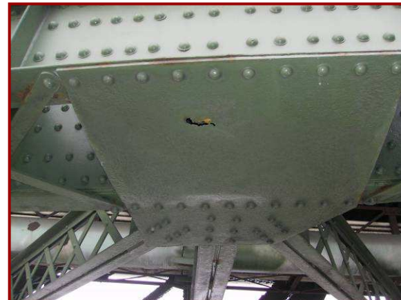
The lateral bracing connection plate/bottom cover plate CL131 is perforated with a 4" diameter hole.
