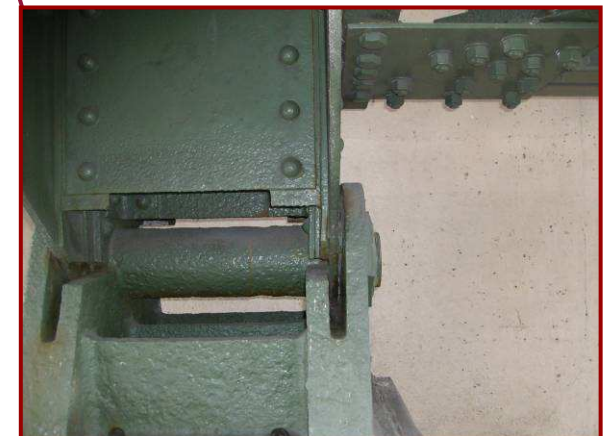
The bearing components at BL133 exhibit 1/8" pitting on all surfaces, with isolated pitting up to 1/4". Additionally, surface rust is reactivating between built up members.
