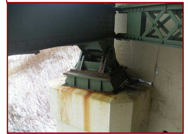
The bearing components at AL131 exhibit 1/8" pitting and activating surface rust throughout.
