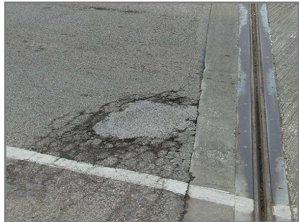
Photo 67– Map cracking around patched pothole in approach pavement.
