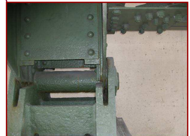
The bearing components at BL133 exhibit 1/8" pitting on all surfaces, with isolated pitting up to 1/4". Additionally, surface rust is reactivating between built up members.
