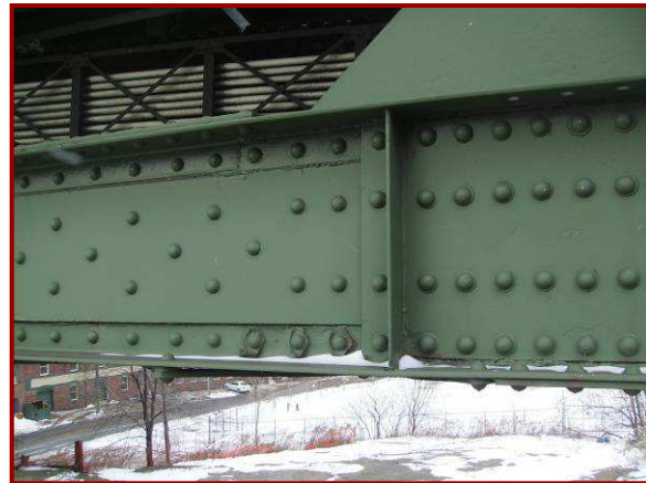
The south web fill plate exhibits 100% section loss below the bounds of the splice plate as well as 1/8" pitting on the bottom angles.
