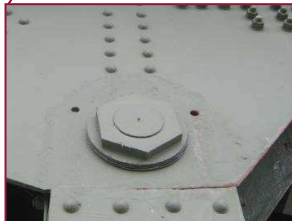
The north gusset plate at AU97 exhibits localized areas with pitting up to 1/4" adjacent to the lower pin and 1/8" pitting along the free edges of the plate.
