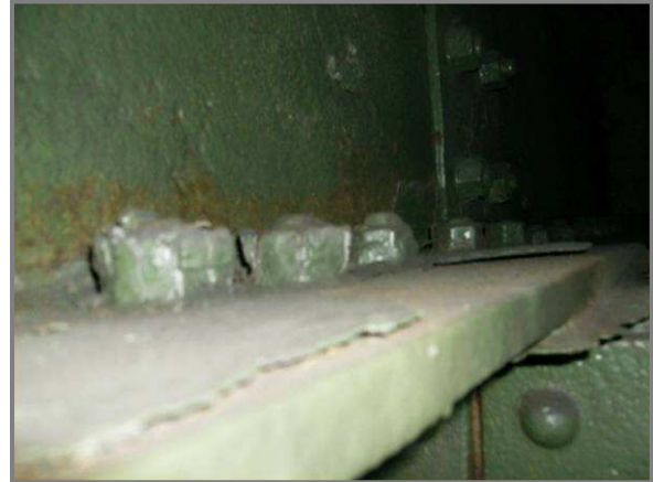
Photo 14 – Isolated 1/4" pitting over the lower fifth of the web of floor beam 78 adjacent to Panel Point CU78.
