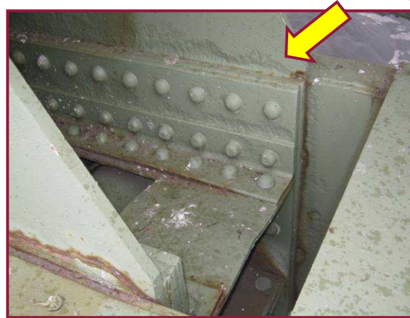
Active rusting is typical along the seams of the built up members at DL58. The south face of the north gusset plate exhibits 1/8" pitting that has been cleaned and painted, while the same location on the south gusset plate exhibits up to 1/4" loss (arrow). Additionally, note that the horizontal stiffener plate between the two gussets is bowed up, measuring approximately 1" from its original plane.
