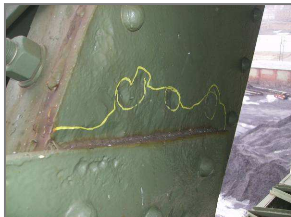
Photo 23 – Typical pitting up to 1/4" (circled in yellow) along interface with gusset plate.
