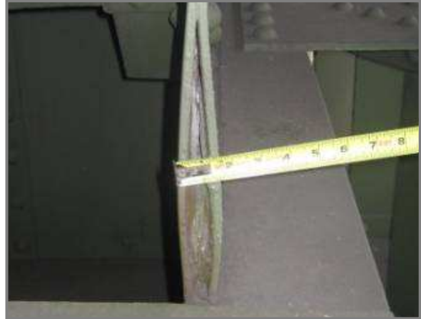
Photo 41 – Laminar split of gusset plate CL70S.
