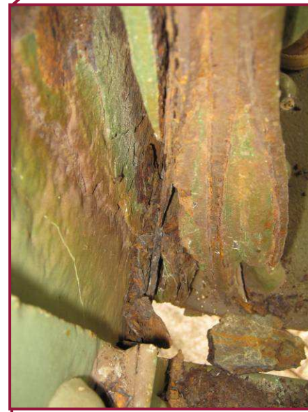
CL12-CL13 exhibits advanced section loss and heavy pack rust at the sliding pin location at CL12. A thin internal fill plate has rusted away at this location, and built up member connections are becoming distressed due to the pack rust and subsequent distortion of the web members, as shown.
