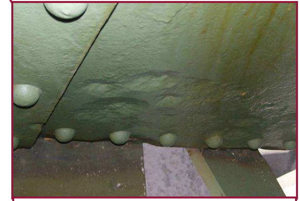
The lower half of the interior face of the DL64-DL65 north web plate exhibits pitting up to 5/16" deep adjacent to the DL64 gusset plate. This condition is typical for Truss D lower chord web plates at the panel interfaces throughout Span 11; however, pitting varies from 1/8" to the 5/16" depth at DL64.
