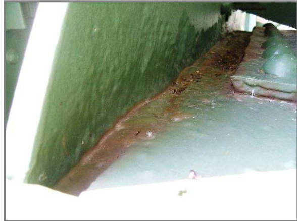
Photo 36 – Typical section loss along the chord member. Exterior of gusset plate DL2N shown.
