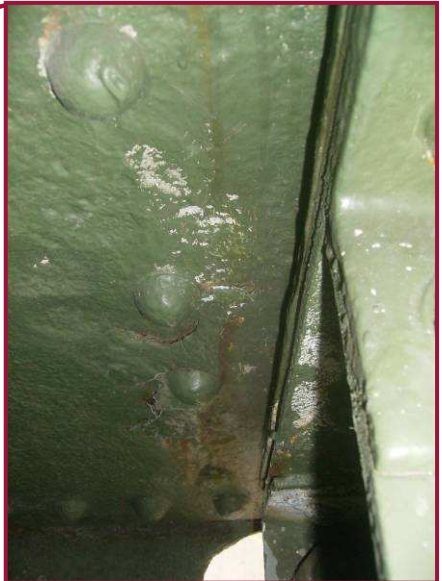
The interior face of the south web plate of BL113-BL114 exhibits full height pitting up to 1/4" deep at the interface with the BL113 gusset plate.
