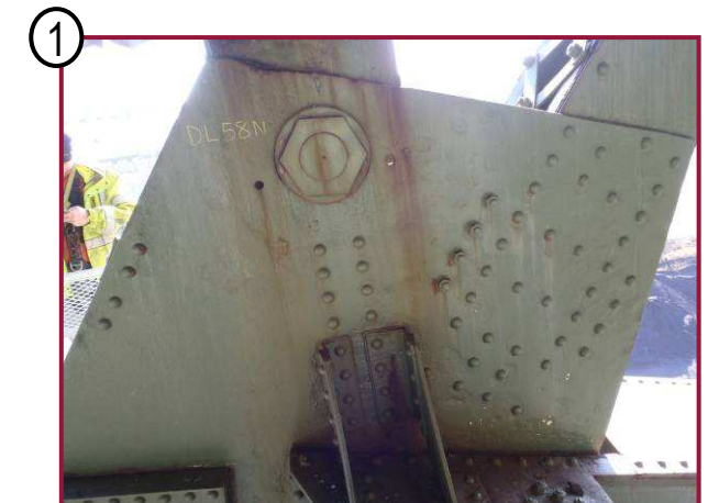
The north gusset plate at DL58 exhibits up to 3/16" pitting, a condition typically found at the expansion locations throughout the structure.
