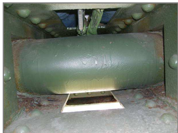
Photo 55– Sliding pin at BL41 seized due to impacted rust.
