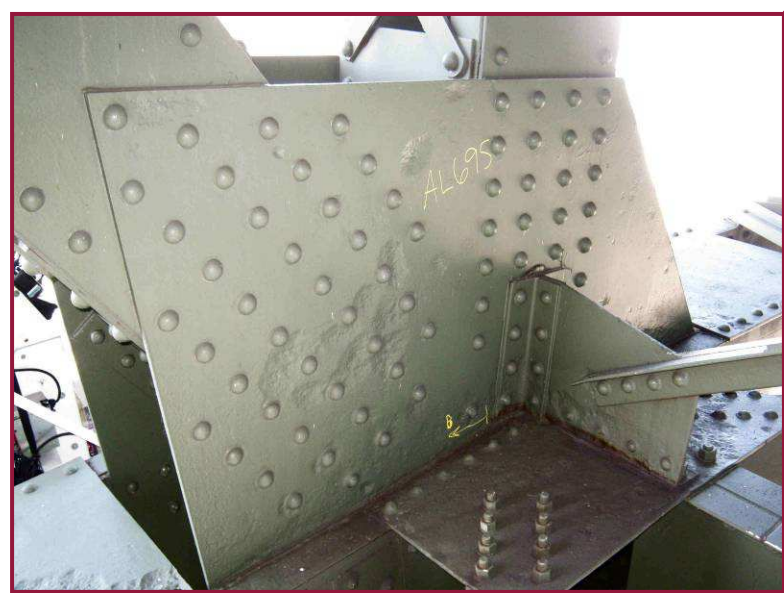
The south face of the south gusset plate at AL69 exhibits heavy pitting along the lower chord interface and adjacent to isolated rivet heads. Note the heavy pitting of the lateral connection plates at this location as well.
