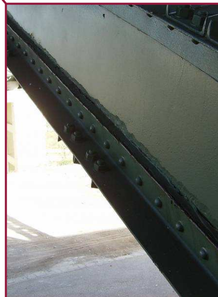
Pitting up to 1/8" deep is present in the bottom 4" of the north web plate along the bottom flange angle at BL0-BL1.
