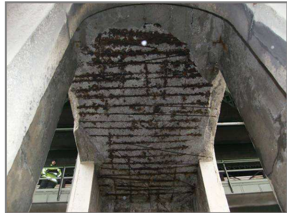
Photo 57– Advanced spall with exposed rebar on roof of Pier 12 tower above bearings. Note hanging exposed rebar.
