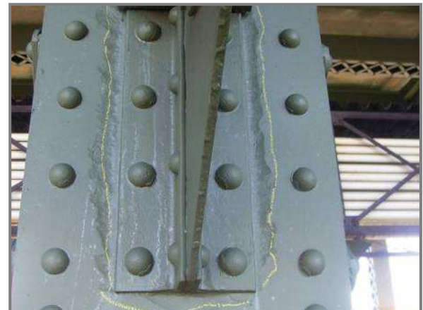
Photo 19 – Pitting up to 1/8" surrounding the sway bracing connection to the north web plate of member BL59-BU59.
