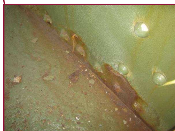
DL12-DL13 exhibits moderate corrosion and pitting up to 1/4" deep over the lower 1/3 of north web plate, with a 2" Ø hole near the bottom cover plate interface.
