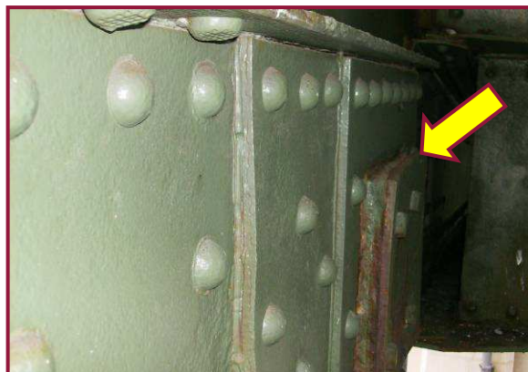
DL58-DL59 exhibits pack rust measuring approximately 1.5" thick between the two outermost pin plates at DL58. Losses surrounding the pack rust are approximately 1/8" on each plate. Similar conditions were noted at DL63 with 1/2" thick pack rust.
