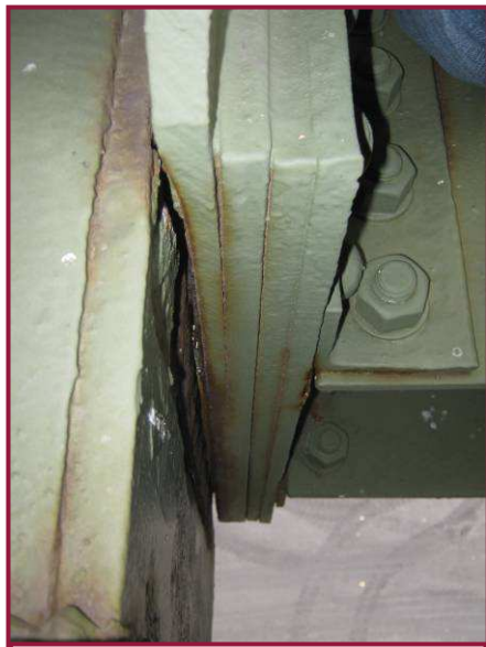
Pitting up to 1/4" deep is present on both members at the interface of the south pin plates and the south web plate of AL58-AL59.
