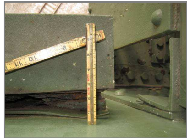
Photo 35 – Impacted rust up to 2 1/2" between the south web plate of CL12-CL13 and gusset plate CL12S.
