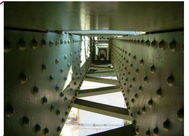
The interior of the lower chord box section is typically cleaned and painted, typically with little or no active rusting (CL6-CL7 shown).
