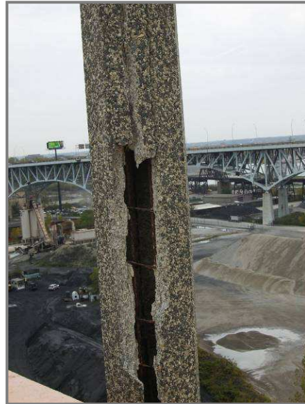
Photo 70– 5'x6" spall in light pole with exposed rebar located along the south sidewalk in Span 10.
