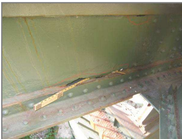
Photo 30 – Holed-through section of north web plate 2'Lx2"H of member DL0-DL1 adjacent to gusset plate DL0N.
