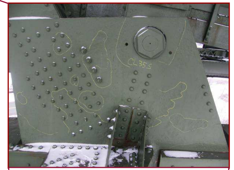
The south gusset plate at CL35 exhibits 1/8" deep pitting throughout areas of the south face, with small areas with up to 1/4" deep pits on the north face of the plate along the lower chord.
