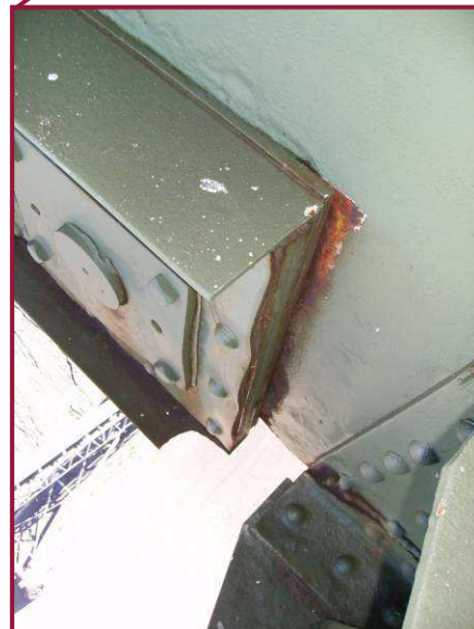
The north gusset plate at BL58 shows signs of abrasion with the lower chord at the sliding pin location, indicating movement of the suspended span. Note also the swelling of the pin plates between rivets on the lower chord member.
