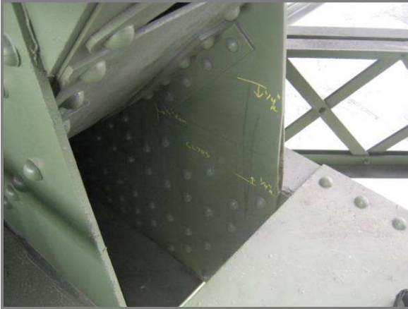
Photo 40 – Bounds (marked by yellow paint stick) of lamellar tear at CL70S (west end of plate).
