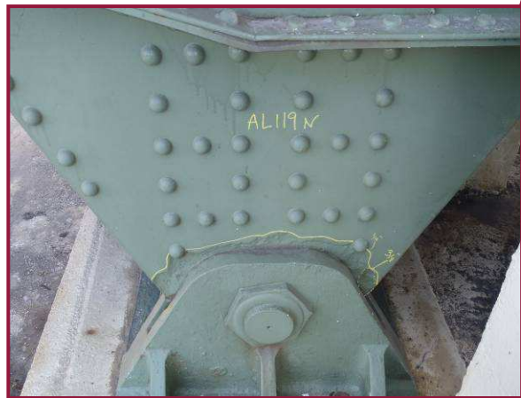
The north gusset plate at AL119 exhibits 1/4" deep around the bearing plate above the pin, with one 3" diameter area with up to 3/8" pitting.
