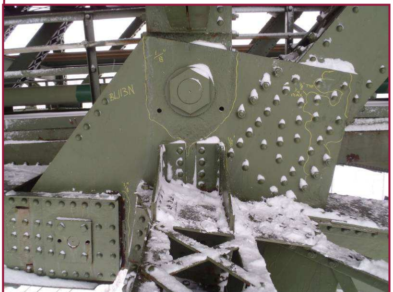
The north gusset plate at BL113 exhibits localized pitting up to 1/4" deep. The areas outlined on the plate are representative of typical losses at pinned gusset plates throughout the structure.
