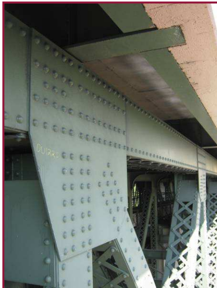
The Truss D upper chord in Span 18 is typically clean with paint intact and no significant deficiencies. DL122 is shown looking east.
