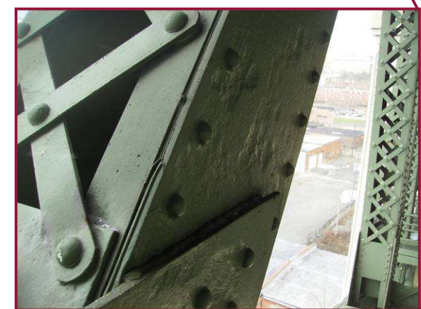
Heavy pitting is present along the web of AL73-AU74 at the lower gusset plate interface (Section A-A).
