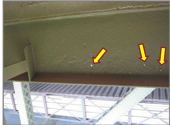
Photo 11 – First interior stringer adjacent to Panel Point DU165 with holed-through sections up to 1" diameter.
