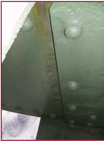
The lower chord, north web plate at DL69 exhibits pitting up to 1/4" deep along the gusset plate interface. This condition is common throughout Span 12; however, losses are typically less, consisting of 1/8" deep across the section. Also note the minor pitting along the interior face of the gusset plate adjacent to the lower chord.
