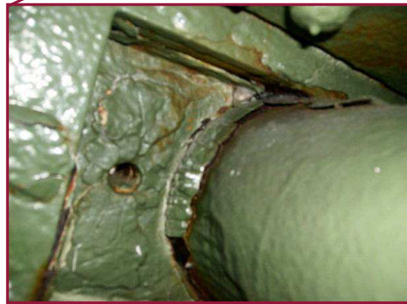
The lower sliding pin at AL63 is heavily corroded with rust scaling at the pin to pin plate interface. Rust is reactivating throughout these components.
