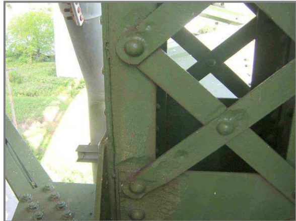
Photo 20 – Isolated pitting up to 1/4" on vertical DL21-DU21 adjacent to lacing bars.
