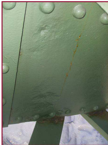
The south web plate of AL48-AL49 has heavy pitting up to 1/4" deep for approximately half the web height near AL49. Similar conditions are found at AL 51.
