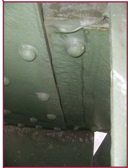
DL50-DL51 exhibits up to 1/4" deep pitting over the full height of the north web at DL50. 1/8" pitting is typically found at similar locations throughout the lower panels in Span 10.
