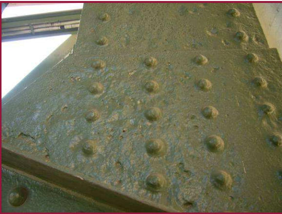
The north gusset plate at CL0 exhibits heavy pitting throughout with areas with pits up to 3/8" deep.
