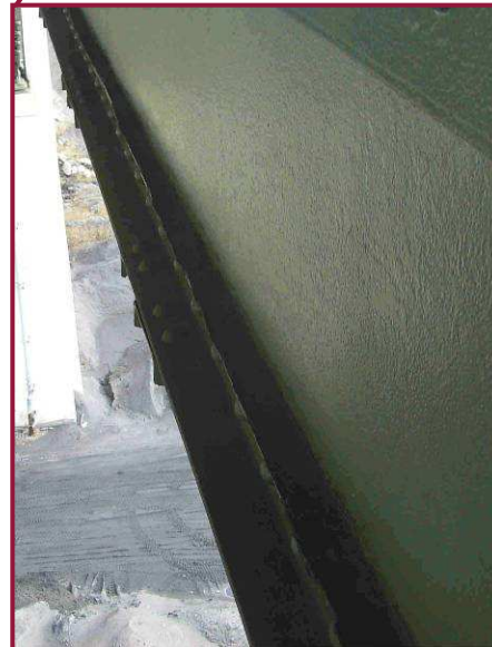
The lower chord member DL69-DL70 exhibits pack rust up to 2" thick between the north web plate and the lower flange angle. Pitting up to 3/16" was noted on the north web plate along the flange angle.
