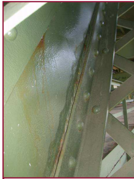
The interior face of the south web plate at BL12-LU11 exhibits 1/8" deep pitting along the lower flange angle.
