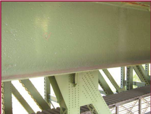
Stringer 2 exhibits pitting up to 1/4" deep on the top of the bottom flange and typical 1/16" pitting with isolated 1/4" pitting throughout the web.
