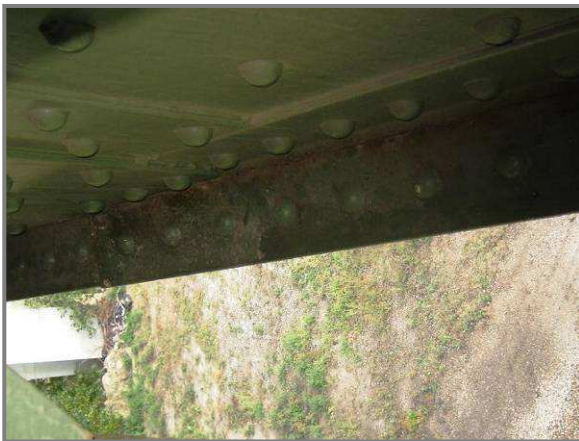
Photo 34 – Crack in bottom flange angle of BL13-BL14 near BL13 within the bounds of the bottom flange batten plate.
