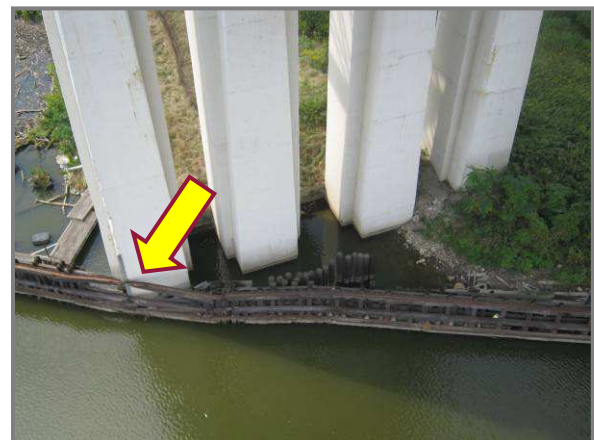
Photo 63– West bank fender system with collision damage at the southernmost pier column.
