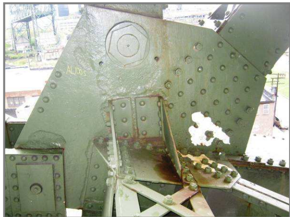
Photo 37 – Typical pitting at a lower pin gusset plate (AL100N). Note pitting around pin and chord members as well as isolated peeling top coat.
