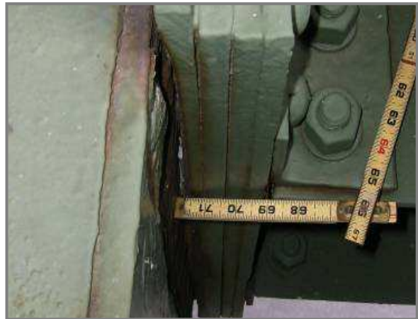
Photo 42 – Typical gusset plate loss measurable along the free edge at sliding pin locations.
