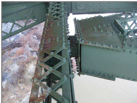
Photo 44– Typical wind lock with minor surface corrosion at strut.
