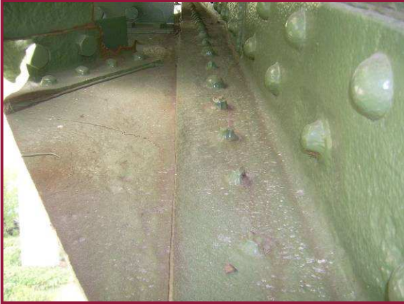
Heavy pitting is typical along the horizontal surfaces of members at DL23, including approximately 50% loss of 9 of the 20 rivet heads connecting the lower lateral gusset plate to the lower chord flange at this location (cleaned and painted).
