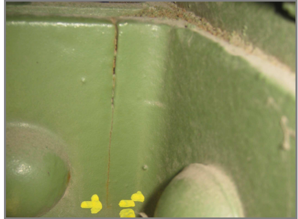
Photo 17 – Utility deck floor beam connection angle to gusset plate BL15S exhibits 3" long rolling flaw.
