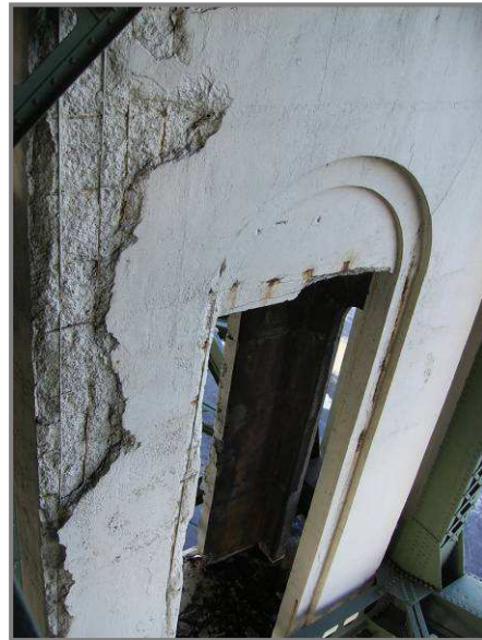
Photo 56– Typical spall with exposed rebar pier tower.
