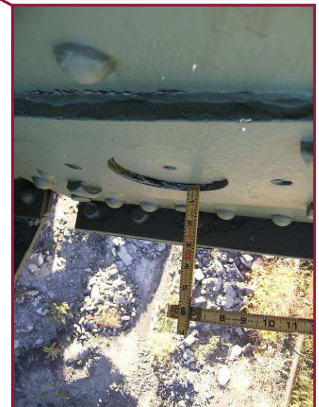
Pack rust at BL83 has pushed the sliding pin plates outward.
