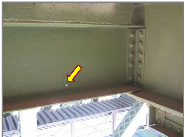
Photo 12 – First interior stringer near DU16 with isolated holed through sections.
