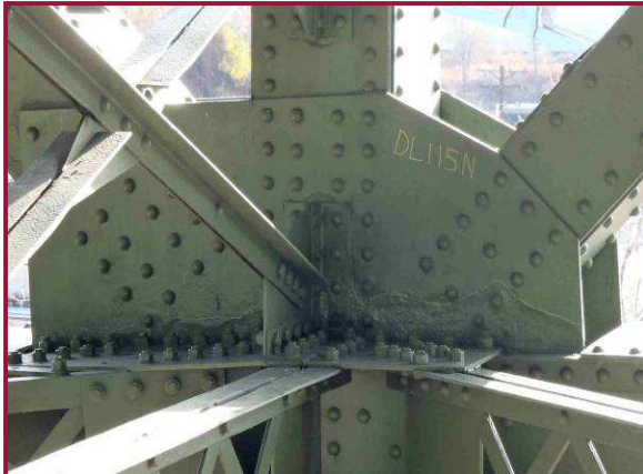
DL115N exhibits heavy pitting along the lower chord interface. The pitting is typically between 6" and 12" tall and extends the length of the plate. DL114N exhibits similar conditions.
