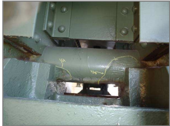
Photo 45– Bearing pin at AL119 with up to 1/4" pitting (cleaned and painted) around the bearing casting.
