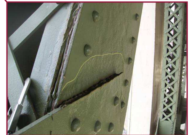
The south web plate of AL43-AU44 exhibits 1/4" deep pitting across the full height of the plate at the lower gusset plate interface.
