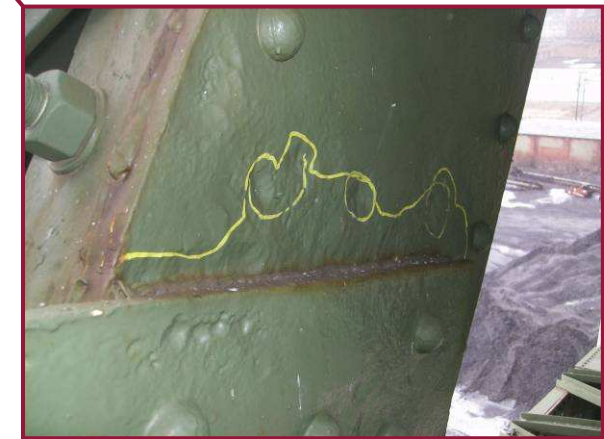
The south web plate of AL63-AU64 exhibits 1/4" deep pitting across the full height of the web, with three small areas with 5/16" loss. The north plate exhibits 1/8" loss in the same section (see Section A-A).
