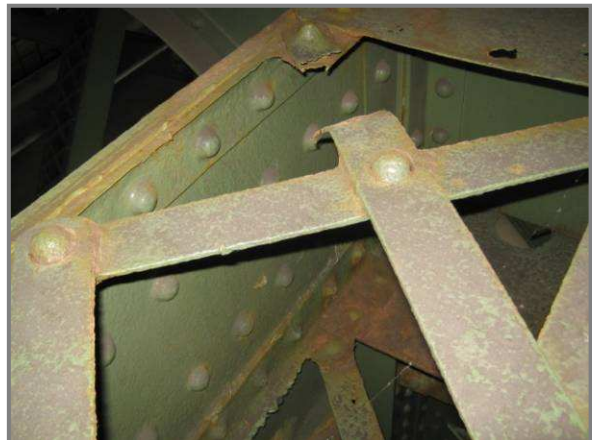
Photo 27 – AU120-AU121 exhibits 100% section loss to lacing bars and horizontal leg of flange angles over a 1' length within the bounds of gusset plate AU120.
