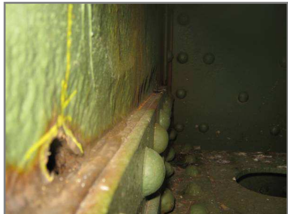
Photo 43 – 1" diameter hole in DL12S along interface with interior diaphragm.
