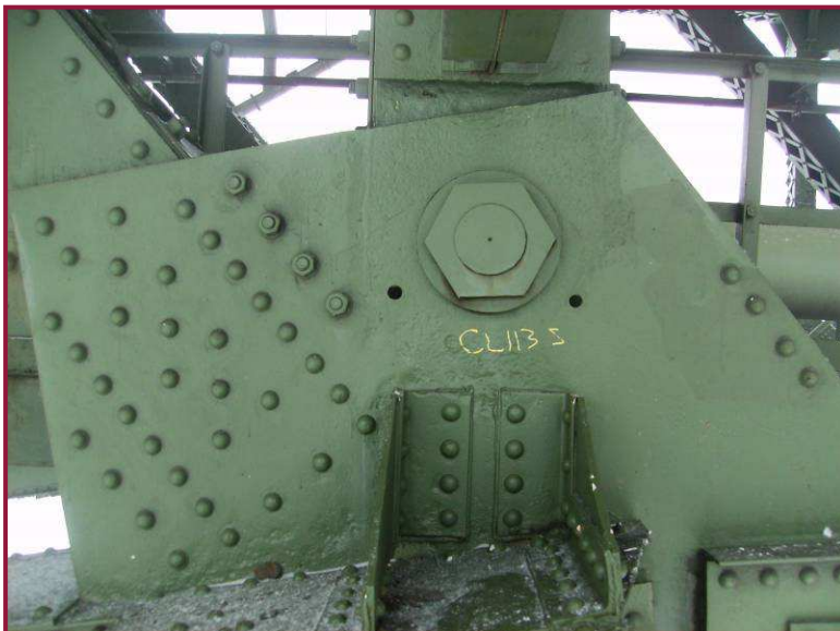
The north gusset plate at CL113 exhibits heavy pitting throughout the north face with up to 1/4" deep areas isolated among the more typical 1/8"-3/16" deep pitting. The deepest pitting is found along the interface of the gusset with the lower chord top flanges and vertically along the lateral knee brace.
