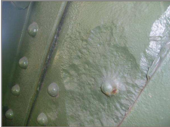
Photo 24 – 3/8" pitting (cleaned and painted) on the interior face of the south web plate near the interface with gusset plate DL36 between flange angles.
