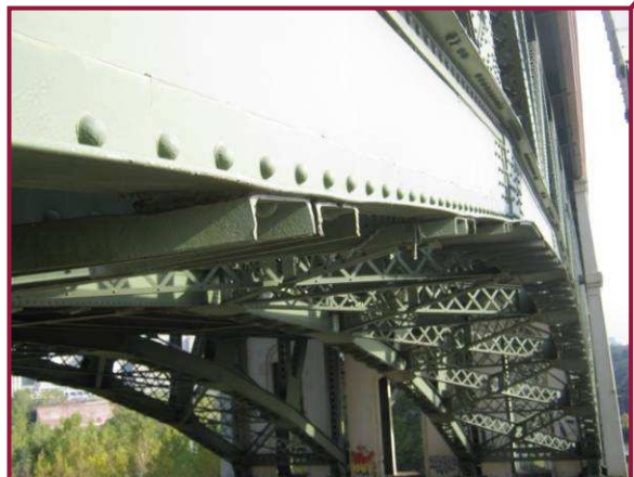
The horizontal legs of bottom flange angles are warped slightly throughout the bridge at isolated lacing connections due to pack rust between the angles and the lacing channels.
