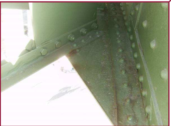
The lower lateral bracing connection plates typically exhibit pitting between 1/16" and 1/8" deep, with localized pitting up to 1/4" deep. The adjacent bottom flange angles exhibit similar pitting. Light surface corrosion is typically forming at these locations.
