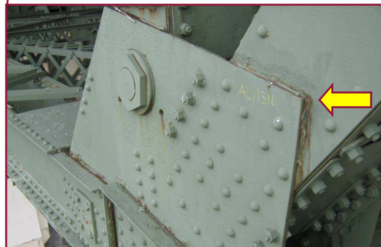
The north gusset plate at AL113 exhibits areas of 1/8" pitting scattered throughout the north face. The north web plate of the diagonal member AU112-AL113 exhibits 1/8" deep pitting along the full height of the web plate.
