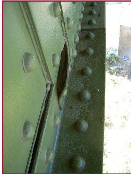
The bottom flange angle splice plate at CL11 is bowed out approximately 1.5" due to heavy pack rust.
