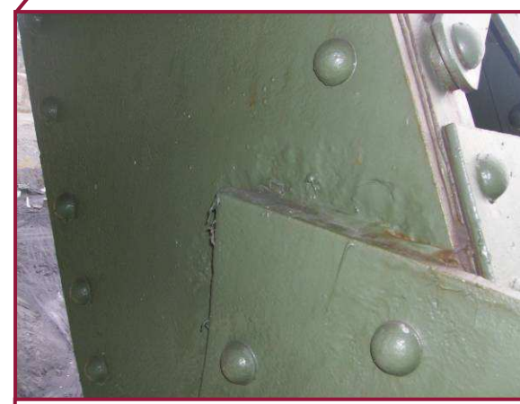
Pitting of the north web plate at the gusset plate interface on diagonal member DL64-UL65 is up to 3/16" deep with light surface corrosion along the seam between the two plates. This condition is typical for Span 11, Truss D for other web members. Only member DL59-UL58 in Span 11 exhibited heavier pitting at this interface, with up to 5/16" loss.
