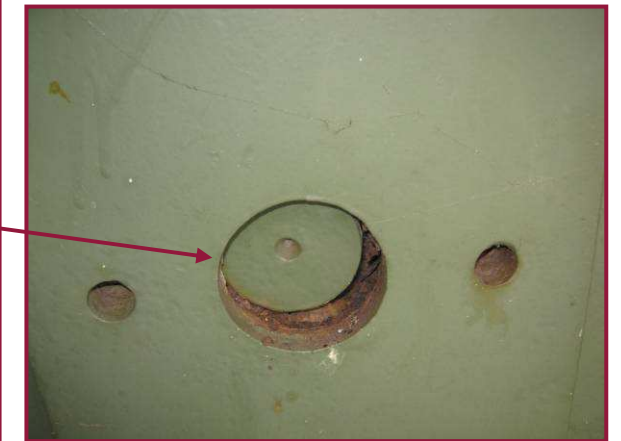
The lower chord sliding pin at CL12 is not bearing on the keeper plate, exhibiting lateral misalignment.
