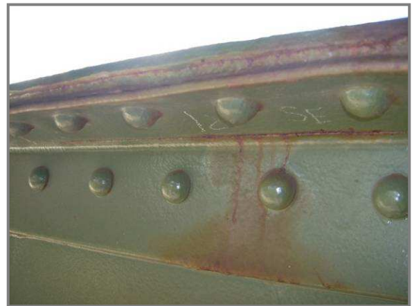
Photo 33 – Crack in top flange angle of DL15-DL16 near DL15 within Bounds of top batten plate.
