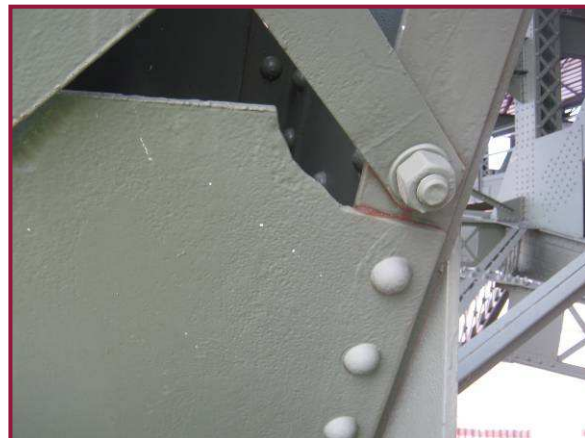
The lower cover batten plate of AL23-AU22 has been flame-cut to accommodate previous repair work done at this location. Note retrofit bolt at the lower lacing connection.
