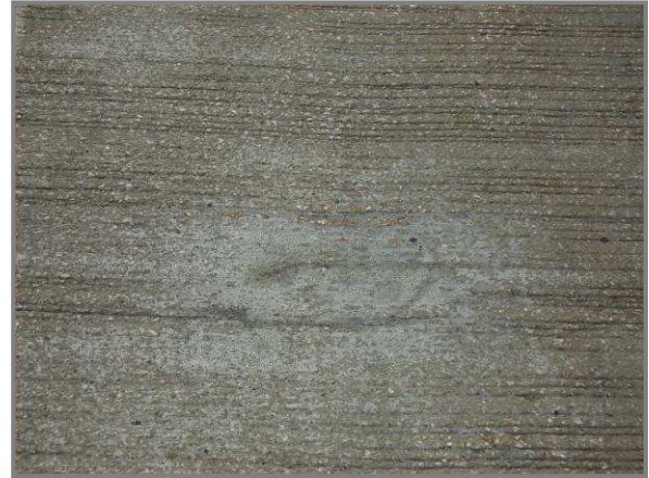
Photo 4 – Isolated area of worn wearing surface in bike lane.
