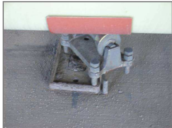
Photo 72– Misaligned support for 40" gas main on utility deck adjacent to Pier 15.
