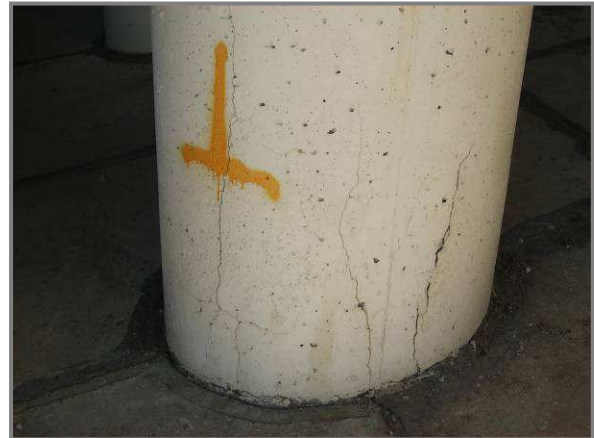
Photo 60– Vertical hairline cracks in Bent 1 columns.
