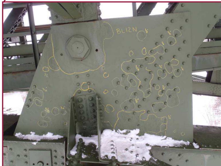
Gusset plate BL12N exhibits small areas of deep pitting up to 5/16" throughout. All locations exhibiting greater than 3/16" deep pitting are highlighted with field markings. The south plate at BL12 exhibits conditions similar to those shown, while losses at BL17 are considerably less severe, typically 1/8" deep.
