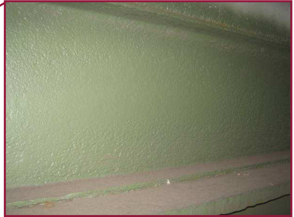
Pitting up to 1/8" deep is freckled throughout the south face of Stringer 2 between Floorbeams 53 and 54. This condition is common for Stringer 2 throughout Span 10.
