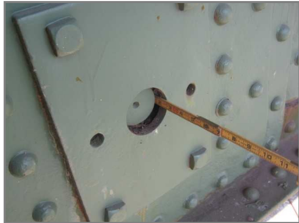
Photo 52 – Sliding pin at CL12S not fully bearing on the outermost pin plate due to impacted rust between the web plate and gusset plate.
