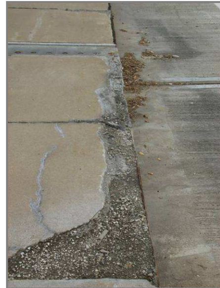
Photo 5 – Isolated sidewalk spall in Span 19 on the north sidewalk.
