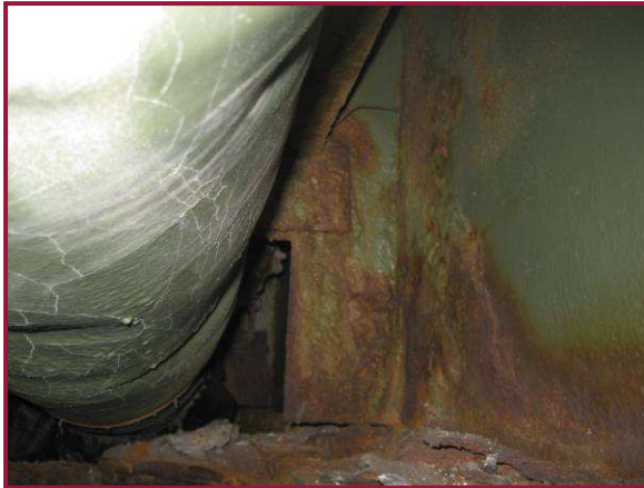
Floorbeam 58 exhibits widespread moderate corrosion with 1/16"-1/8" pitting adjacent to the drainage trough. This condition is typical for floorbeams at expansion joint locations due to joint deficiencies.
