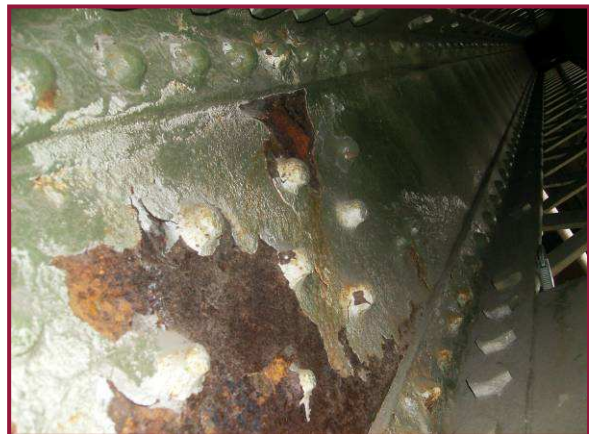
The interior of BU112-BL113 exhibits failing paint throughout with minor active corrosion near BL113. The rivets connecting the diagonal member to the gusset plates are heavily pitted, with an estimated 50% loss of rivet head section.
