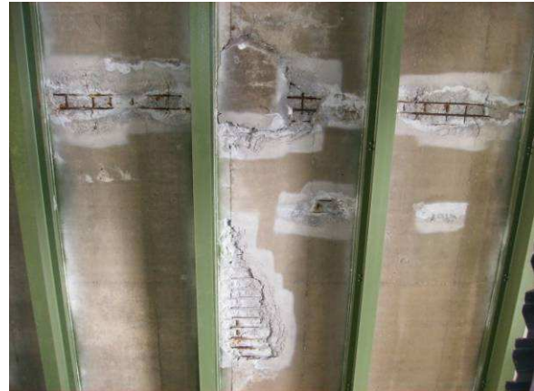
Photo 1 – Span 9 between FB 33 and FB34 roadway deck underside. Note several spalls have been sealed.
