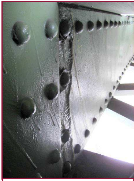
The south web plate of CL95-CL96 exhibits advanced section loss across the full height of the plate at the interface with the south gusset at CL96. Pitting up to 3/8" was noted at this location.
