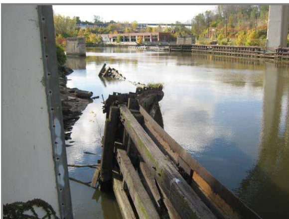
Photo 62– East fender system collapsed towards river centerline (looking south).
