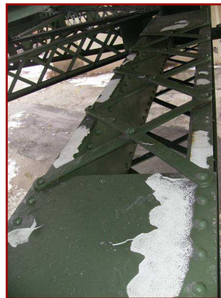
BL130-BL131 exhibits extensive areas of peeling paint.
