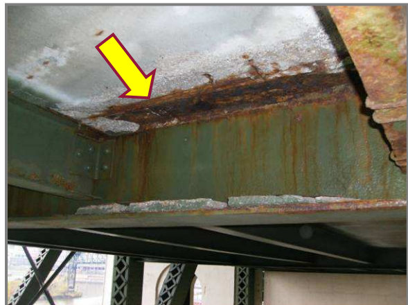
Photo 3 – Typical utility deck haunch spall adjacent to floor beam 53 top flange in Bay 5.
