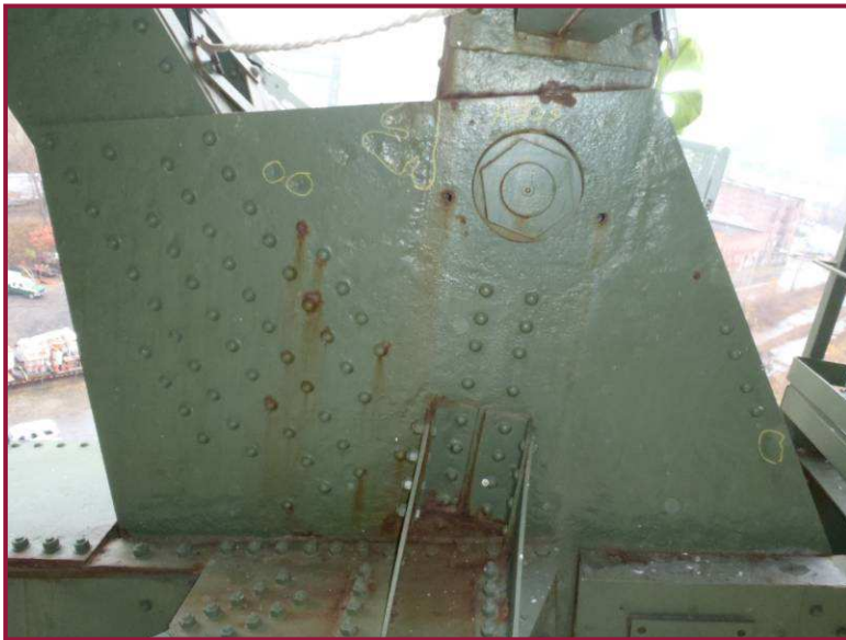
AL35S exhibits heavy pitting throughout the south face of the plate, with 1/4" losses in isolated areas.
