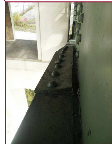
The top flange splice plate at CL74S is distorted due to pack rust.
