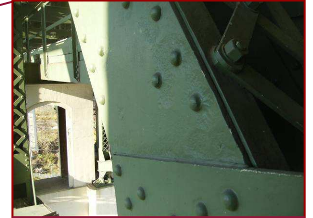
The south web plate of CL35-CL34 exhibits 1/8" deep pitting along the full width of the plate at the interface with the lower gusset plate.
