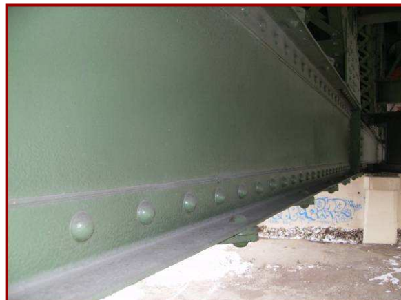
BL128-BL129 exhibits conditions typical for lower chord members throughout Truss B in Span 20.
