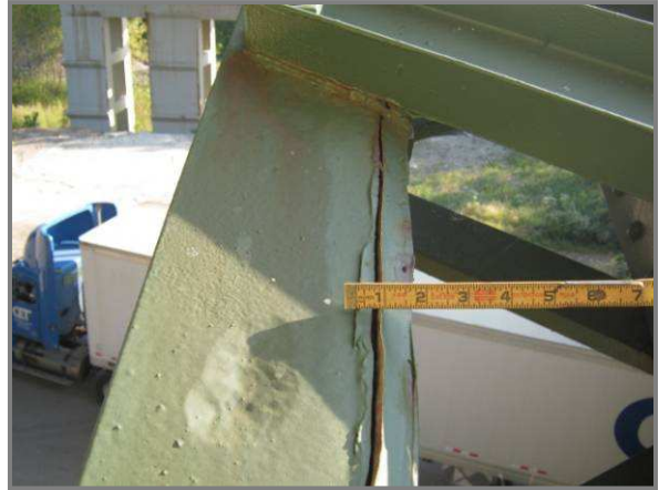
Photo 32 – Typical evidence of sealed impacted rust reactivating.
