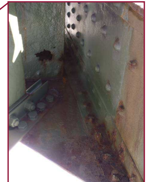
The lower chord below DL113 exhibits heavy pitting of the north web plate and flange angles. The stay plate of the lateral bracing is perforated with a 6"Ø hole.
