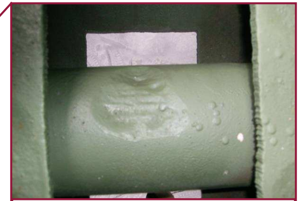
The lower sliding pin at DL63 has a 4" diameter area exhibiting up to 5/16" deep pitting. This location has been cleaned and painted with no active rusting.
