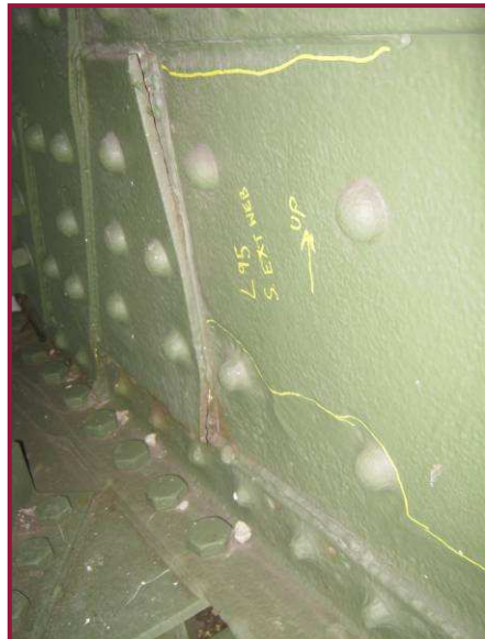
The south web plate of AL95-AL96 at AL95 exhibits 1/8" and 1/4" deep pitting along the top and bottom flanges, respectively. The bottom flange angle has 1/8" deep pitting on the vertical leg, with isolated pinholes measuring approximately 1/4" diameter.
