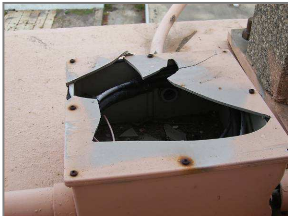
Photo 71– Broken electrical box cover with exposed electrical wires in Span 14 of the north sidewalk overhang.
