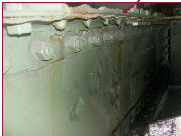
Lower chord member AL112-AL113 exhibits advanced section loss at several components of the built up member at AL113. These losses are depicted in Section A-A. Note multiple retrofits at this location.
