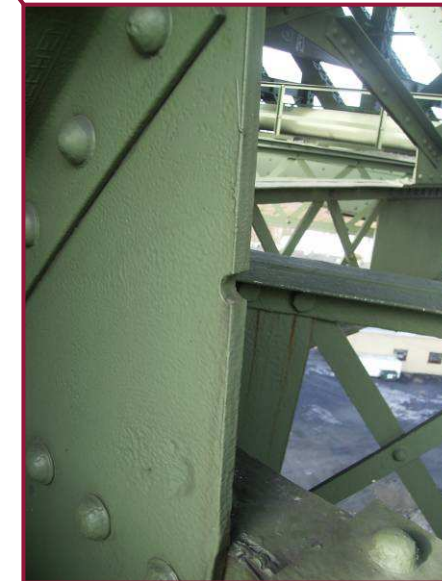
Both gusset plates at DL71 have misplaced drill/punch holes along the east free edge.
