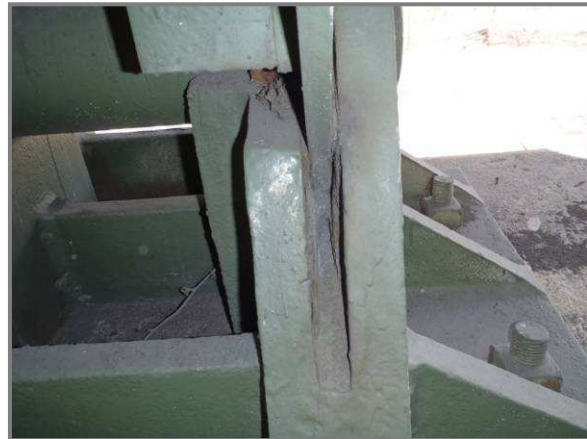
Photo 46– CL119 impacted rust between bearing casting and gusset plate seizing panel point from free rotation.
