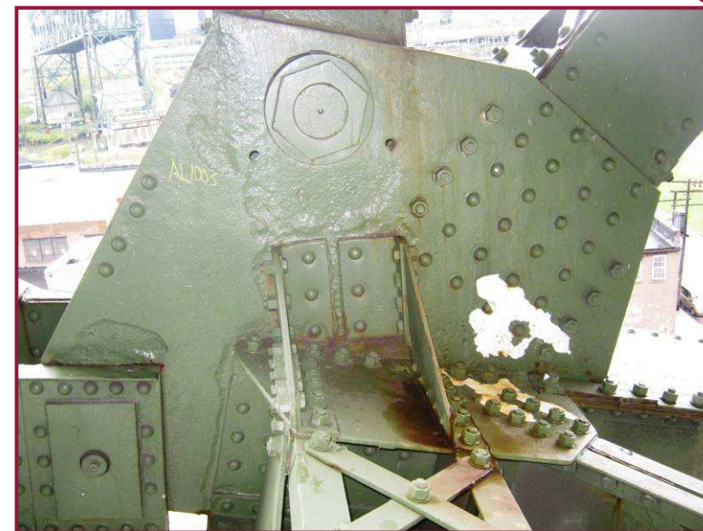
The south gusset plate at AL100 exhibits widespread heavy pitting, with locations up to 1/4" common, especially adjacent to connecting members.
