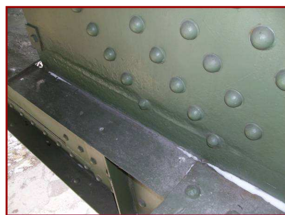
Up to 1/8" pitting is present on the south face of gusset plate AL129S along the bottom row of rivets.
