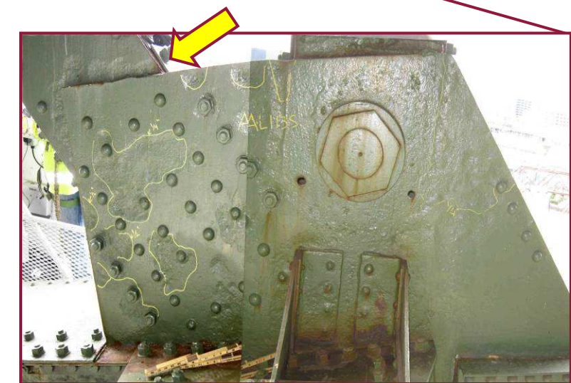
The south face of the south gusset plate at AL113 exhibits widespread heavy losses. The areas highlighted on the plate in yellow exhibit pitting of 1/4" deep or greater. The interior face of the south plate exhibits isolated areas with up to 1/4" loss. Additionally, note the 1/4" deep pitting along the full height of the web of the diagonal member AU112-AL113 near the gusset plate interface.
