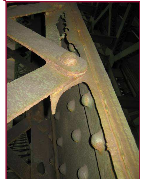
The horizontal leg of the flange angle of AU120-AU121 exhibits advanced section loss with a large area completely corroded. Rust is beginning to reactivate in this area.
