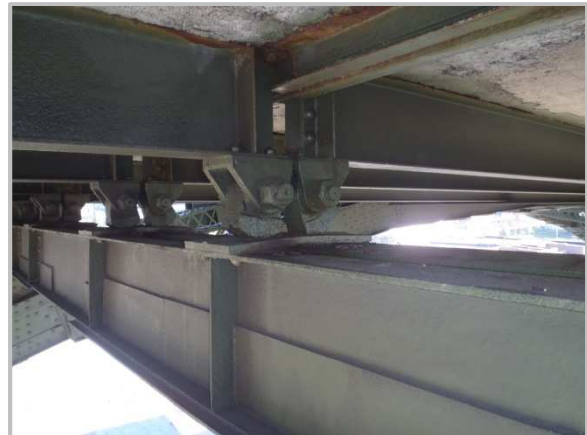
Photo 47 – Excessive rotation of rocker bearings at utility deck Floorbeam 78 below Stringers 3 and 4.
