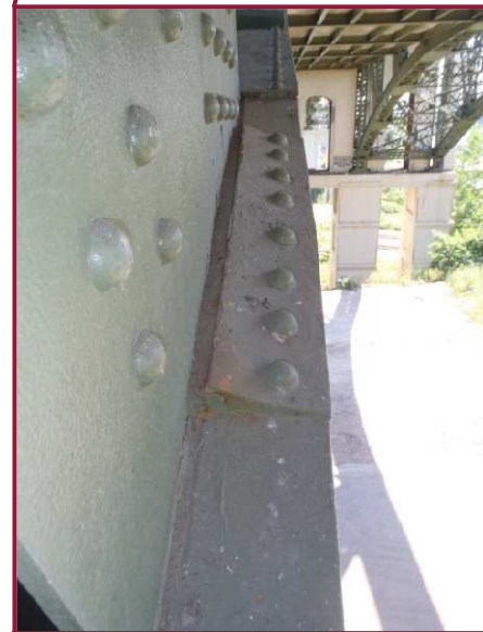
Heavy pack rust up to 1" has formed between the lower chord top flange and flange splice plate at BL1S.
