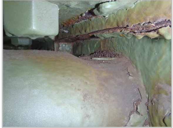
Photo 52 – North side of pin at DL97 with laminate rust and isolated section loss up to 1/2".
