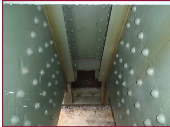
The truss bearing at AL45 was filled with standing water at the time of inspection.
