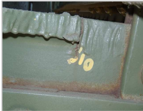
Photo 14 – Crack in utility deck floorbeam at connection to gusset plate CL37S.
