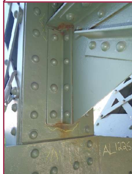
The south web plate of member AL122-AU122 exhibits 1/4" pitting on both sides of the sway brace connection and 3/16" pitting along the bottom of the connection. The north web plate exhibits 1/8" pitting along the full width of the section along the lower chord gusset plate.
