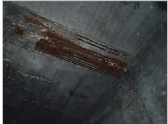
Photo 17 – Spall with exposed, corroded reinforcing bars in Floorbeam 5 underside in the north bay of the east cellular unit.
