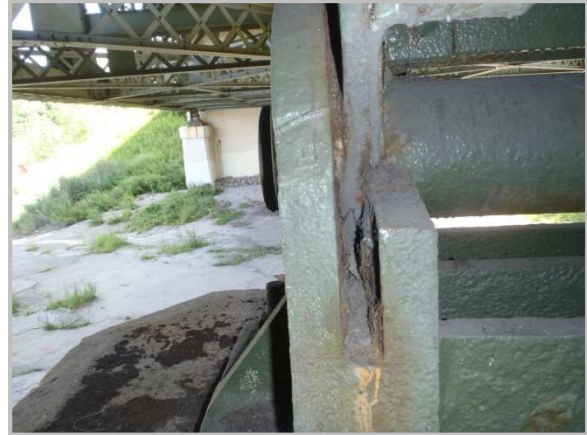
Photo 45 – Pack rust between truss bearing at BL127 and gusset plate BL127N.
