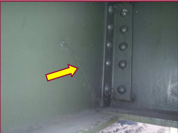
The south fascia stringer just east of Floorbeam 73 has a weld retrofit along the bottom flange cope.
