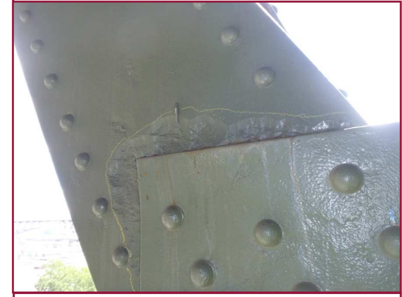
The north web plate of diagonal member DL43-DU44 exhibits 1/4" pitting with isolated 5/16" pitting along gusset plate DL43N for the full height of the section.
