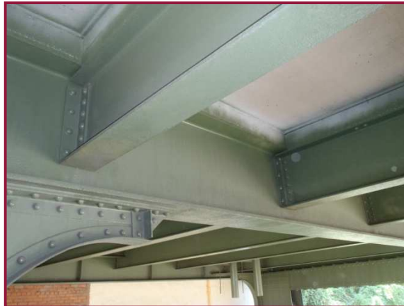
Floorbeam 131 bottom flange exhibits 1/16" pitting (cleaned and painted) for the full width.
