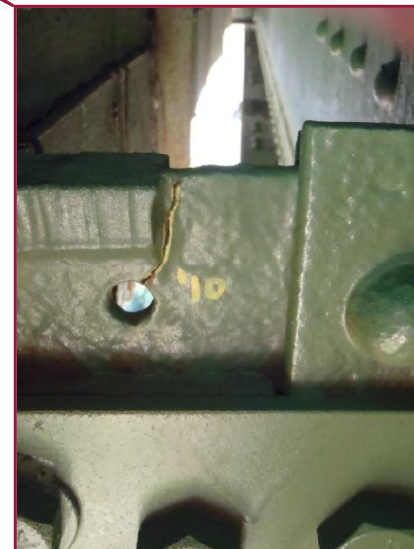
Utility deck Floorbeams 14 and 15 exhibit cracking at the top flange coping near Truss C, extending down into stress relief holes. These cracks are roughly 1-3/4" long and do not appear to have propagated beyond the stress relief holes (Floorbeam 14 shown).
