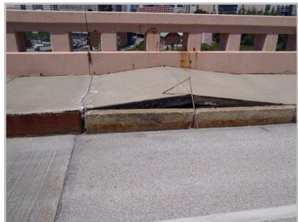
Photo 6 – Buckled section of north sidewalk adjacent to the joint between the east approach slab and east approach roadway.
