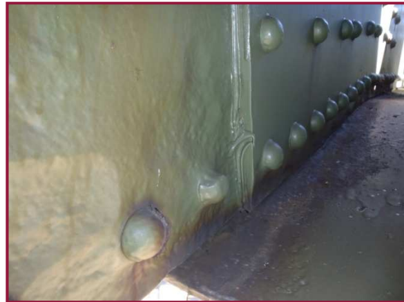
The north web plate of member DL119-DL120 exhibits 1/4" pitting over the bottom 1/4 of the height along the gusset plate interface. Pack rust has built up between this web plate and gusset plate DL120N.
