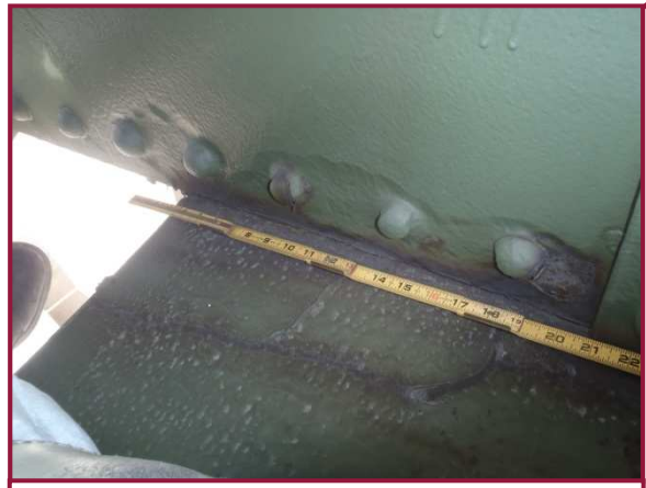
The north interior web plate of DL104-DL105 exhibits 1/16" pitting around the bottom row of rivets for the first 18" from gusset plate DL105N.
