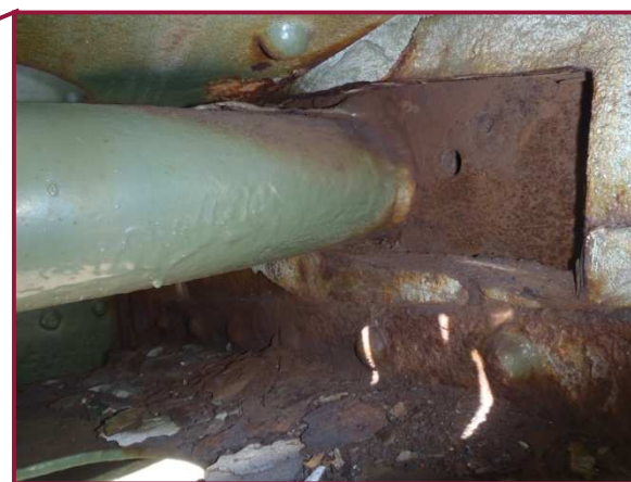
Note active corrosion and wear on north DL12-DL13 lower chord sliding pin at DL12.
