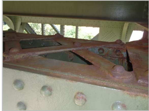
Photo 27 – Active corrosion on DU4-DU5 top flange angles and lacing bars near Panel Point 5.
