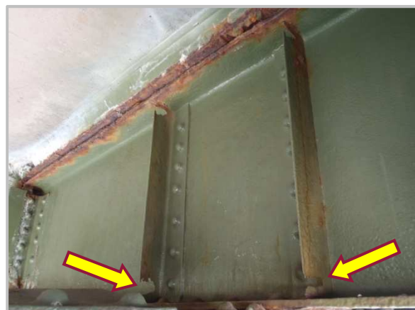
Photo 15 – East face of Floorbeam 100 with 100% section loss to web stiffeners adjacent to Truss A.
