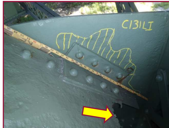
The north face of gusset plate AL113S exhibits 1/4" pitting along the top of the diagonal 24" long by 5" high. This gusset plate also exhibits pitting up to 1/4" between the lower chord rivets. Also note the area of 100% section loss at the base of the diagonal member cover plate.
