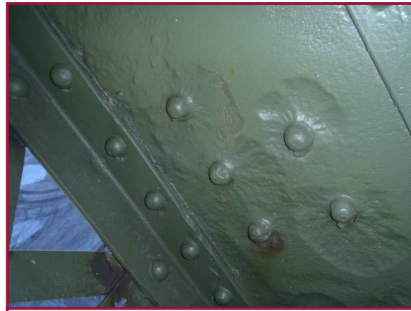
1/4" deep pitting is present across the width of the north web plate of AL78-AU77 adjacent to the lower gusset plate rivets. The south web plate exhibits pitting up to 1/8" deep.
