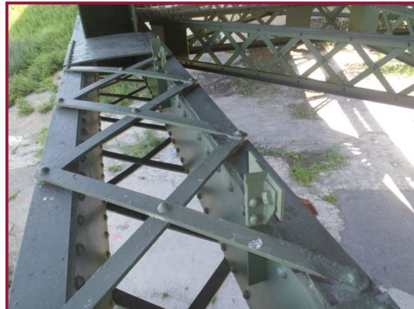
Abandoned bolted connections to the interior south web plate of AL128-AL129
