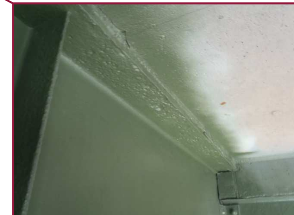
The west side of Floorbeam 122 exhibits 1/4" pitting to the top flange and 25% section loss to the bottom flange.
