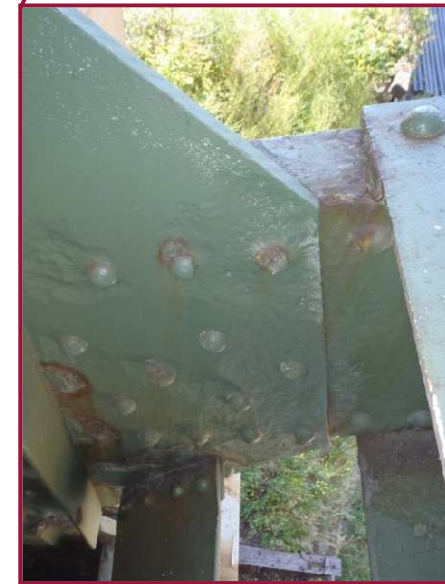
Member DL125-DL126 exhibits 3/16" pitting for the full height of the south web plate along the interface of gusset plate DL126S.
