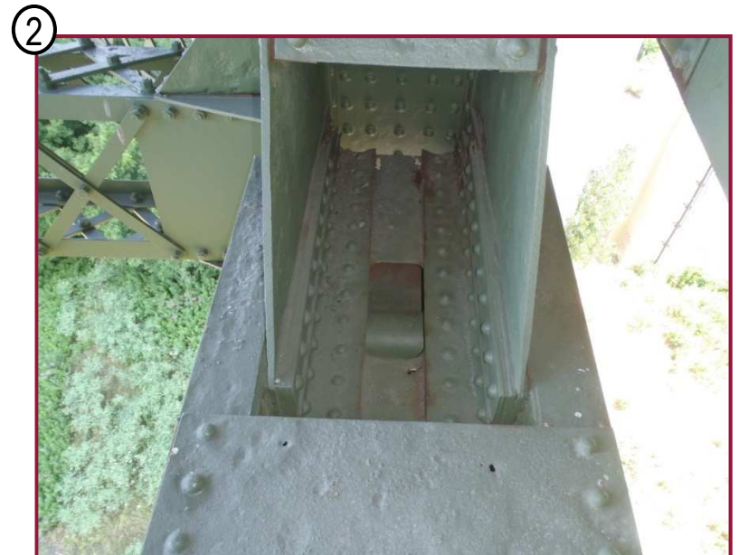
The pin diaphragm plate for lower chord BL16-BL17 at BL17 exhibits 3" diameter holed through sections at the east end. There are isolated holes up to 3/4" diameter in the top lower chord batten plate near this location, as well as minor pitting to top flange angles within the gusset plate bounds.
