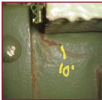
Photo 19 – View of same crack location during 2010 inspection
