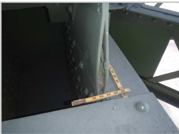
Photo 35 – Lamellar tear along west edge of gusset plate CL70S.
