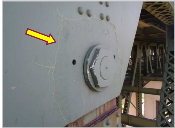
Photo 34 – Typical 1/4" pitting surrounding pin (gusset plate DU113S shown).
