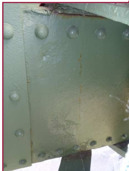
The south web plate of AL48-AL49 has heavy pitting up to 1/4" deep for approximately half the web height near AL49. Similar conditions are found at AL51.
