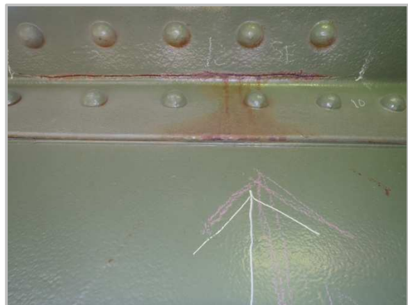
Photo 33 – Crack in top flange angle of DL15-DL16 near DL15 within bounds of top batten plate. This crack has not propagated since the last inspection.
