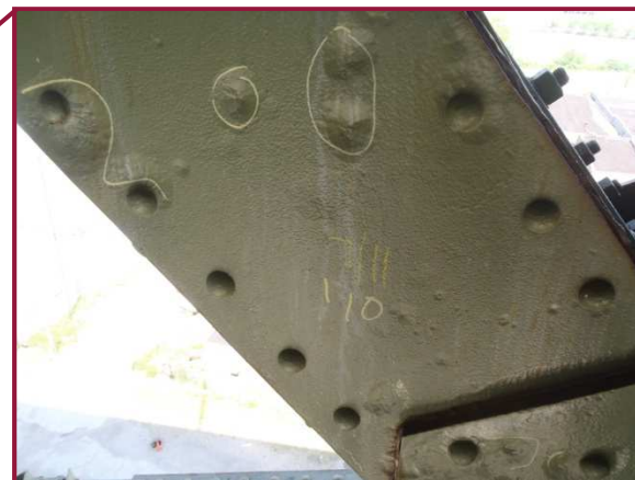
The exterior south web plate of AU96-AL97 exhibits areas of 3/16" pitting (cleaned and painted).
