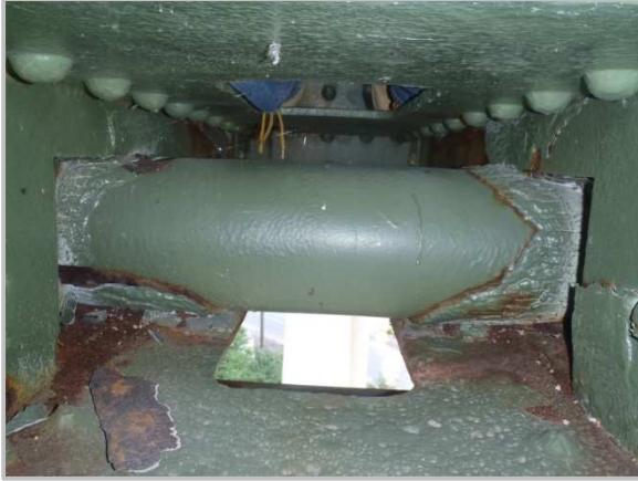
Photo 51 – Sliding pin at AL17 seized due to impacted rust which has been painted over.
