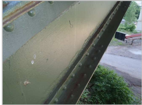
Photo 30 – South web plate of AL0-AL1 with 1/8" pitting along the bottom flange angle.
