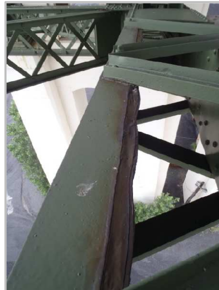
Photo 32 – Previously sealed impacted rust beginning to reactivate between the north web plate and top flange angle of member BL53-BL54.
