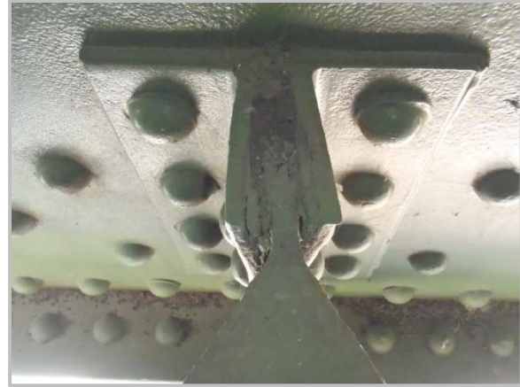
Photo 20 – Pack rust at utility deck floorbeam web and connection angles to gusset plate CL4S.
