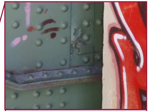
Advanced corrosion at the south web fill plate at BL8 has resulted in a 6" diameter hole.
