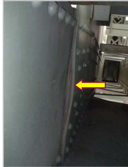
Photo 42 – Pack rust between BL57S free edge and BL57-BL58 south web plate.
