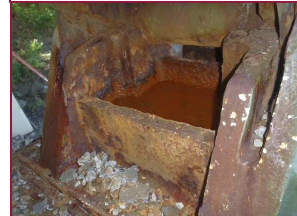
The bearing components at AL131 exhibit 1/8" pitting and activating surface rust throughout. The east side of the bearing contained standing water at the time of the inspection with moderate to heavy rusting in this area.
