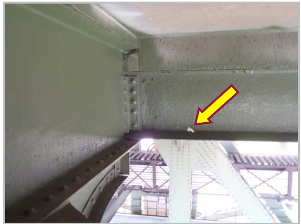
Photo 11 – 3" diameter holed-through section on the first interior stringer near AU118N.
