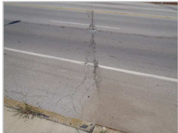
Photo 58 – Transverse crack up to 3/4" wide in west approach pavement.
