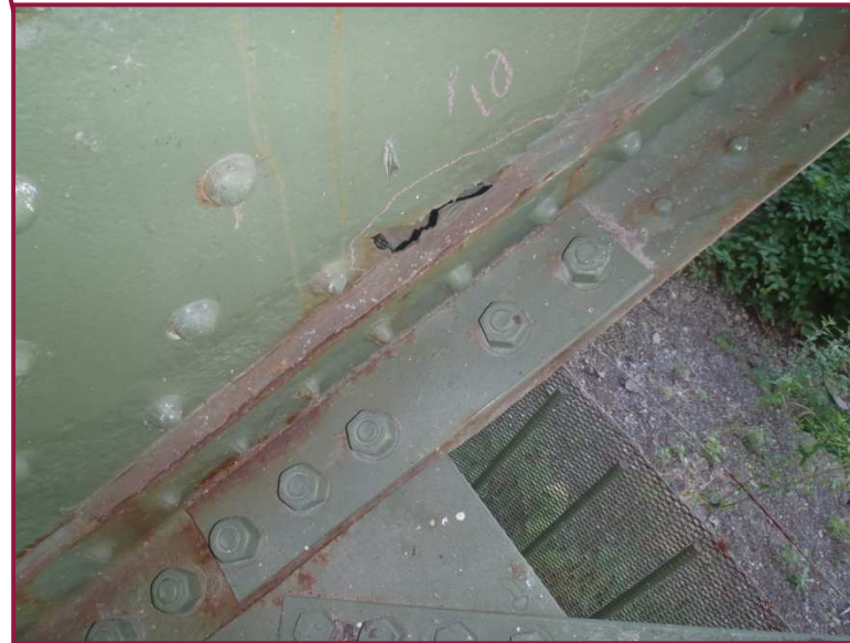
The south web plate of AL0-AL1 exhibits a 2" high by 6" long hole along the bottom flange angle. Note the bolted retrofit plate on the bottom flange outstanding leg at this location.
