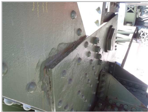
Photo 24 – Member DL116-DU117 with 3/8" pitting on the north web plate along the lower chord gusset plate.
