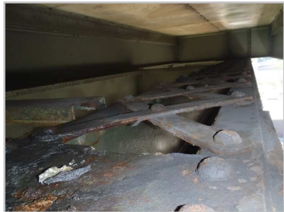
Photo 28 – Pitting up to 1/8" on top flange angles and lacing bars with active corrosion at DU80-DU81 subdrain location.
