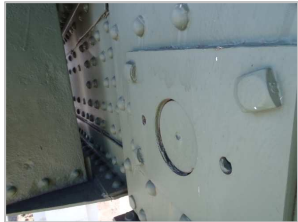
Photo 50 – Sliding pin at BL83 with impacted rust causing 5/16" of pin not to bear on north BL82-BL83 pin plates.
