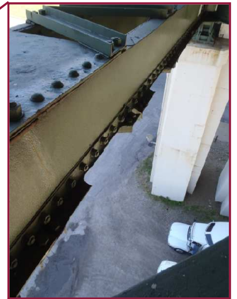
The south bottom flange angle of member AL100-AL101 exhibits isolated holes with sections cut out of the outstanding legs.
