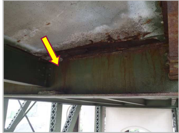
Photo 4 – Typical utility deck haunch spall in Bay 5 adjacent to the top flange of Floorbeam 53.
