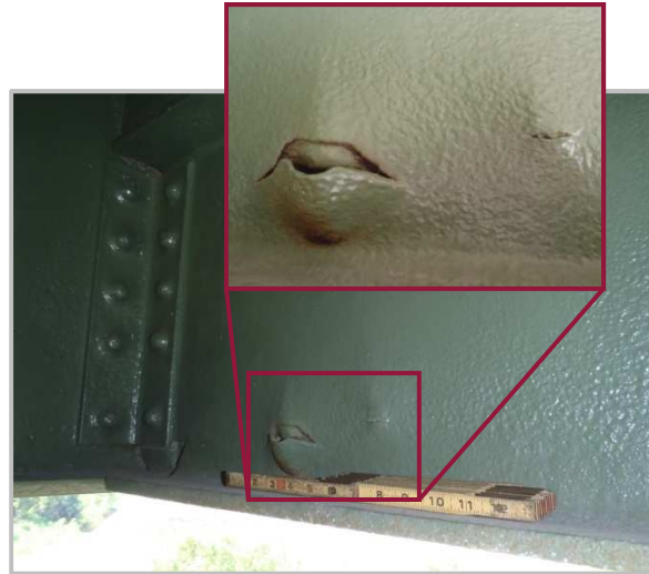
Photo 13 – Tears in web of north fascia stringer just east of Floorbeam 25 with concrete seepage.
