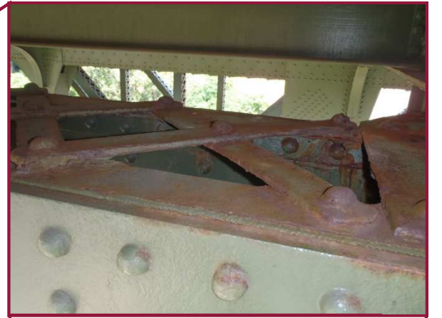
extensive rust and corrosion
