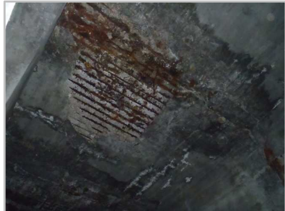
Photo 1 – 10' diameter spall with 100% section loss to 7 consecutive transverse reinforcing bars within the east cellular unit.
