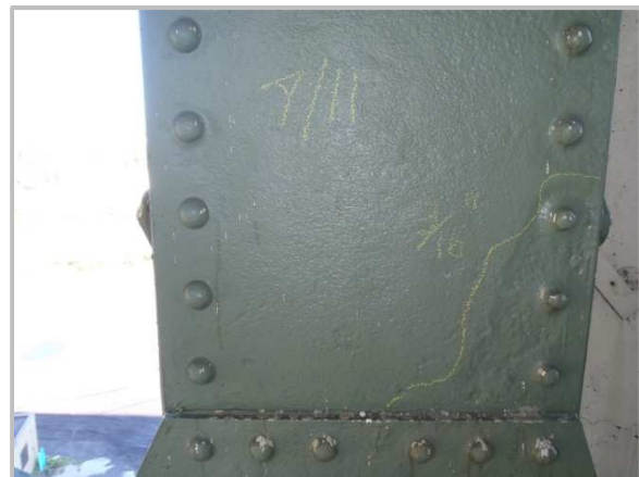
Photo 22 – AL65-AU65 with 3/16" pitting on south web plate along lower chord gusset plate.
