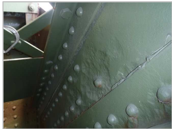
Photo 25 – 3/8" pitting (cleaned and painted) on interior face of the south web plate of member DL35-DU34 between flange angles adjacent to the lower chord gusset plate.
