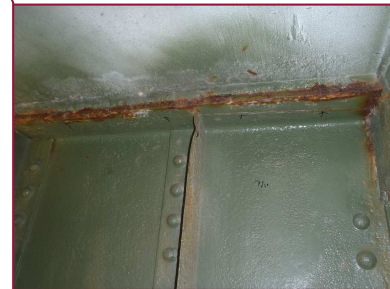
Floorbeam 17 exhibits a lamellar tear approximately five feet long on the bottom of the top flange between Stringer 7 and the interior bearing stiffeners.
