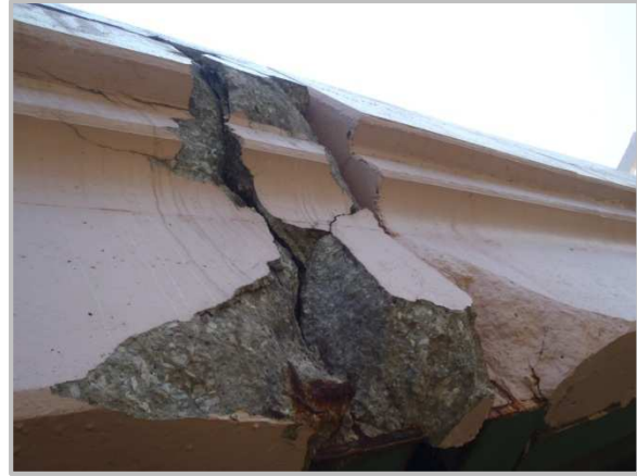
Photo 8 – Spall with exposed reinforcing in fascia soffit over Panel Point AU12.
