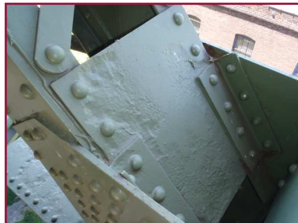
The top batten plate of AL121-AU120 exhibits heavy section loss (cleaned and painted) with isolated locations of paper thin section.
