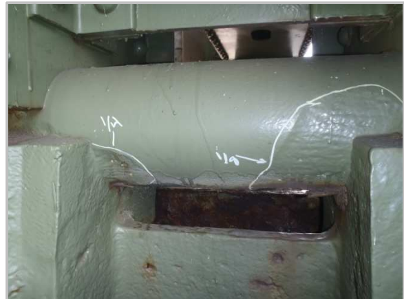
Photo 46 – Section loss up to 1/4" on east face of Pier 18 east bearing at Truss A.
