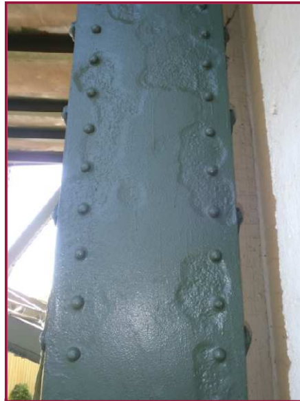
The north and south web plates of BL0-BU0 exhibit 1/8" to 1/4" deep pitting (see Section A-A).
