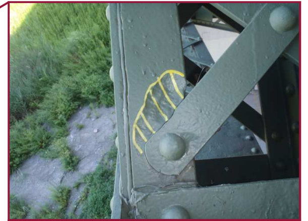
Member AL131-AU132 exhibits 1/4" pitting for the full width of the north top flange horizontal angle leg adjacent to the cover plate.
