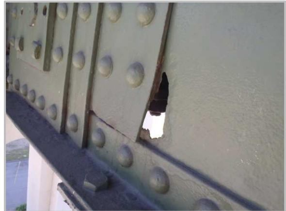
Photo 10 – 4" high by 5" wide holed-through section in south web plate of member CL113-CL114 near CL113 pin location.
