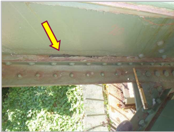
Photo 31 – Holed-through section of DL0-DL1 north web plate 24" long by 2" high adjacent to gusset plate DL0N.
