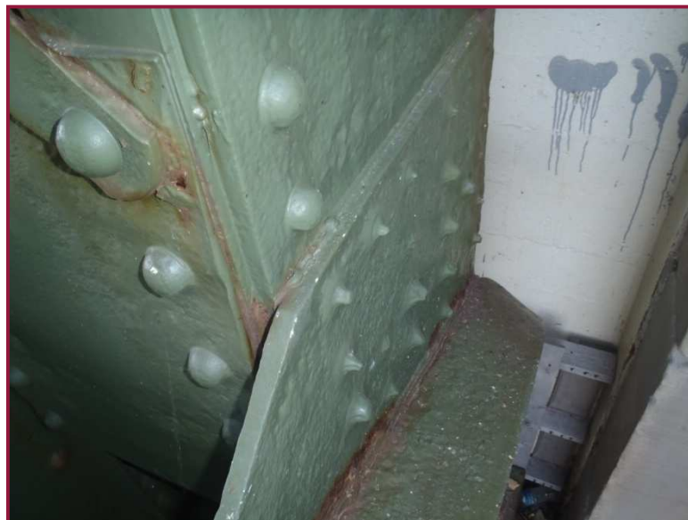
Gusset plate AL0N rivets above the lower chord exhibit section loss up to 100% on 17 of 25 rivet heads. 12 of 25 rivet heads exhibit at least 50% loss.
