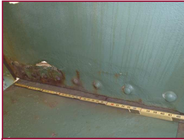
section of 1/8" to bottom of the north side, approximately 9" high and
