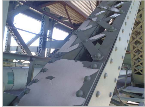
Photo 49 – Isolated paint peeling on diagonal member CL106-CU107 in Span16.
