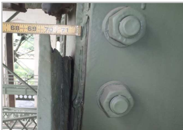
Photo 43 – 1 1/2" pack rust between CL58S free edge and CL58-CU58 south web plate.
