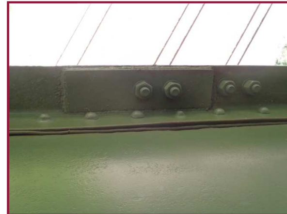
welded plate retrofits on the north side of the outstanding leg of DL5-DL6.
