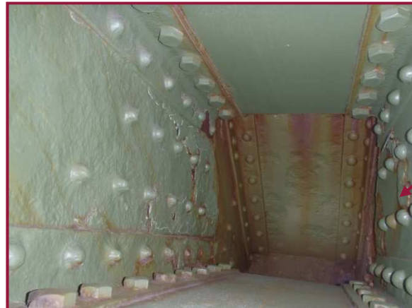
The interior web plates of AU96-AL97 exhibit laminate rust with 1/8" loss on the interior, as well as isolated areas of 3/16" pitting on the interior and exterior faces of this member.
