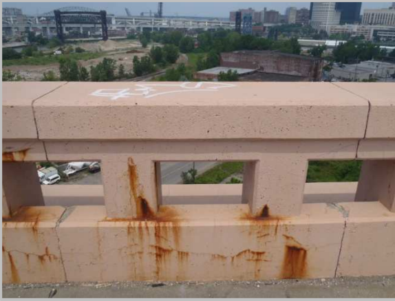
Photo 7 – Typical parapet hairline cracks with rust staining.
