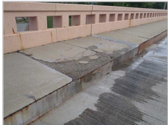
Photo 5 – Shallow spalls in north sidewalk surface adjacent to East Abutment joint.
