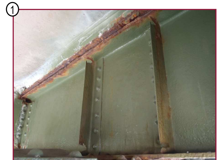
The bearing stiffeners on the east face of Floorbeam 100 adjacent to Truss A exhibit isolated locations of 100% section loss.
