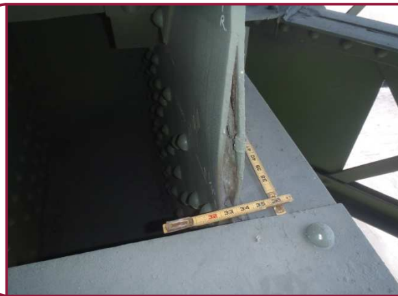
Detail view of lamellar tear taken in 2011.
