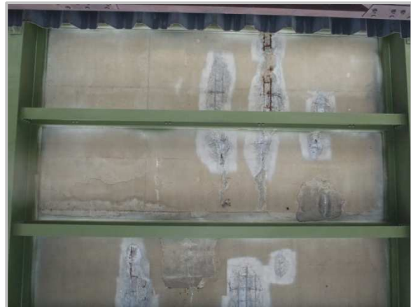
Photo 2 – Roadway deck underside in Span 16 between Floorbeams 107 and 108. Note several spalls have been sealed.
