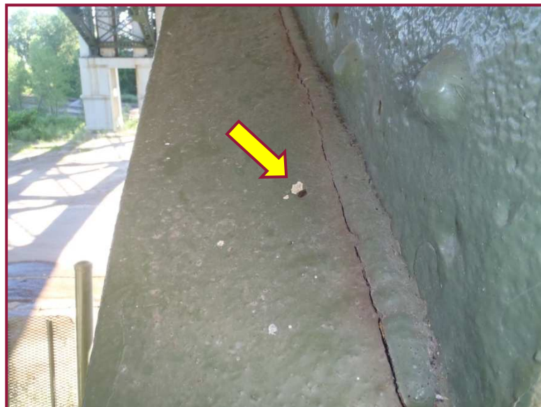
The north top and bottom flange angles adjacent at CL0 exhibit up to 100% section loss as large as 1/2" diameter within the bounds of the gusset plate.
