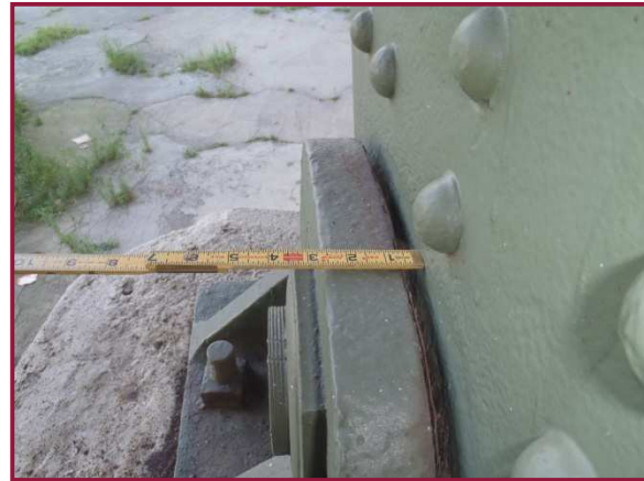
The truss bearing at AL127 exhibits impacted rust up to 5/8" between the gusset plates and bearing casting (north side shown).
