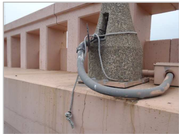
Photo 60 – Light post above AU120 with exposed wires and broken access box cover.
