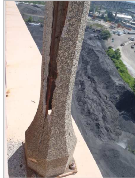
Photo 59 – 8' high by 6" wide spall with exposed rebar and cracking in Span 10 light pole.
