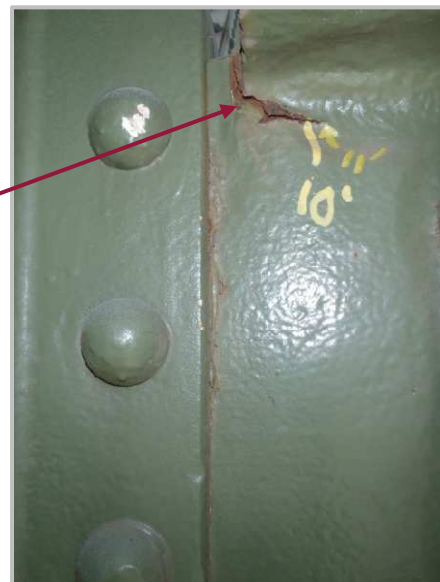
Photo 18 – Crack in utility deck floorbeam at connection to gusset plate CL36N.
