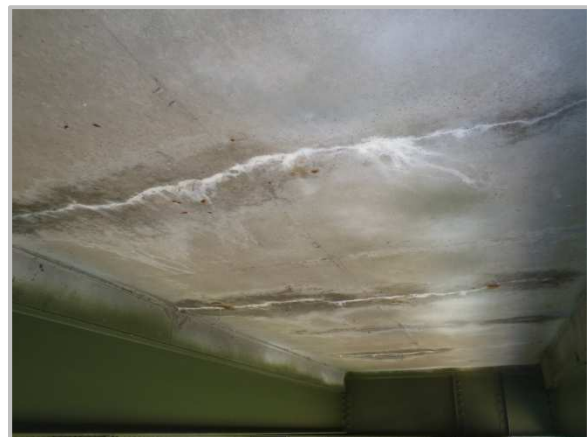
Photo 3 – Transverse cracks with efflorescence and stalactite formations between Floorbeams 28 and 29.
