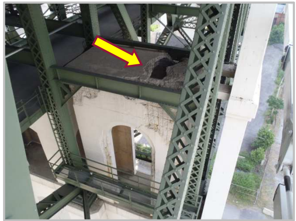
Photo 53 – Pier 15 tower between Truss A and Truss B with 8' by 3' hole in top.
