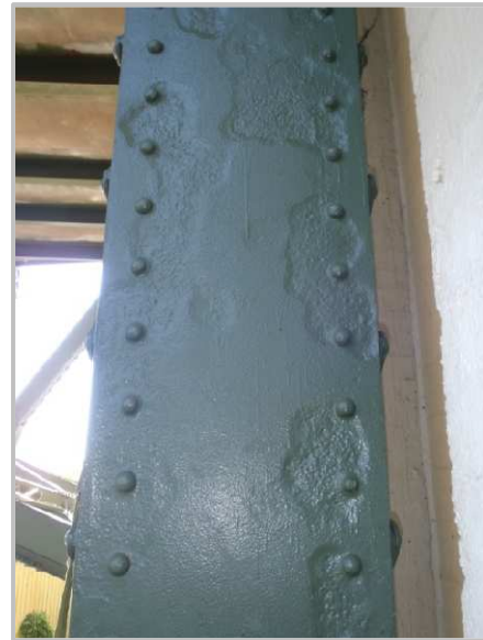
Photo 21 – 1/8" pitting on member BL0-BU0 with isolated 1/4" pitting over the lower half of the north web plate.
