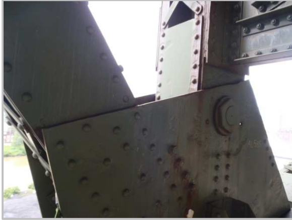
Photo 48 – Active minor surface corrosion at Panel Point AL58.
