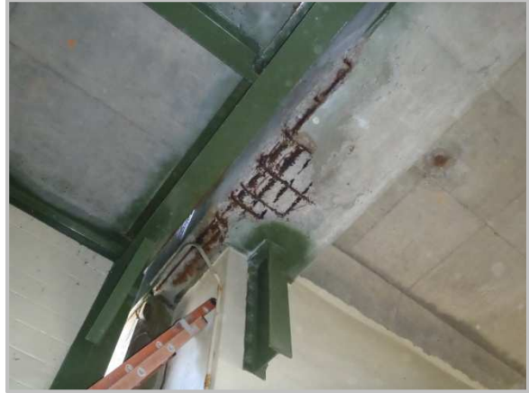
Photo 16 – Spall with exposed reinforcing at north end of west end floorbeam in Pylon Span 5.
