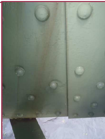
The DL52-DL53 north web plate exhibits an area of 1/4" deep pitting 5" tall (cleaned and painted) along gusset plate DL53N.
