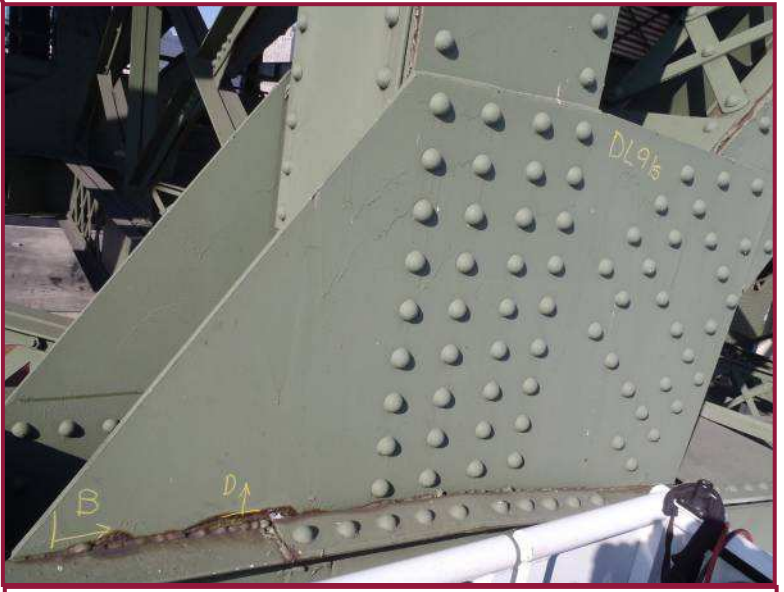
Gusset plate DL91 exhibits conditions typical of the exterior gusset plates throughout Span 14, Truss D, with activating rust along the interface at the lower chord and associated minor pitting (Photo taken 2010).
