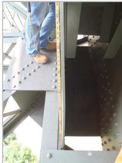
Photo 44 – 1/2" bow on east free edge of CL43S. Note that this plate does not meet the edge stiffness requirements of AASHTO 10.16.11.3
