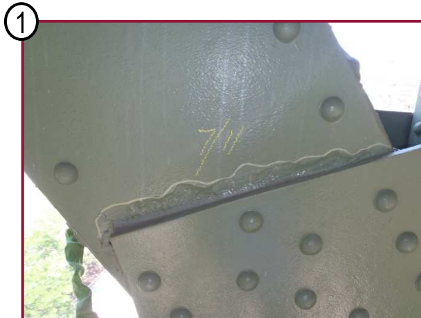
The south exterior web plate of AL113-AU112 exhibits 1/4" deep pitting 1" tall along the interface with the lower chord gusset plate.
