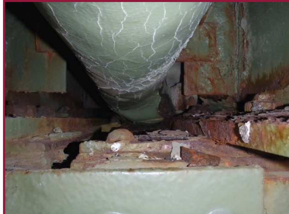
Floorbeam 35 exhibits active corrosion of the bottom flange and adjacent web and vertical stiffener plates with up to 1/16" deep pitting. The joint trough at this location has failed with water and debris leaking onto the superstructure elements.
