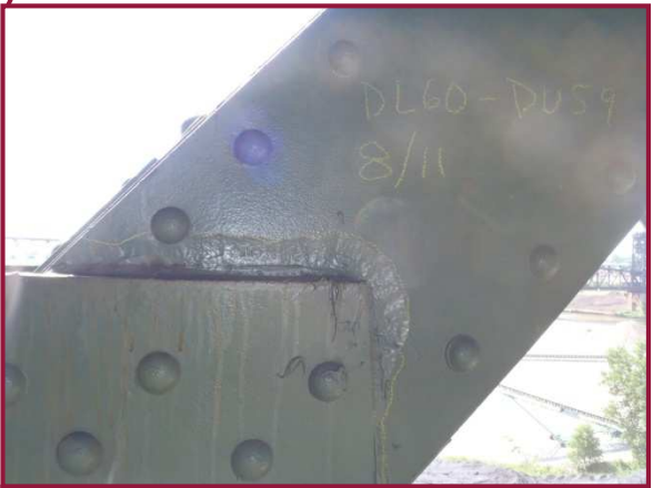
The north web plate of member DL60-DU59 exhibits 1/8" pitting (cleaned and painted) for the full height of the section along the interface with gusset plate DL60N.
