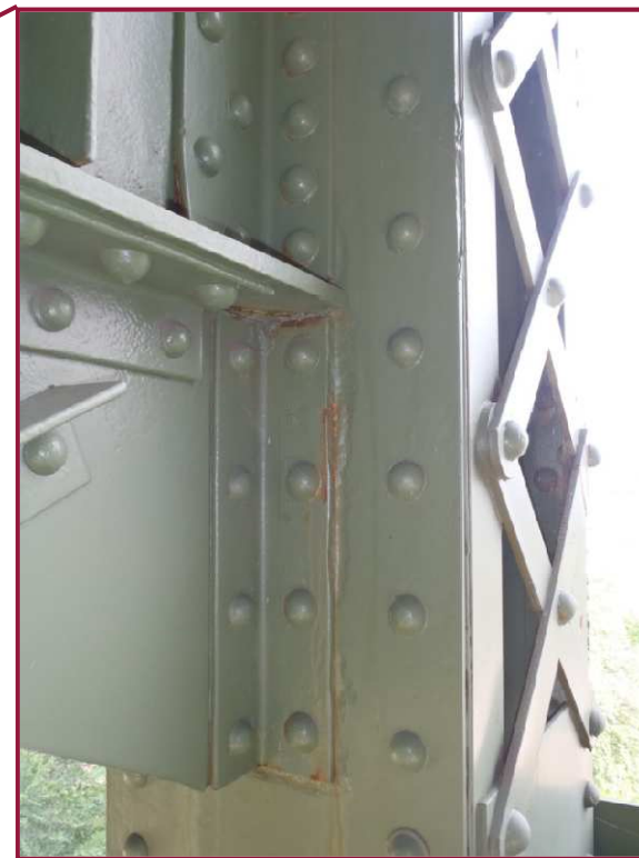
The north web plate of vertical member AL27-AU27 exhibits typical 1/8" pitting around the sway brace connection.
