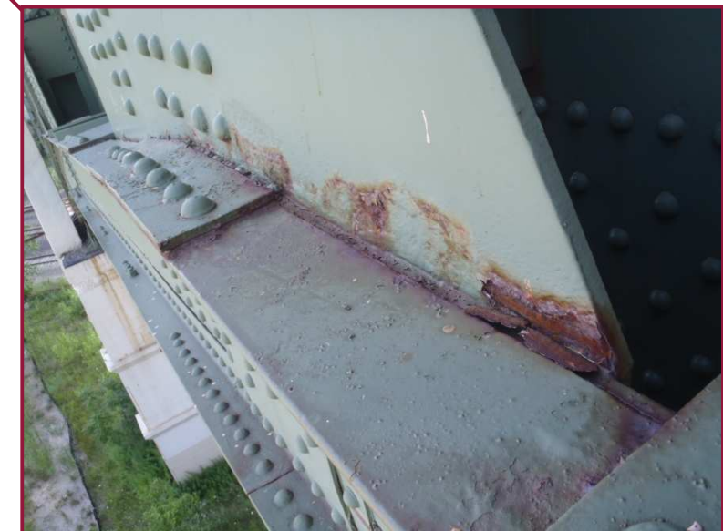
There is active corrosion on gusset plate AL5N along the top flange angle of AL4-AL5 with associated 1/16" pitting.
