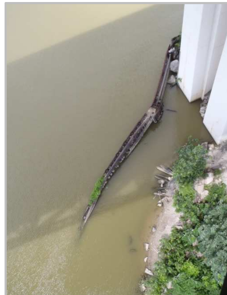
Photo 55 – South half of the east bank fender system collapsed toward river centerline.
