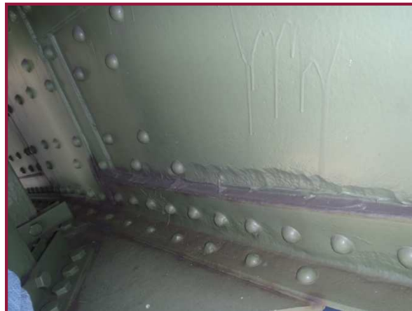
The south web plate of member AL77-AL78 exhibits 1/4" pitting approximately 2" high along the bottom flange angle.
