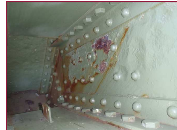
Pitting with active surface rust to the interior south web plate adjacent to gusset plate AL113S
