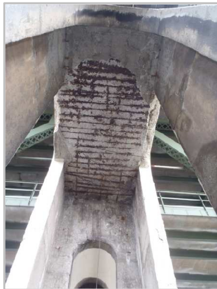
Photo 54 – Pier 12 tower with 20' by 5' spalled area with exposed reinforcing.
