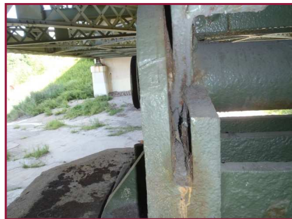
The truss bearing at BL127 exhibits impacted rust between gusset plate BL127N and the bearing casting.
