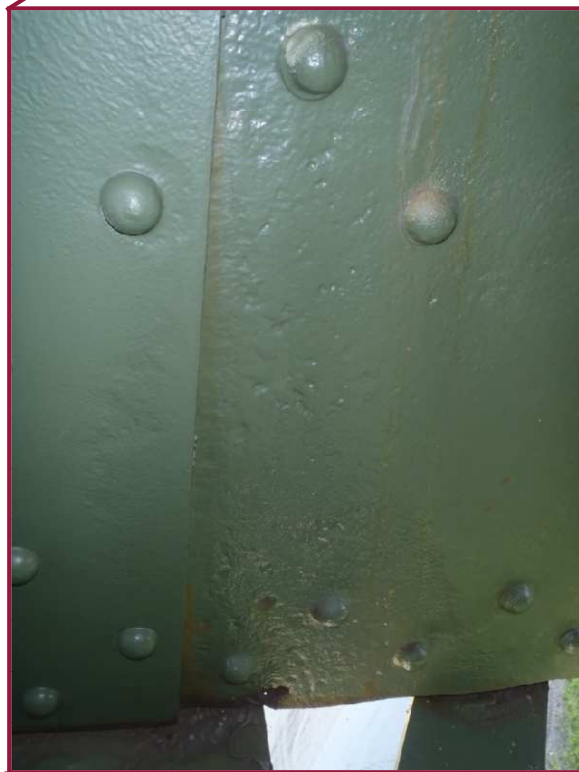
The north and south web plates of chord member AL24-AL25 exhibit 3/16" pitting over the full height of the plate along the interface with Panel Point AL25 gusset plates, with an isolated 1" diameter hole in the south plate (south plate shown).
