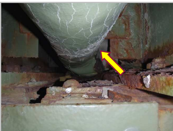
Photo 9 – Isolated torn neoprene trough and active corrosion to framing members adjacent to Panel Point DU35.
