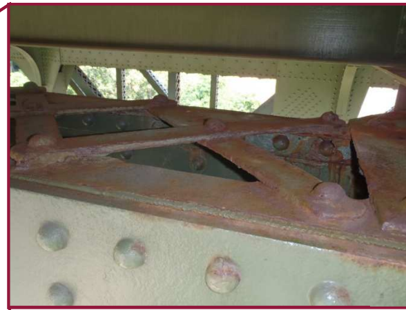
extensive rust and corrosion
