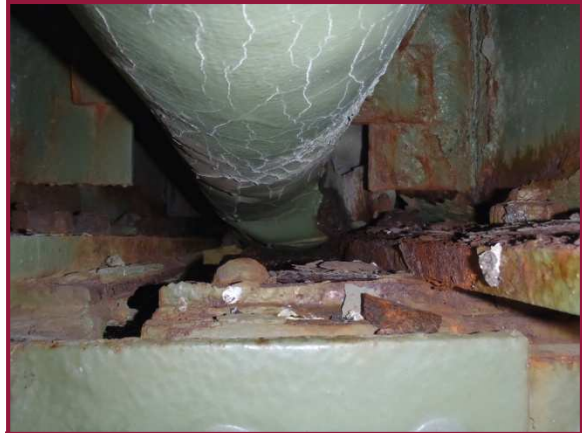
Floorbeam 35 exhibits active corrosion of the bottom flange and adjacent web and vertical stiffener plates with up to 1/16" deep pitting. The joint trough at this location has failed with water and debris leaking onto the superstructure elements.
