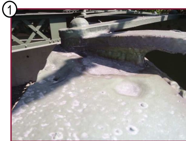
The north top flange angle of CL131-CL132 exhibits a 3" diameter area of section loss up to 100%, including one 3" diameter hole, in the outstanding leg. Also note the heavy pack rust between the flange angle and lacing bar.
