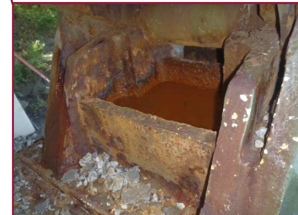
The bearing components at AL131 exhibit 1/8" pitting and activating surface rust throughout. The east side of the bearing contained standing water at the time of the inspection with moderate to heavy rusting in this area.
