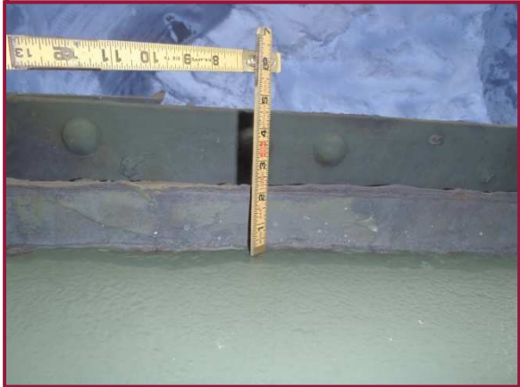
The lower chord member DL69-DL70 exhibits pack rust up to 2" thick between the north web plate and the lower flange angle. Pitting up to 3/16" was noted on the north web plate along the flange angle.
