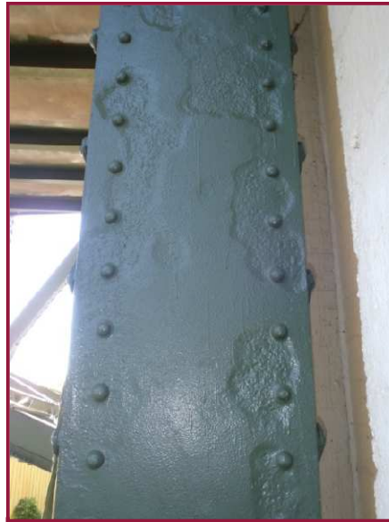
The north and south web plates of BL0-BU0 exhibit 1/8" to 1/4" deep pitting (see Section A-A).
