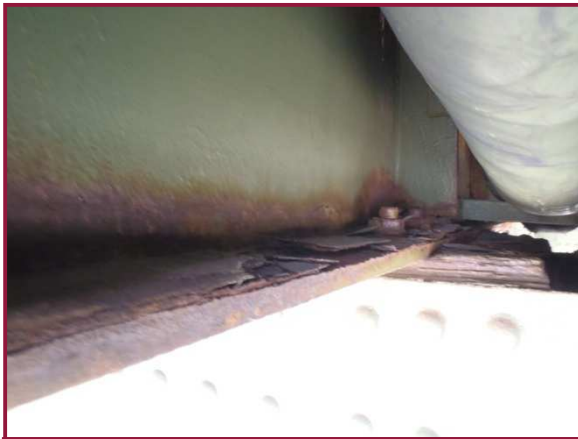
The west bottom flange of Floorbeam 97' at AU97 exhibits active laminate rust with 1/16" section loss.
