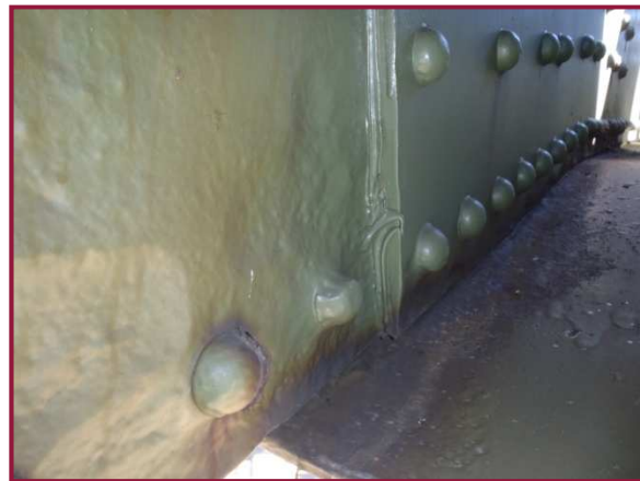
The north web plate of member DL119-DL120 exhibits 1/4" pitting over the bottom 1/4 of the height along the gusset plate interface. Pack rust has built up between this web plate and gusset plate DL120N.
