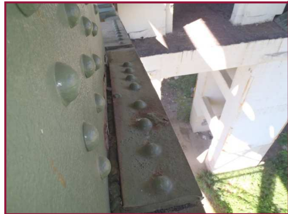
The bottom flange angle splice plate at CL11 is bowed out approximately 1-1/2" due to heavy pack rust.
