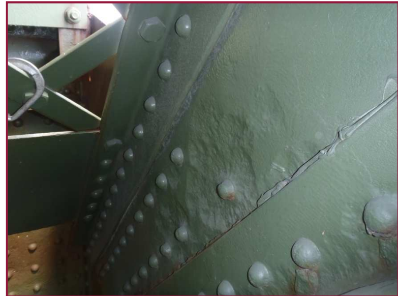
The south web plate of DL35-DU34 exhibits 3/8" deep pitting on the interior face between the flange angle legs. This area is located approximately 1' above the lower gusset plate (see Section A-A).
