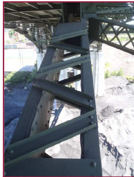
Pack rust is showing signs of reactivation between lower chord web plates and flange angles.
