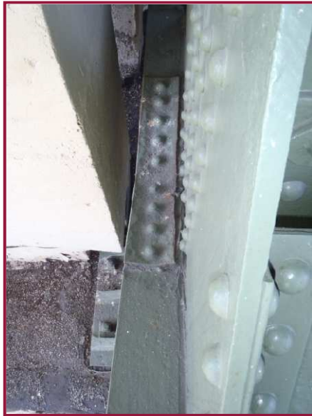
The top flange splice plate at BL9 exhibits 1/8" pitting.
