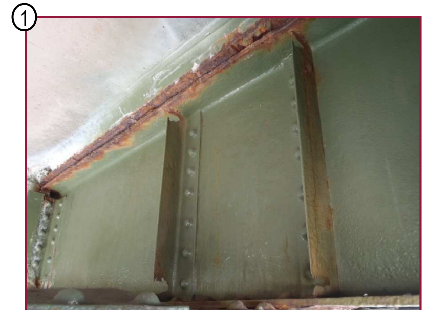
The bearing stiffeners on the east face of Floorbeam 100 adjacent to Truss A exhibit isolated locations of 100% section loss.
