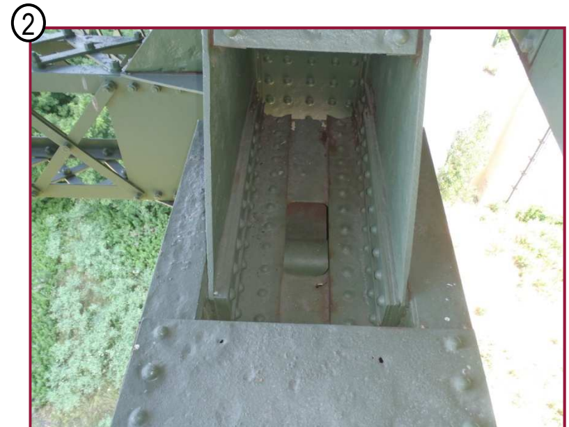
The pin diaphragm plate for lower chord BL16-BL17 at BL17 exhibits 3" diameter holed through sections at the east end. There are isolated holes up to 3/4" diameter in the top lower chord batten plate near this location, as well as minor pitting to top flange angles within the gusset plate bounds.
