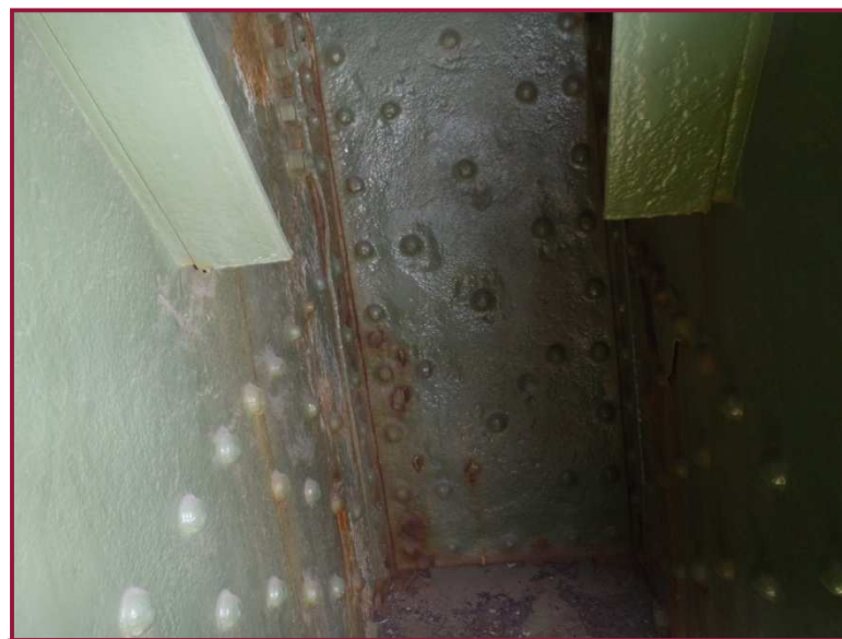
The internal diaphragm plate at CL12 exhibits heavy pitting with active corrosion around the rivet heads and along the edge of the plate at the gusset plate interfaces.
