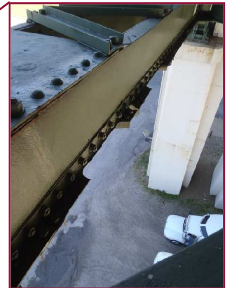
The south bottom flange angle of member AL100-AL101 exhibits isolated holes with sections cut out of the outstanding legs.
