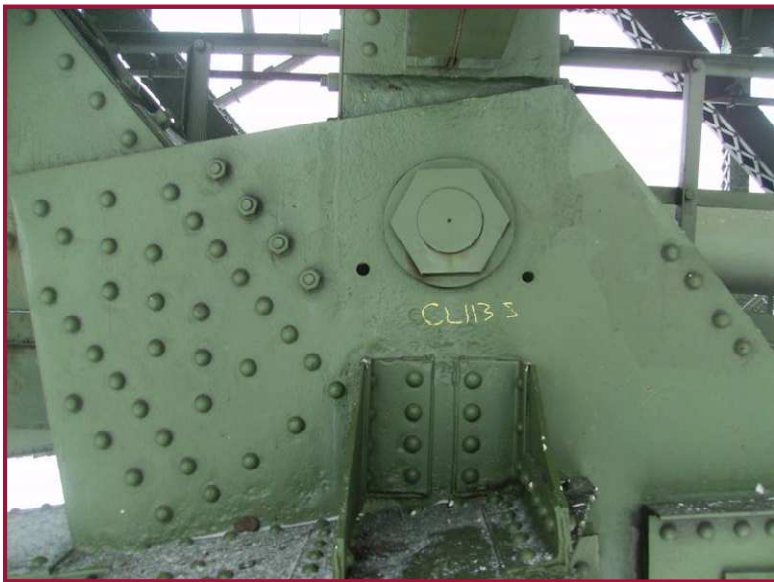
hibits heavy pitting throughout areas isolated among the more deepest pitting is found along lower chord top flanges and (Photo taken 2010).
