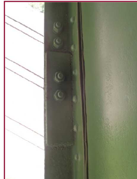
DL11-DL12 has a welded retrofit plate on the outstanding leg of the north bottom flange. A similar plate is located on the south bottom flange at this location.
