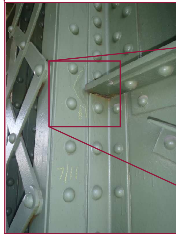
The north web plate of vertical member BL5-BU5 exhibits 1/8" pitting around the sway brace connection.
