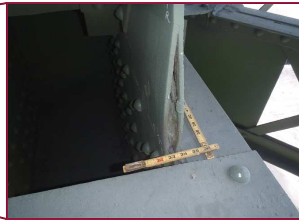
Detail view of lamellar tear taken in 2011.
