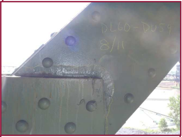
The north web plate of member DL60-DU59 exhibits 1/8" pitting (cleaned and painted) for the full height of the section along the interface with gusset plate DL60N.
