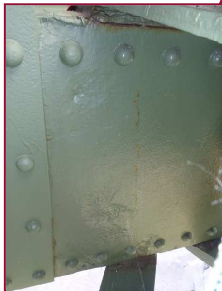
The south web plate of AL48-AL49 has heavy pitting up to 1/4" deep for approximately half the web height near AL49. Similar conditions are found at AL51.
