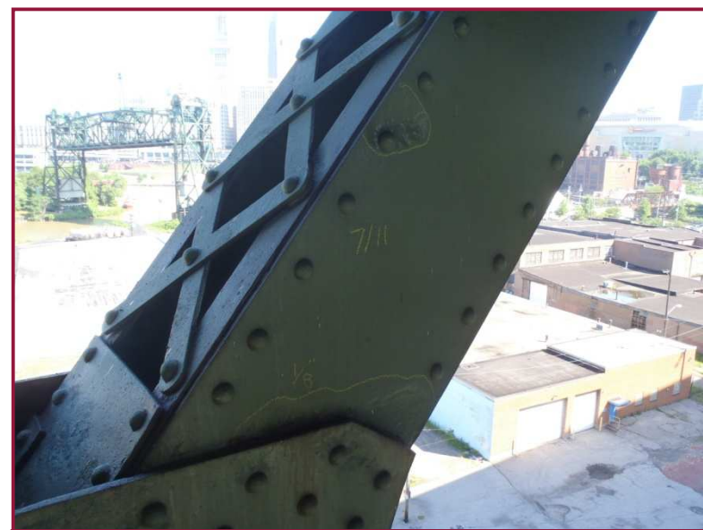
The south web plate of member AL83-AU84 exhibits 1/8" pitting along the lower chord gusset plate and in isolated locations along the member.
