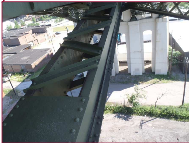
The lower chord south web plate exhibits pitting up to 3/16" deep pitting along the bottom flange angle in the lower half of the plate. The pitting extends approximately 3/4 of the length of CL88-CL89.
