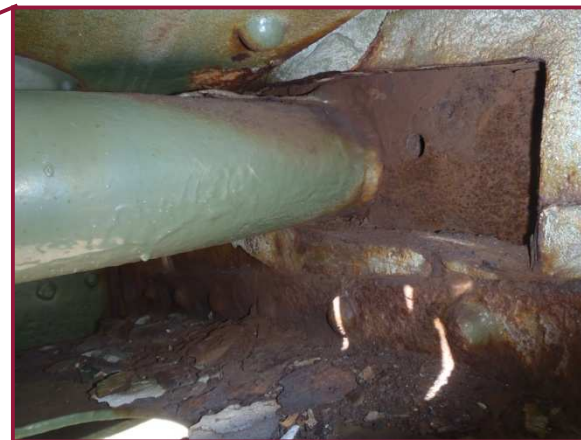
Note active corrosion and wear on north DL12-DL13 lower chord sliding pin at DL12.
