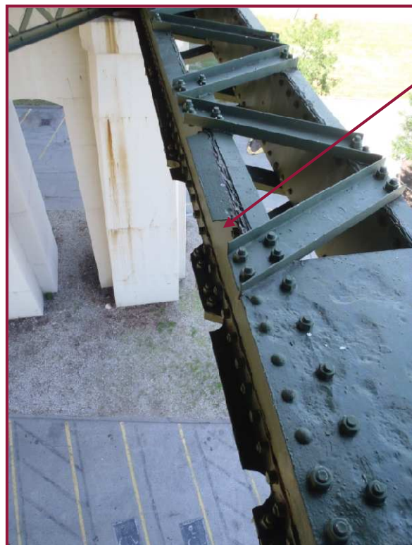
Lower chord member AL112-AL113 exhibits advanced section loss at several components of the built-up member at AL113. These losses are depicted in Section A-A. Note multiple retrofits at this location.
