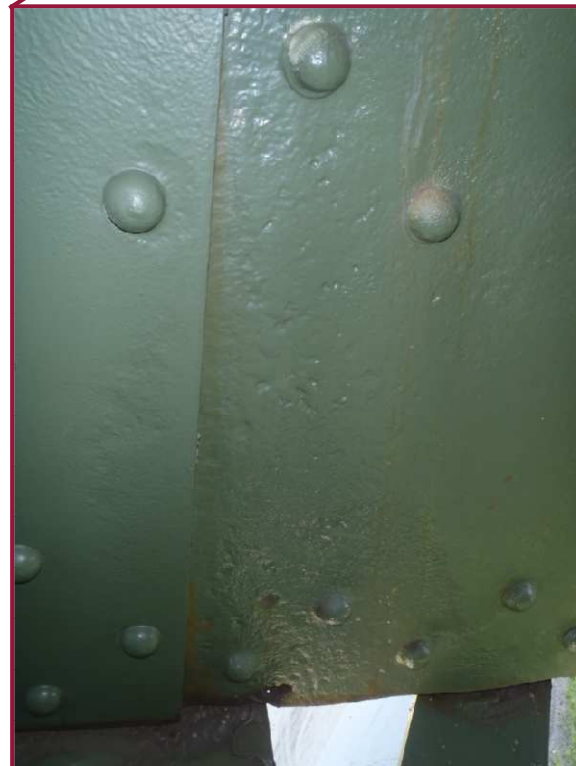
The north and south web plates of chord member AL24-AL25 exhibit 3/16" pitting over the full height of the plate along the interface with Panel Point AL25 gusset plates, with an isolated 1" diameter hole in the south plate (south plate shown).
