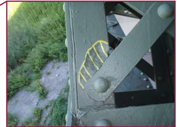
Member AL131-AU132 exhibits 1/4" pitting for the full width of the north top flange horizontal angle leg adjacent to the cover plate.
