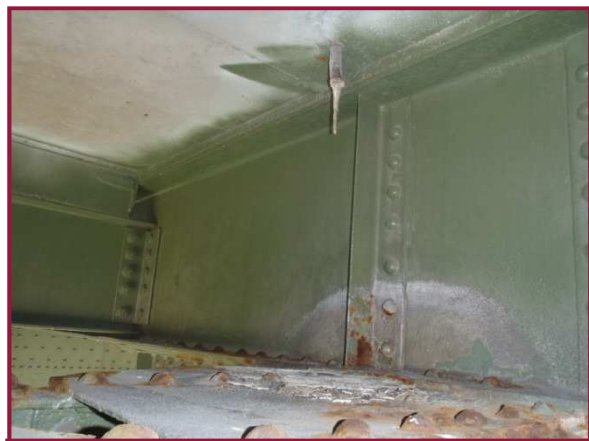
Deck subdrain location on the west side of Floorbeam 47 with 1/16" pitting and active corrosion to the top chord cover plate, lacing bars and flange angles. Note stalactite formation.
