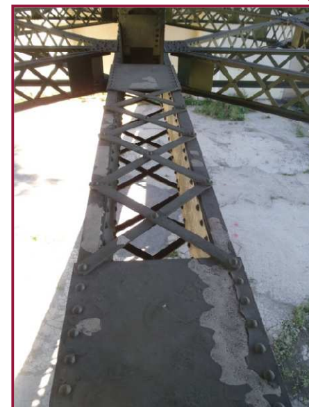
Lower chord BL130-BL131 exhibits extensive areas of peeling paint.
