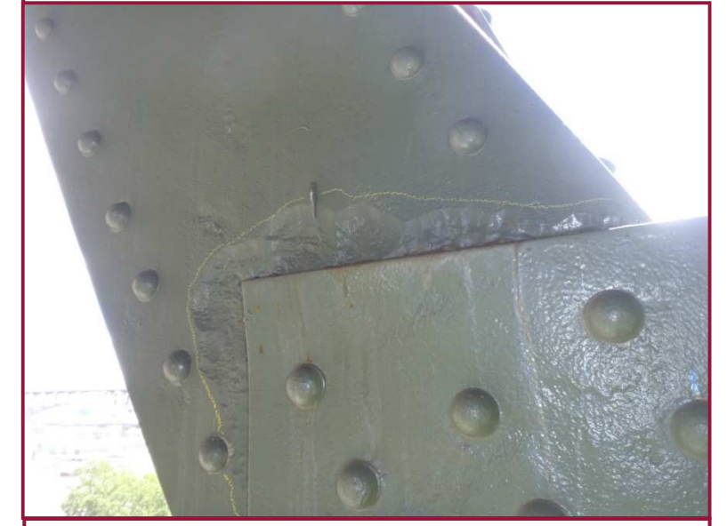
The north web plate of diagonal member DL43-DU44 exhibits 1/4" pitting with isolated 5/16" pitting along gusset plate DL43N for the full height of the section.
