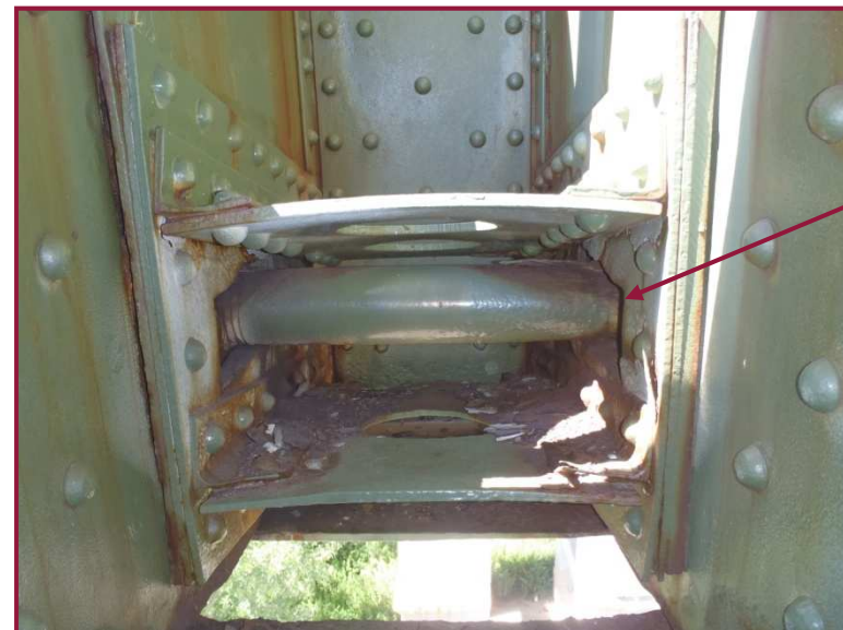
The sliding pins at gusset plate location DL12 are worn. The internal diaphragm between gusset plates above the pin appears to have buckled due to pack rust.
