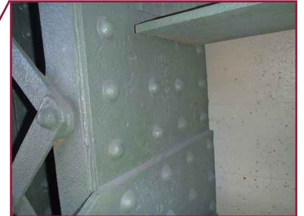
The south web plate of member BL133-BU133 exhibits 1/16" pitting for the full width of the section with isolated 1/8" pitting (cleaned and painted) adjacent to the lower gusset plate.
