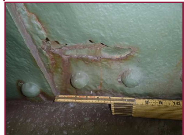
area of DL1-DL2 exhibits a section loss adjacent to area of 1/4" pitting with a
