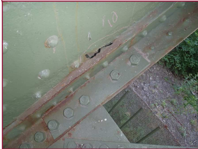
The south web plate of AL0-AL1 exhibits a 2" high by 6" long hole along the bottom flange angle. Note the bolted retrofit plate on the bottom flange outstanding leg at this location.
