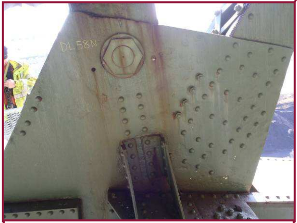
The north gusset plate at DL58 exhibits up to 3/16" pitting, a condition typically found at the expansion locations throughout the structure (Photo taken 2010).
