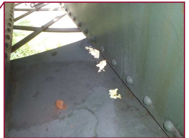
The bottom cover plate at CL133 exhibits a 12" long by 3" wide area with up to 100% section loss.
