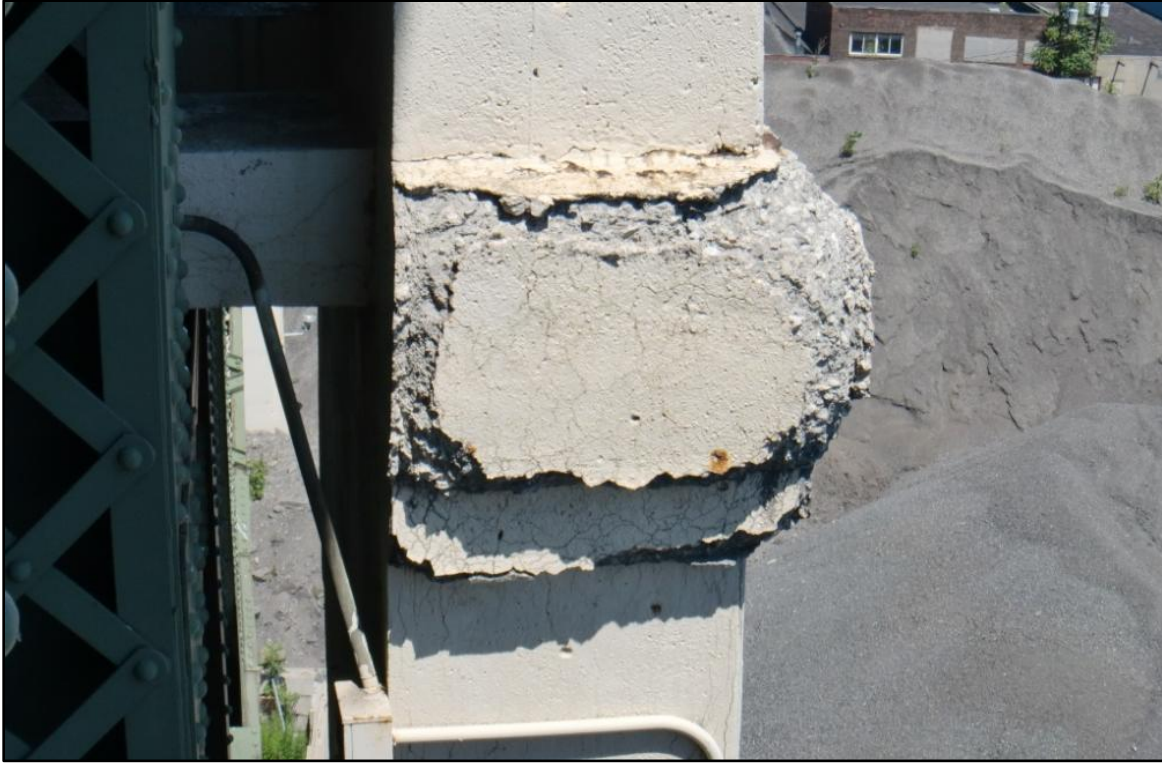
Photo 42 – Scaled Architectural Band, South Pilaster, Pier 8.
