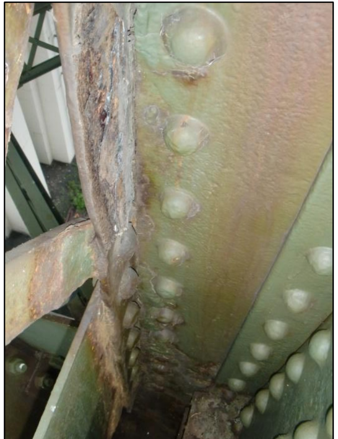
Photo 32 – Active Corrosion on Flange Angle Interior, SE U 17 L 17 , Span 9.
