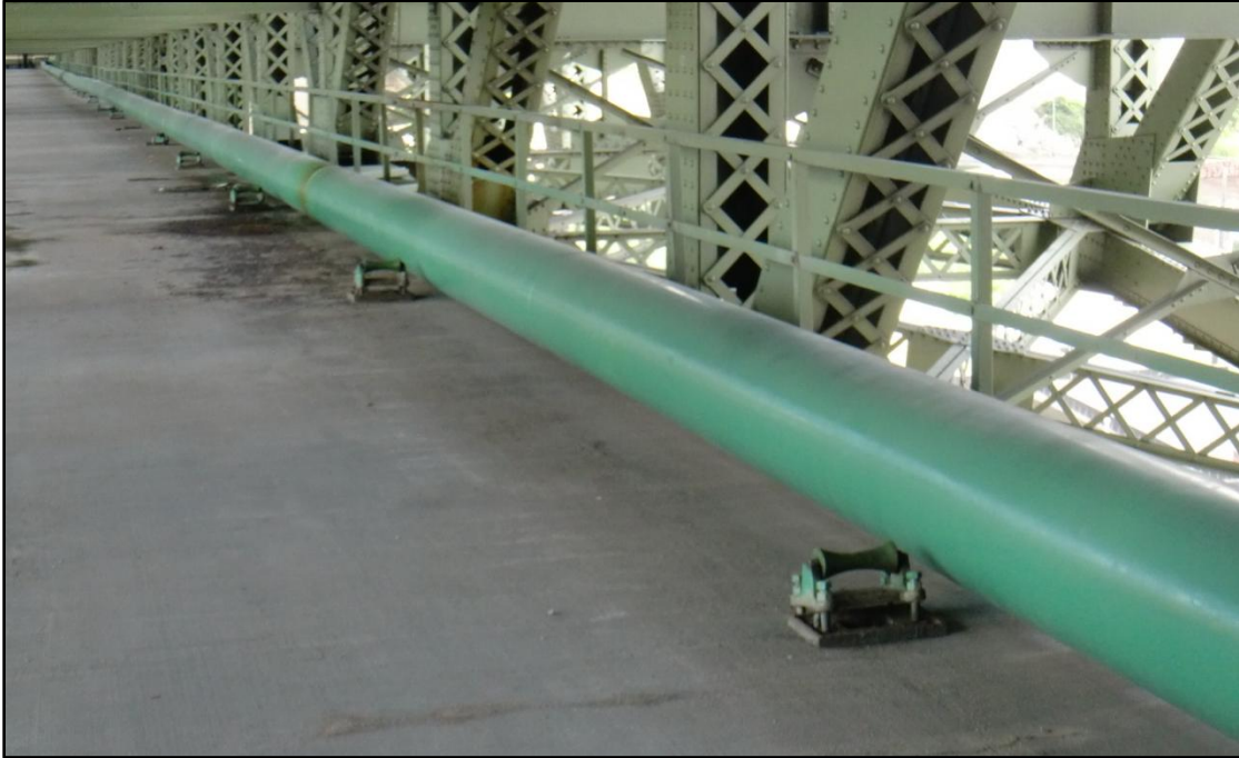
Photo 47 – 200-ft. Long Length of Fallen Gas Line, Span 3.
