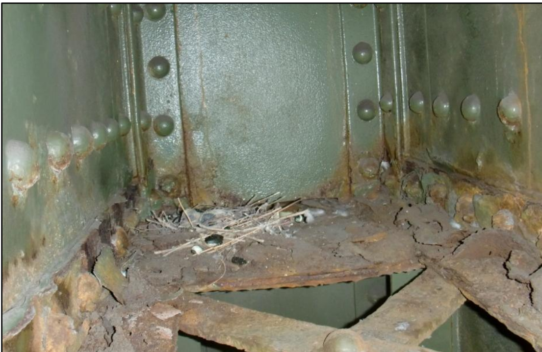
Photo 24 – Isolated Corrosion Beneath Abandoned Pull Box Drain.
