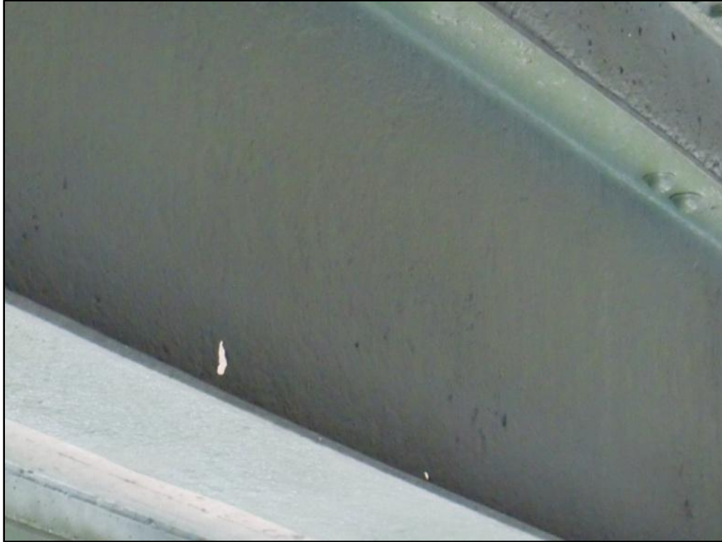
Photo 21 – 2-inch High Web Perforation, Stringer 11, Panel 4, Span 7.
