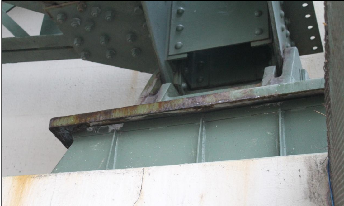
Photo 35 – Active Corrosion on Grease Box Cover, Bearing South L6, Wheeling & Lake Erie Span.
