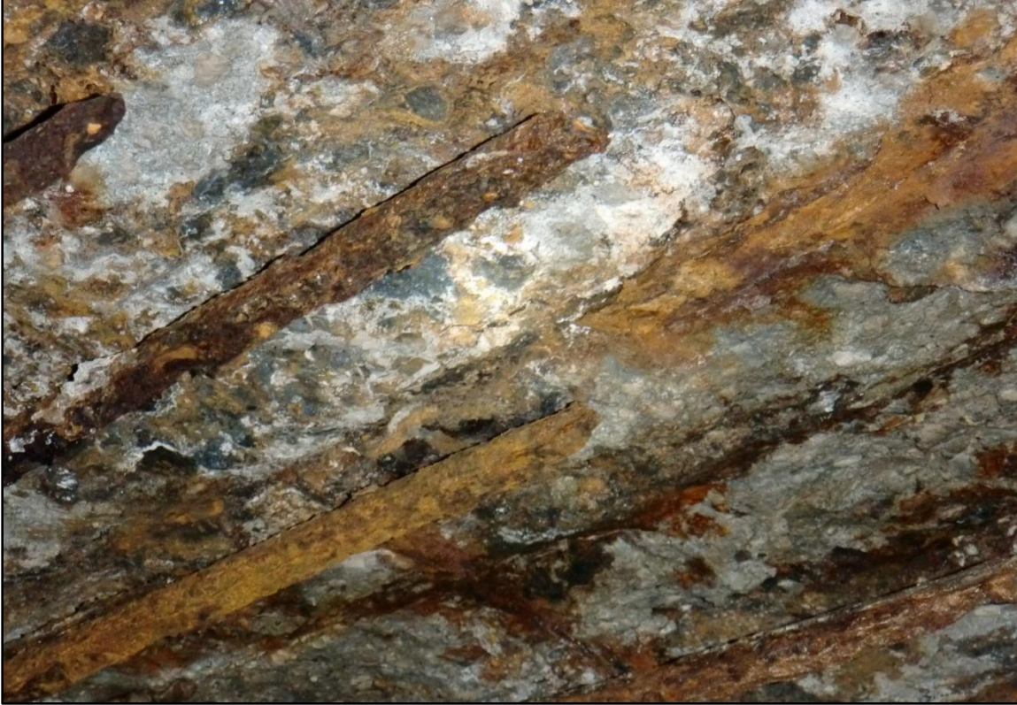
Photo 8 – Close-up of Severed Broken Reinforcement, Panel 3 South, East Subway.
