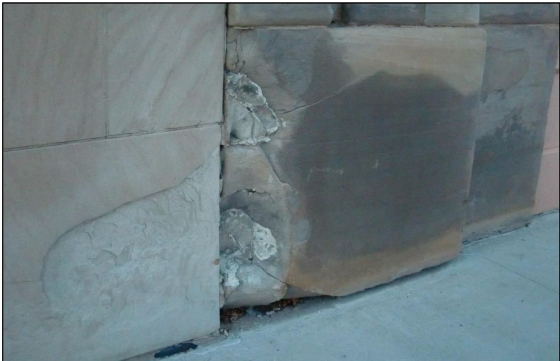
Photo 52 – Spalled Sandstone at Sidewalk, Northeast Pylon.
