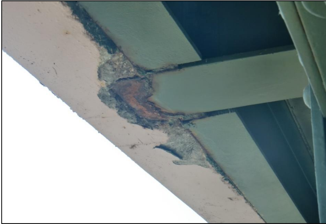
Photo 9 – Fascia Spall at Upper Deck Floor Beam, Span 11, Occurring Since 2002 Sealing.
