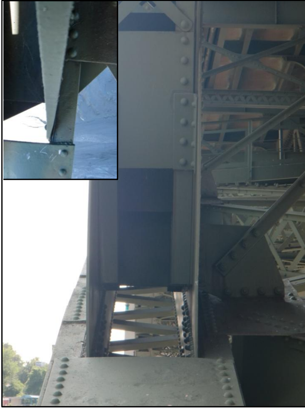
Photo 31 – Slight Bow to North Gusset Plate East Pylon at SE Truss.
