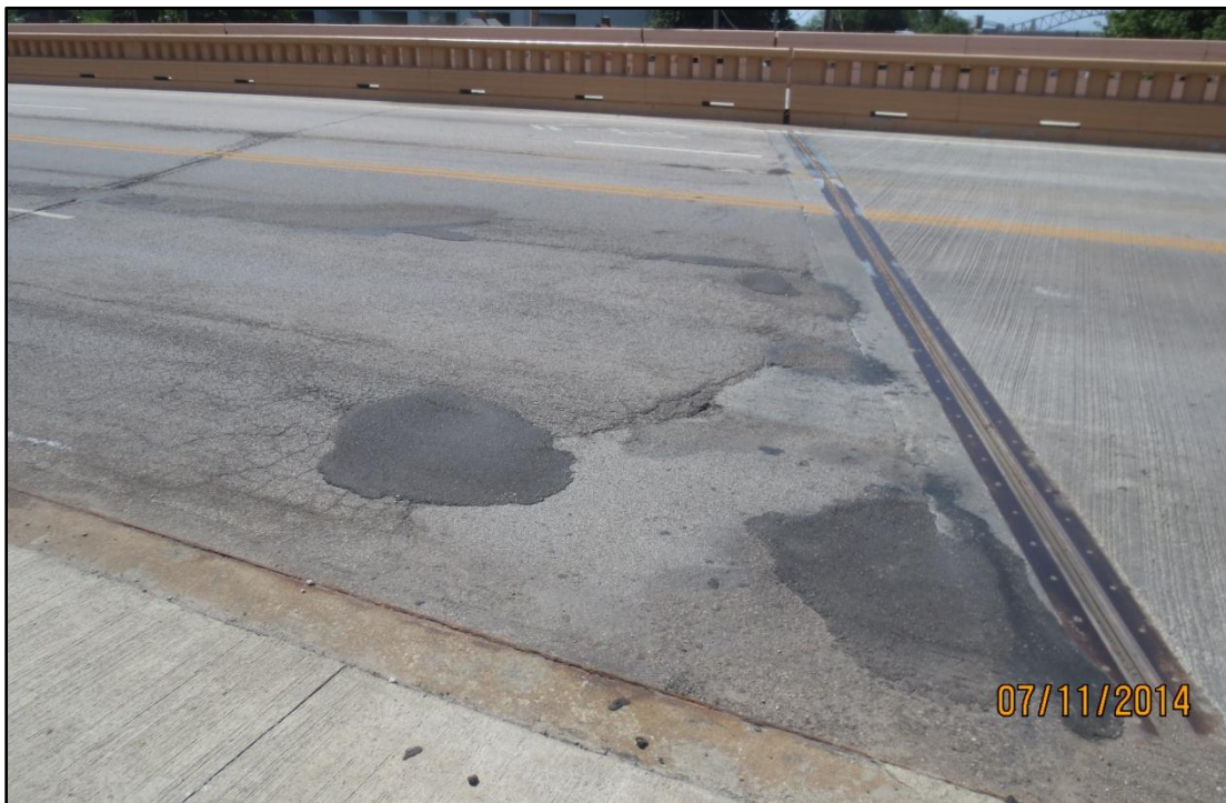
Photo 45 – Moderate Rutting with Patches, West Approach Pavement.
