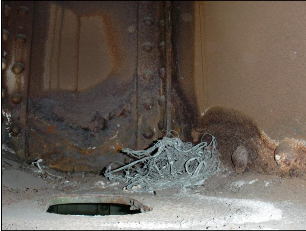
Photo 28 – Typical Corrosion & Debris Inside Lower Chord Between Pier Bearings (Interior of SE L 12 L 13 , Span 7 Shown).
