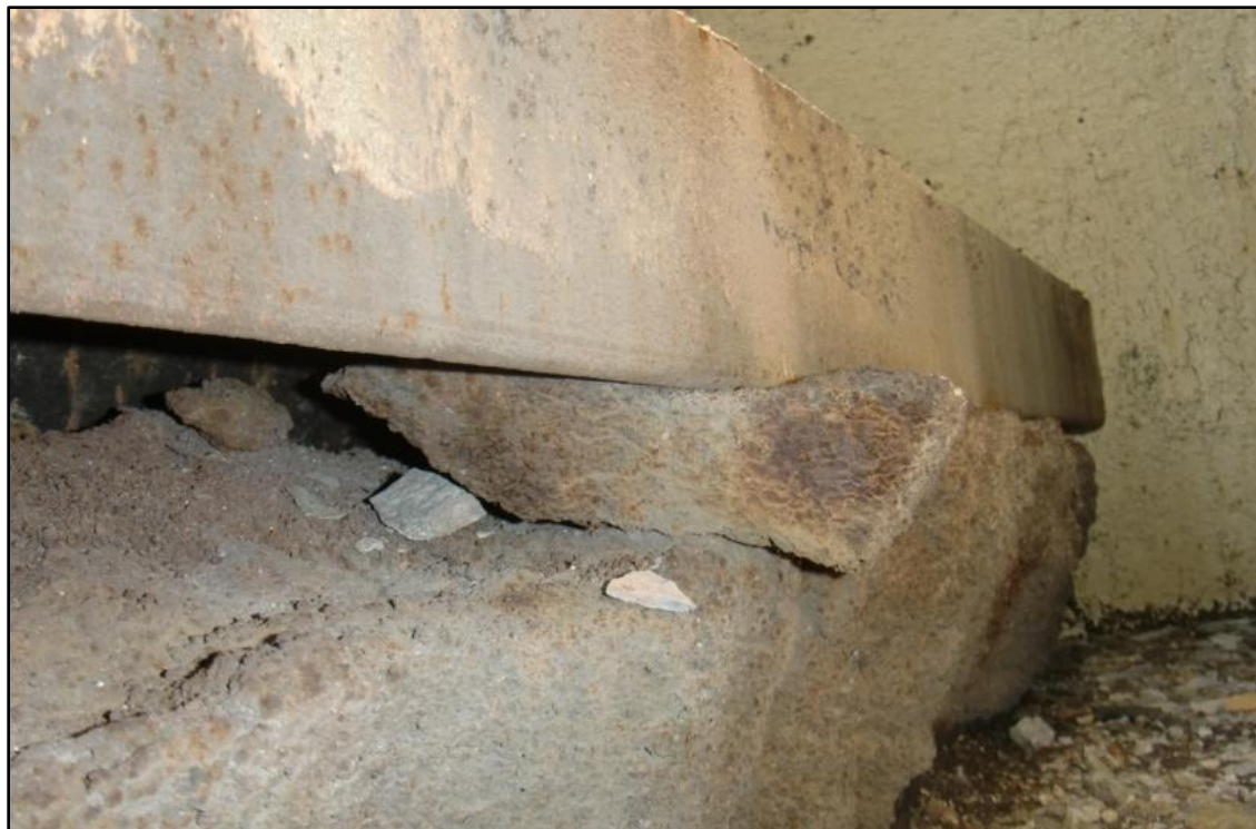
Photo 34 – Steel Shot Accumulation within Expansion Bearing Cover & Rollers, Panel Point L 10 , Span 1.
