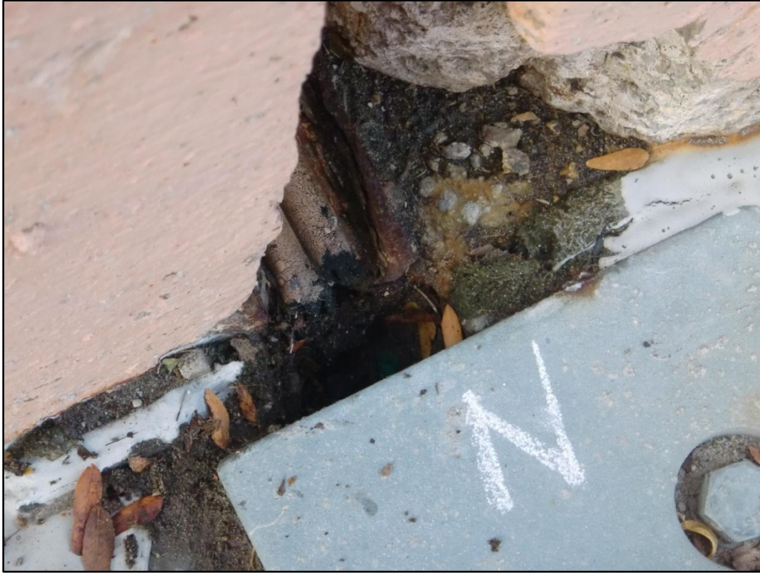
Photo 18 – Cut Expansion Joint Membrane & Open Drainage, North Sidewalk Retrofit.
