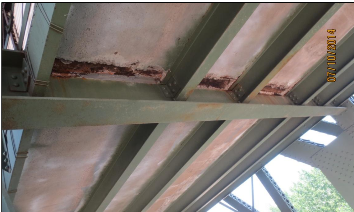
Photo 13 – Water Infiltration through Maintenance Deck & Corrosion of Maintenance Deck Floor Beam Top Flange.
