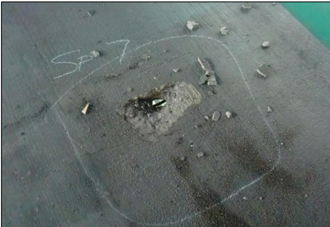
Photo 11 – Recent Popout & Full Depth Spall, Maintenance Deck near Pier 7.
