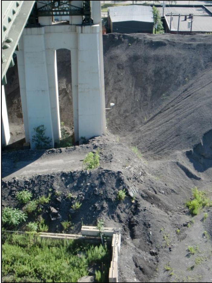
Photo 50 – Encroaching Stockpile on Pier 5 South Exterior Column.
