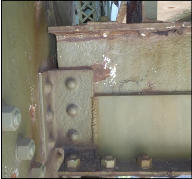
Photo 22A – Crack Propagation. North Interior End of West Face, Maintenance Deck Floor Beam 15, Span 7.
