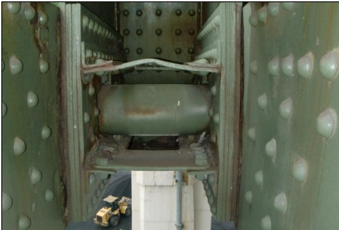
Photo 37 – Frozen Hinge Due to Pack Rust with Buckled Diaphragm, SE L 15 , Span 7.
