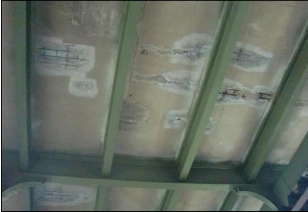
Photo 4 – Corrosion on Steel Reinforcement with Missing Sprayed-On Cathodic Protection.
