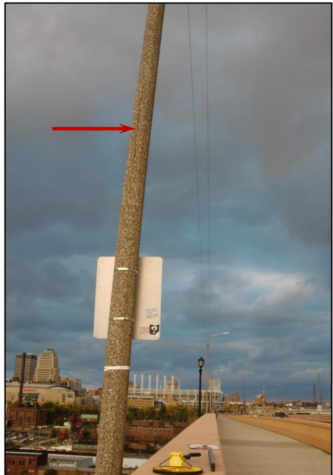
Photo 20 – Leaning Concrete Light Pole with Open Vertical Crack (at Red Arrow), Span 8, North Fascia (Light Standard No. 5N).
