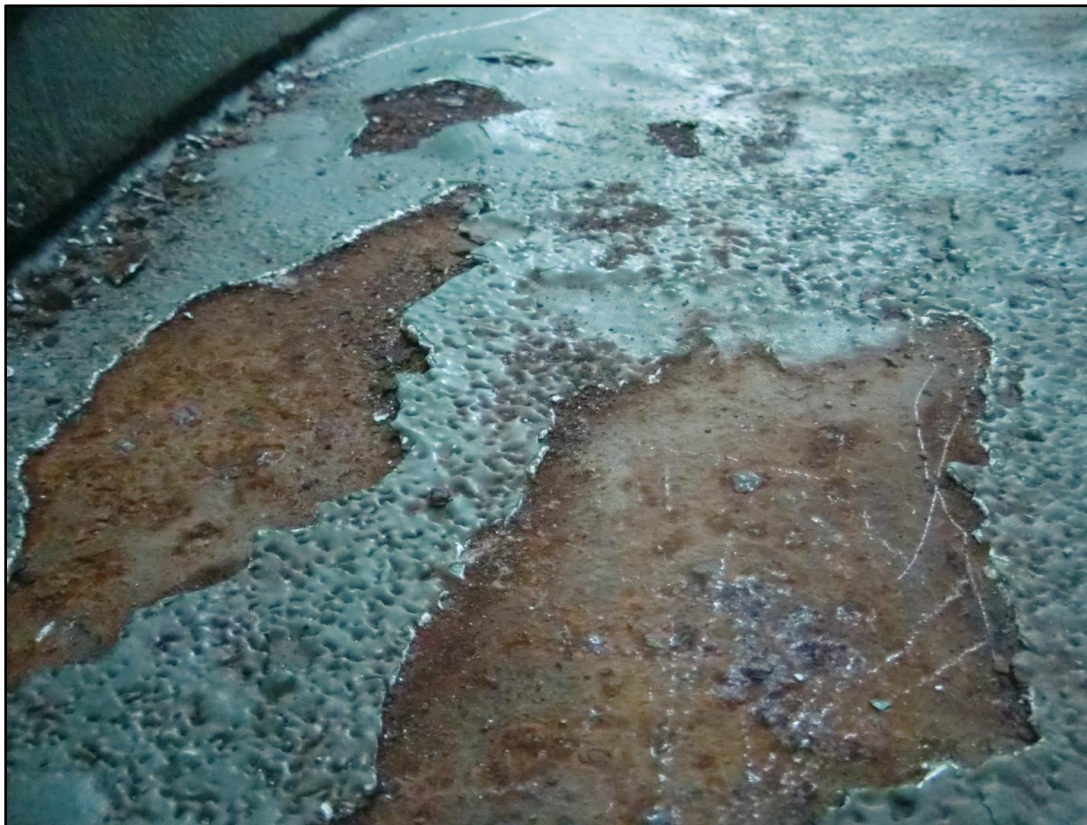
Photo 35 – Poorly Prepped Steel & Locally Failed Protective Coating System.
