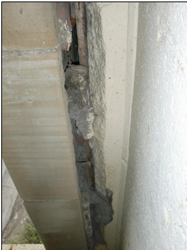
Photo 39 – Backwall Loss & Missing Anchorage for East Pylon Sandstone Facing.
