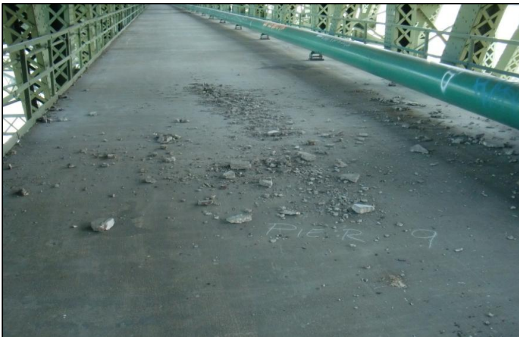
Photo 3 – New Fallen Concrete from Upper Deck, Span 9.
