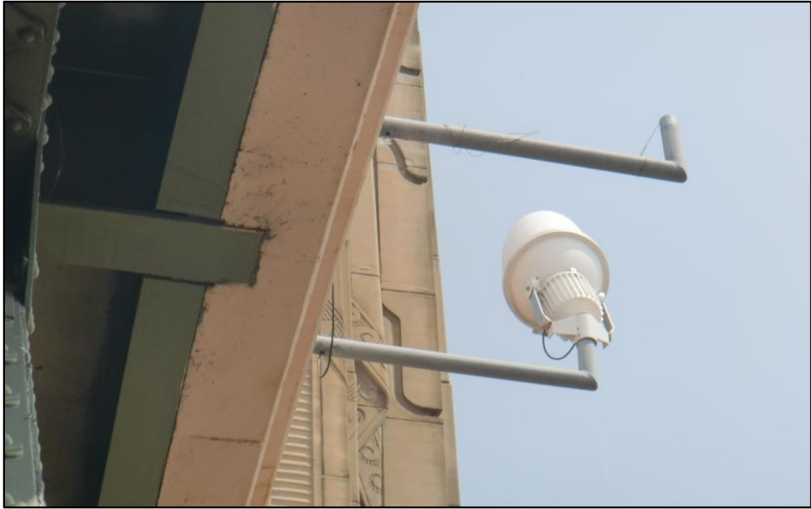
Photo 51 – Missing Architectural Spot Light, West Face, South East Pylon.
