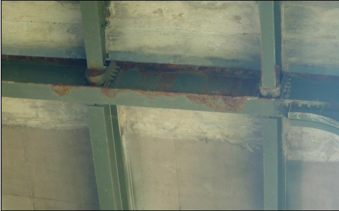
Photo 34 – Protective Coating System Failure below Upper Deck Joint F3, Spans 5 & 6.
