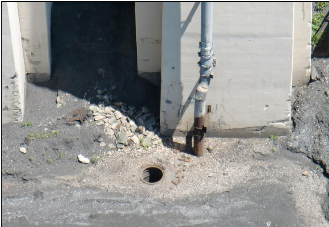
Photo 17 – Missing Manhole Cover, Pier 6 SE Column.
