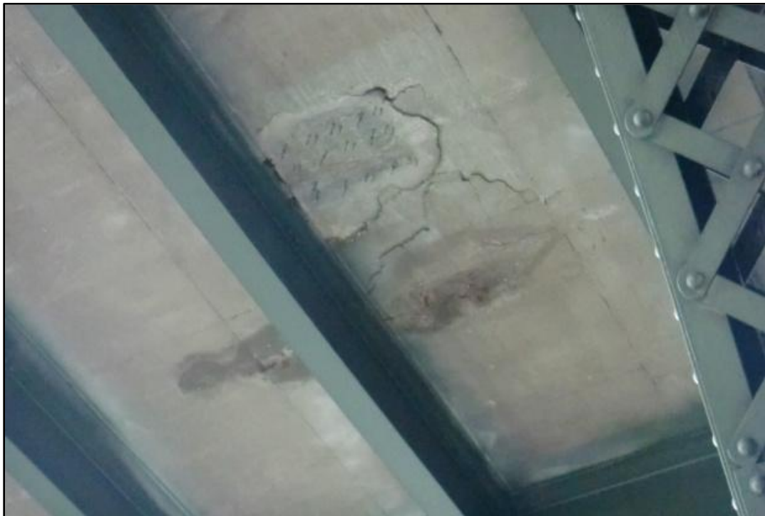
Photo 5 – Deck Delamination Adjacent to 2001 Full-Depth Patch.
