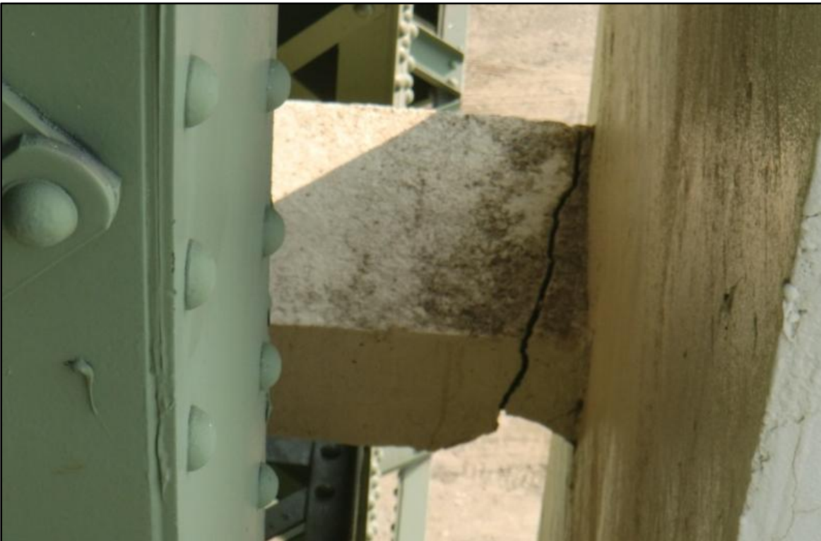
Photo 43 – Full Depth Crack, East Bracket, Pier 1 South Pilaster.
