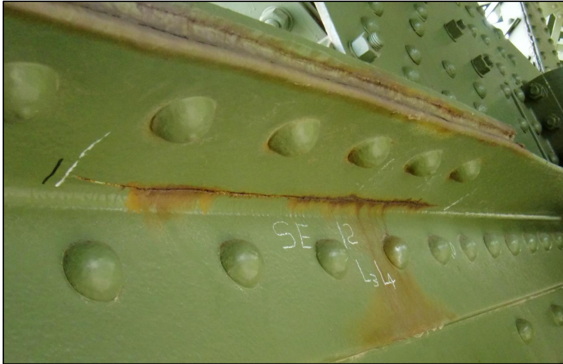
Photo 27 – Stress Corrosion Crack, Top North Flange Angle, SE L 3 L 4 , Span 12.
