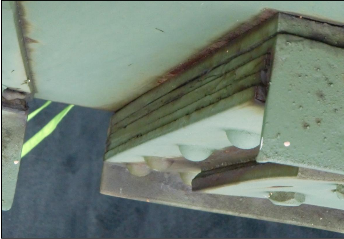
Photo 36 – Wear to Paint Indicating Hinge Movement, SE L 13 , Span 3.
