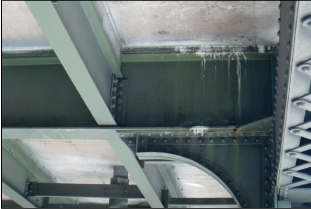
Photo 6 - Upper Deck Water Infiltration & Efflorescence, Floor Beam 13, Span 5
