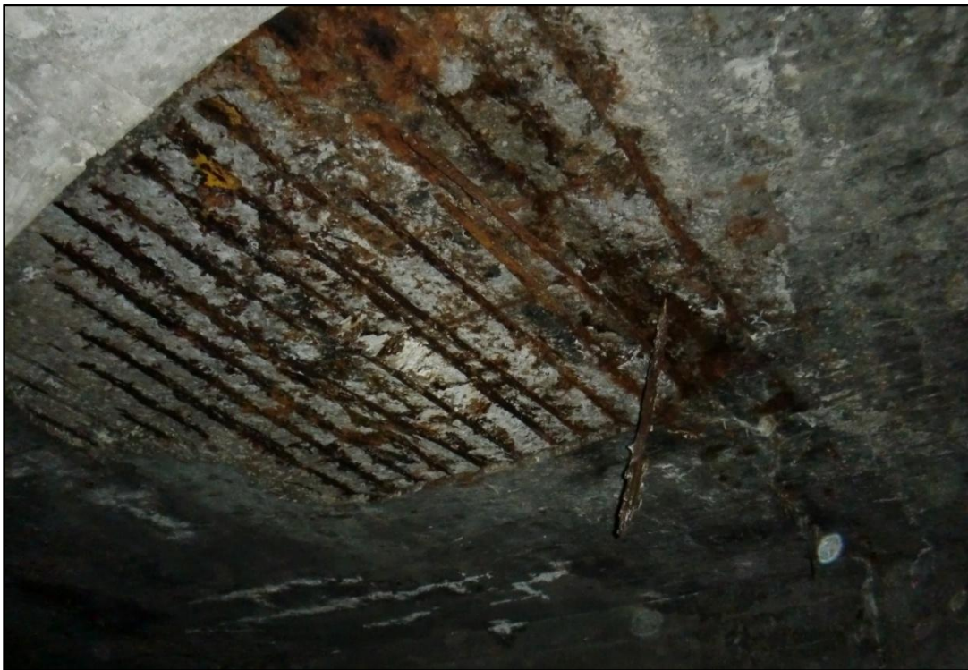
Photo 7 - Spall with Broken Reinforcement, East Subway.
