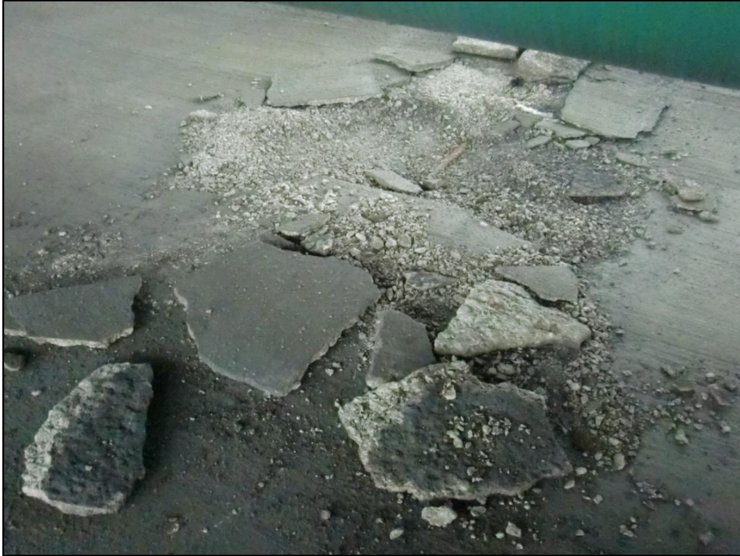
Photo 10 – Typical Local Deteriorated Concrete, Maintenance Deck.
