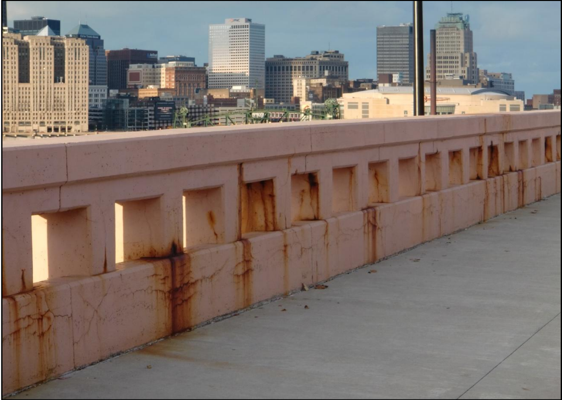
Photo 15 – Cracked North Railing with Active Corrosion, Span 11.
