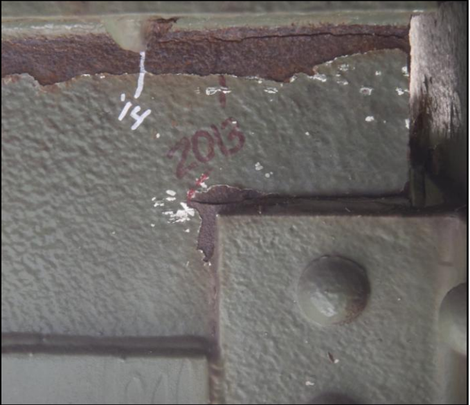
Photo 22B – Crack Propagation. North Interior End of East Beam, Maintenance Deck Floor Beam 15, Span 7.
