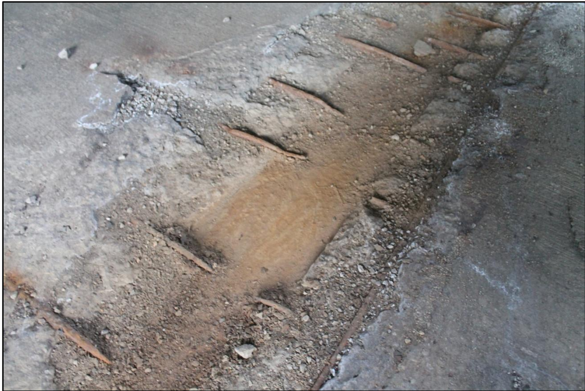
Photo 14 – Complete Fracture & Removal of Maintenance Deck above Floor Beam 3, Span 11 (Note: Exposed top flange visible).
