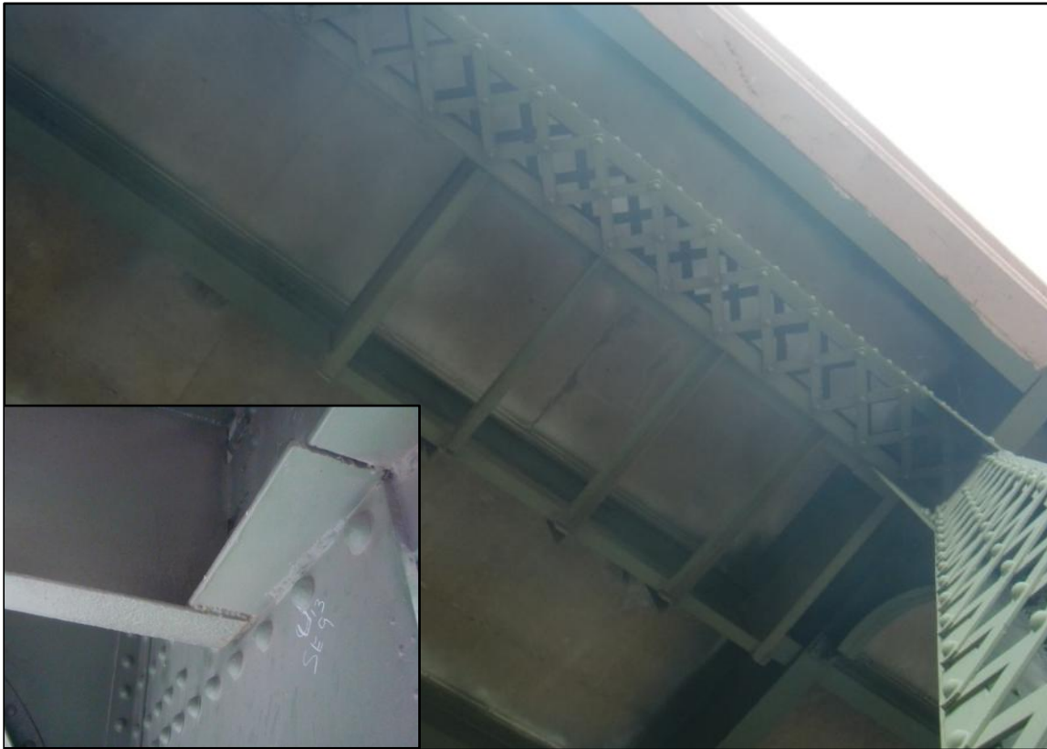
Photo 38 – Occasional Welded Frame to Upper Chord & Gusset Plate.
