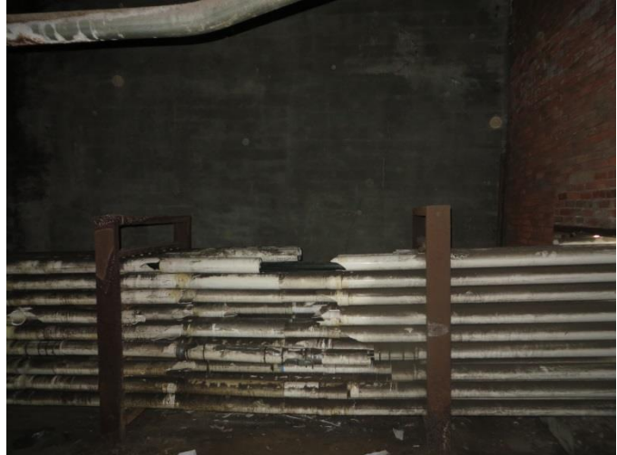
Damaged conduit in east tunnel
