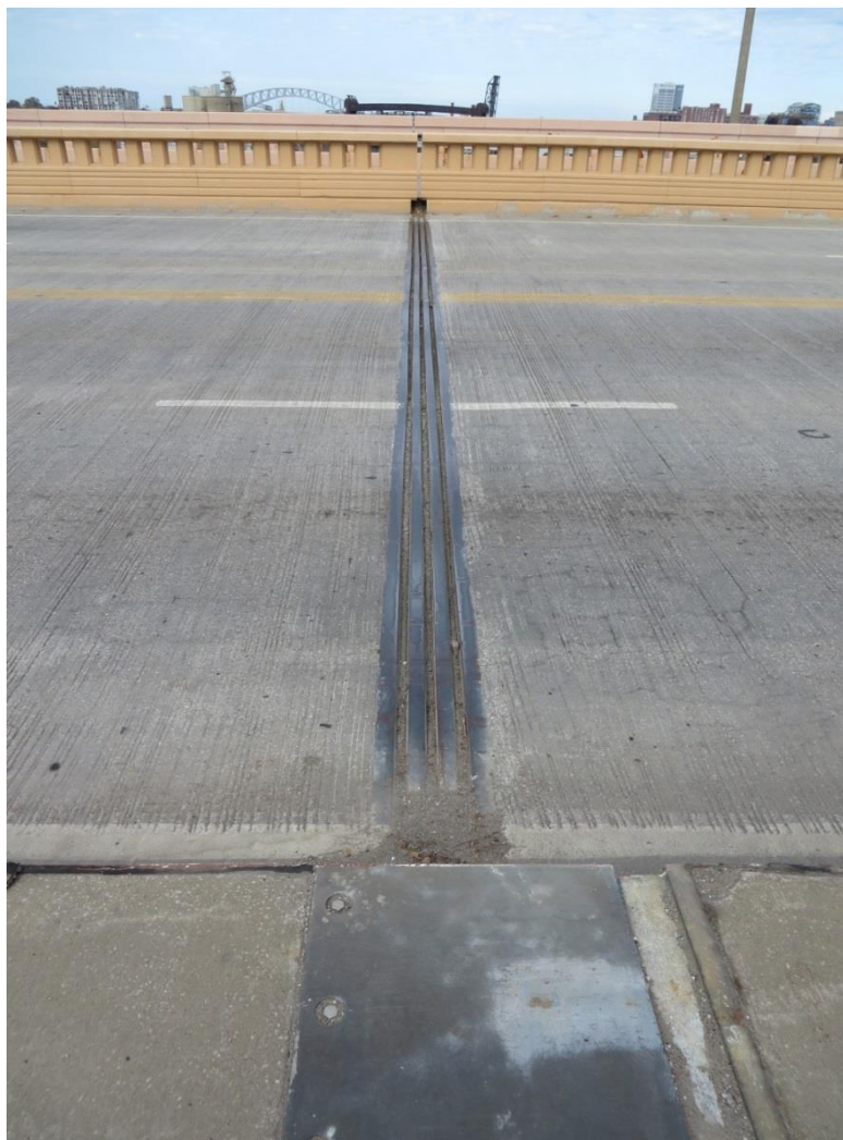
Debris and leakage common in deck joints
