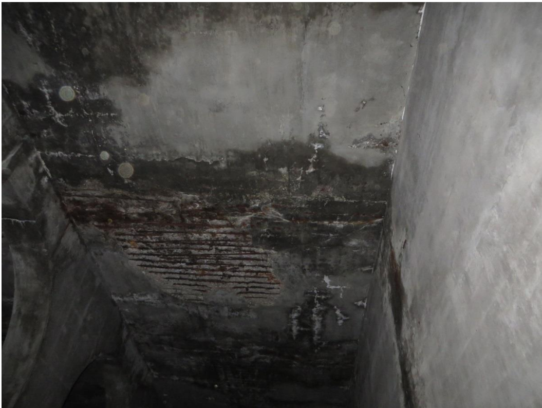
Large saturated and spalled areas with exposed and broken bars in east tunnel
