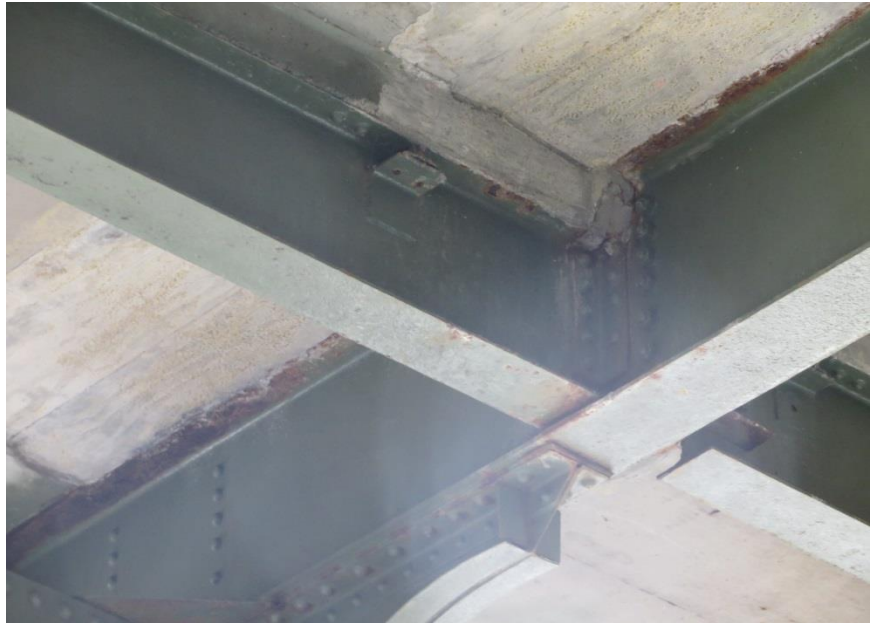
Section loss in stringer floorbeam connection adjacent to expansion joint
