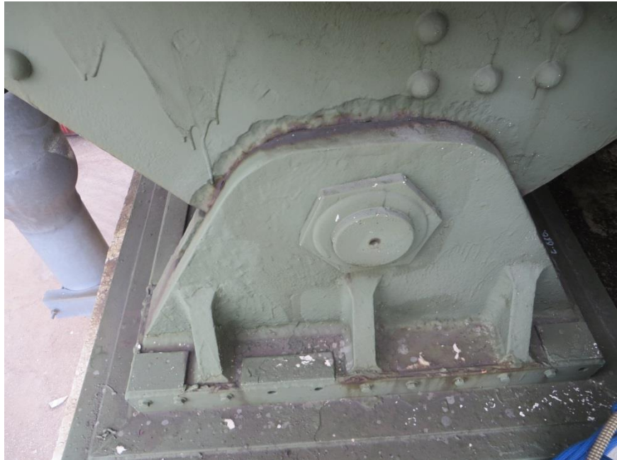
Section loss at A-S05-LC-11 Bearing
