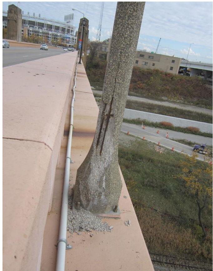
Spalled light post on south railing
