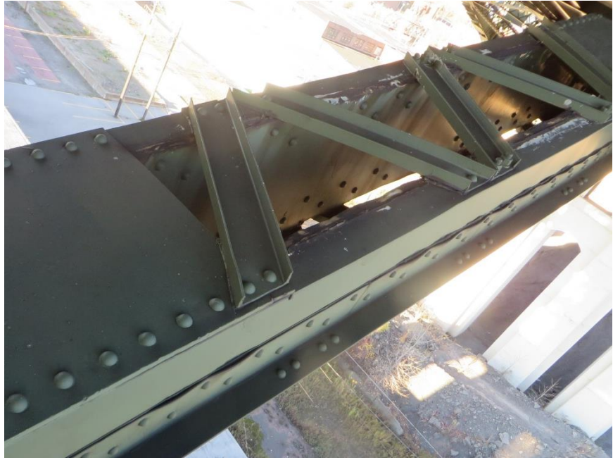
Pack rust in the angles and web plates of C-S07-LC-14
