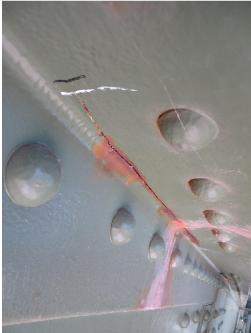
Crack in lower chord D in Span 12 between PP 03 and 04
