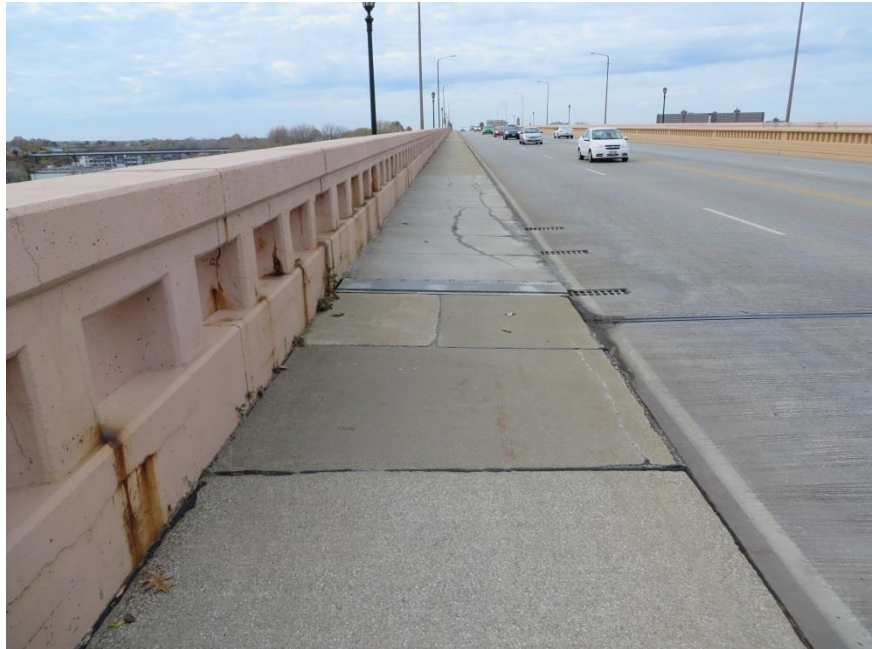
Cracks in previously repaired walk sections
