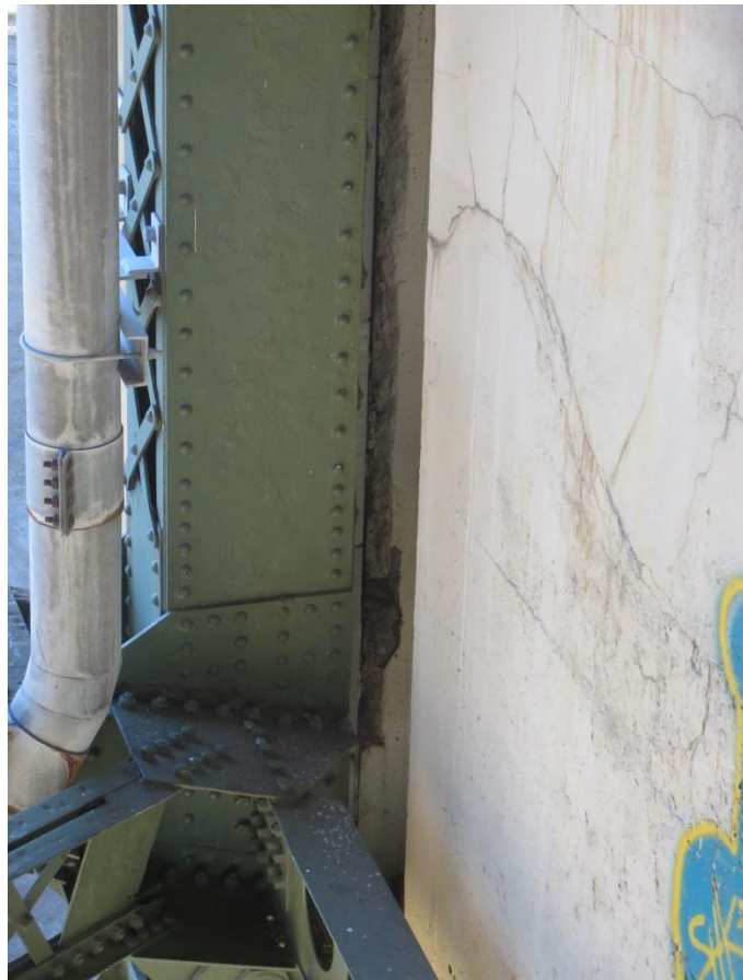
Crack in east pylon backwall
