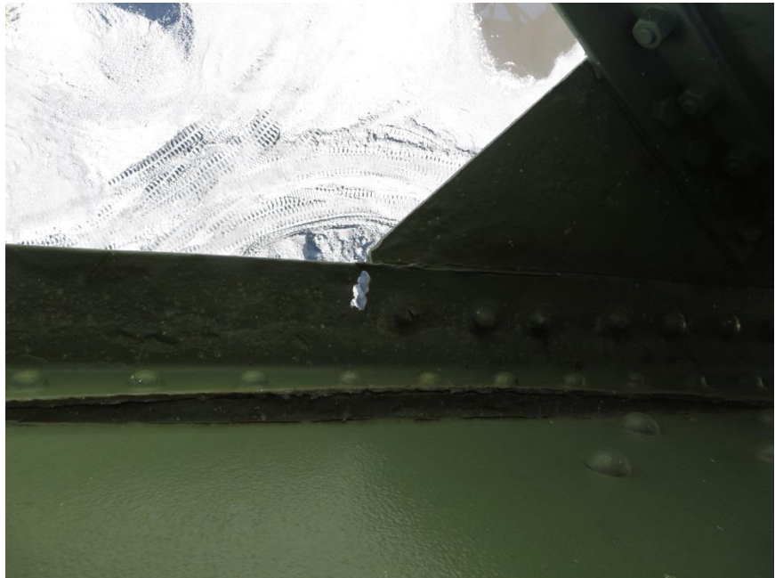
Through hole in lower angle of D-S09-LC-11
