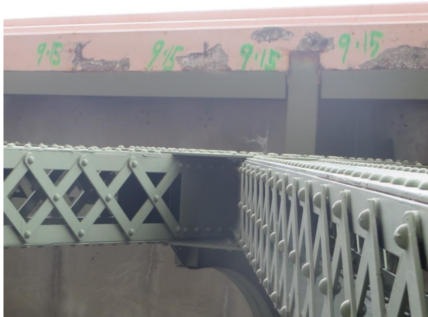
Previously removed spalls on north deck edge
