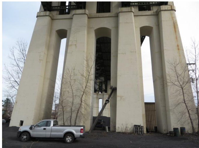
Pier 8 west face showing patches, cracks, and hole in left tower
