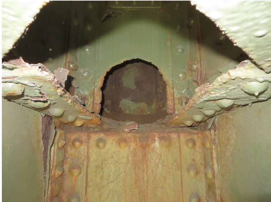
Corrosion inside D-S03-UC-13
