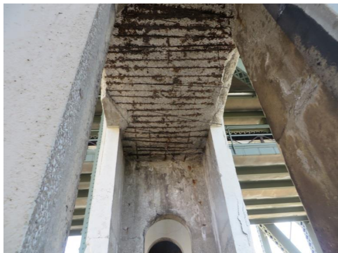
Degrading pier tower roof
