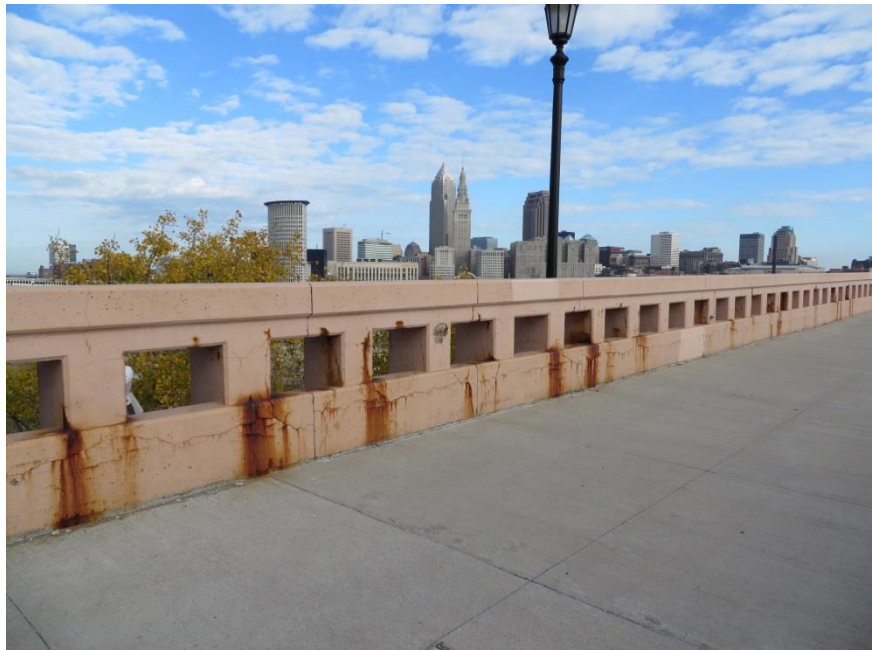
Typical railing cracking and staining pattern
