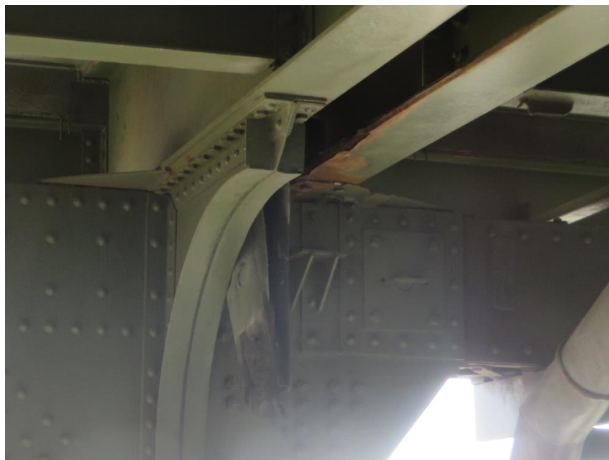
Corrosion in lower flange of D-S03-UC-13 floorbeam
