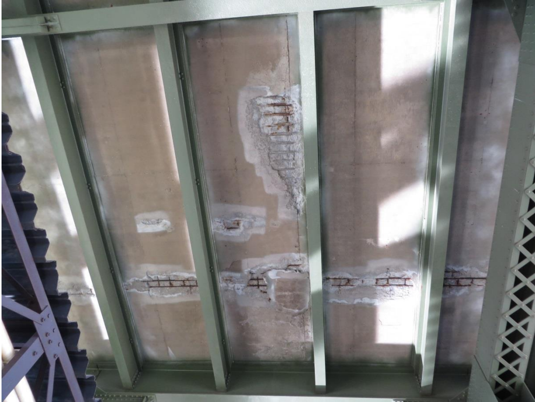
Spalled areas with rust inhibitor and fresh spalls without, common throughout entire deck underside
