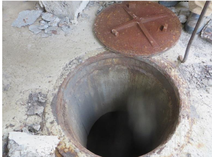
Deteriorated manhole casting in Pier 9
