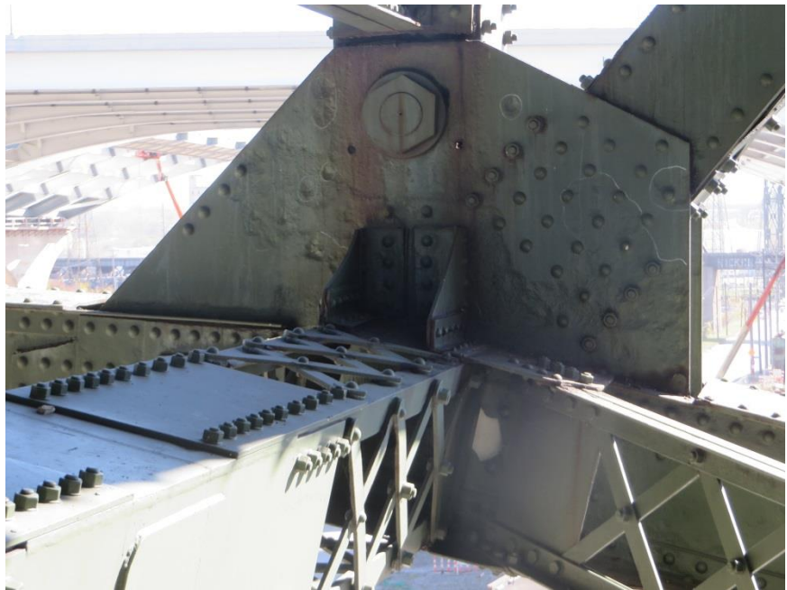
Section loss in D-S05-LC-14
