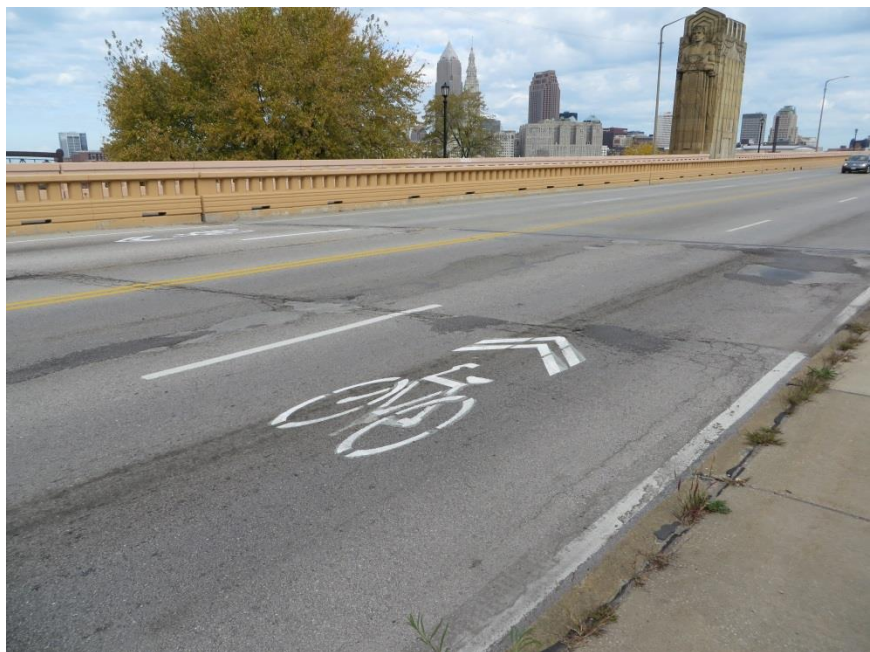
Cracks and patches in west approach wearing surface
