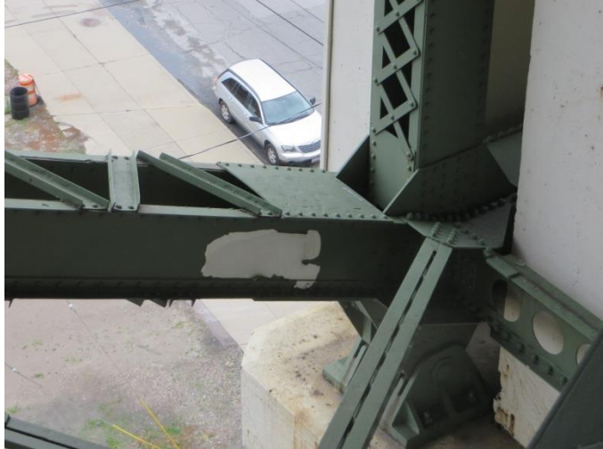
Large PCS failure in lower chord A
