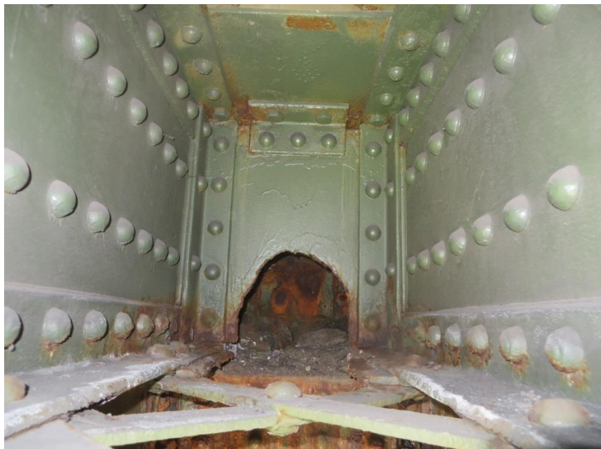
Corrosion inside D-S07-UC-15
