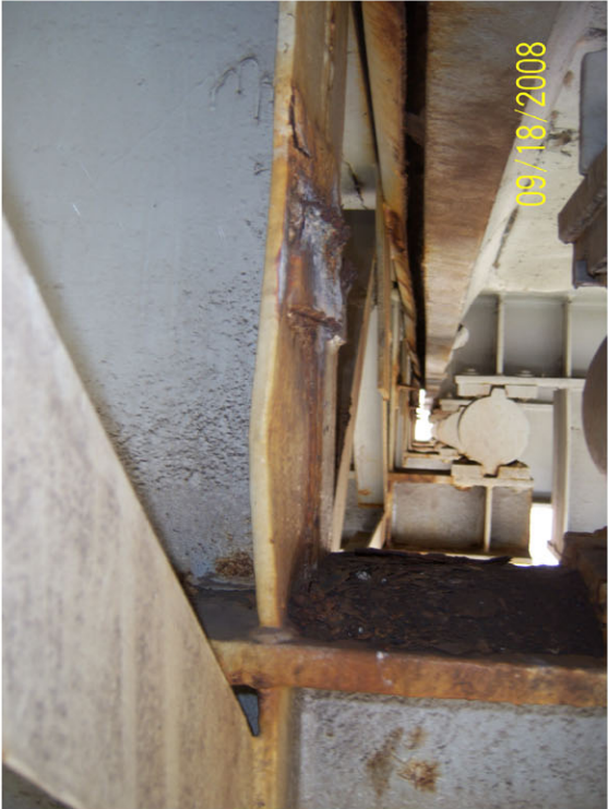
Under Joint 1A bent stiffener of Beam 3.JPG
