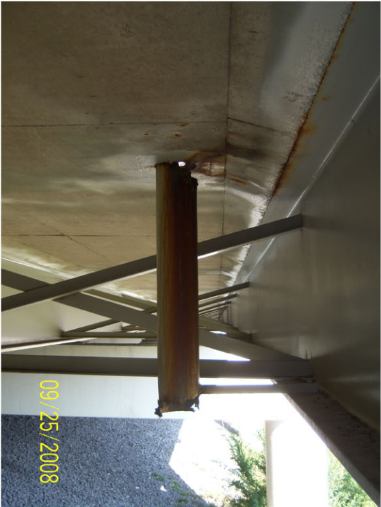
Holes top and bottom at downspout 1R near star...
