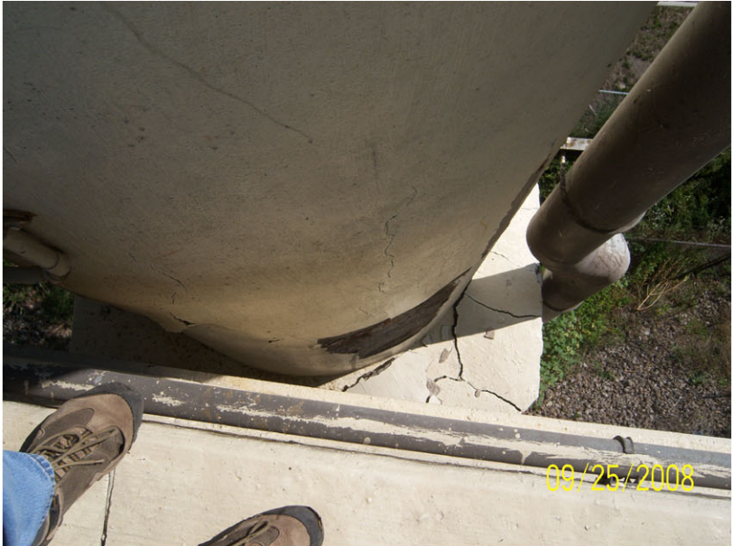
Spalls and delams of right column of Pier14 .JPG
