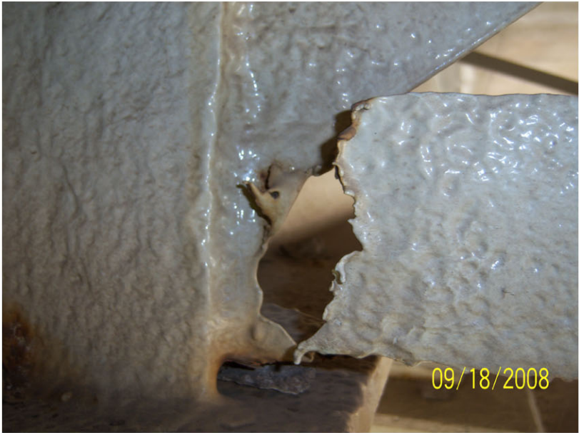
Under Joint 2A rust severed xframe angle in Bay...
