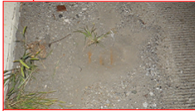
Typical clogged drain.
