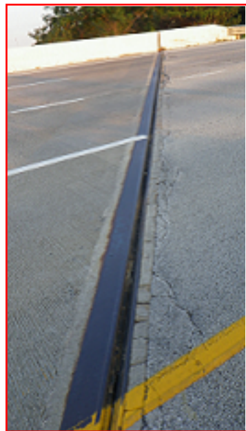
Typical map cracking along expansion joint.
