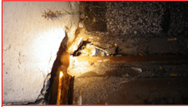
Large erosion hole at approach slab near North Abutment AW.
