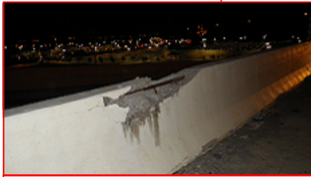
Spall with exposed reinforcing steel at barrier.
