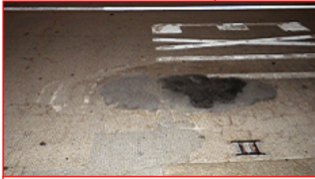
Typical failing asphalt patch.
