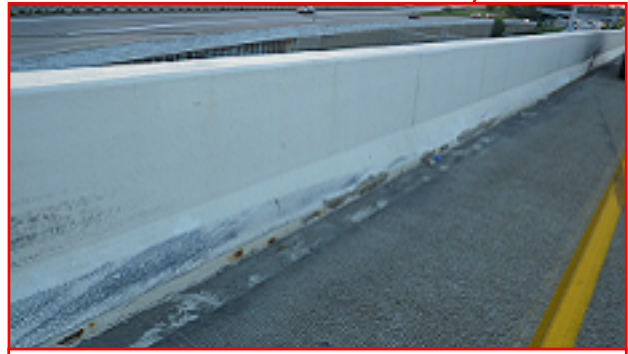
Typical spall at toe of barrier.
