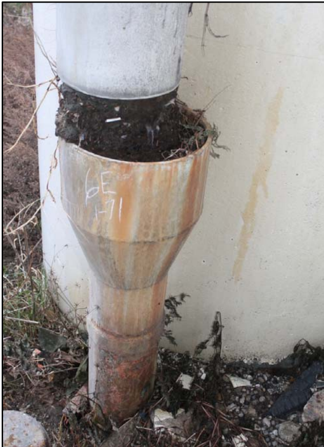
Photo 15 – Clogged Collector and Drain Pipe, Pier 6E.
