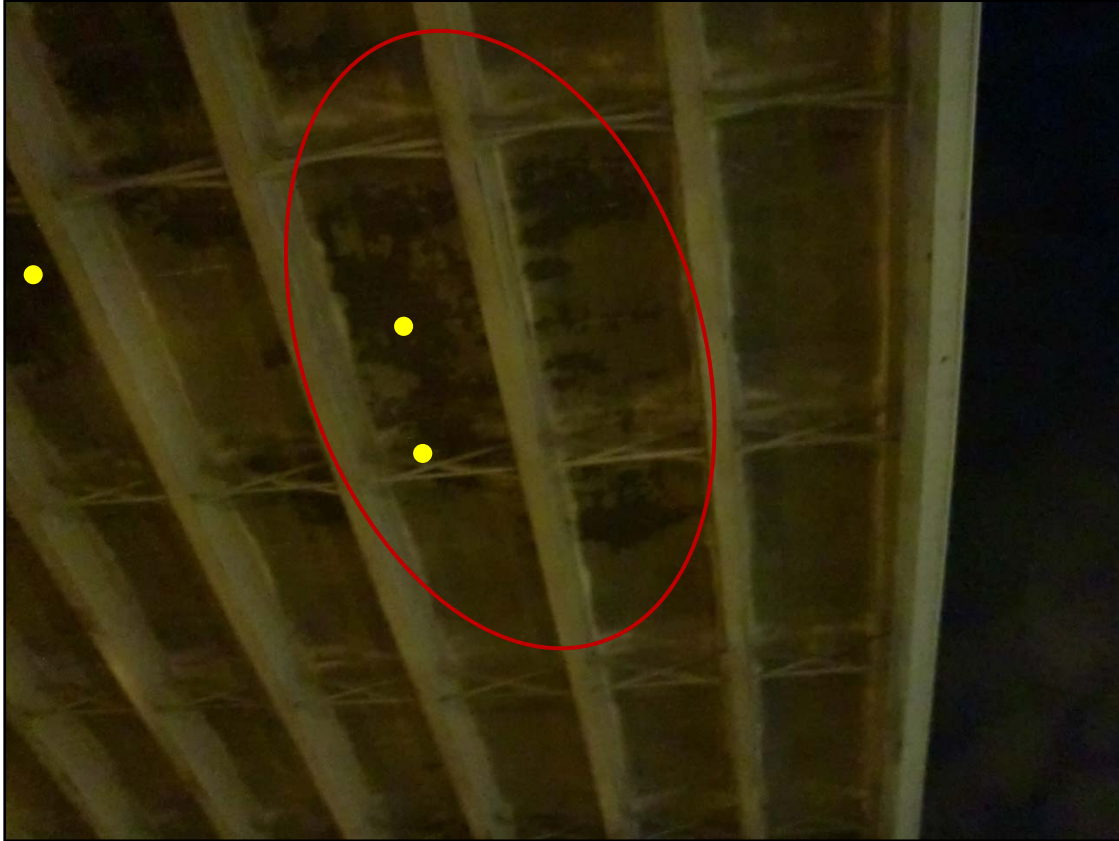
Photo 6 – Water Infiltration Through Floor Following Rain. (Note: Area circled is location of mottled concrete in Photo 5, Locations marked with yellow dot are spalled surfaces.)
