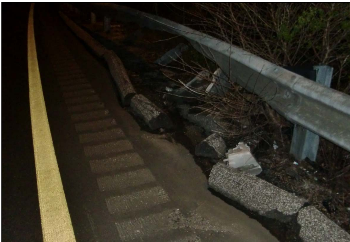
Photo 39 – Broken Asphalt Curb, South Approach.
