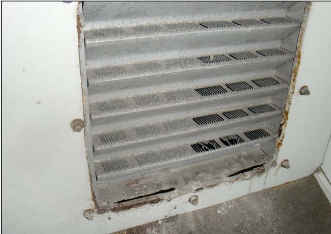
Photo 36 – Galvanic Corrosion & Perforations on Aluminum Vent, East End of Steel Pier Cap 17.
