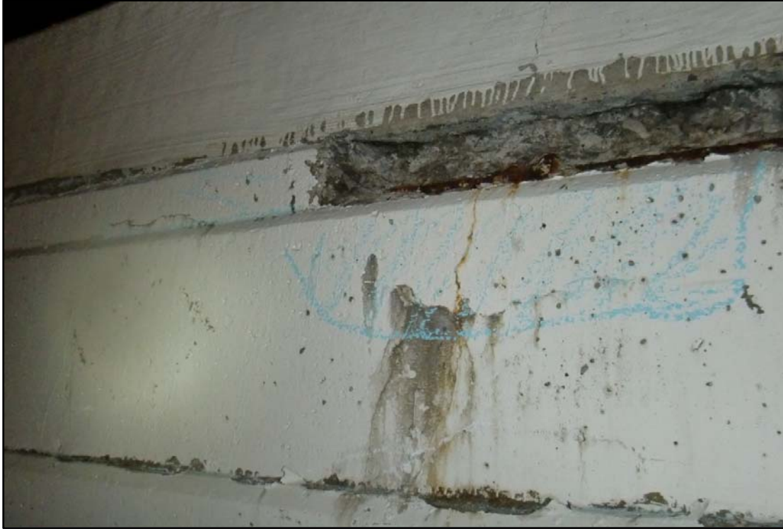
Photo 13 – Loose Concrete Removed With New Delamination Below (Highlighted in Chalk), Span 2 over SR 176 SB.
