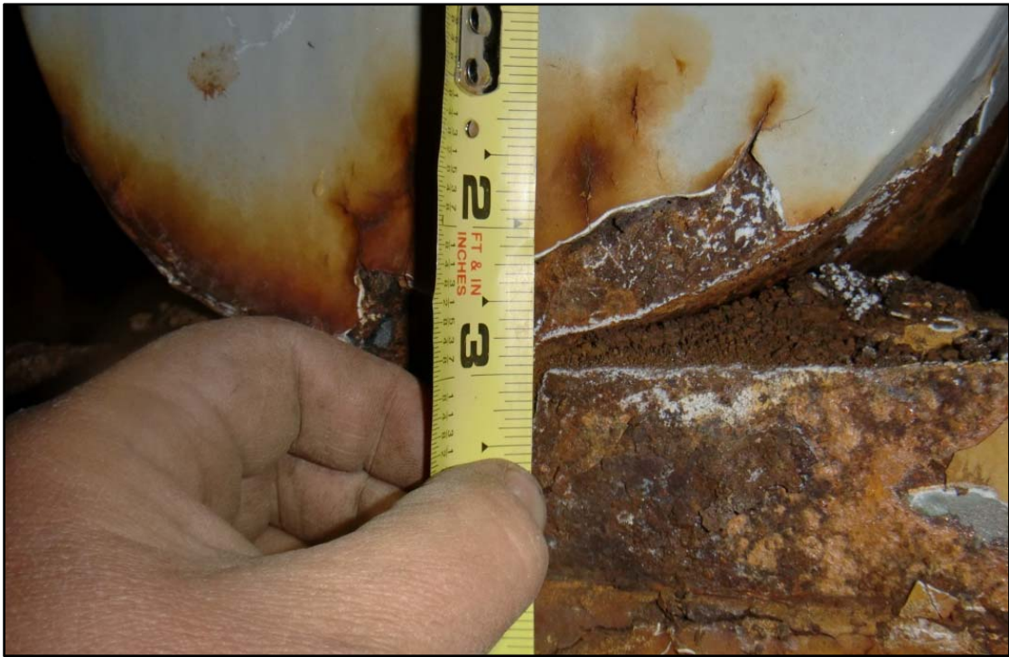
Photo 26 – 1/4" Debris Build-Up Beneath Hinge Roller.
