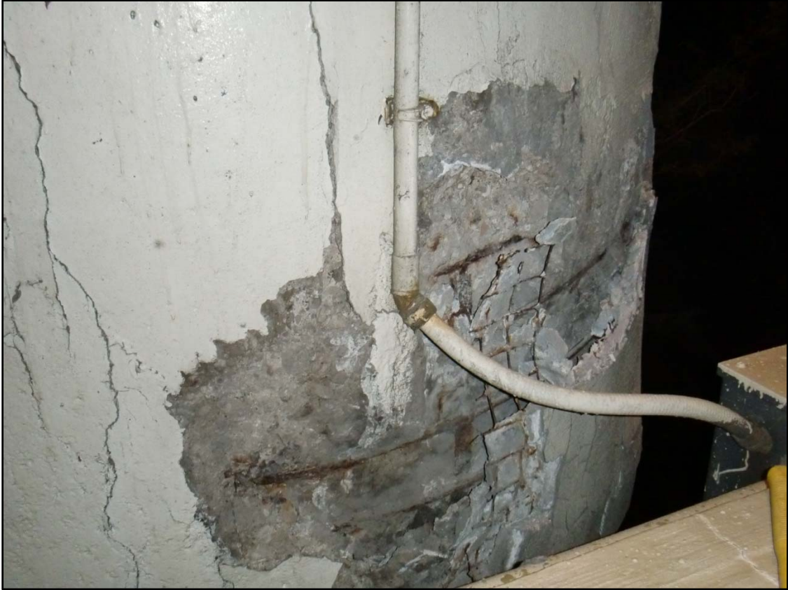
Photo 32 – Failed Patch With Surrounding Delamination, Pier 14 East Column.
