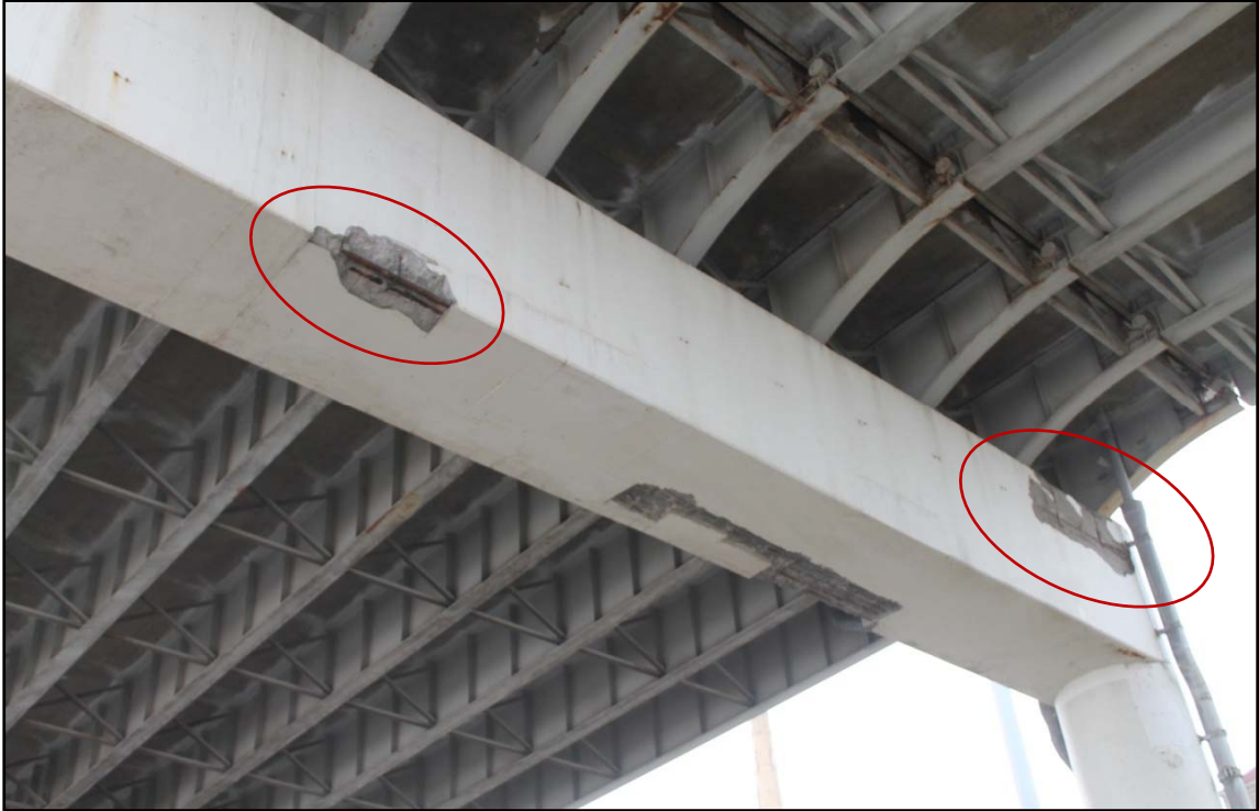
Photo 30 – Active Spalled Concrete (Circled) With Removed Deteriorations (Center), Pier 6.
