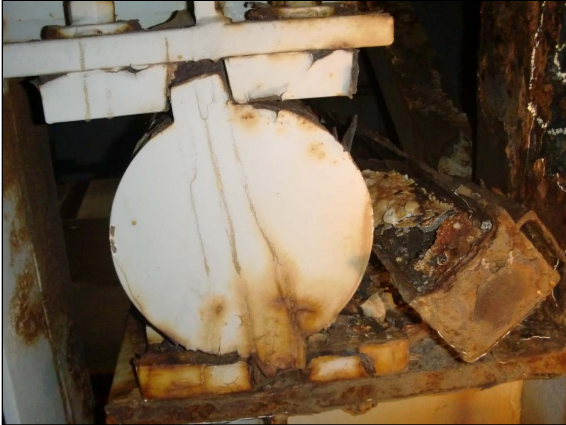
Photo 25 – Excessive Expanded Hinge Position at 55°F.
