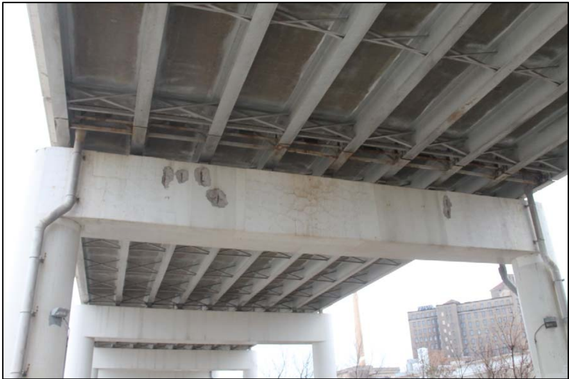
Photo 31 – Local Spalls With Rust-Stained Map Cracking, North Face of Pier 11 Cap.
