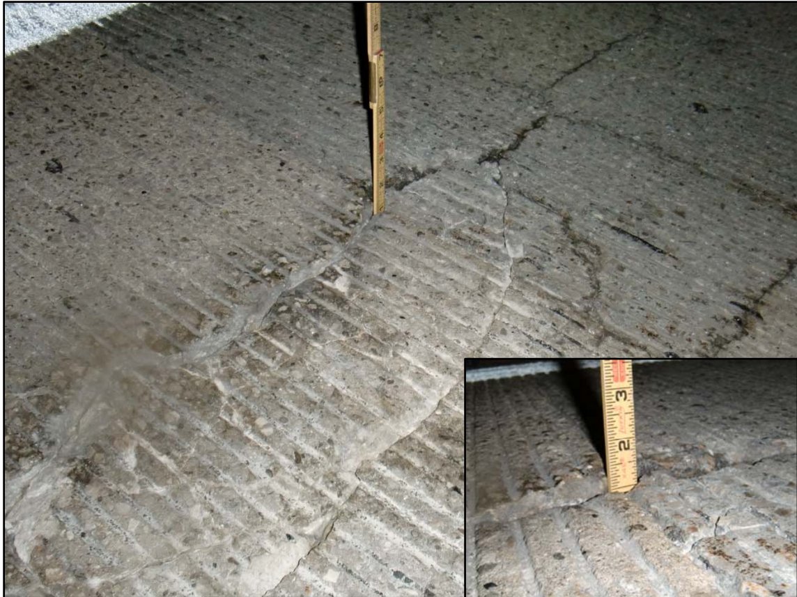
Photo 12 – Wide Crack in Wearing Surface, Over One-Inch Deep, Span 16.
