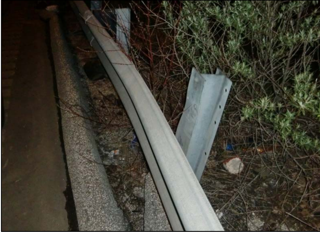
Photo 41 – Detached Approach Guard Rail, Left Side of South Approach.
