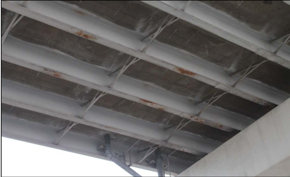
Photo 19 – Typical Isolated Failed OZEU Paint on Girder Bottom Flanges.
