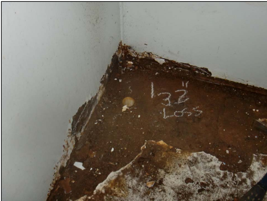
Photo 34 – Minor Section Loss at Drain Hole, Interior of Steel Pier Cap 17.
