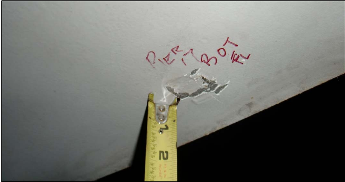
Photo 33 – Weldment on Bottom Flange, Steel Pier Cap 17.
