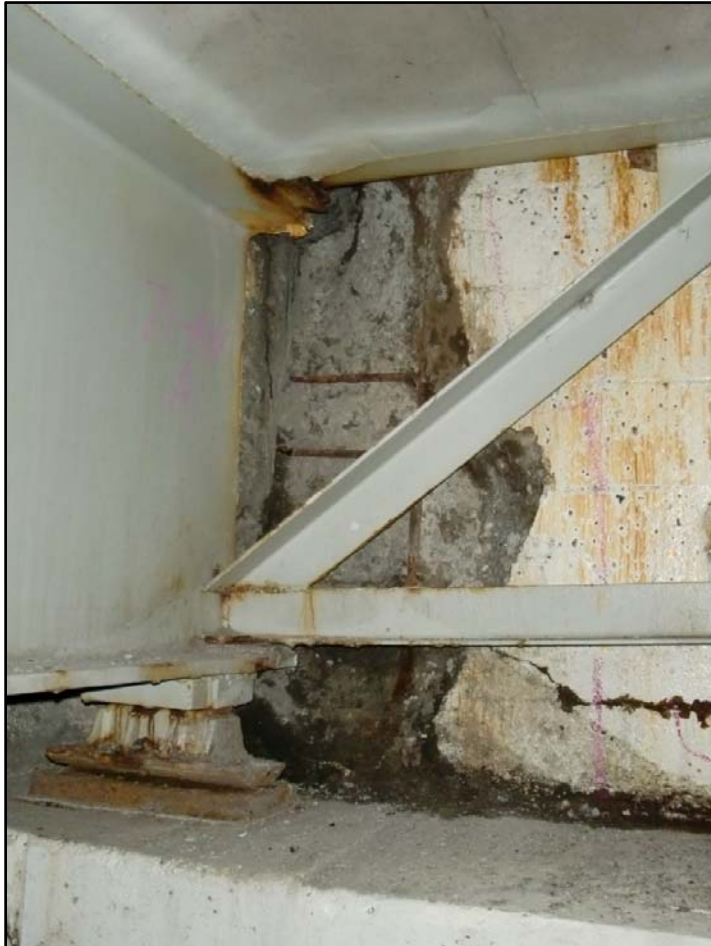
Photo 29 – Backwall Spall Below Failed Expansion Joint Membrane, North Abutment AW.
