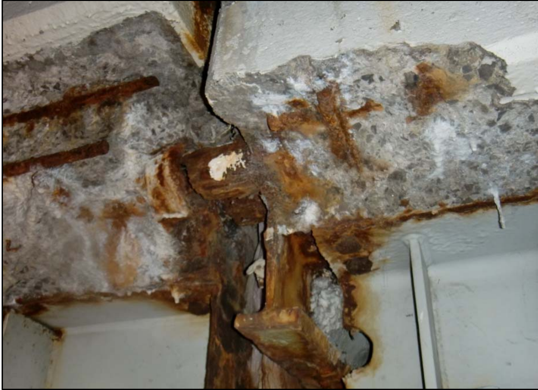
Photo 7 – Advanced Spalls on Edge of Floor at Expansion Joint 1A.
