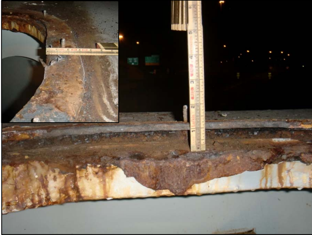
Photo 35 – Pack Rust & Section Loss (See Inset) Along Hatch Rim, Steel Pier Cap 17.
