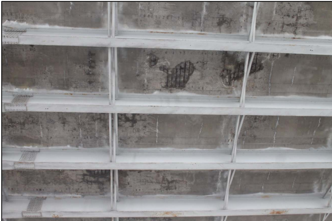
Photo 5 – Spalled Soffit over SR 176 NB Vehicular Lanes with Adjacent Mottled Concrete Surfaces, Span 8.
