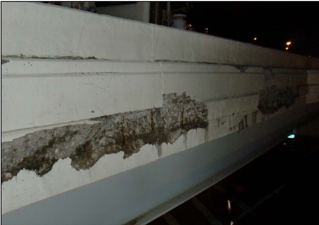
Photo 14 – Loose Lower Exterior Parapet Concrete Removed over SR 176 Traffic Lanes.
