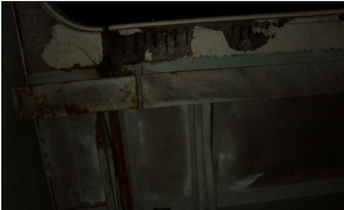
Photo 8 – Spalled Edge of Floor, Spans 17 & 18AW at Expansion Joint 3A.
