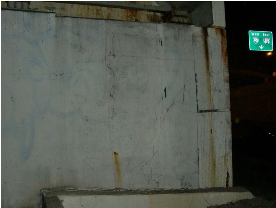
Photo 28 – Delaminated Abutment Barrel Face Between Beams E & F, North Abutment AW.
