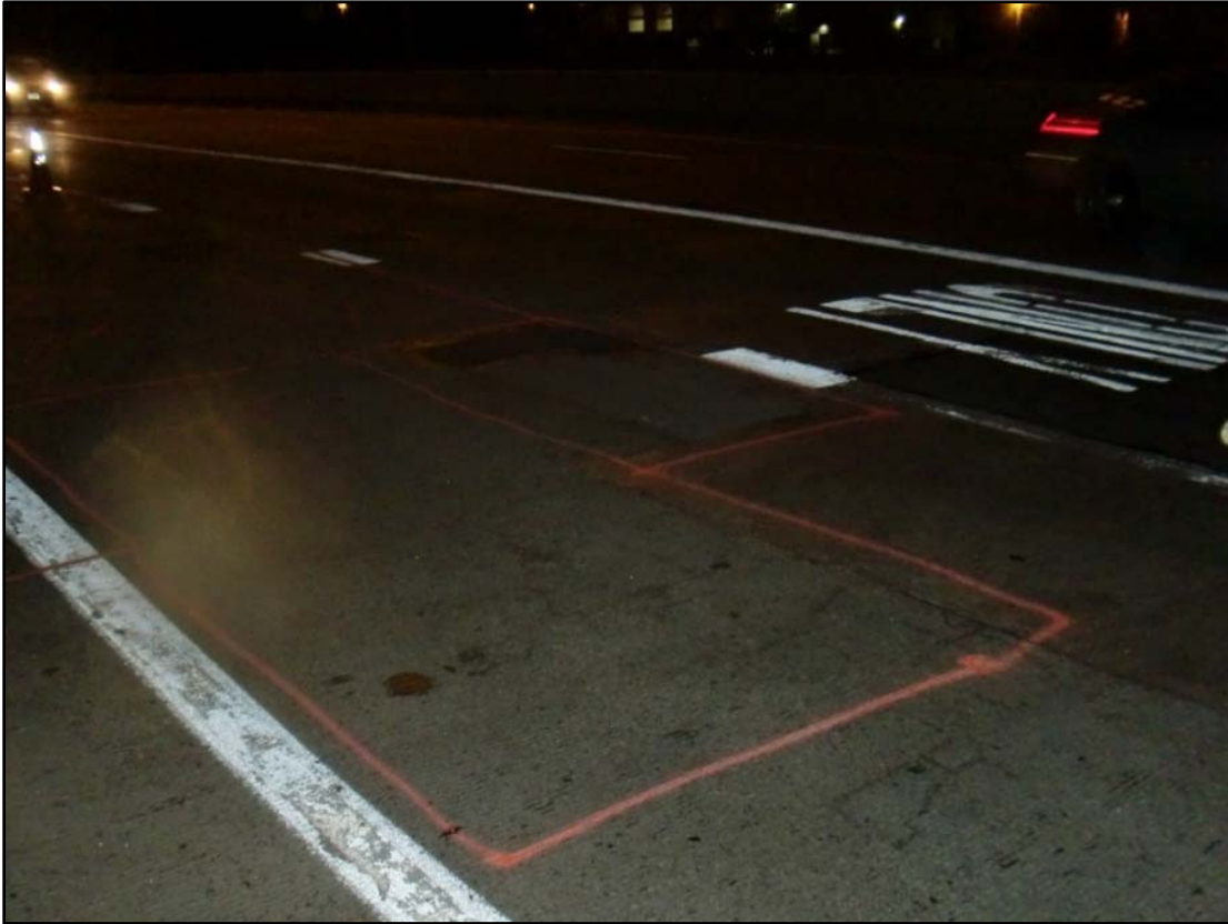
Photo 9 – Large Wearing Surface Delamination, Span 9 Right Lanes.
