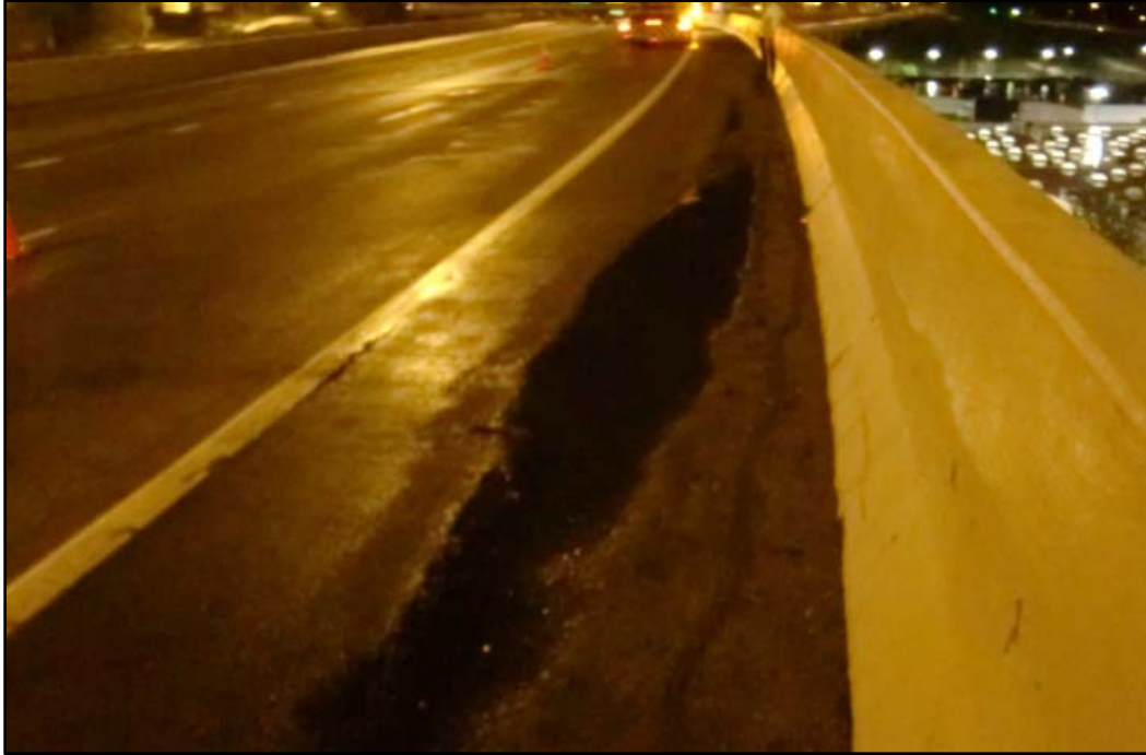
Photo 16 – Right Shoulder Water Ponding, Span 3.
