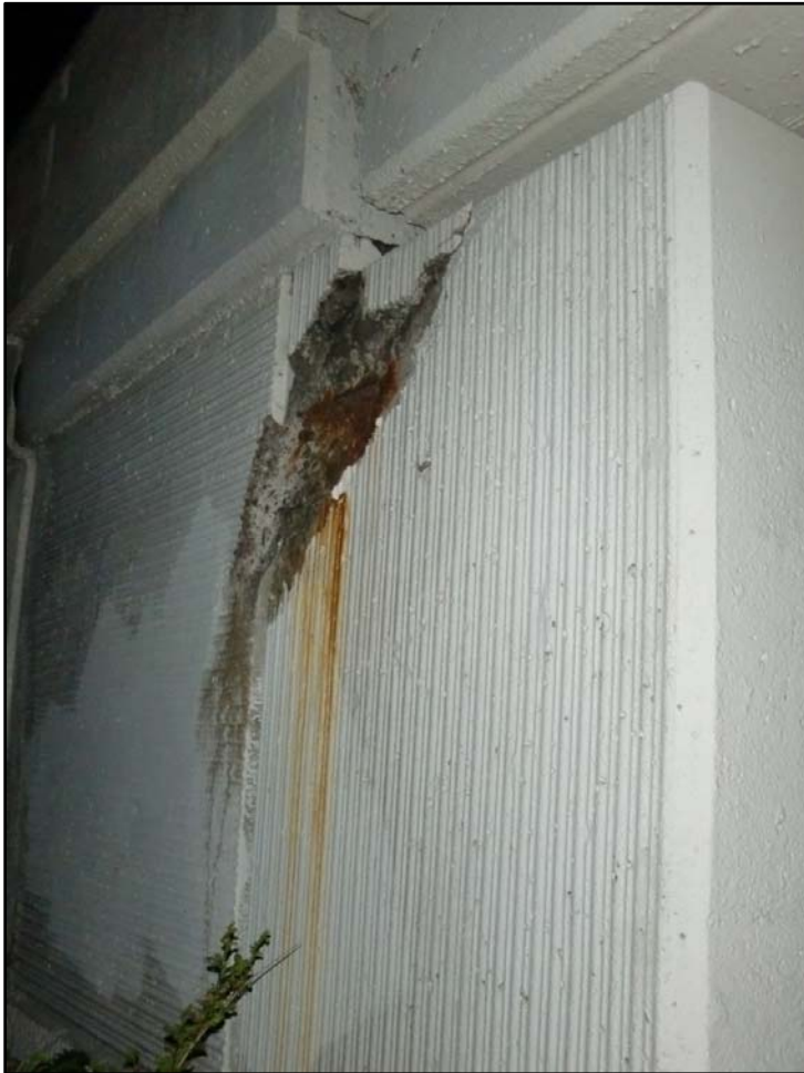
Photo 38 – Increasing Spalls on West Wingwall & Mask Wall, North Abutment AW.
