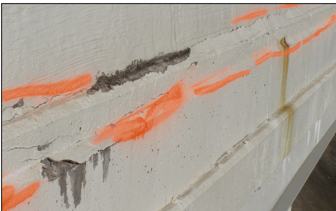
Photo 7 – Cracked Exterior Parapet Face (Note: Upper spall is actually fallen trowelable mortar)
