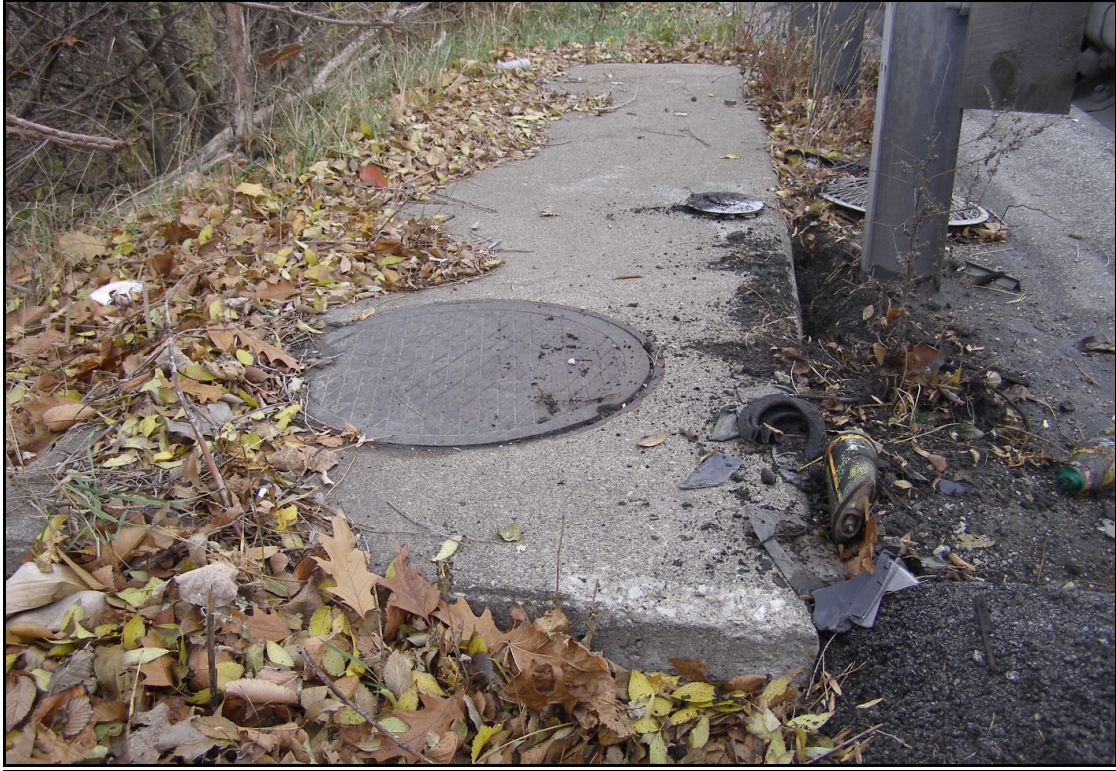
Photo 46 – Clogged Catch Basin Along South Approach, I-71 Bridge
