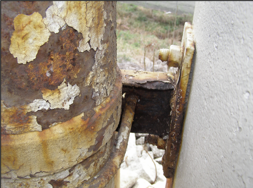
Photo 23 – Heavily Corroded Drainage Bracket, Pier 24BE
