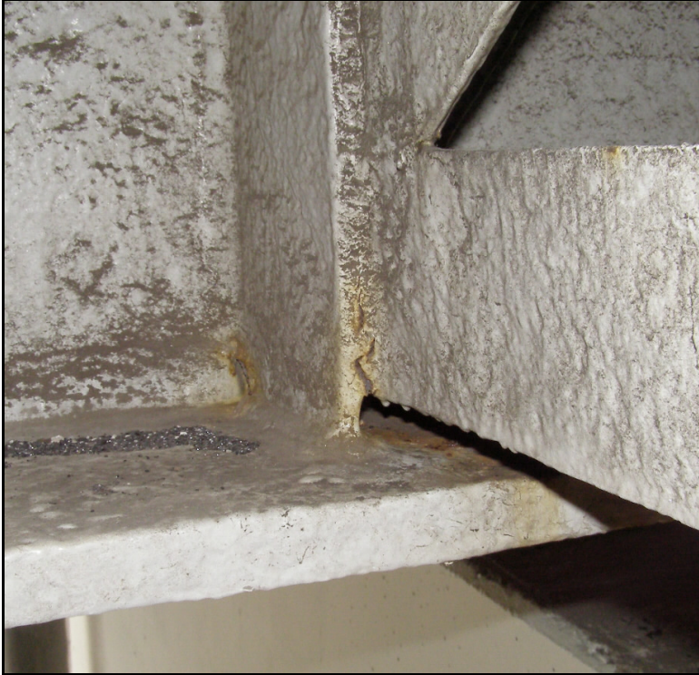
Photo 26 – Cracked Diaphragm Weld Due to Pack Rust
