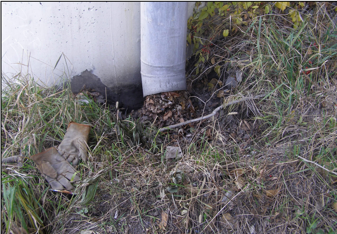
Photo 21 – Typical Debris Back Up into Drain Pipe
