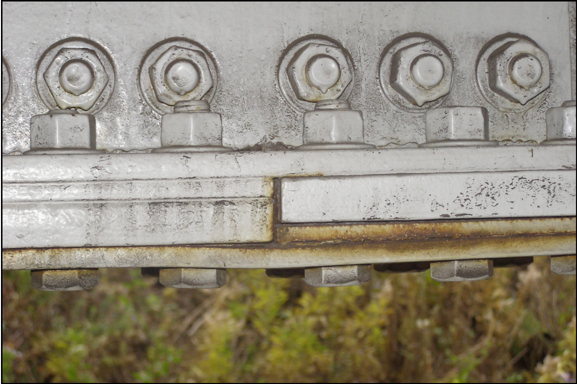
Photo 30 – Typical Pack Rust at Bottom Flange Splice Plates
