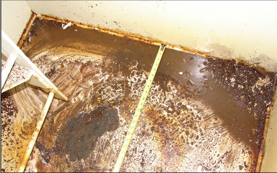
Photo 36 – Small Amount of Standing Water and Light Corrosion to Box Floor, Panel 21
