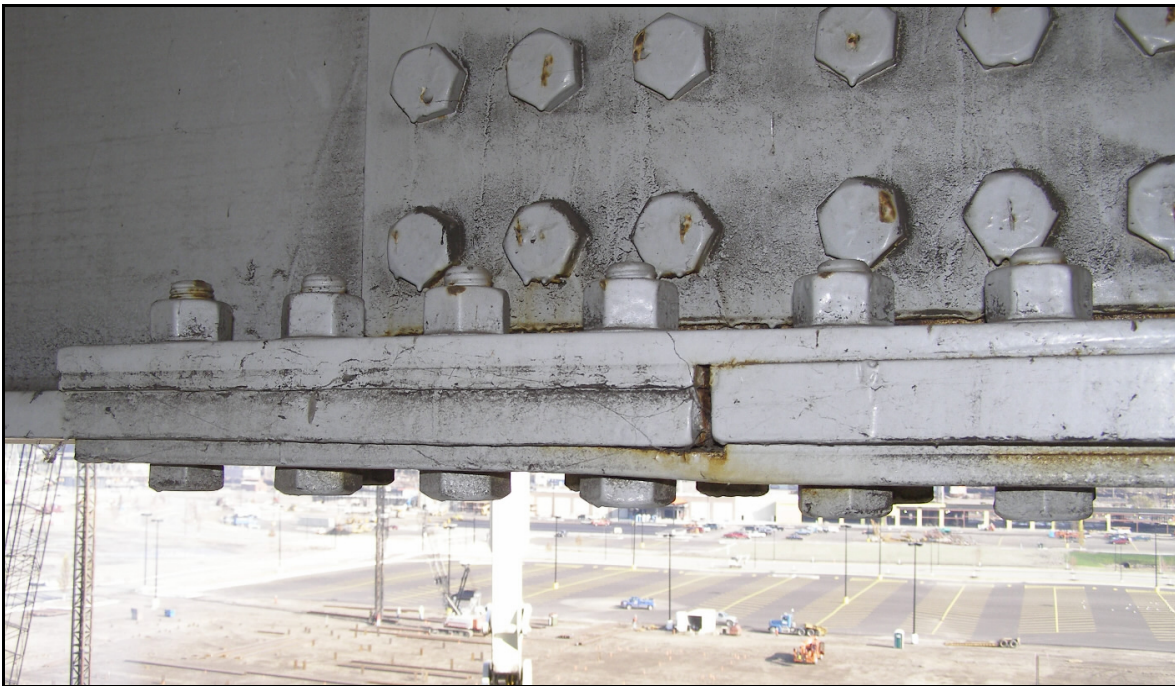
Photo 25 – Draw Down and Corrosion to Bottom Flange Splice Plates, Span 8A Field Splice
