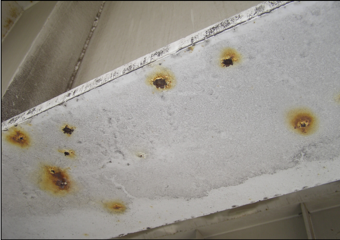
Photo 29 – Typical Corrosion Blooms to Bottom Flange
