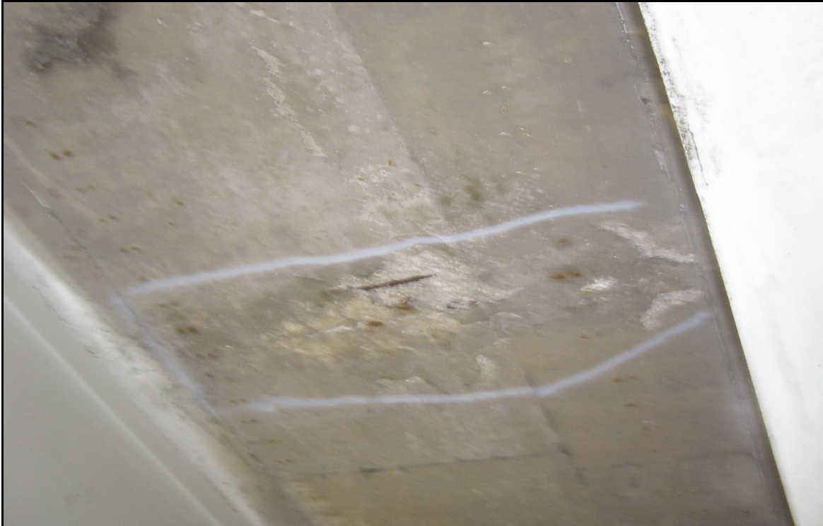
Photo 18 – Underdeck Spall & Delamination, Span 26E
