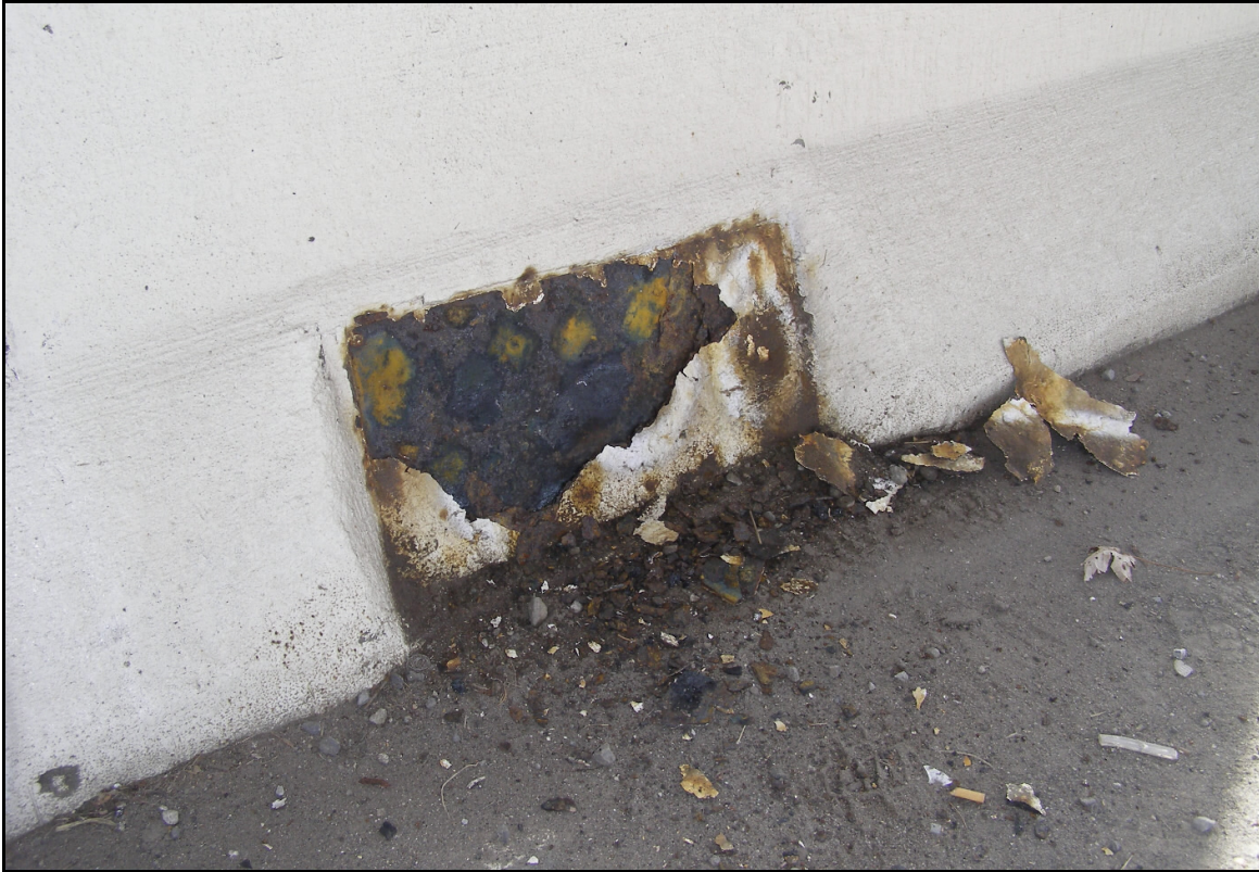
Photo 50 – Typical Heavy Corrosion Pull Box Cover, Jennings Freeway Bridge
