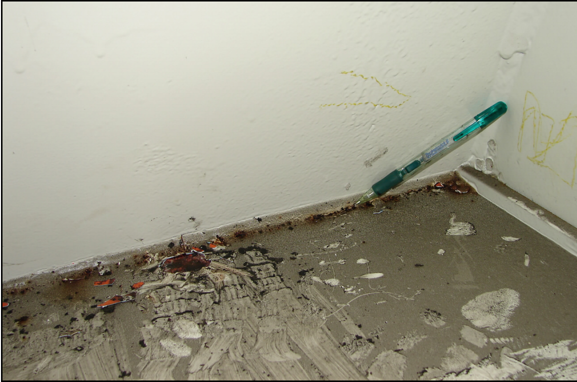
Photo 39 – Slight Corrosion and Dirt to Interior Floor, Panel 3
