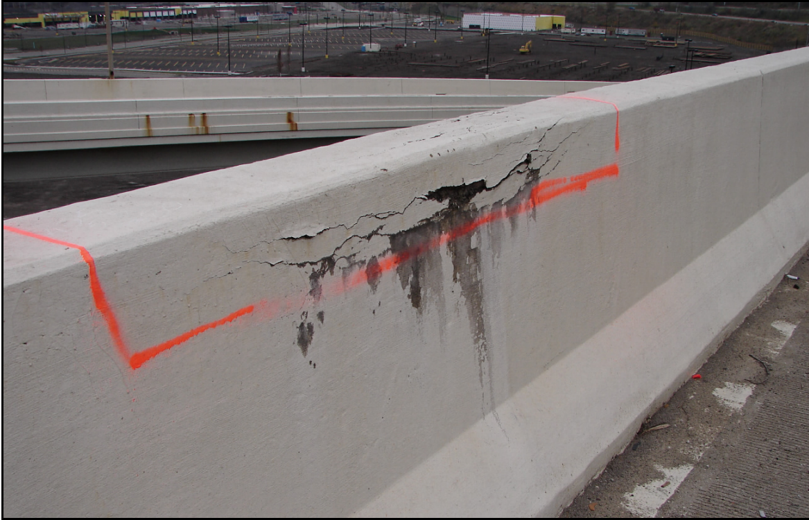
Photo 10 – Deteriorating Safety Parapet Shape, Unit 4AE
