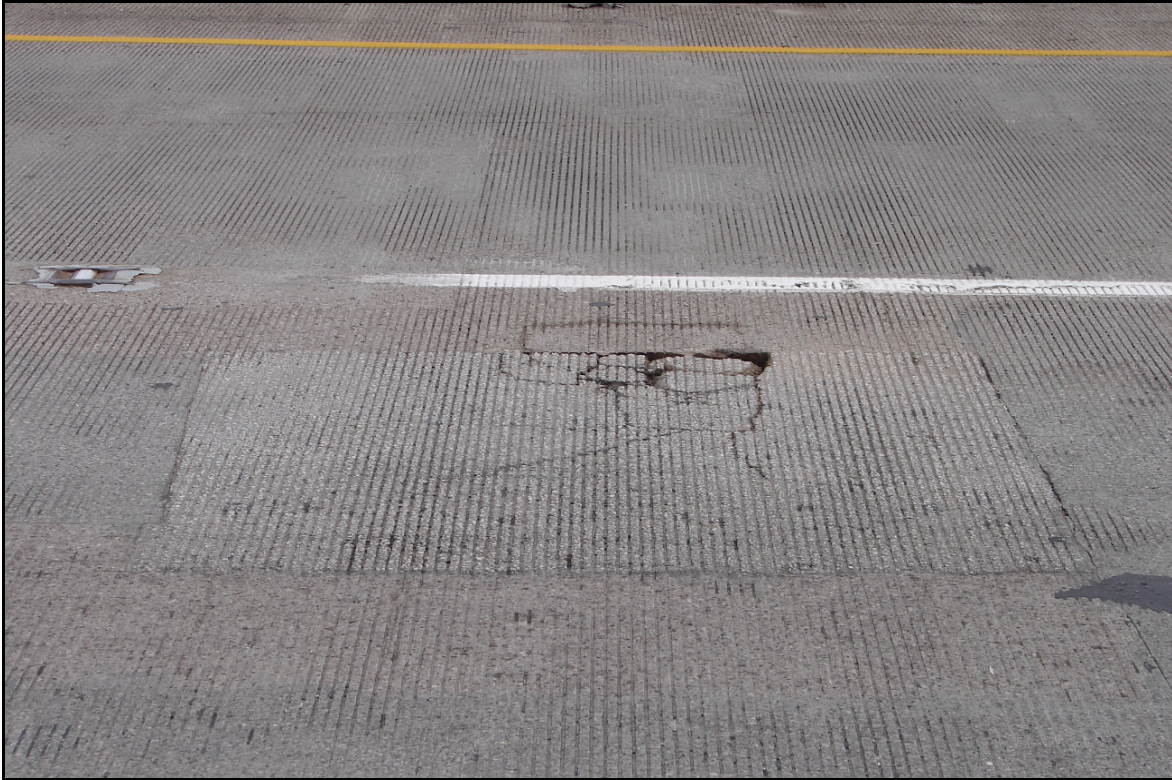
Photo 6 – Cracked Wearing Surface Within 1991 Patch
