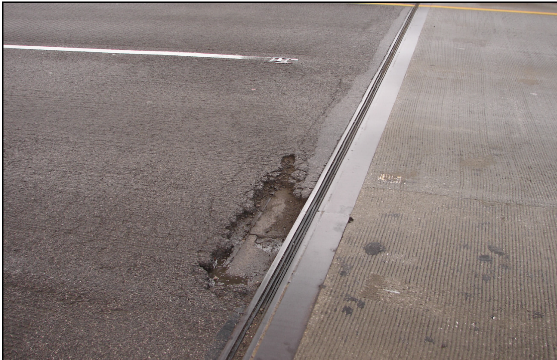
Photo 47 – Approach Slab Spall, Rear Approach, Jennings Freeway Bridge
