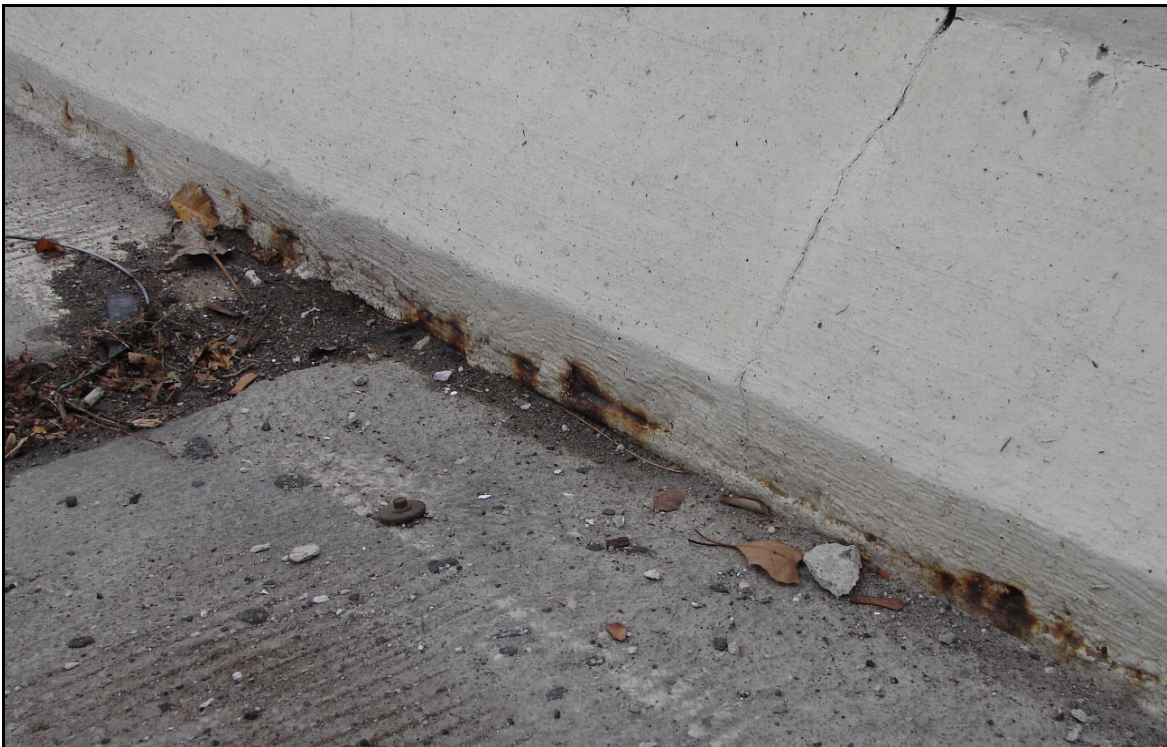
Photo 11 – Concrete Corrosion at Parapet Toe, Unit 4AE
