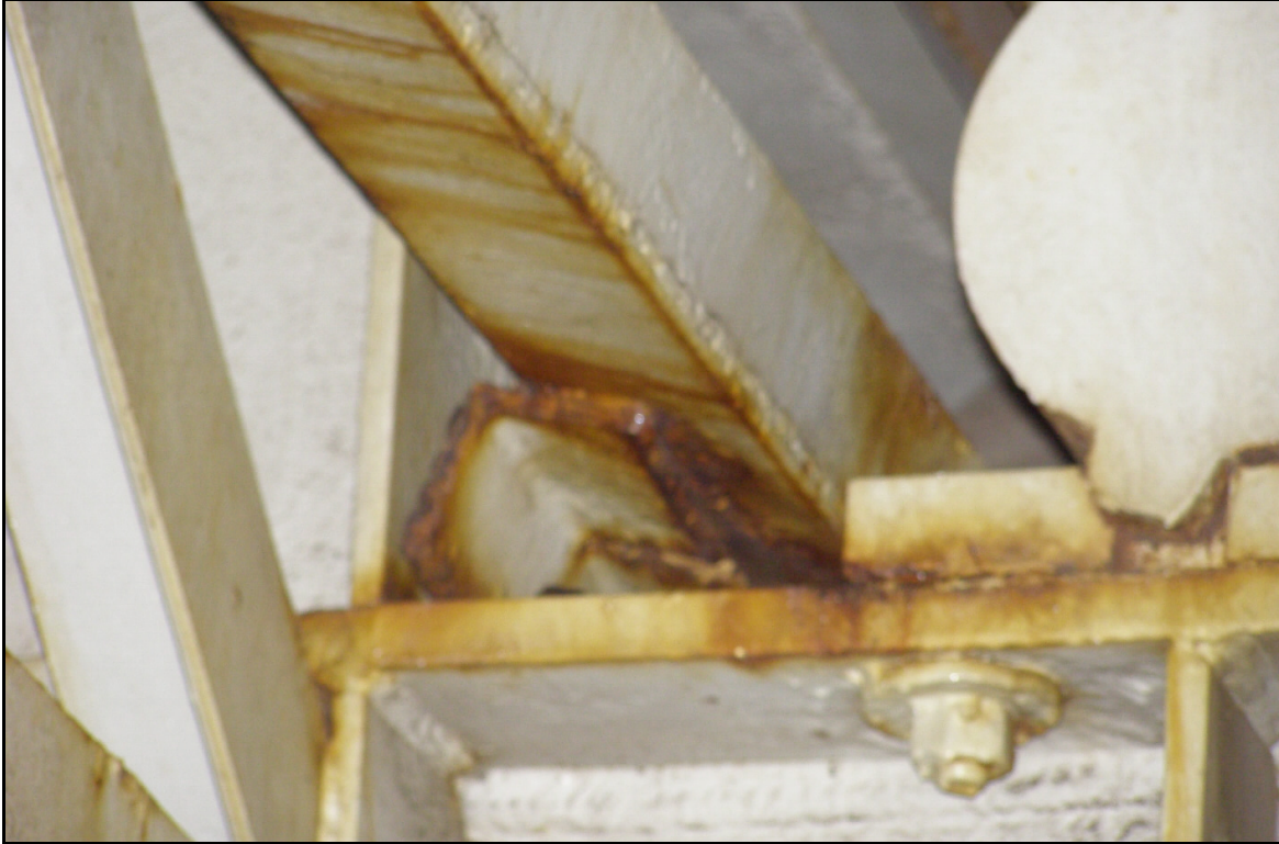
Photo 13 – Broken Drain Trough Bracket and Loose Trough, Expansion Joint 2A
