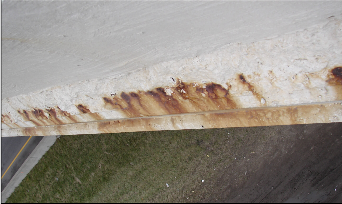
Photo 15 – Active Concrete Corrosion at Parapet Base, Outside Gutterline Ponding
