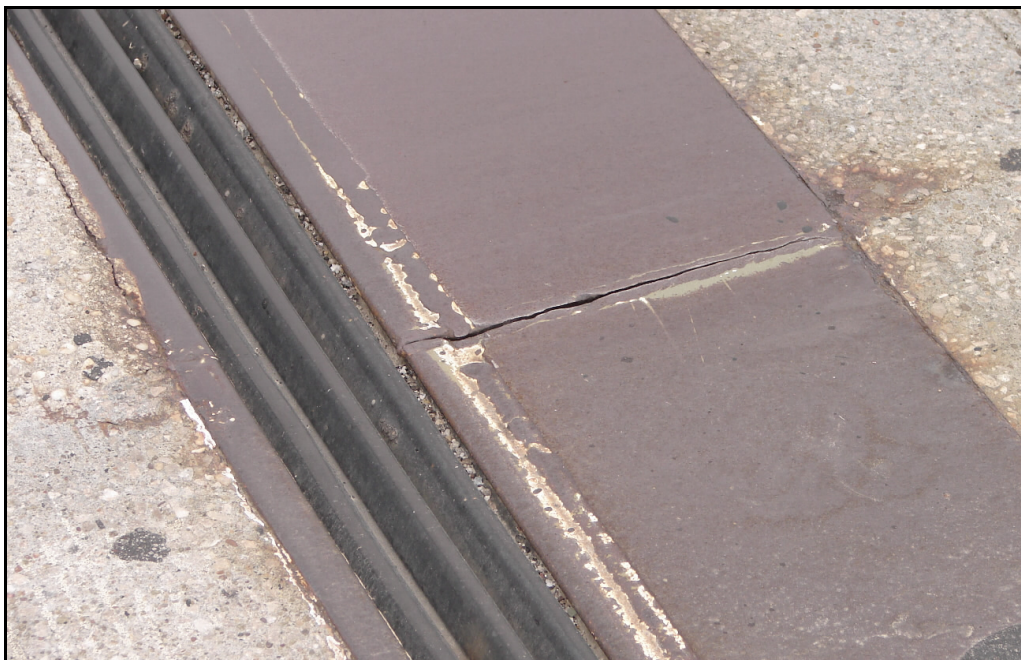
Photo 17 – Missing Seal Weld, Expansion Joint 1A
