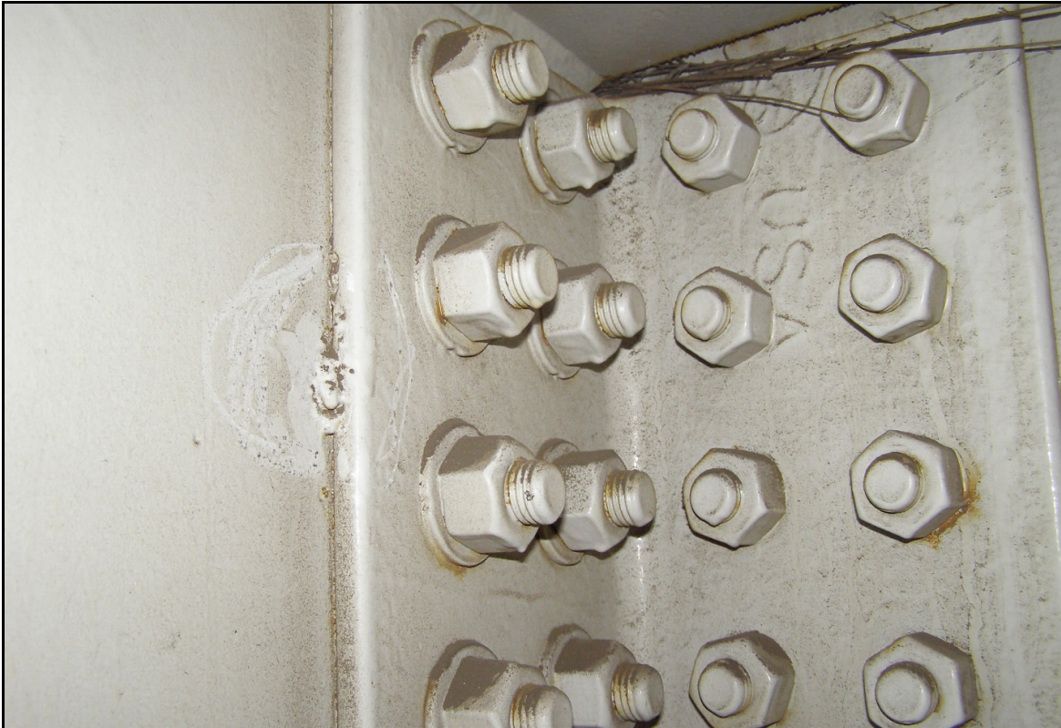
Photo 40 – Tack Weld (Circled) Between Beam A Web and Pier Cap Clip Angle, Pier 22AE
