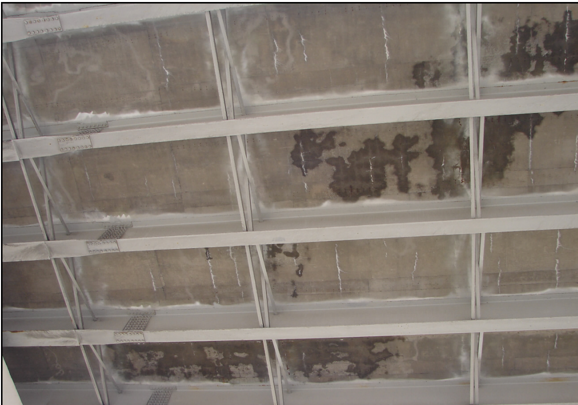
Photo 3 – Damp Areas to Underside of Floor, Span 7
