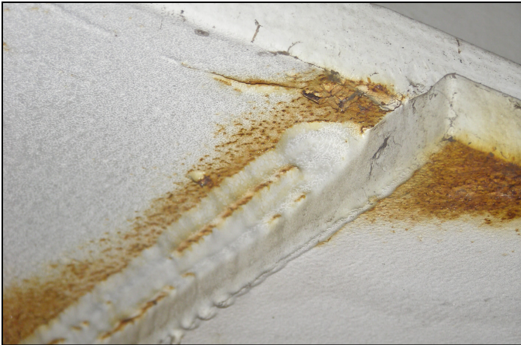
Photo 33 –End Weld to Bottom Flange Cover Plate (Embedded Top Flange Cover Plate Welds Assumed Similar)
