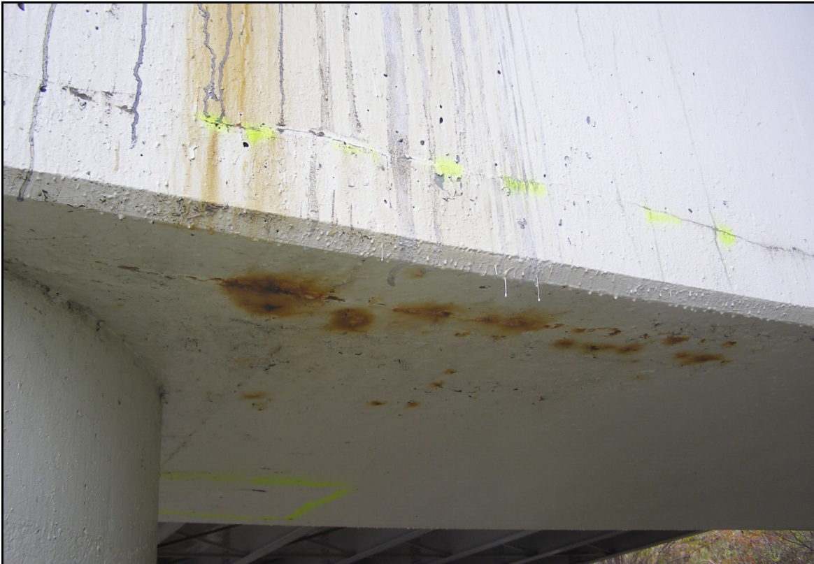
Photo 42 – Early Delamination Crack to Pier Cap Horizontal and Bottom Faces, Pier 11, East End
