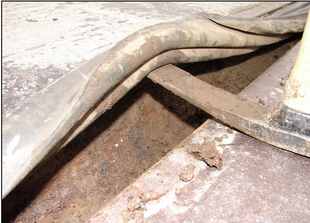
Photo 16 – Torn Membrane, Expansion Joint 1A
