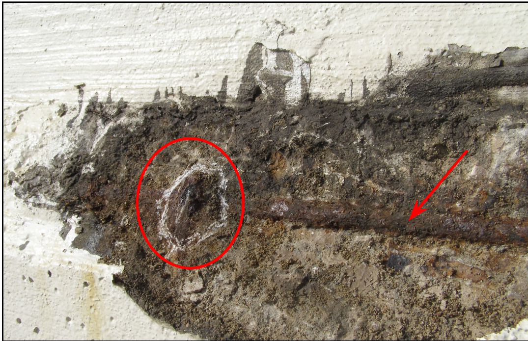
Photo 9 – Close-up of Parapet Spall with Deficient Cover to Original Rebar (Original vertical bar circled and horizontal bar noted with arrow.)
