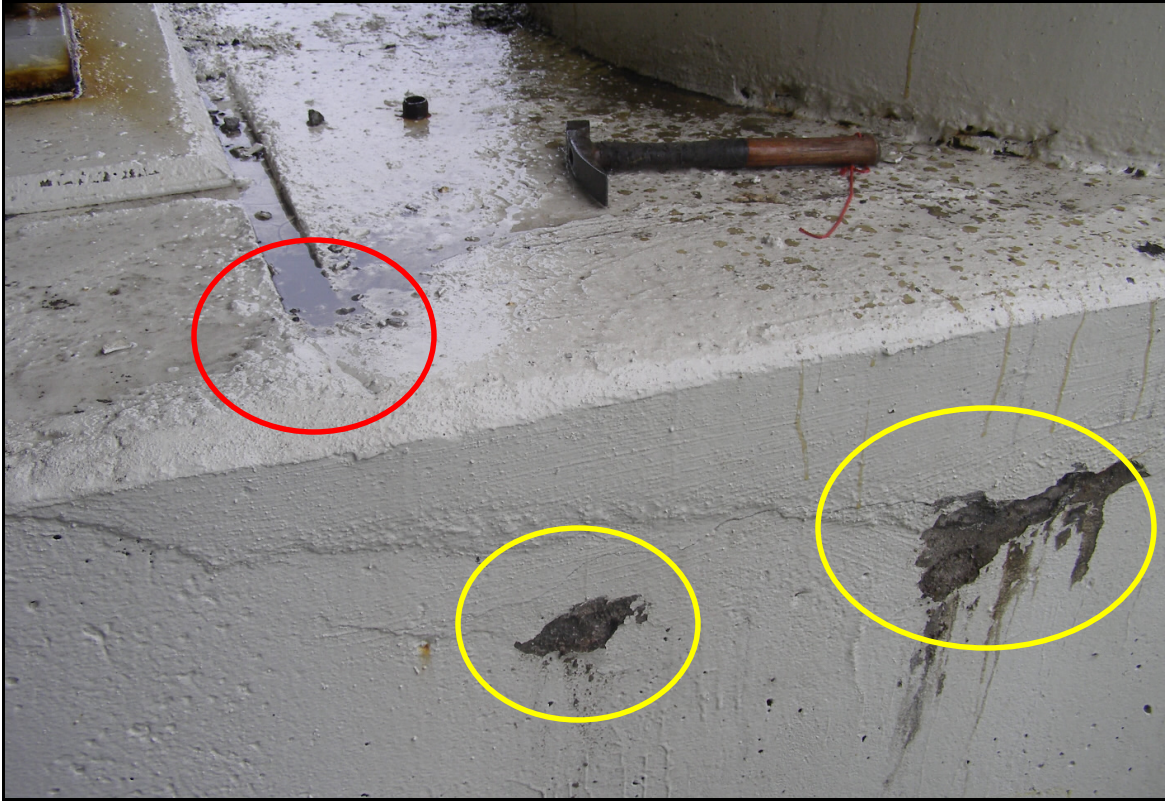
Photo 43 – Concrete Dam (Circled in Red) and Blistering Sealer (Circled in Yellow)
