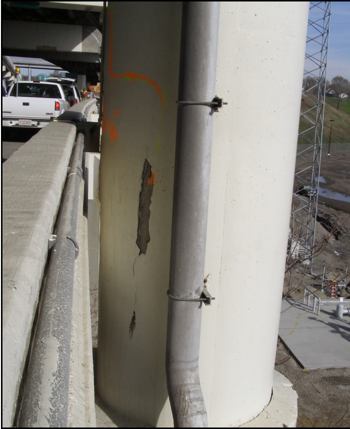
Photo 34 – Delaminated Concrete to Pier Column along Jennings Freeway Traffic, Pier 14, I-71 Bridge
