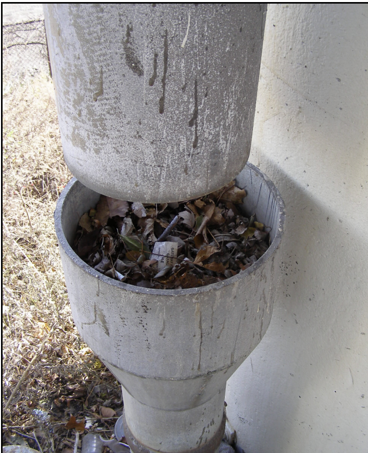
Photo 12 – Clogged Drainage Collector, Pier 6
