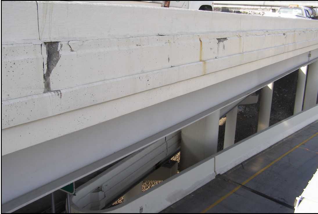
Photo 8 - Spalled and Delaminated Concrete to Parapet over NB Jennings Freeway to W. 14 th Street Ramp
