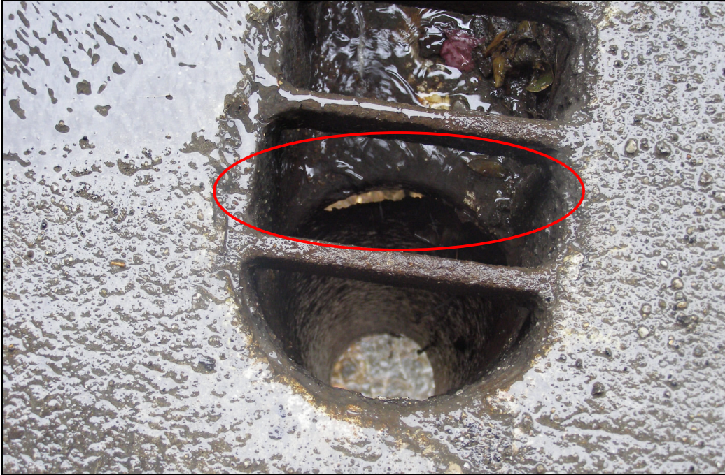
Photo 22 – Corroded Pipe (Circled) at Bottom of Deck Level, Near South Abutment B
