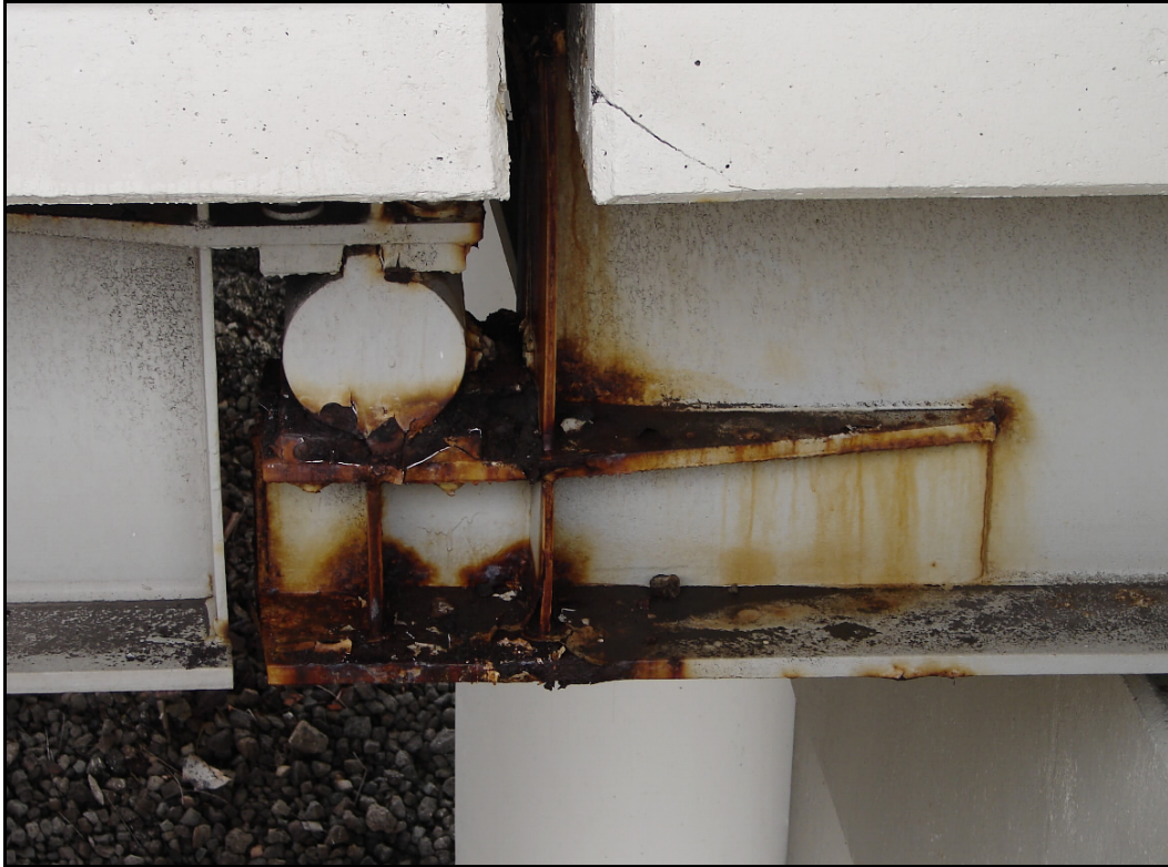
Photo 32 – Typical Corrosion at Expansion Hinge
