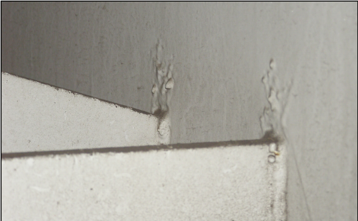
Photo 24 – Typical Diaphragm Weld Undercut to Beam Web
