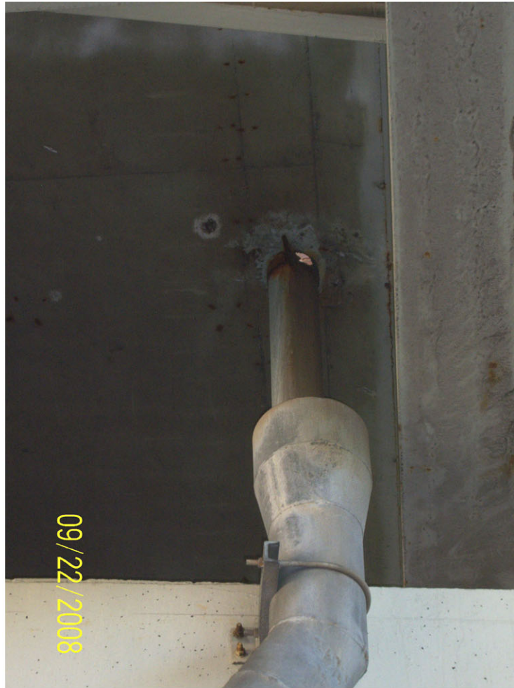
Thru Hole in downspout at Pier 18 AW.JPG
