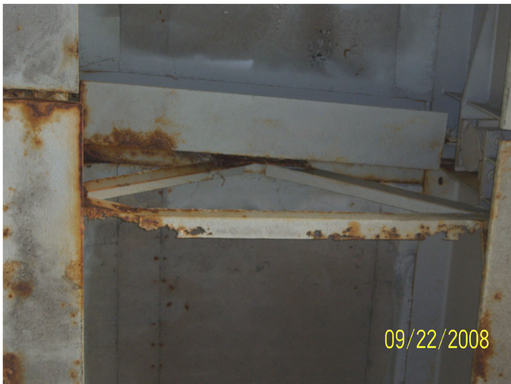
Thru holes in xframe at Intermediate Expansion 2 BW.JPG
