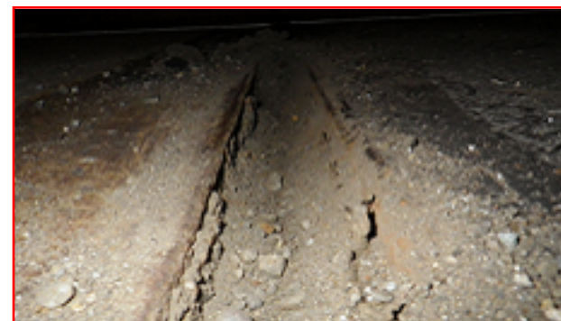
Elastomeric sealer missing from right portion of abutment joint.
