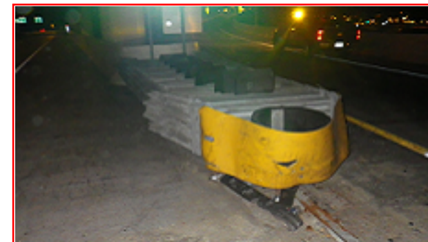
Impact attenuator has been hit by vehicle.
