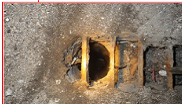
Typical clogged drain.
