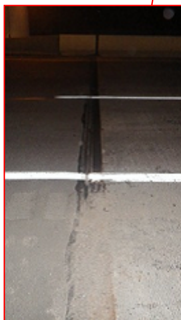
Abutment joint has debris covering part of joint.
