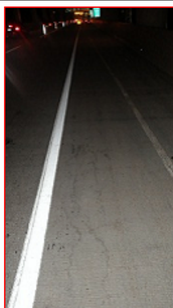
Longitudinal cracking in right shoulder.
