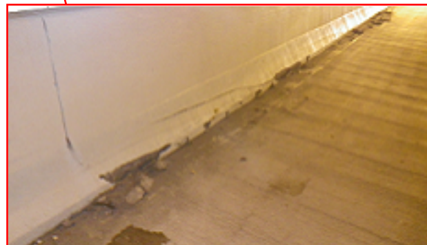
Typical spall at toe of barrier.
