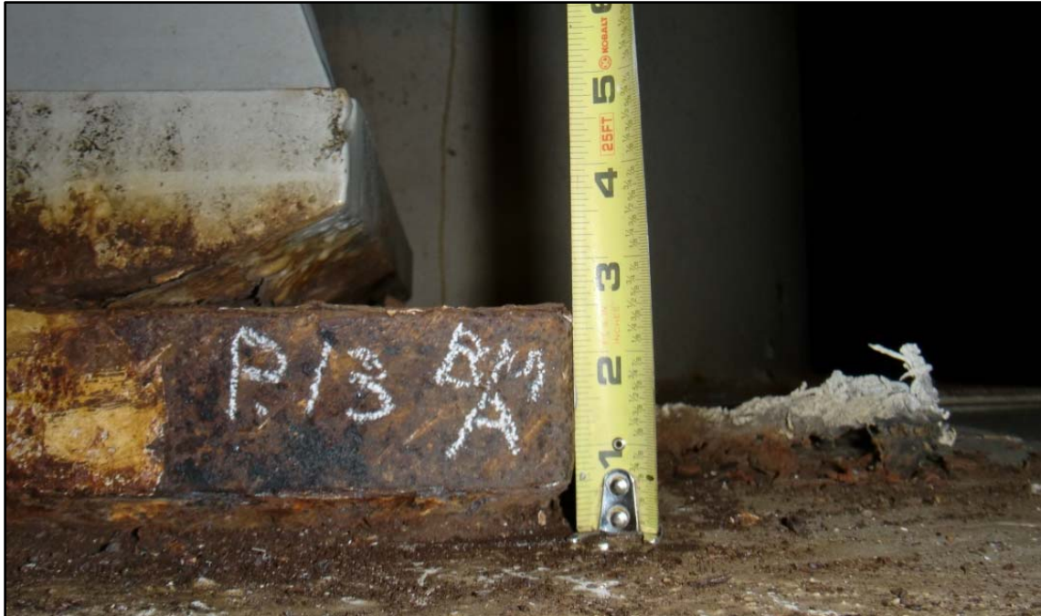
Photo 22 – Rust Accumulation & \frac{9}{16} -Inch Lift on Bearing Plate, Beam A, Pier 13.
