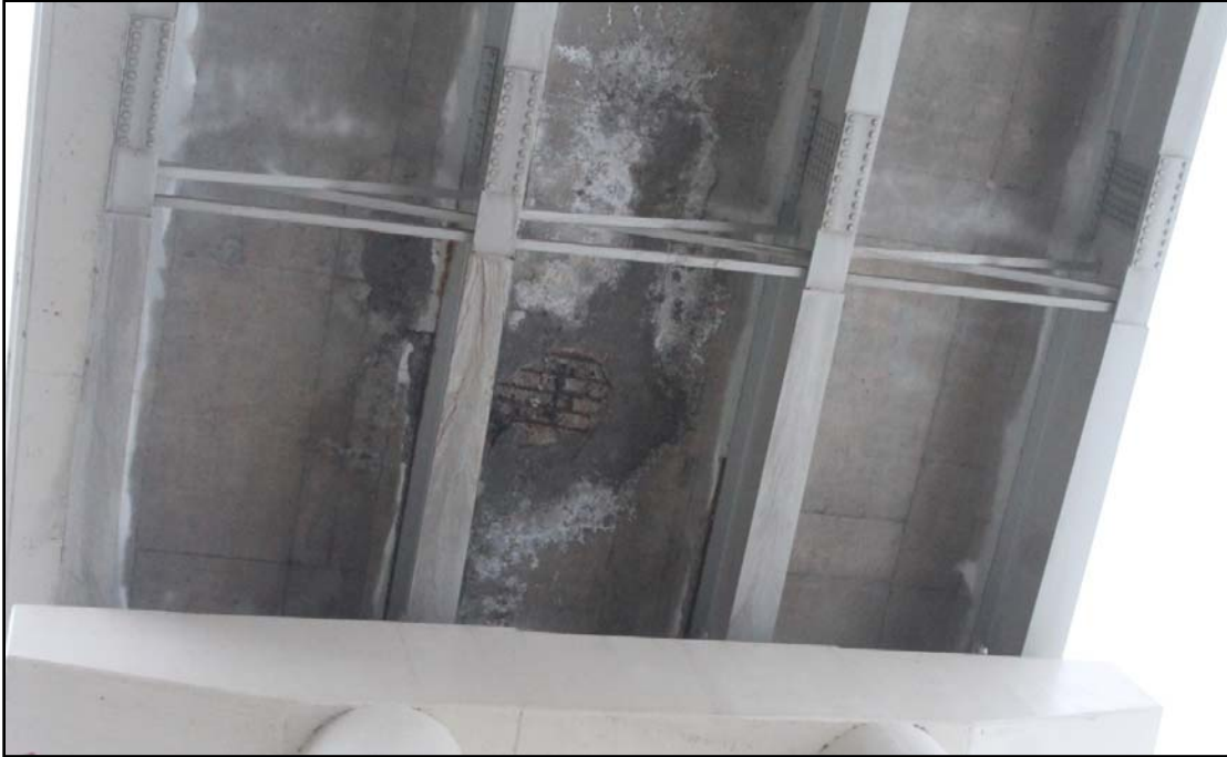
Photo 6 – Floor Spall, Span BE.
