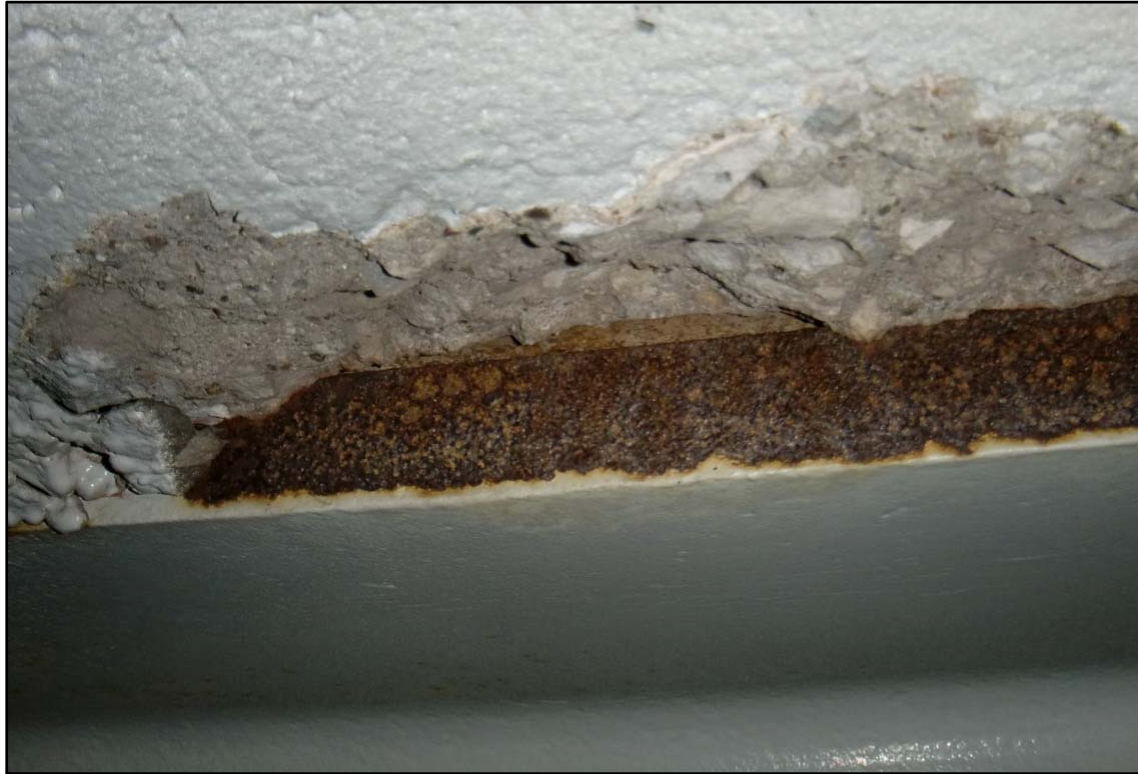
Photo 7 – 1/4 -Inch Haunch Separation at Beam E, Span 18.
