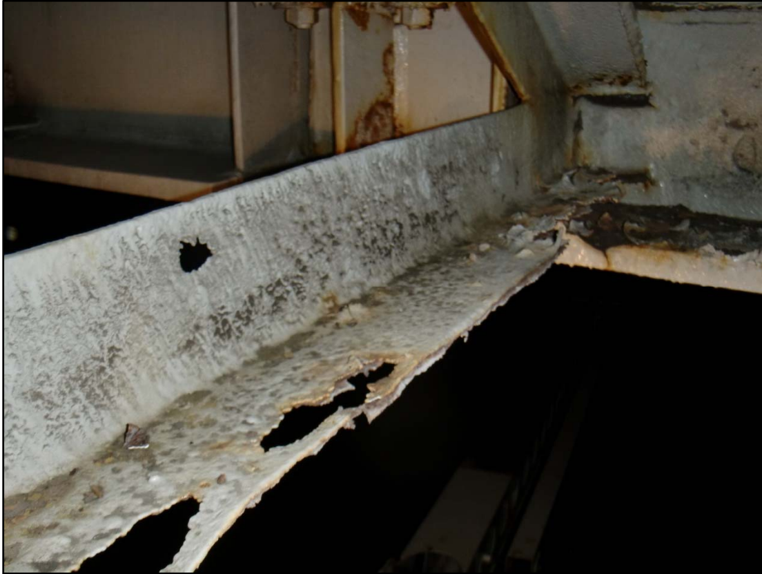
Photo 17 – Advanced Section Loss on Cross Frame Horizontal Member, Beneath Expansion Joint 2-B, Span 18BW.
