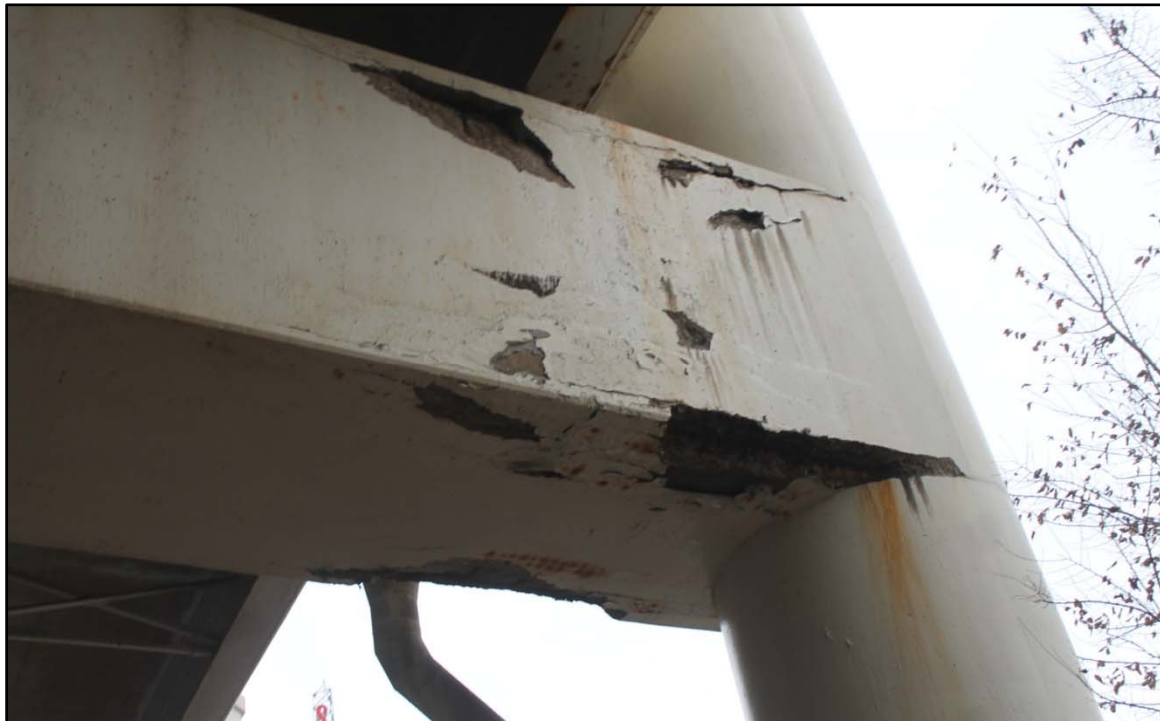
Pier 28 – Pier Cap Spalls & Delaminations, Pier 13 East Face.
