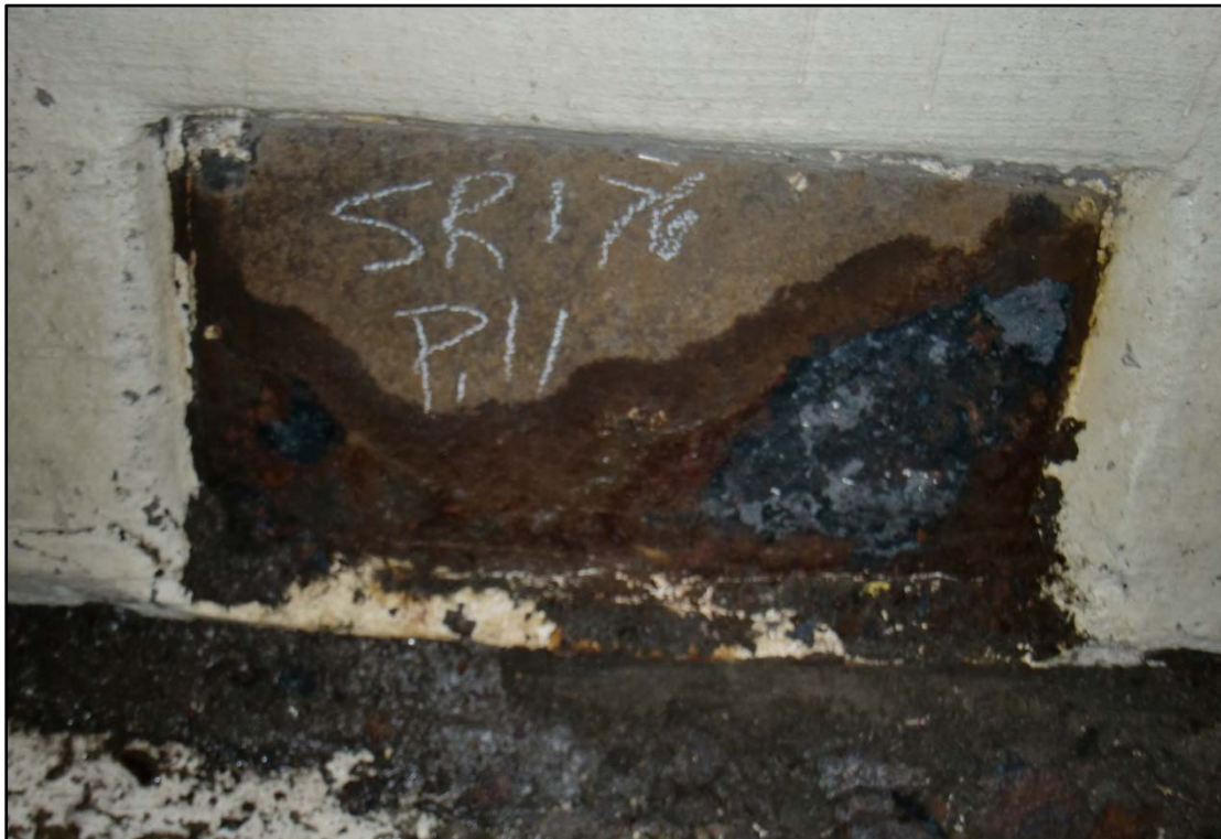
Photo 14 – Corroded & Thin Pull Box Cover, Pier 11.
