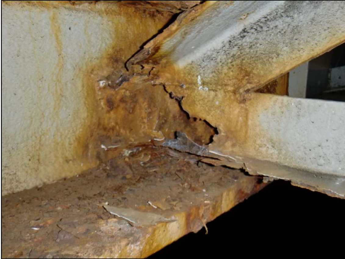
Photo 18 – 100% Section Loss at Cross Frame Connection, Expansion Joint 1-B, Span 13B.
