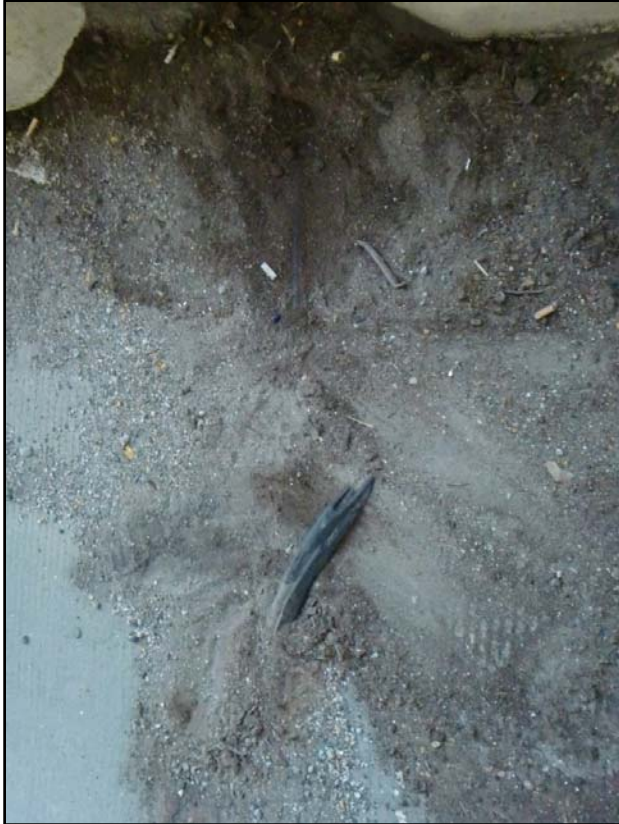
Photo 12 – Torn Expansion Joint Membrane, Joint 1-A.
