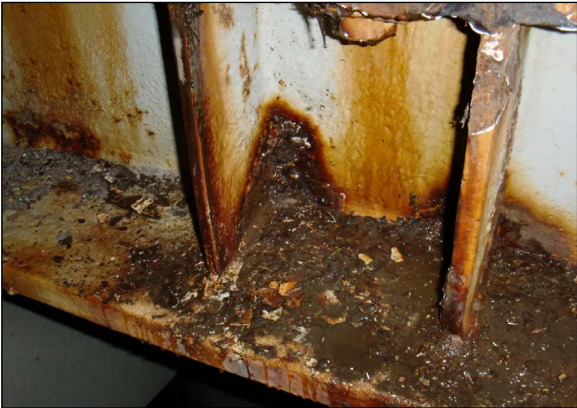
Photo 20 – Typical Failed Paint & Active Corrosion at Hinges.
