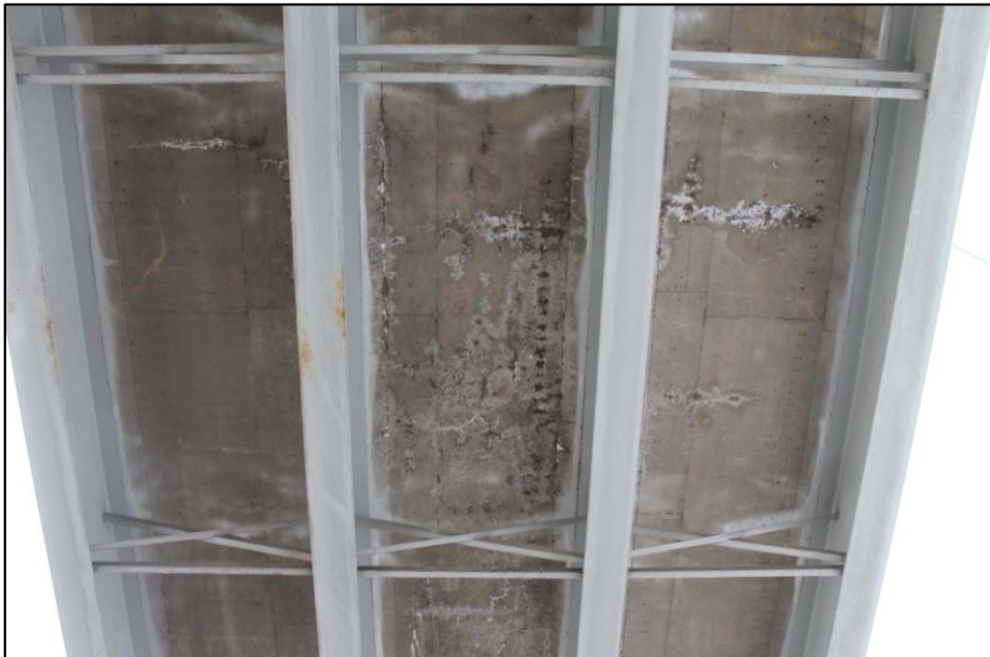
Photo 5 – Mottled Floor Soffit with Efflorescence.
