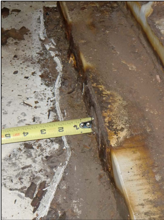
Photo 21 – 1 1/2-Inch Bearing Plate Misalignment, Beam A, Pier 13.
