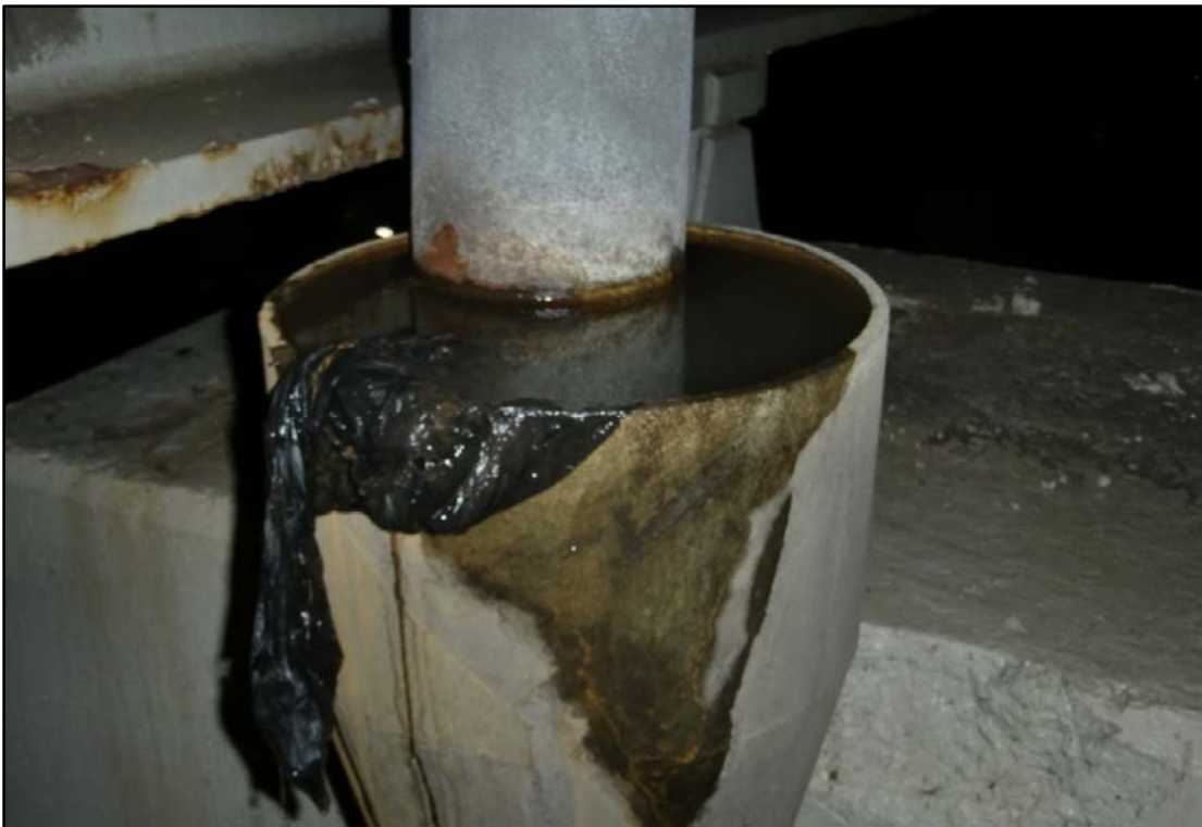
Photo 11 – Clogged Collector & Overflowing Drain Water, Pier 18BE.
