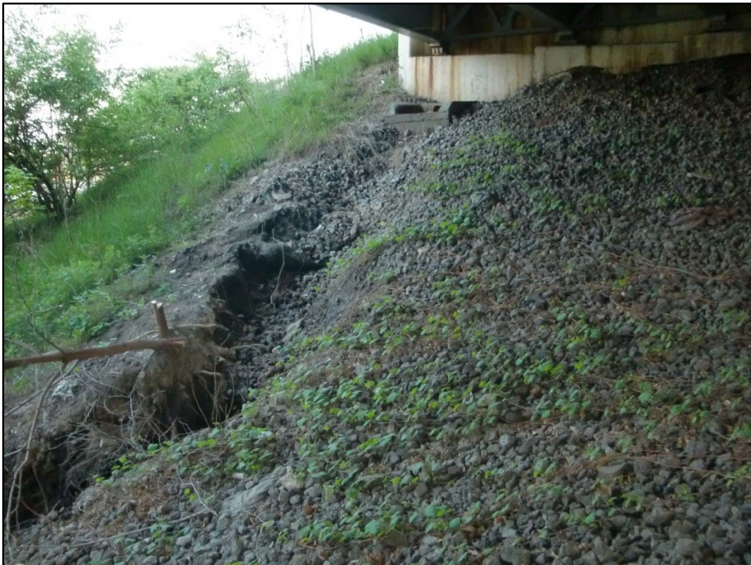
Photo 30 – Slope Protection Erosion, South Abutment.
