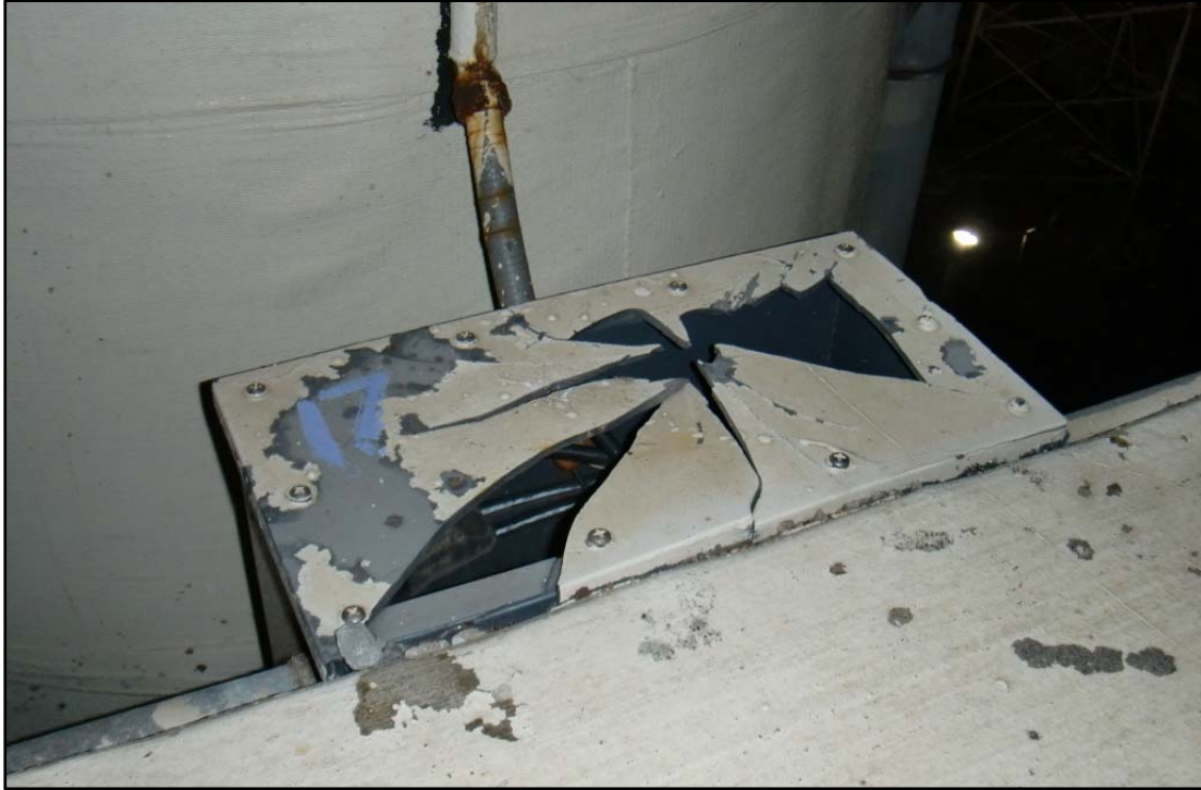
Photo 15 – Fractured Junction Box Cover, Pier 17.
