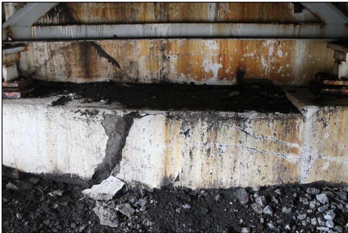
Photo 25 – Delaminated Surface above Horizontal Crack, Abutment BW.
