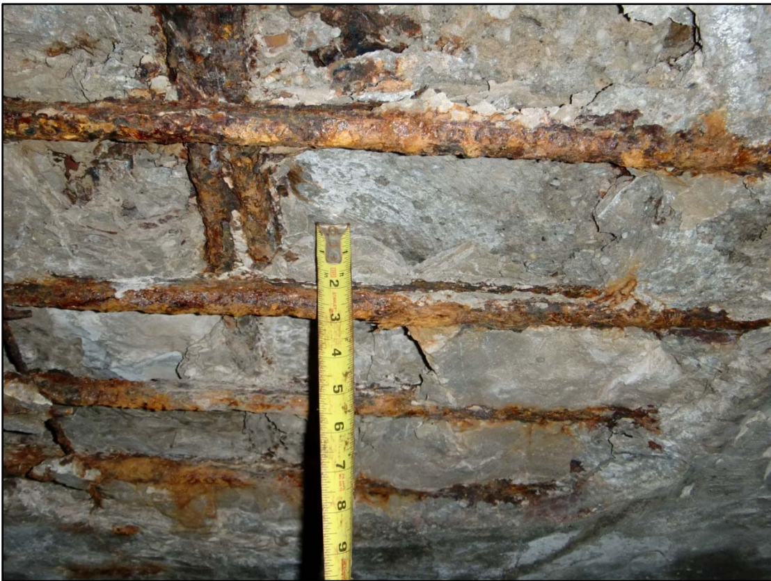
Photo 7 – Four-Inch Deep Floor Spall Close-Up with Primary Reinforcement Section Loss, Span 21BE.
