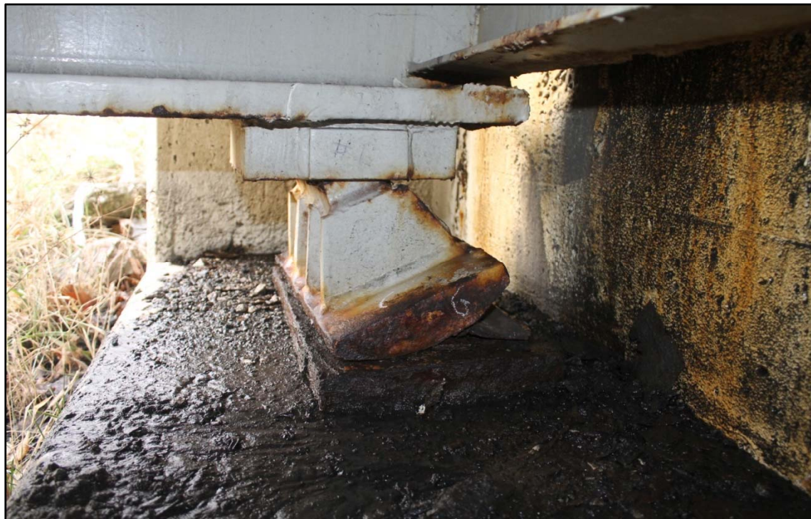
Photo 22 – Maximum Rotation of Bearing G with Shifted Bearing Plate, North Abutment BW.
