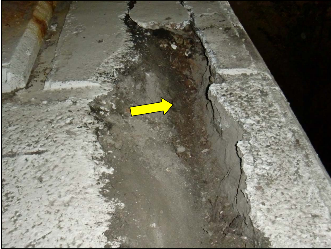
Photo 29 – Diagonal Top Spall approximately 3” Deep to indicated No. 18 Bar, Pier 13.
