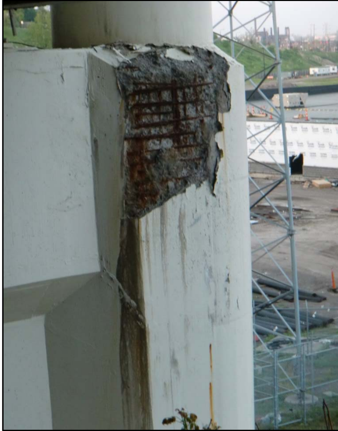
Photo 27 – Nine-foot x Six-Foot Spall on East Pier Column, Pier 15.
