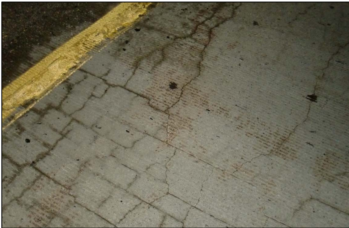
Photo 9 – Map Cracking, Unit 4BE.
