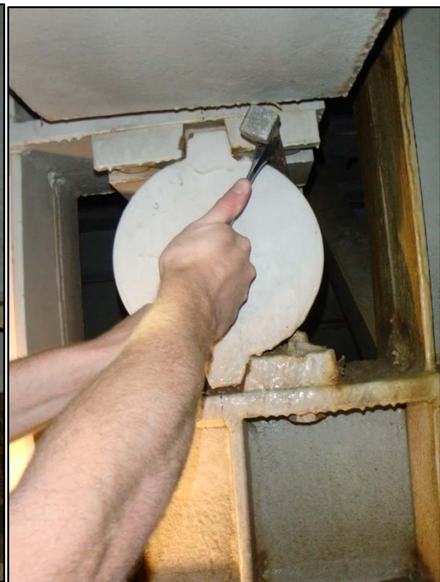
Photo 4 – Prying Action for Hinge Bearing Check.
