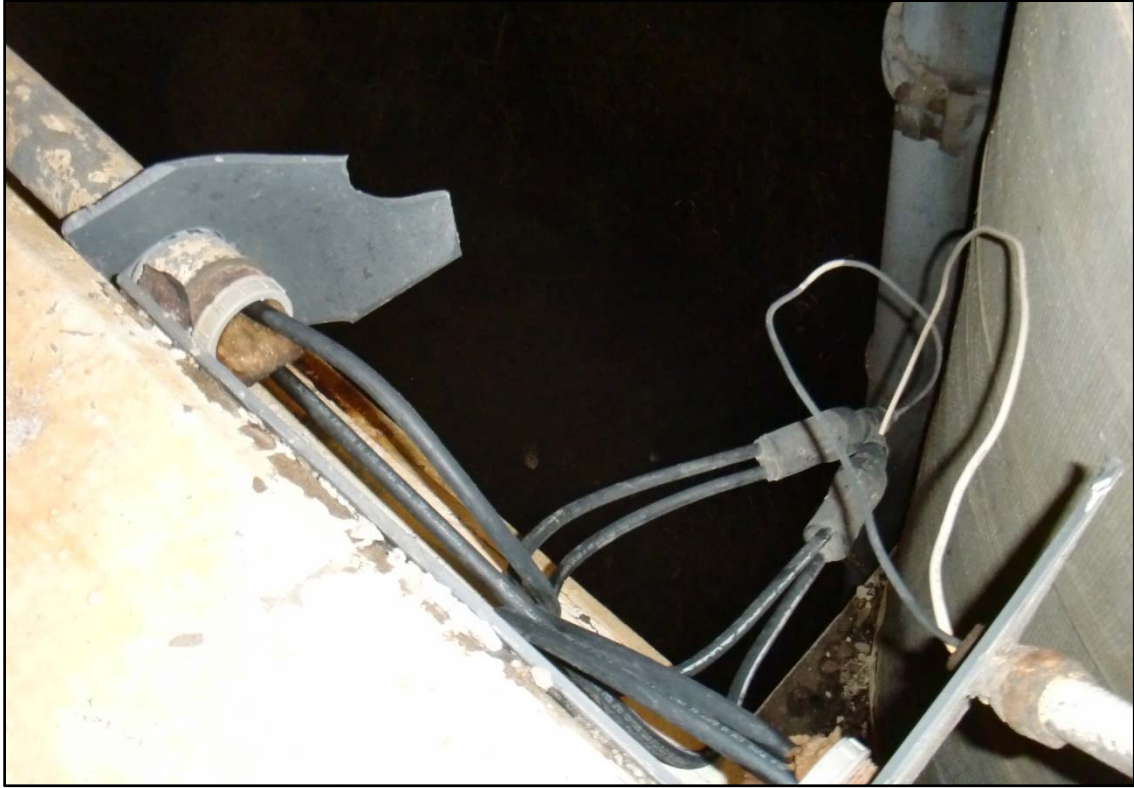
Photo 13 – Broken Conduit & Exposed Wires,, Pier 11.
