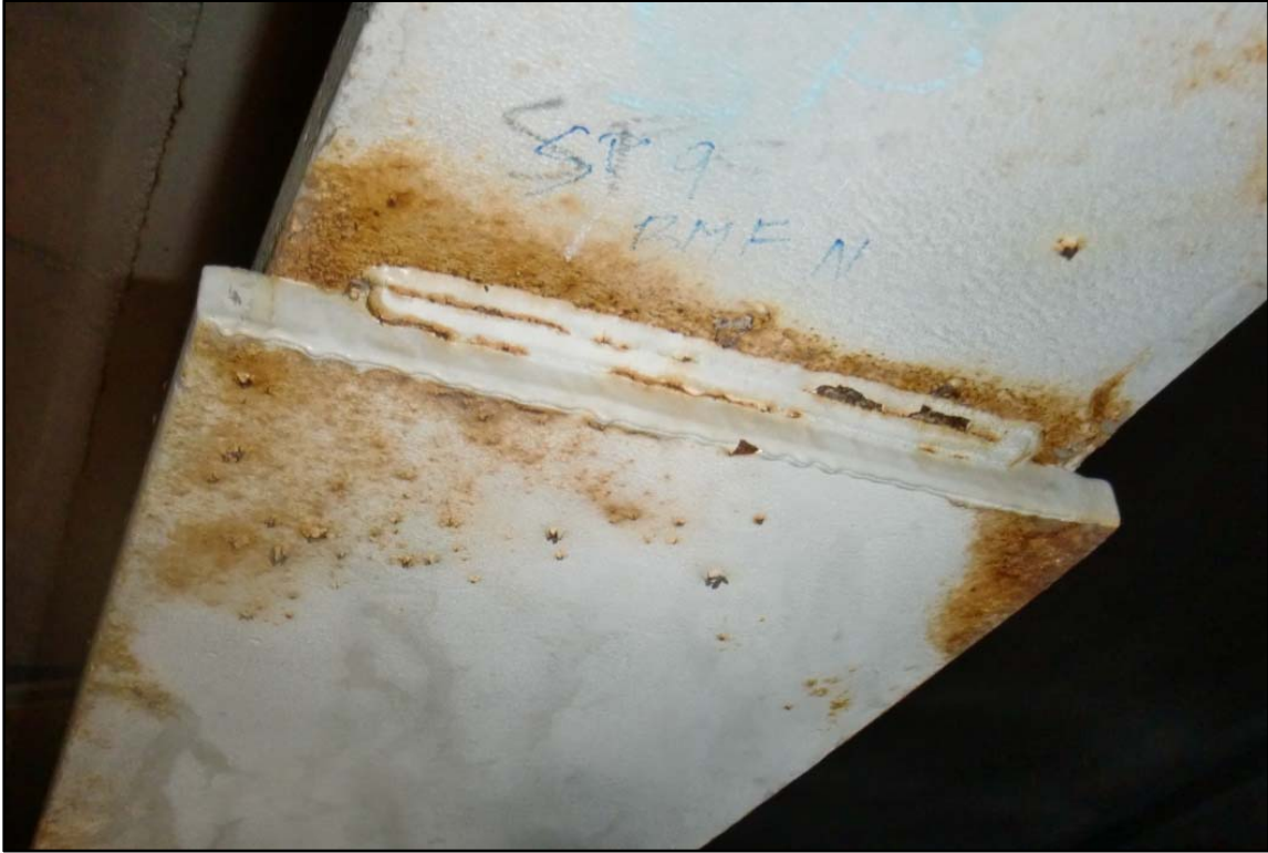
Photo 19 – Typical Freckled Rust on Bottom Flange & Moment Plate Welds
