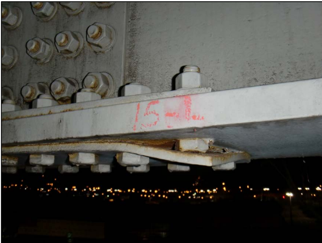
Photo 16 – Mis-erected Bottom Flange Splice Bolt, Beam L, Span 15.
