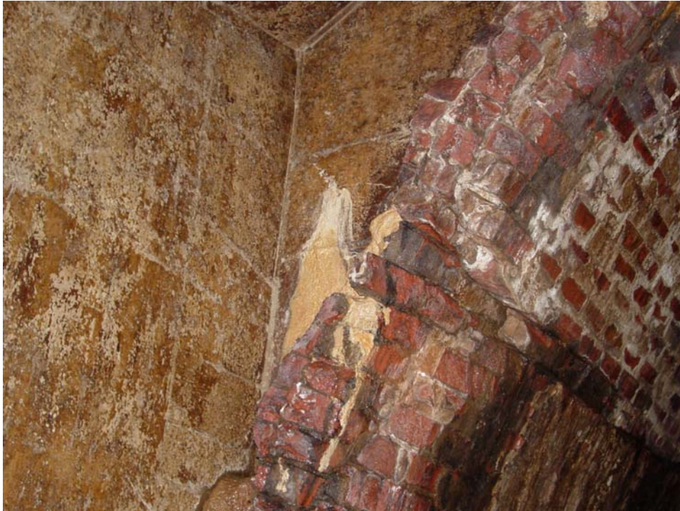
Photo 11 – Facing East. View of view of abutting brick and concrete culvert sections along Finish (North) wall.
