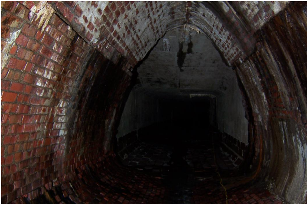
Photo 11 – Facing North at 150 feet from the Arcelor Mittal Steel entry point. 2-inch wide x 3-inch high hole in first layer of brick.
