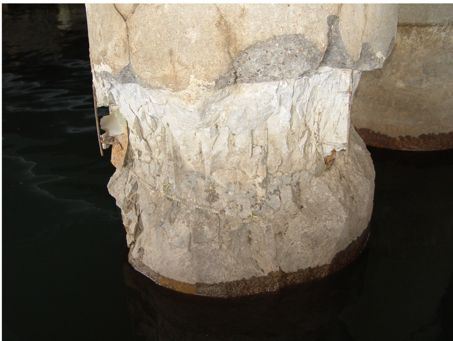
1808311 10_5_05 P8 deep spalling of P1C15.jpg
