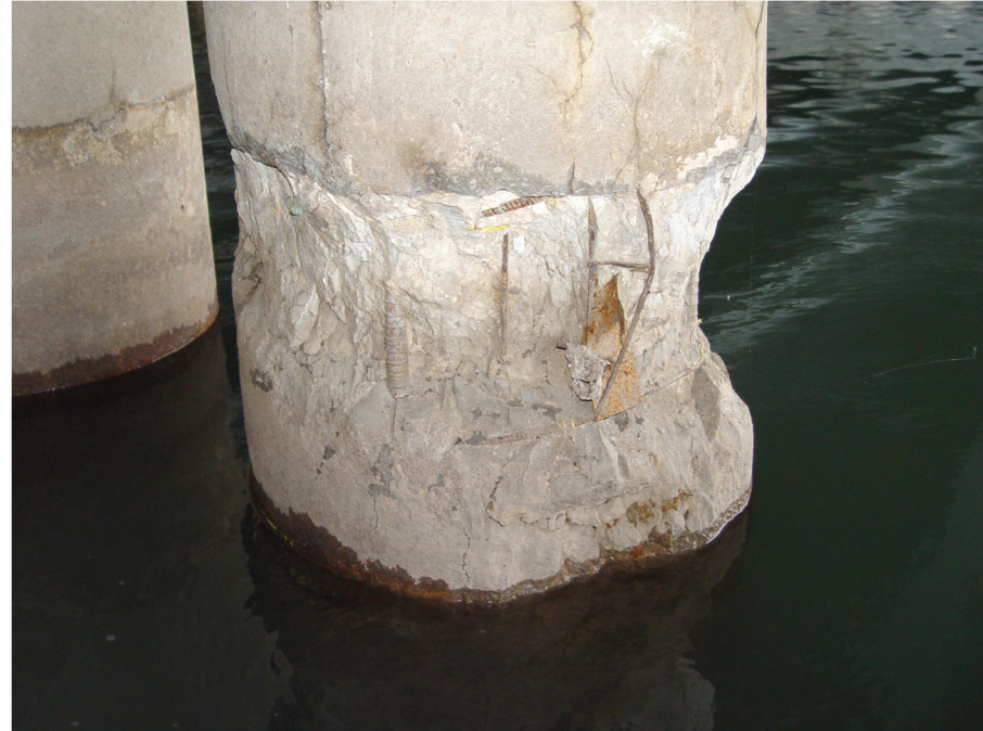
1808311 10_5_05 P7 deep spalling of P1C15.jpg
