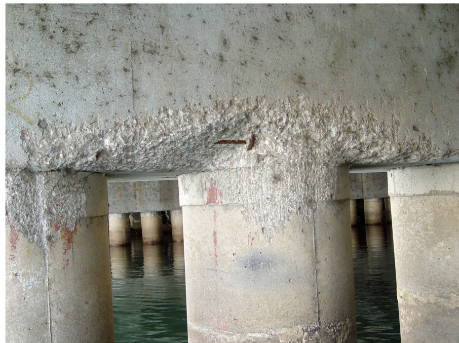
1808311 10_5_05 P9 cap spall above P2C5R.jpg
