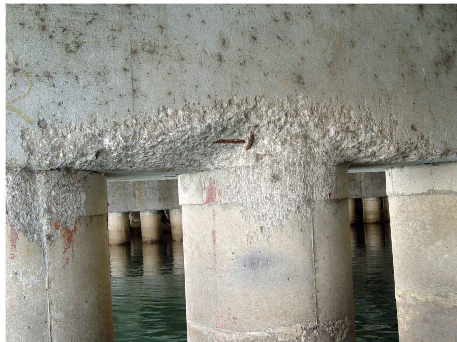
1808311 10_5_05 P9 cap spall above P2C5R.jpg
