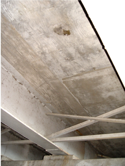
1808311 10_5_05 P1 floor spall span 1 bay 5.jpg
