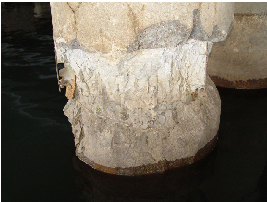
1808311 10_5_05 P8 deep spalling of P1C15.jpg
