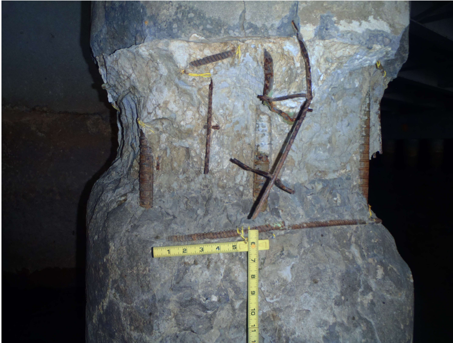
Photo 7 - Bent 2, Pile 6, Spall with Exposed Reinforcement, 1'-3" Below Cap
