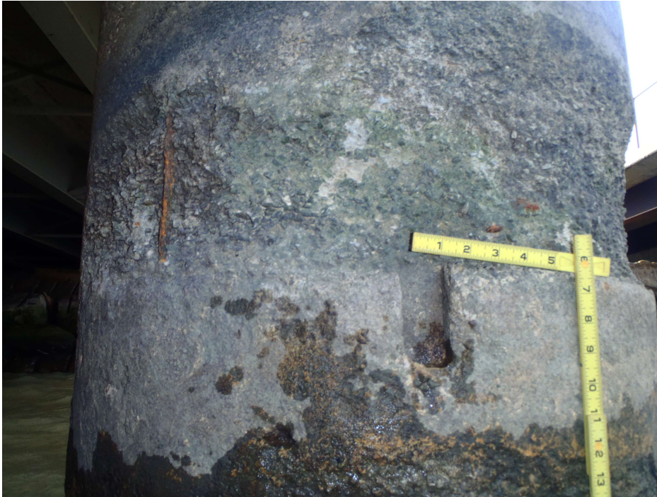
Photo 5 - Bent 1, Pile 1, Abrasion/Spall at the Waterline
