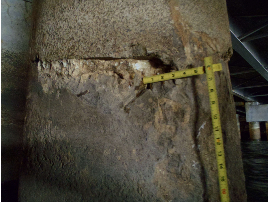
Photo 9 - Bent 2, Pile 17, Spall at the East to North Quadrant, 3' Below the Cap
