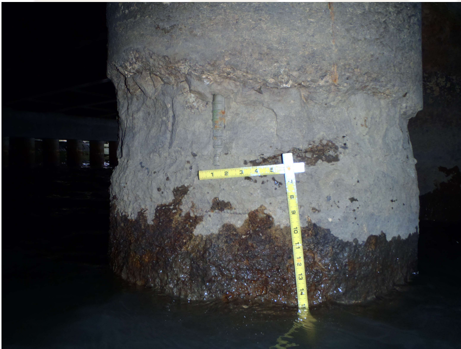
Photo 8 - Bent 2, Pile 15, Spall with Exposed Reinforcement
