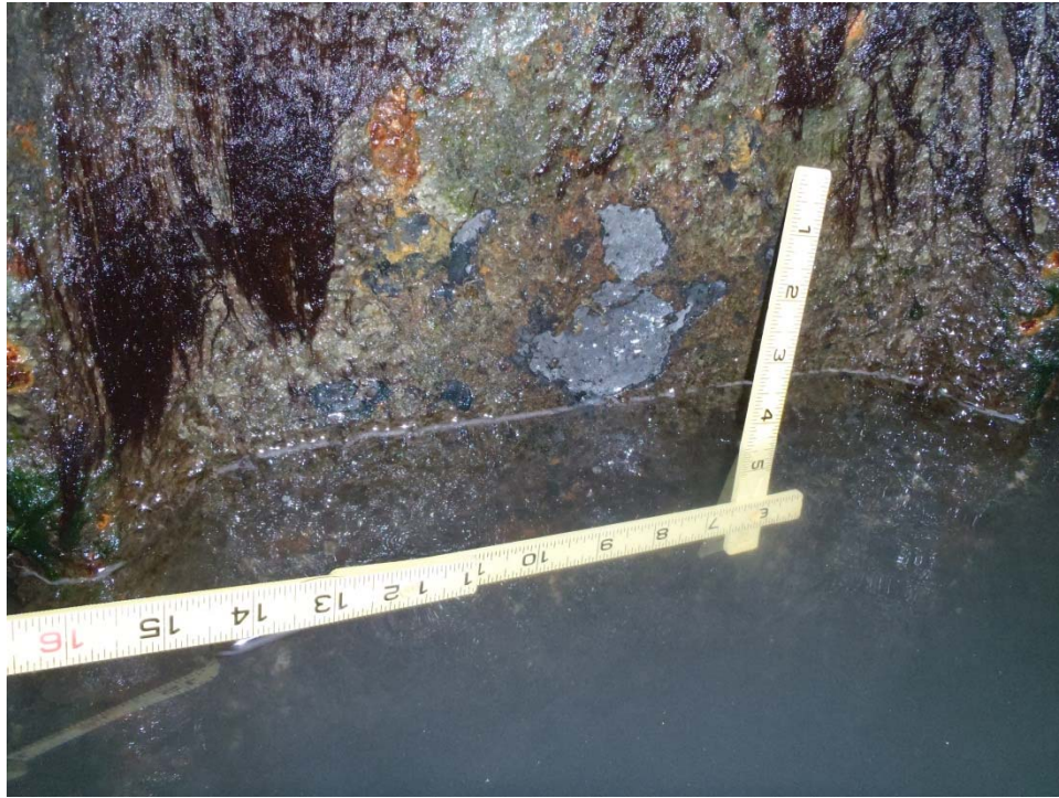
Photograph 7: Typical steel sheet pile condition in a cleaned area at the waterline.
