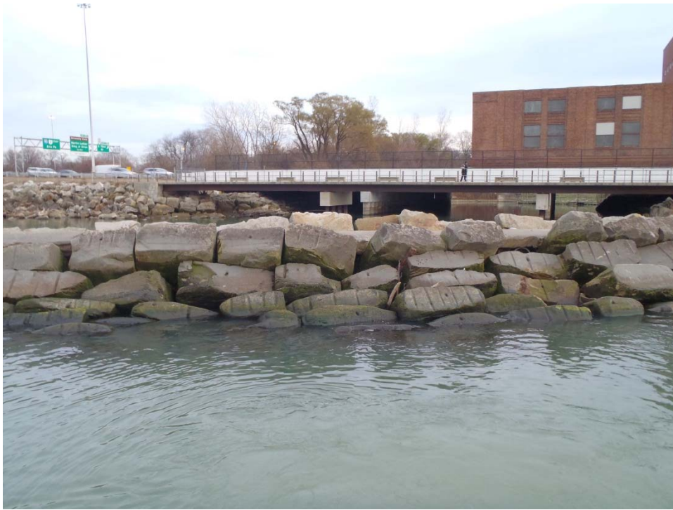
Photograph 3: Concrete jetty at the north end of the intake canal, typical of all concrete jetties.
