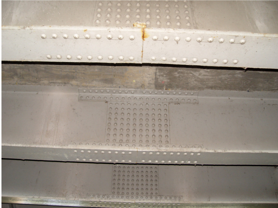
1808745 10_5_05 P1 no lower splice plates.jpg
