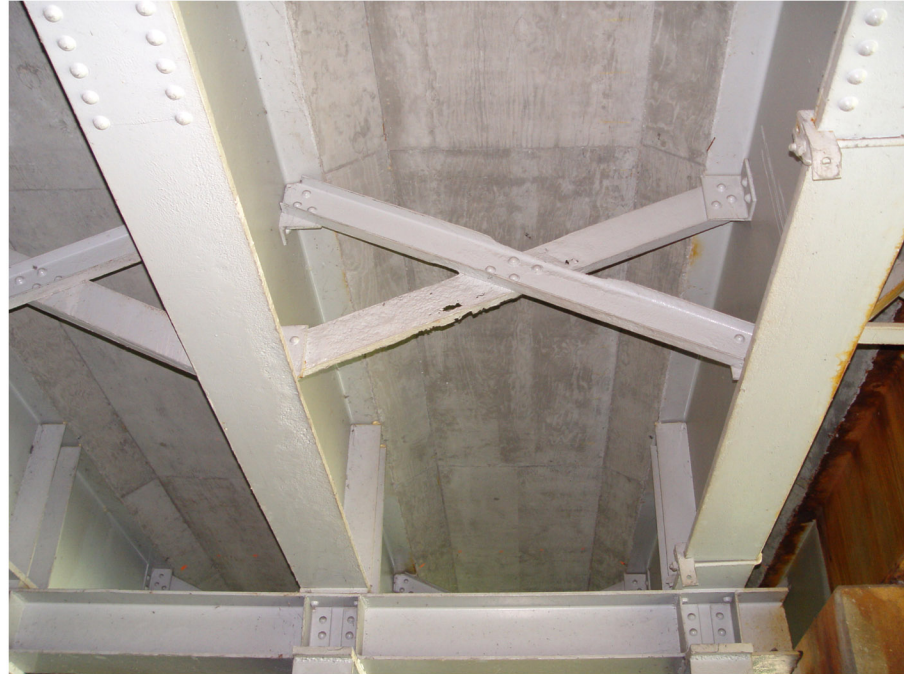
1808745 10_5_05 P2 rusted thru holes in xframe.jpg
