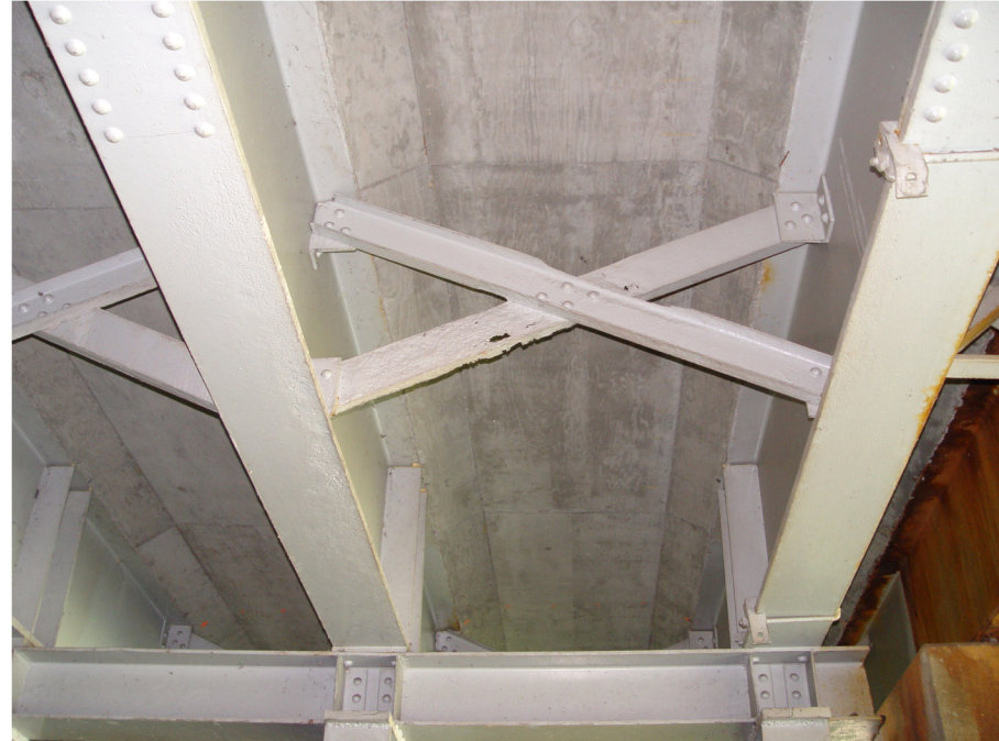
1808745 10_5_05 P2 rusted thru holes in xframe.jpg
