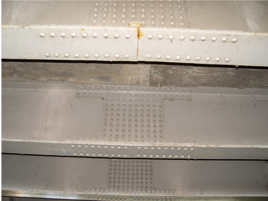
1808745 10_5_05 P1 no lower splice plates.jpg
