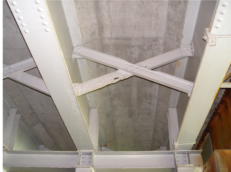
1808745 10_5_05 P2 rusted thru holes in xframe.jpg
