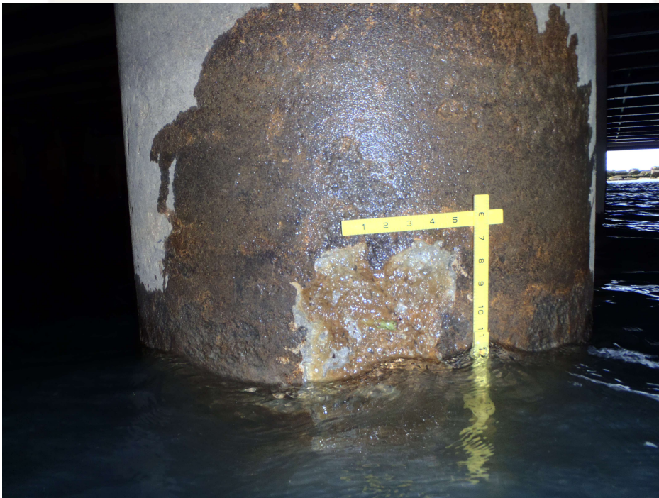
Photo 6 - Bent 2, Pile 9, Typical Area of Hollow Sounding Concrete
