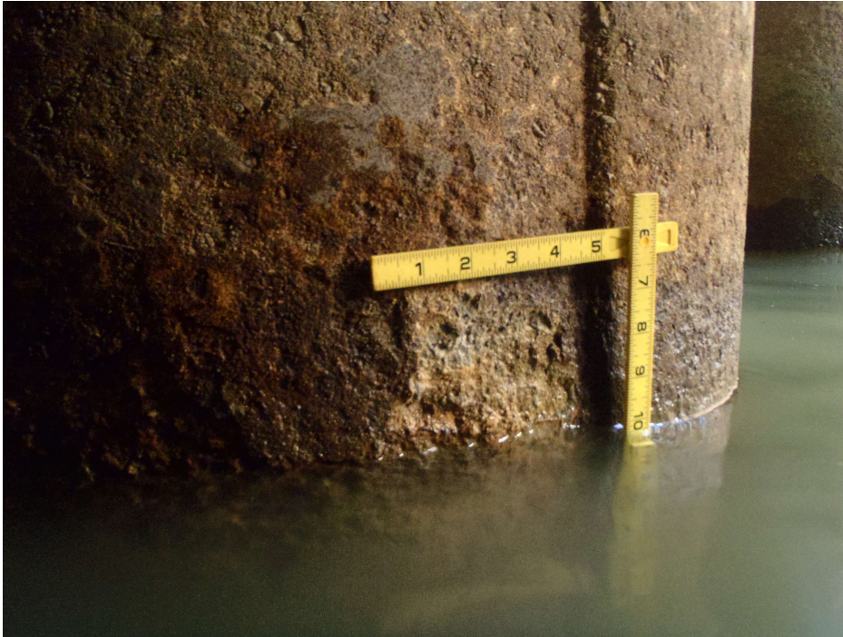
Photo 5 - Bent 1, Pile 14, Typical Condition of Concrete at Hollow Sounding Area
