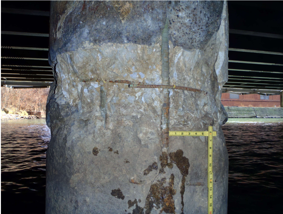
Photo 7 - Bent 2, Pile 4, Spall with Exposed Reinforcement in the Concrete Encasement
