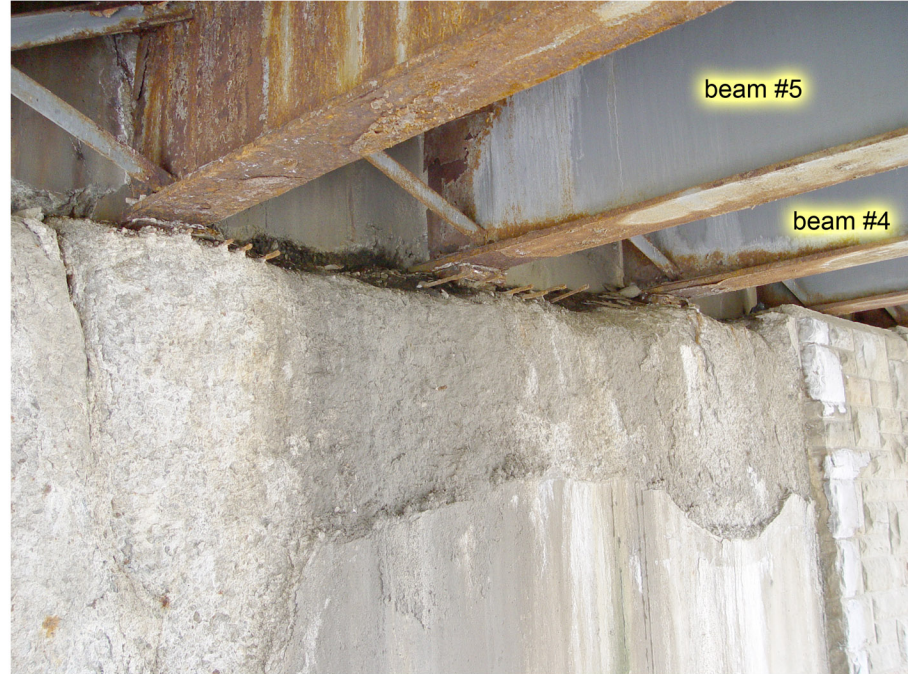
1812246 P2 5_10_05 start abut seat loss.jpg
