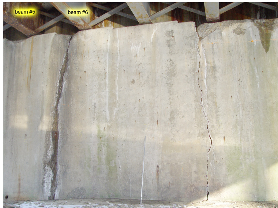
1812246 P4 12_6_05 finish abut cracks.jpg
