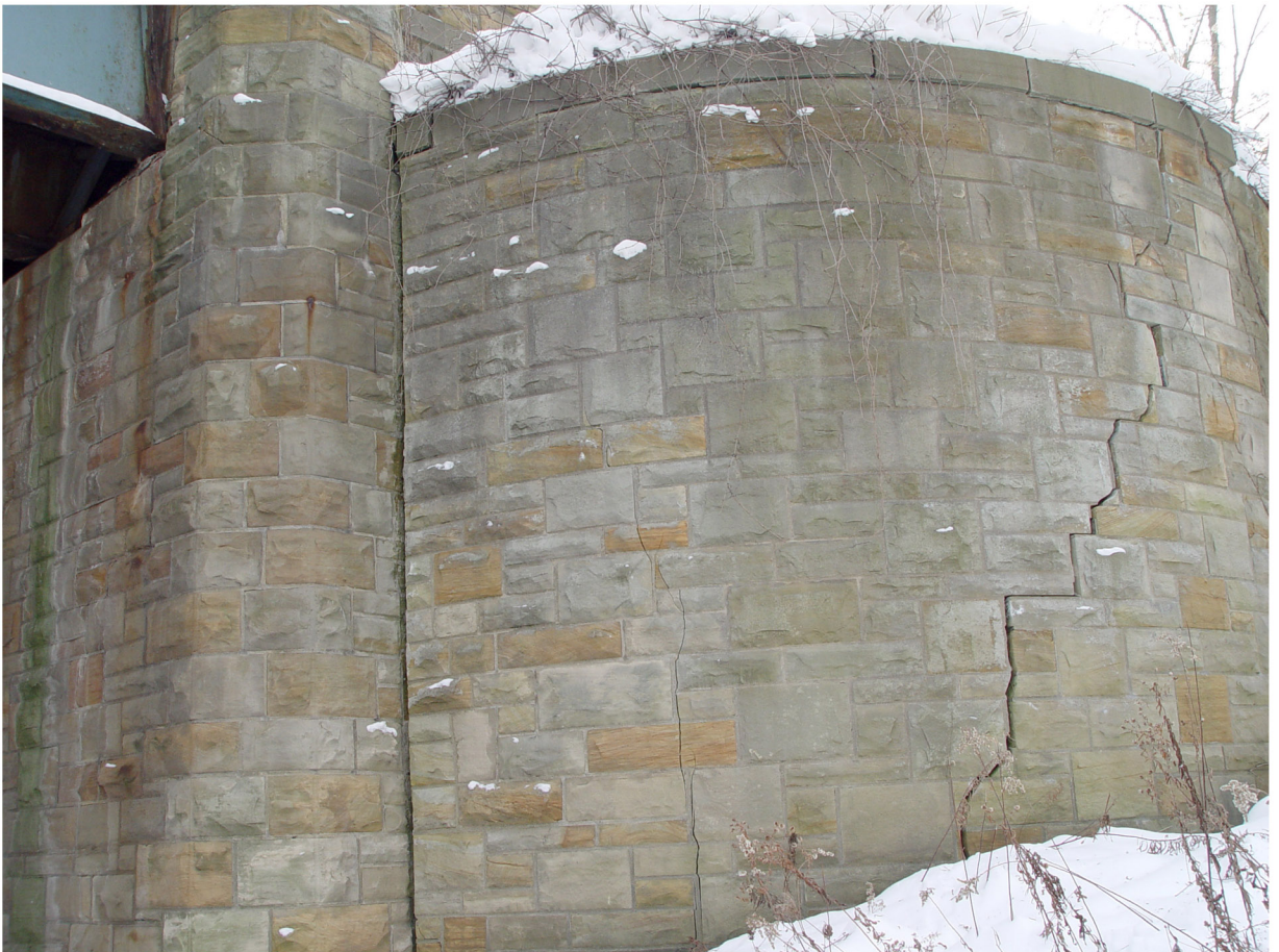
1812246 P6 12_6_05 crack in start left wing wall.jpg
