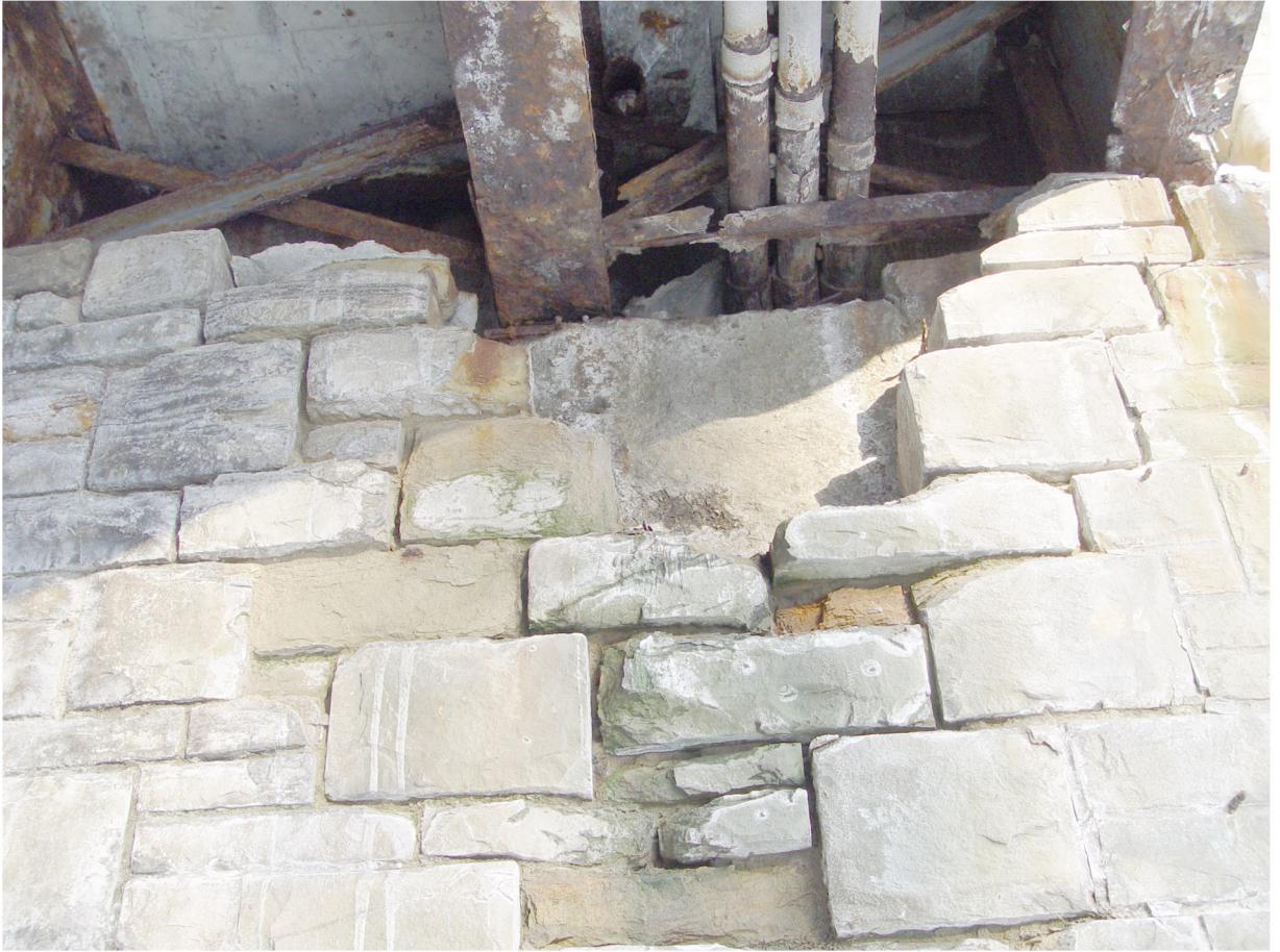
1812246 P5 12_6_05 finish abut missing stone facing.jpg
