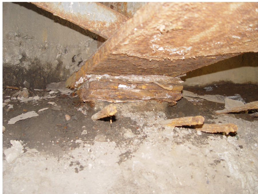
1812246 P3 5_10_05 start abut seat loss at beam 5.jpg
