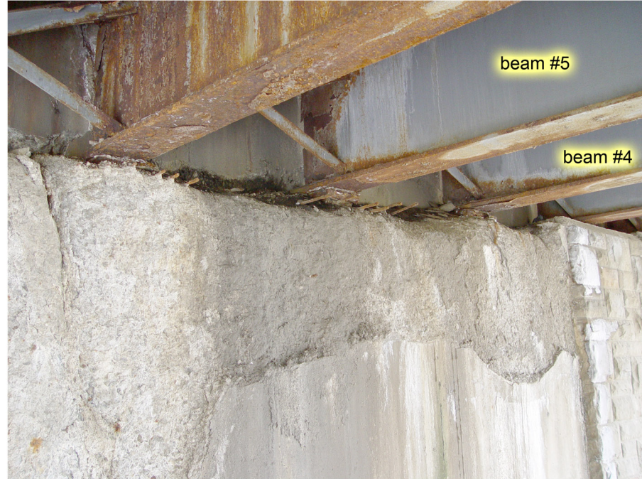
1812246 P2 5_10_05 start abut seat loss.jpg
