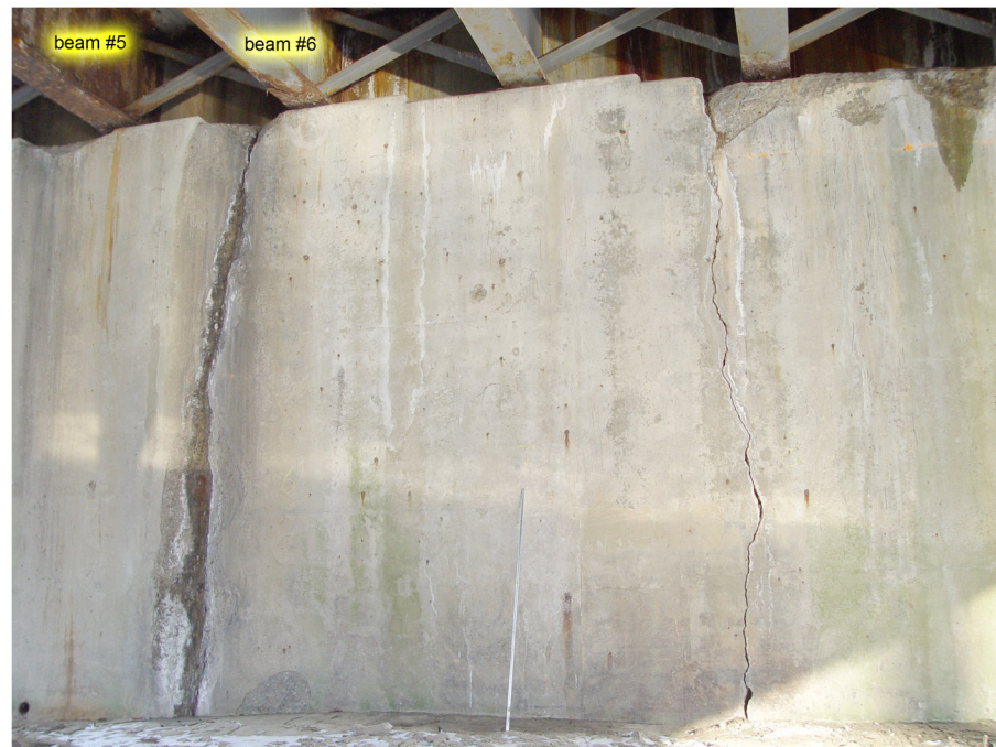
1812246 P4 12_6_05 finish abut cracks.jpg
