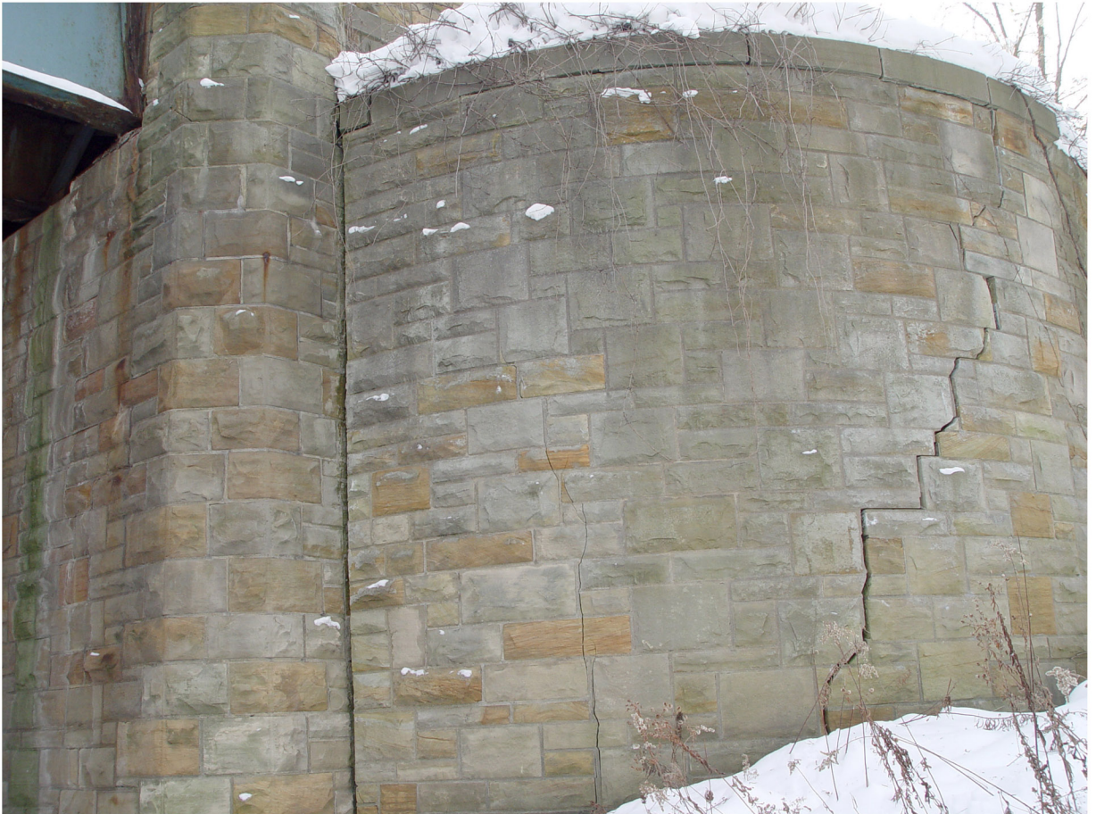
1812246 P6 12_6_05 crack in startleft wingwall.jpg
