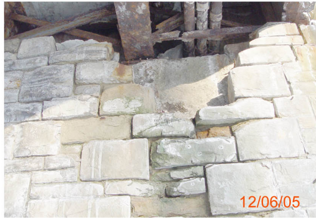
P11: FINISH ABUT UNDER BAY 1R MISSING DECORATIVE STONE.
