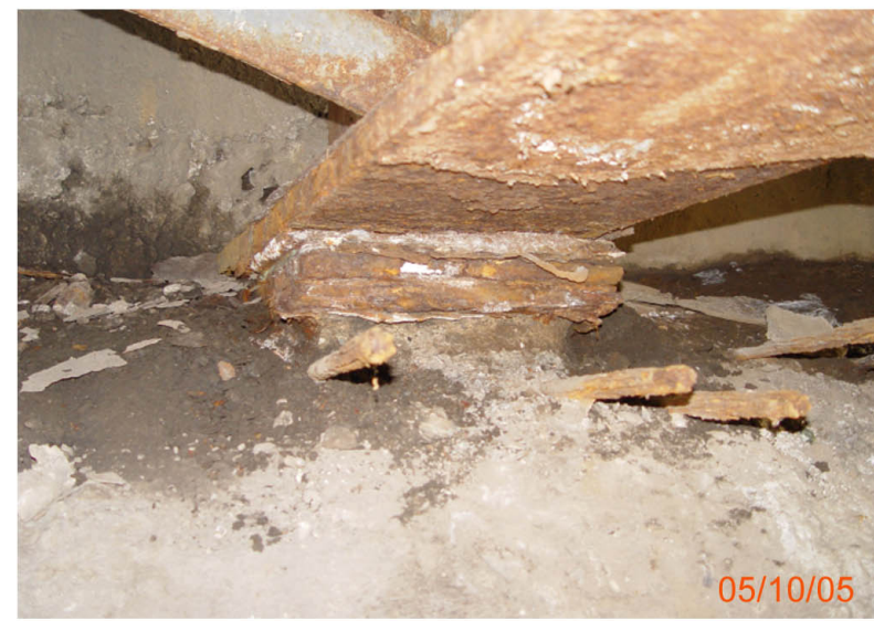
P9: CLOSE-UP OF SEAT LOSS AT BEAM #5 FROM P8.
