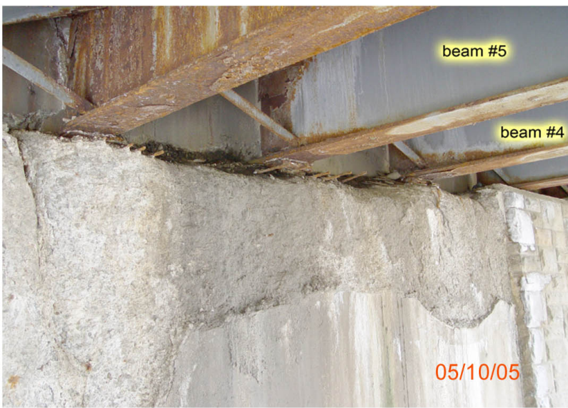
P8: START ABUTMENT SPALLED WITH ABUTMENT SEAT LOSS.
